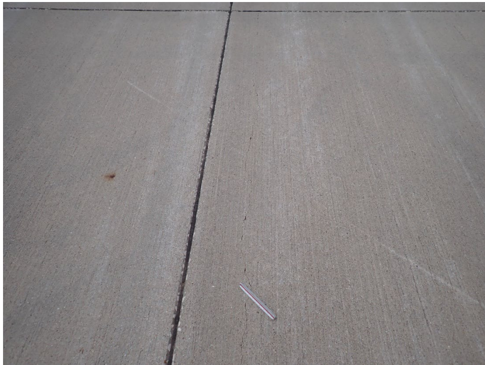
T02HL-01. LTD Cracking (Sample Unit No. 09).
