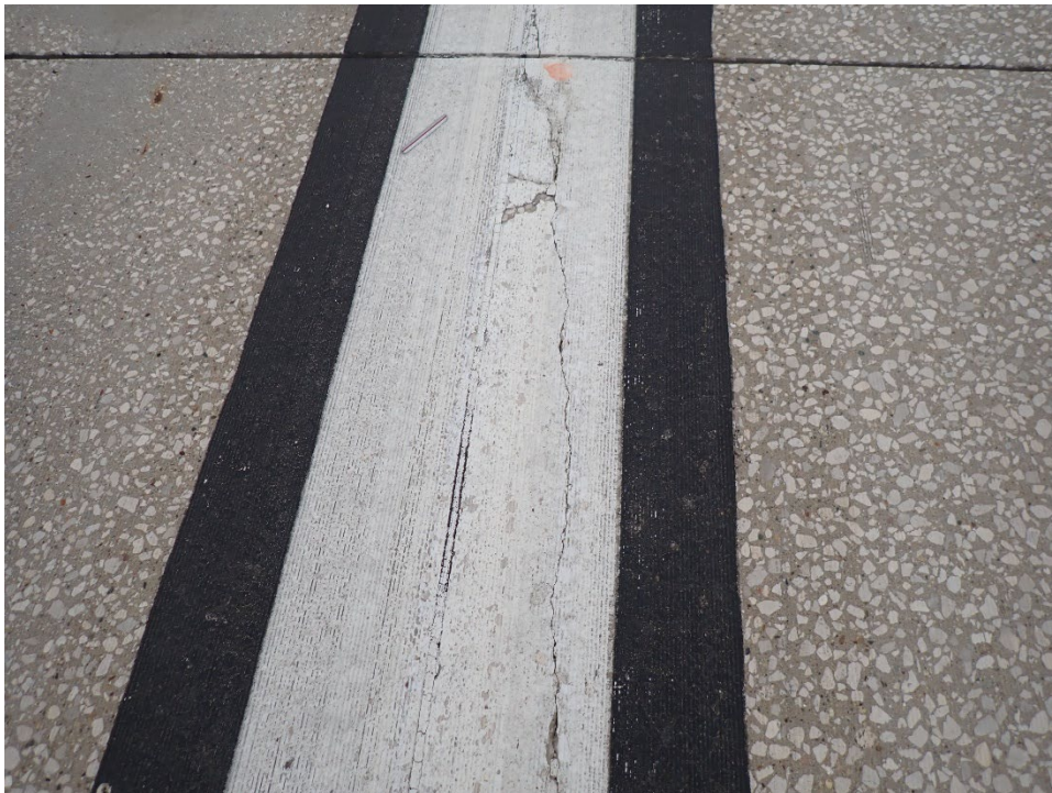
R15HL-01. Joint Spalling (Sample Unit No. 095).
