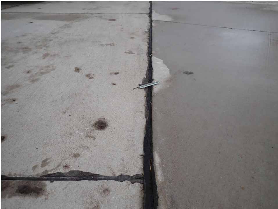
TH01HL-01. Faulting (Sample Unit No. 03).
