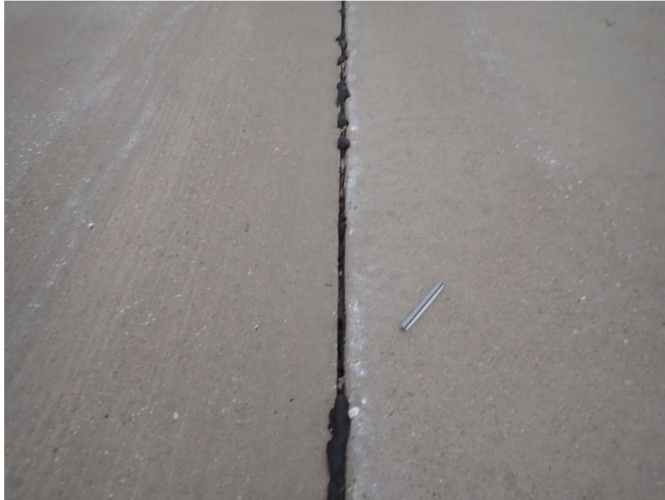
T01HL-01. Joint Seal Damage (Sample Unit No. 02).
