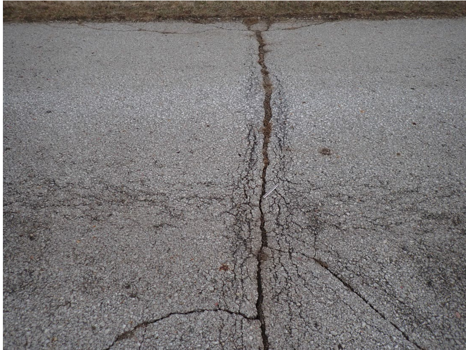
TH01HL-03. L&T Cracking (Sample Unit No. 01).
