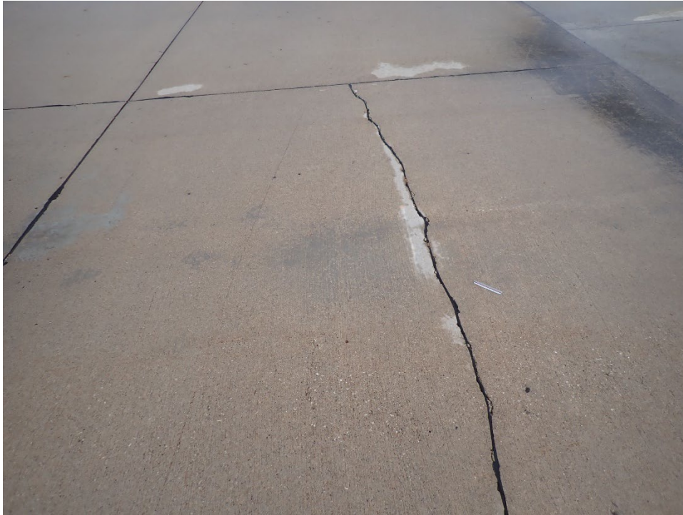
A01HL-02. LTD Cracking (Sample Unit No. 01).
