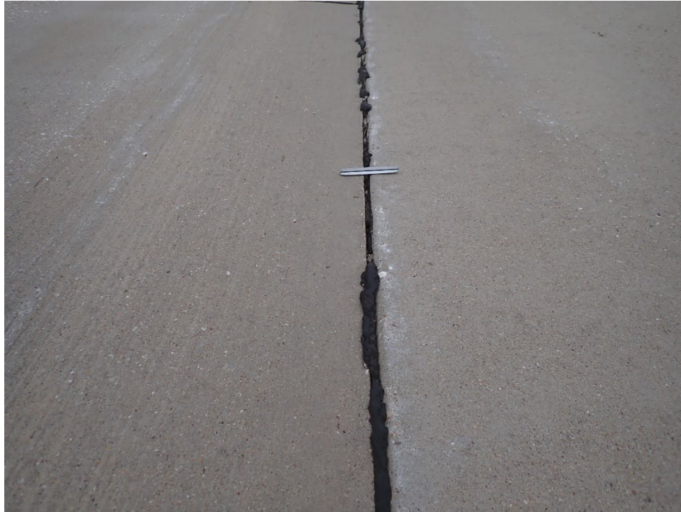
R15HL-04. Faulting (Sample Unit No. 02).
