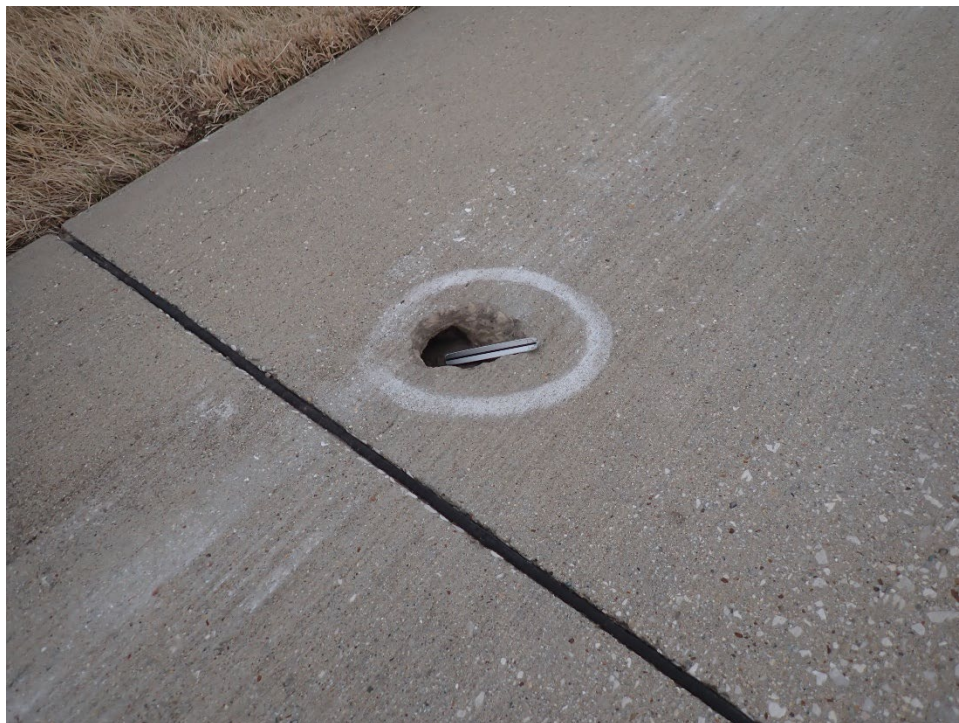
R15HL-04. Small Patching (Sample Unit No. 02).
