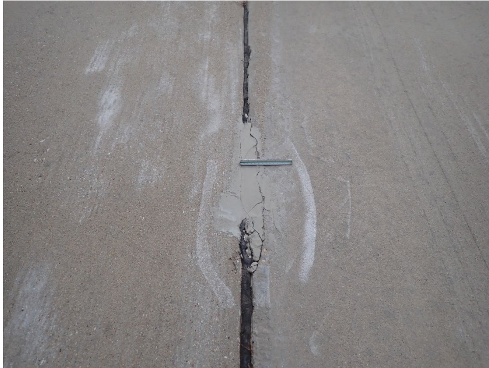
R15HL-05. Joint Seal Damage (Sample Unit No. 07).
