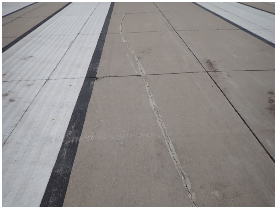
R15HL-05. LTD Cracking (Sample Unit No. 24).
