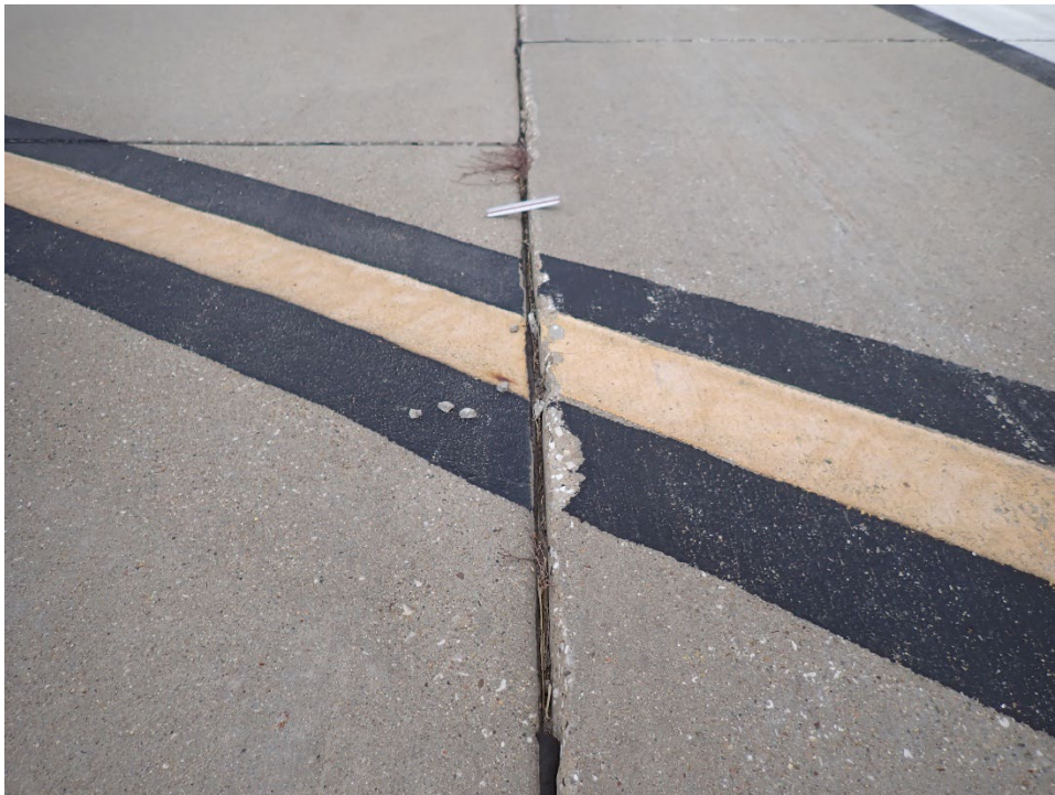
T01HL-01. Faulting (Sample Unit No. 02).
