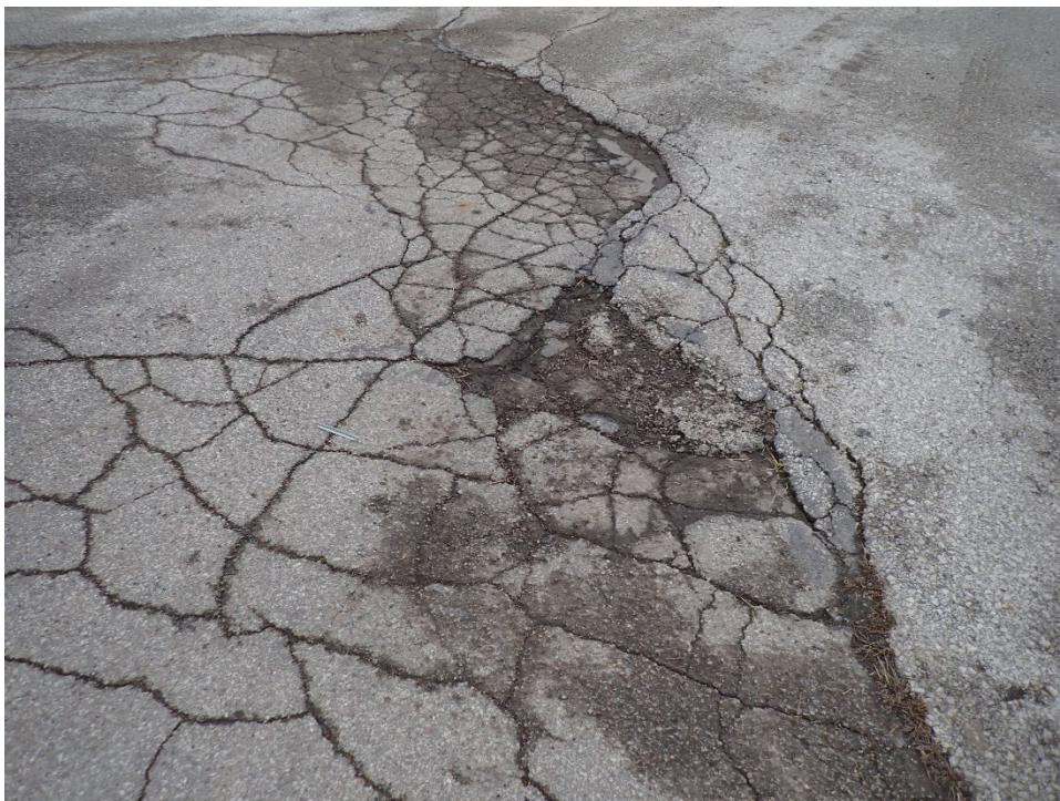
TH01HL-03. Alligator Cracking (Sample Unit No. 01) (2).
