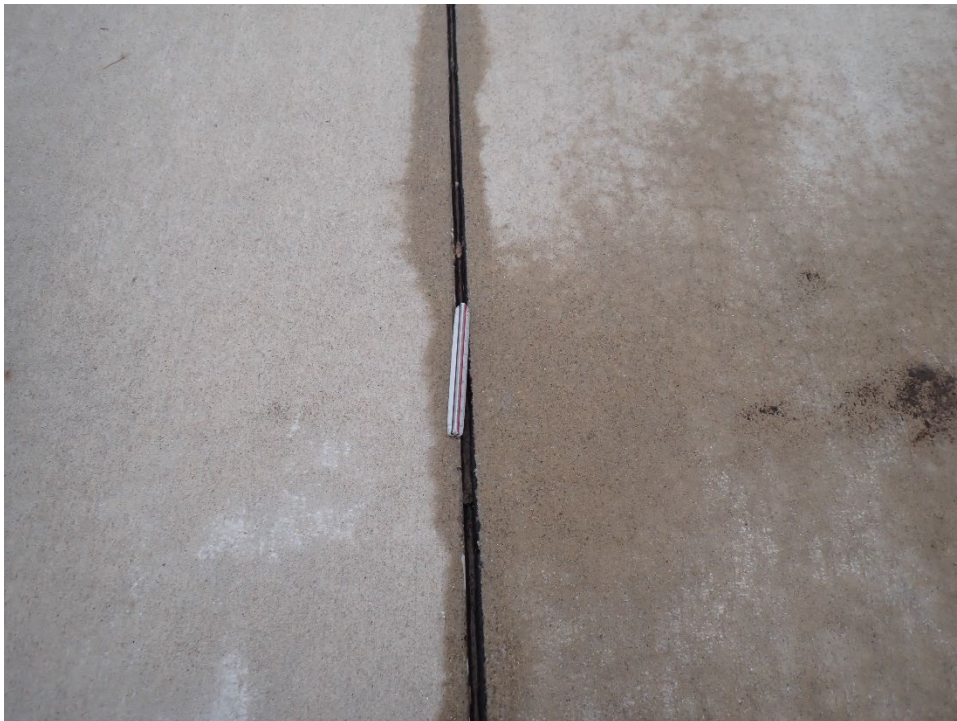
A01HL-01. Joint Seal Damage (Sample Unit No. 11).
