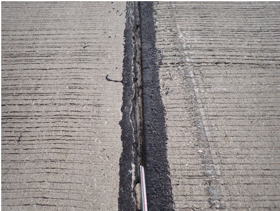
R15HL-03. Joint Seal Damage (Sample Unit No. 03).
