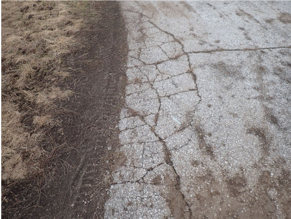
TH01HL-03. Alligator Cracking (Sample Unit No. 01) (1).
