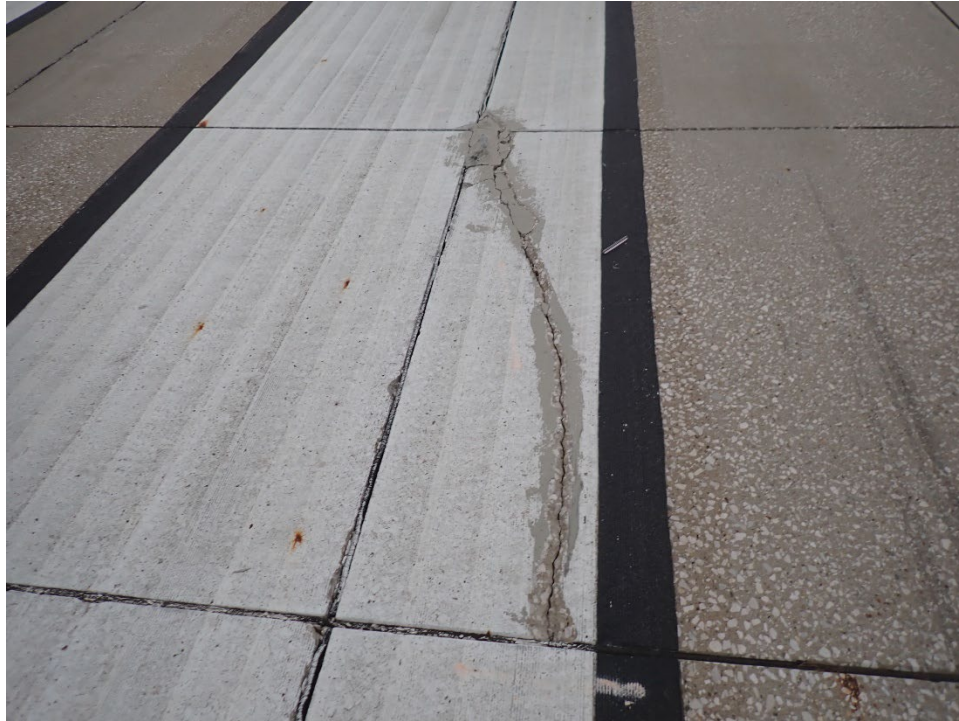
R15HL-05. LTD Cracking (Sample Unit No. 27).
