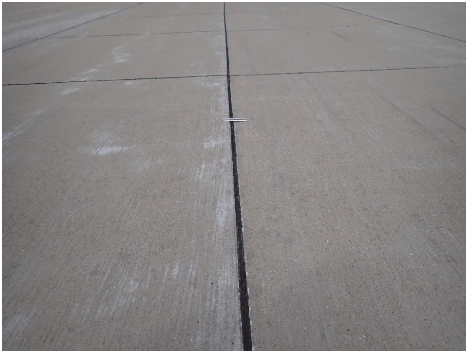
R15HL-05. Faulting (Sample Unit No. 14).
