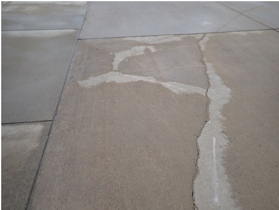
A01HL-02. Shattered Slab (Sample Unit No. 01).
