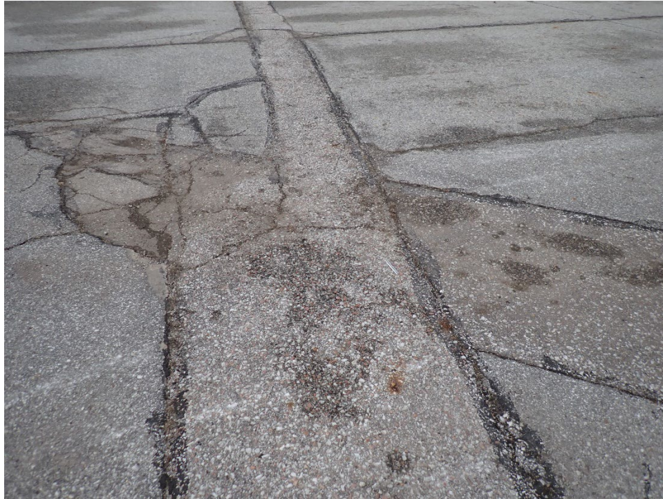
TH01HL-04. Patching (Sample Unit No. 01).
