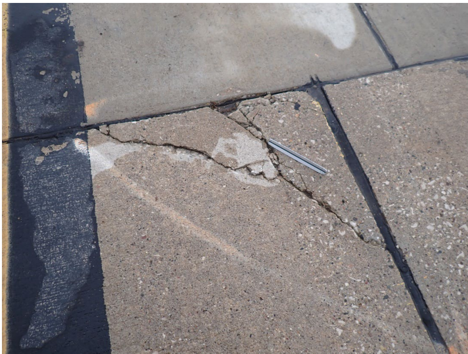
A01HL-02. Corner Spalling (Sample Unit No. 01).
