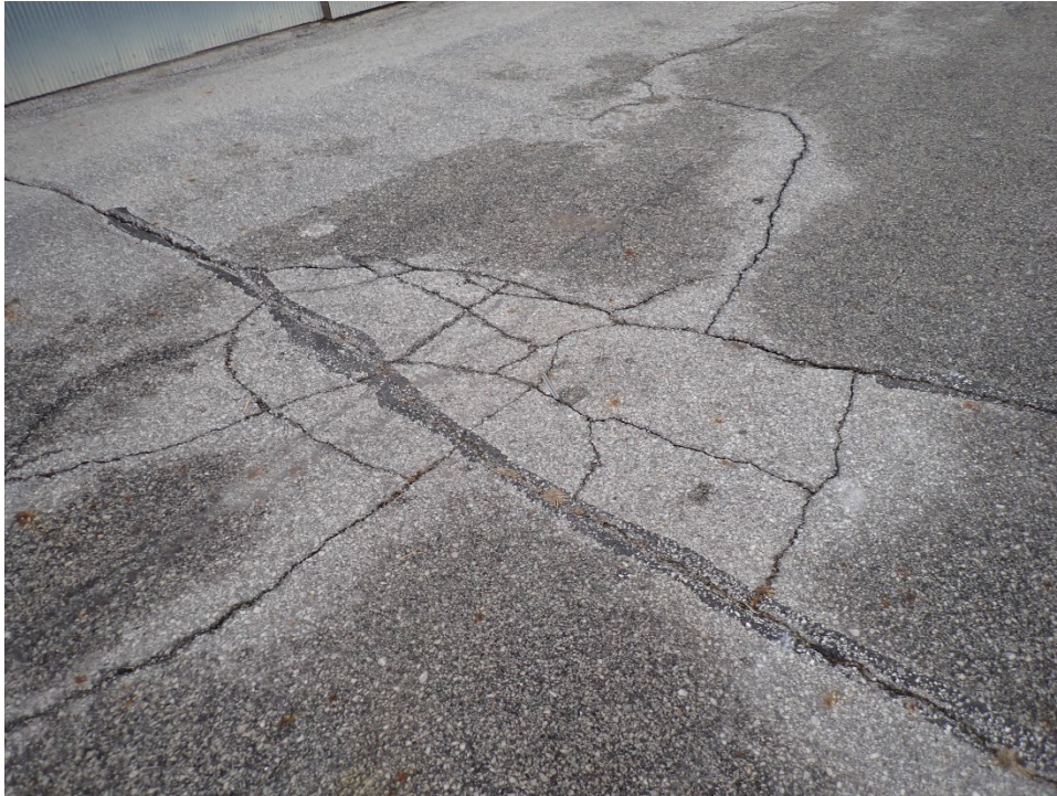
TH01HL-04. Alligator Cracking (Sample Unit No. 01).
