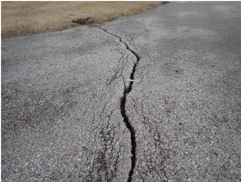
TH01HL-02. L&T Cracking (Sample Unit No. 05) (1).
