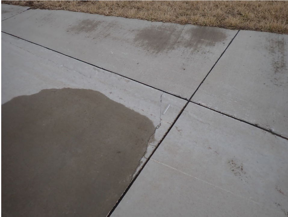
TH01HL-01. Joint Spalling (Sample Unit No. 10).
