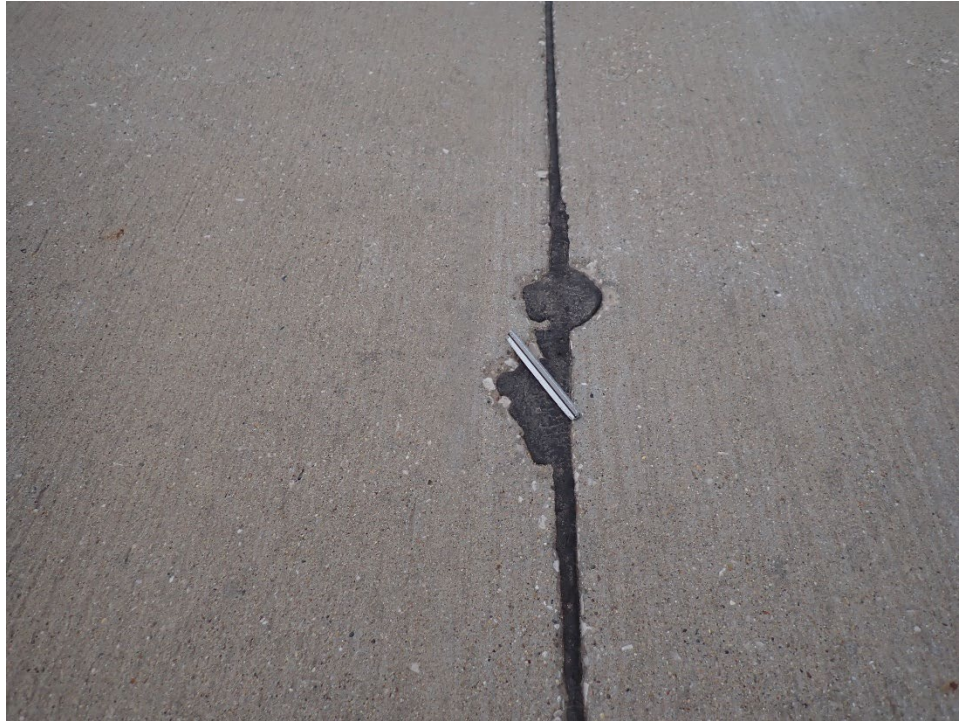
R15HL-02. Joint Spalling (Sample Unit No. 12).
