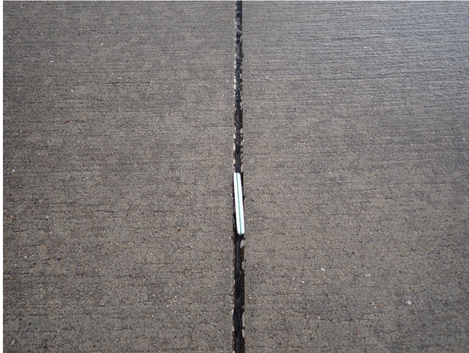
T02HL-03. Joint Seal Damage (Sample Unit No. 35).
