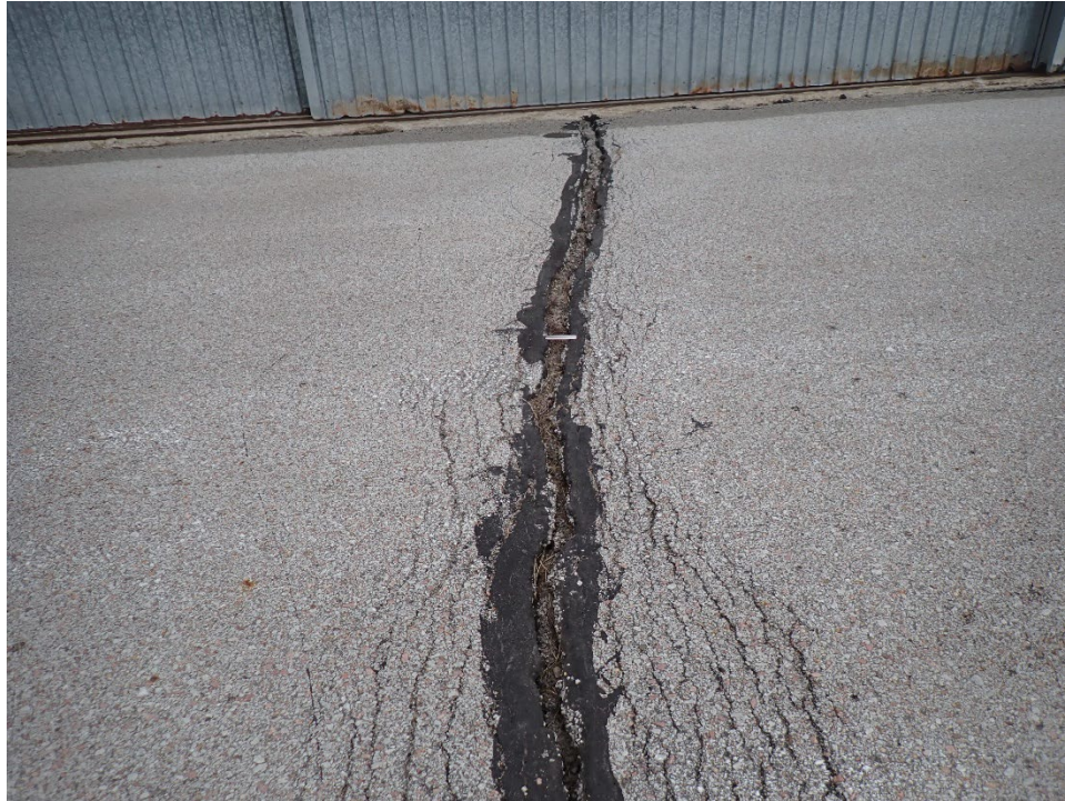
TH01HL-02. L&T Cracking (Sample Unit No. 05) (2).
