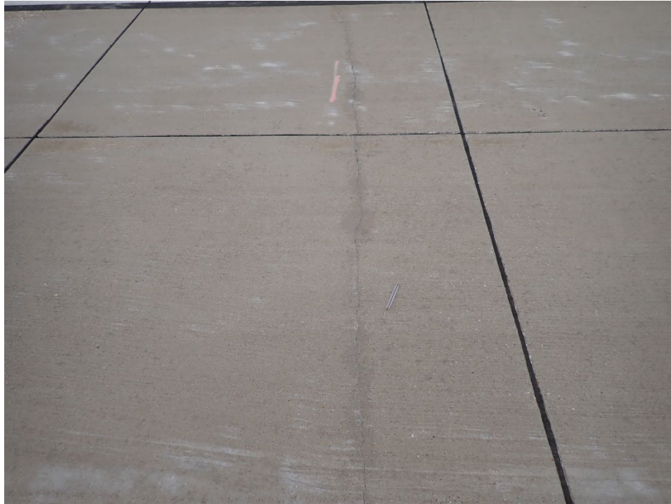
R15HL-01. LTD Cracking (Sample Unit No. 015).
