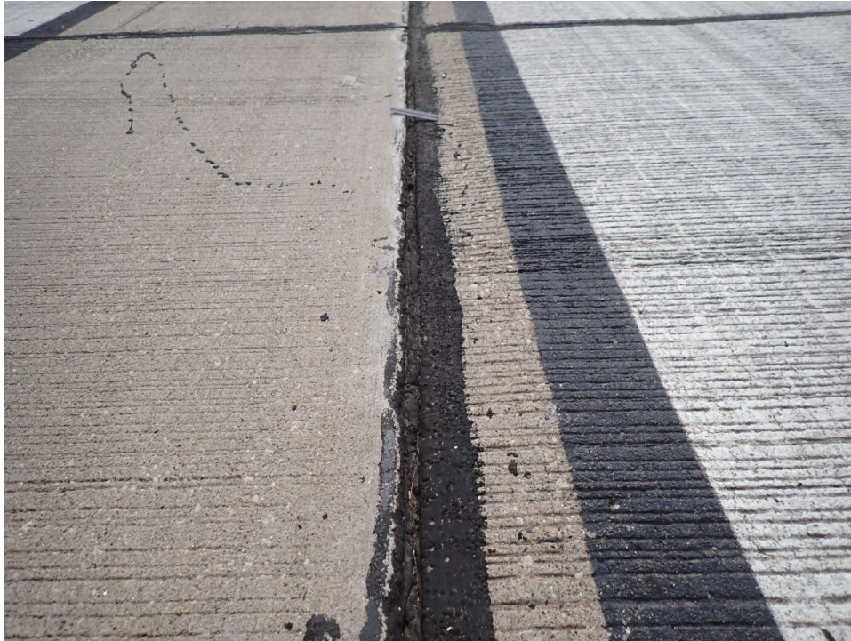
R15HL-03. Faulting (Sample Unit No. 11).
