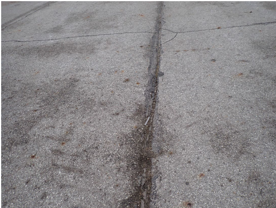
TH01HL-04. L&T Cracking (Sample Unit No. 01).
