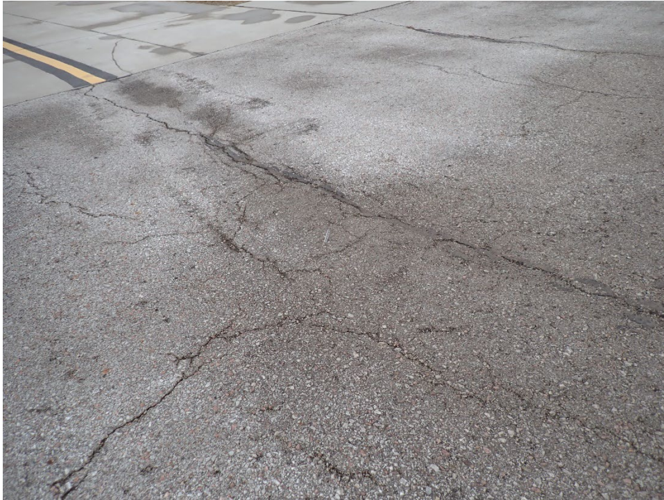
TH01HL-02. Alligator Cracking (Sample Unit No. 06).
