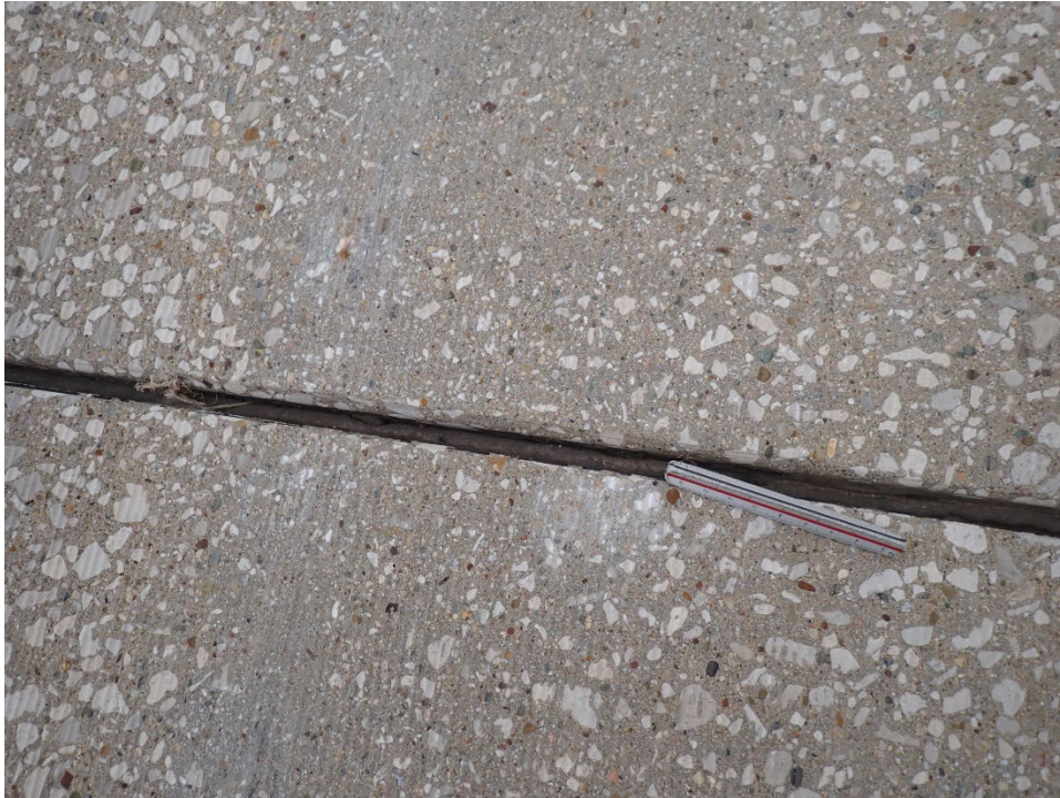
R15HL-01. Joint Seal Damage (Sample Unit No. 065).
