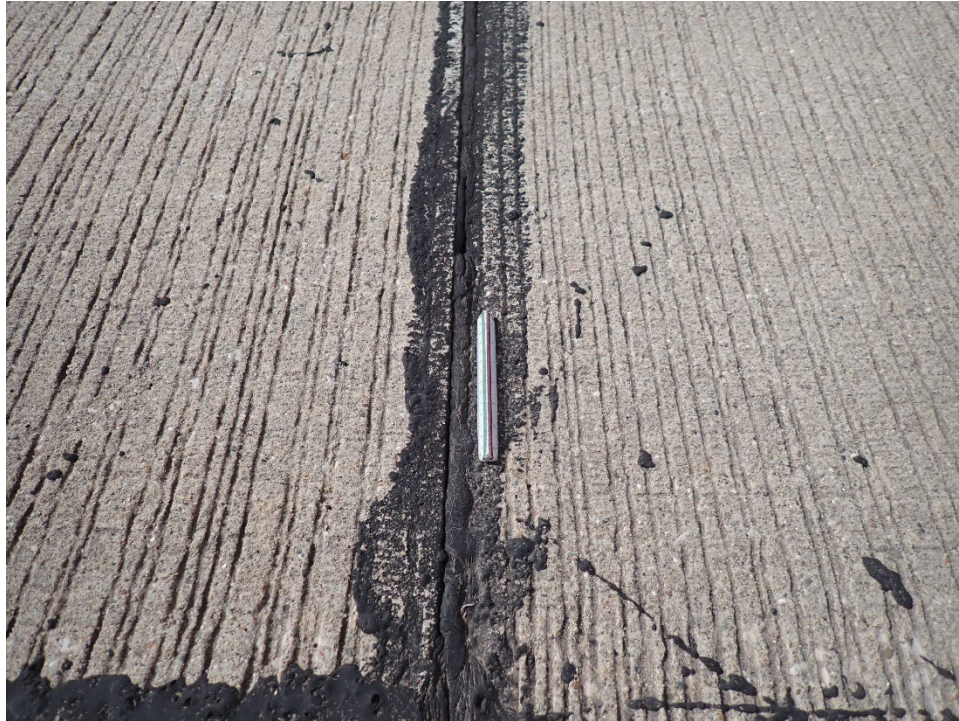
R15HL-03. Joint Seal Damage (Sample Unit No. 08).
