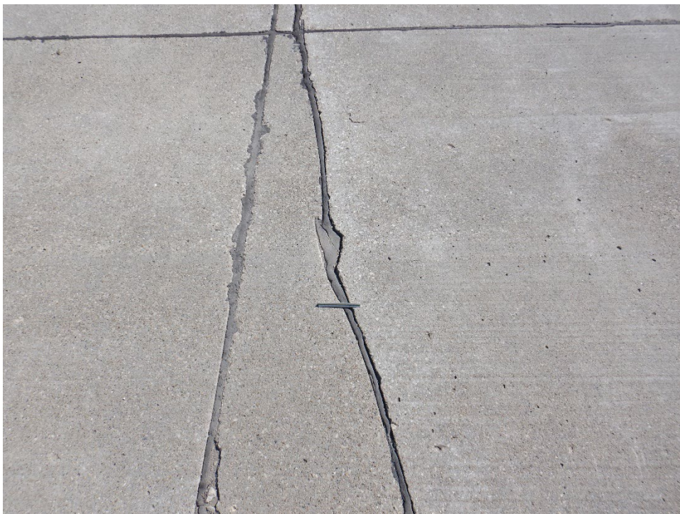
A01GL-03. LTD Cracking (Sample Unit No. 02).
