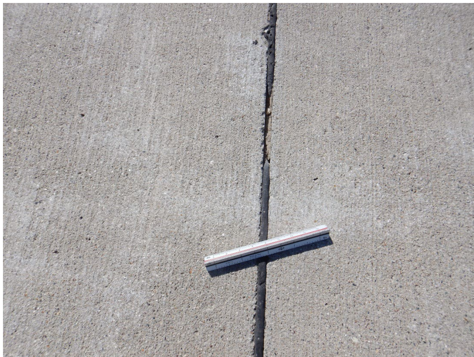
A01GL-06. Joint Seal Damage (Sample Unit No. 01).
