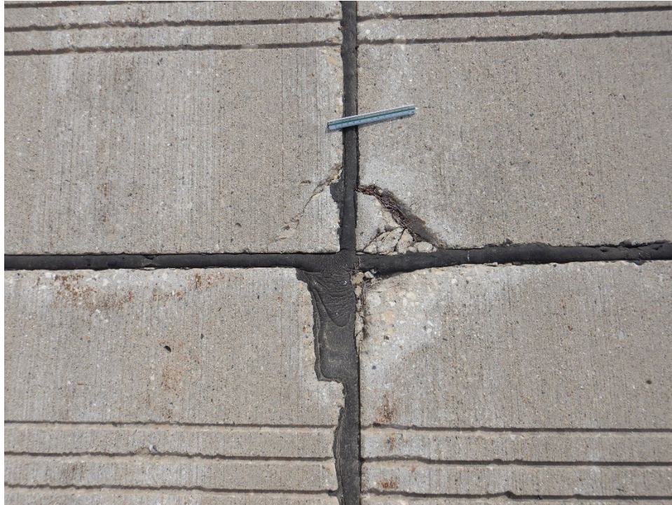
R13GL-02 Corner Spalling. (Additional Sample Unit No. 20).
