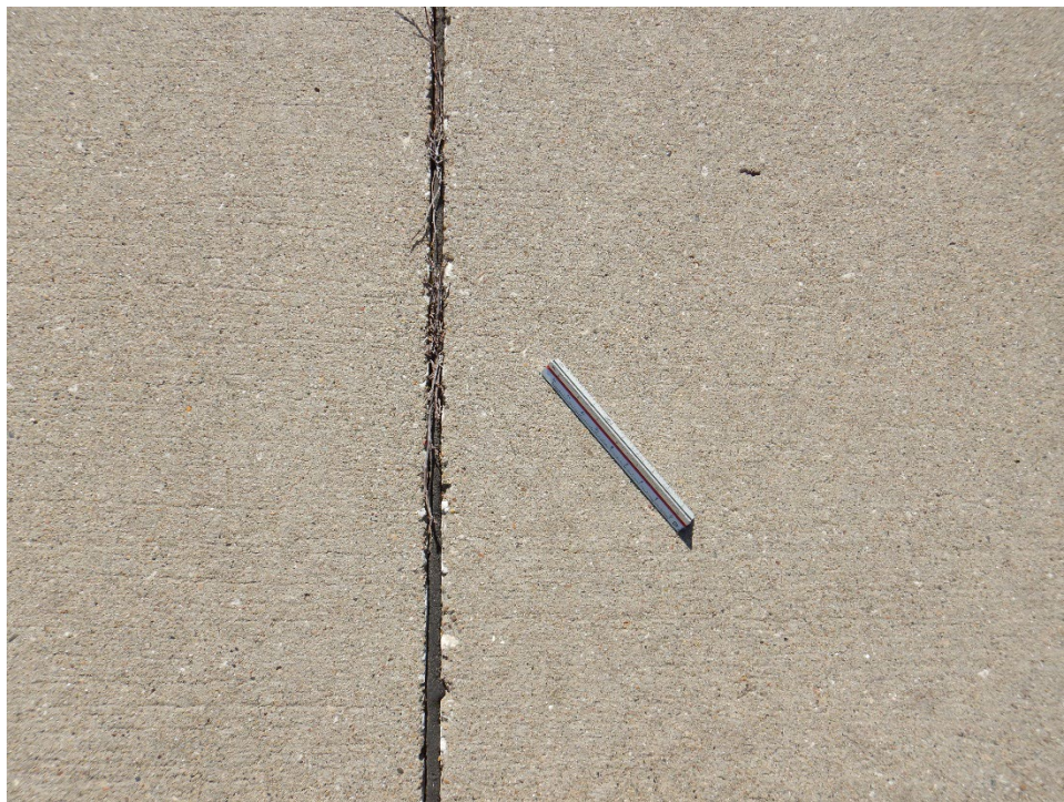
T02GL-01. Joint Seal Damage (Sample Unit No. 01).
