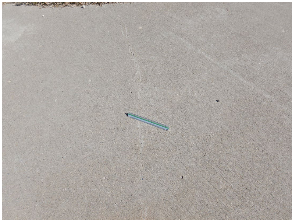
A01GL-05. LTD Cracking (Sample Unit No. 01).
