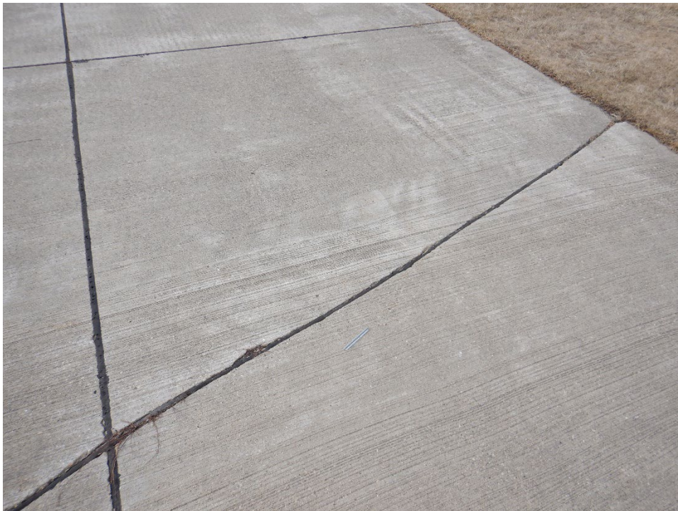
R13GL-04. LTD Cracking (Sample Unit No. 01).
