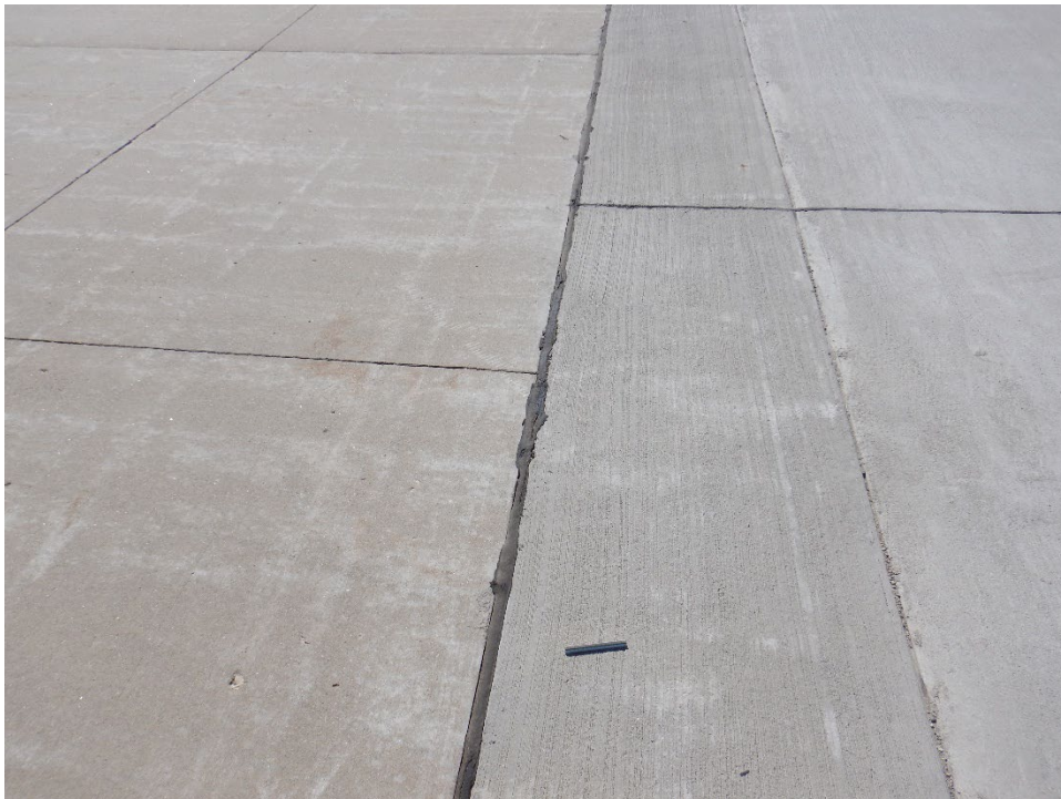
TH01GL-01. Large Patching (Sample Unit No. 05).
