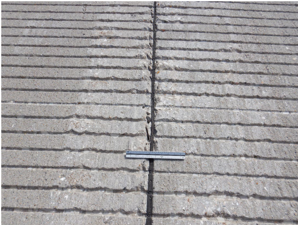
R13GL-01. Joint Seal Damage (Sample Unit No. 135).
