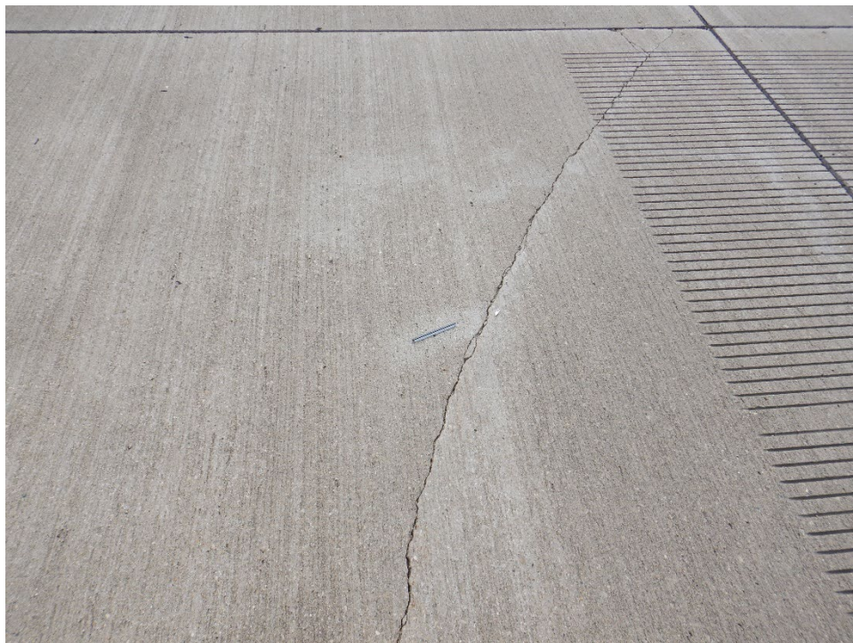
R13GL-02 LTD Cracking. (Additional Sample Unit No. 16).
