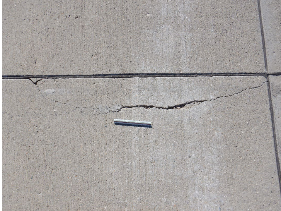
T01GL-01. Joint Spalling (Sample Unit No. 09).
