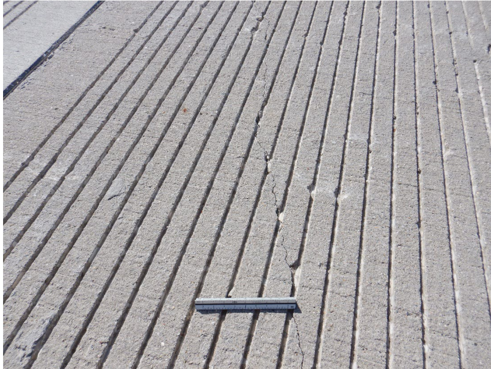
R13GL-01. LTD Cracking (Sample Unit No. 45).
