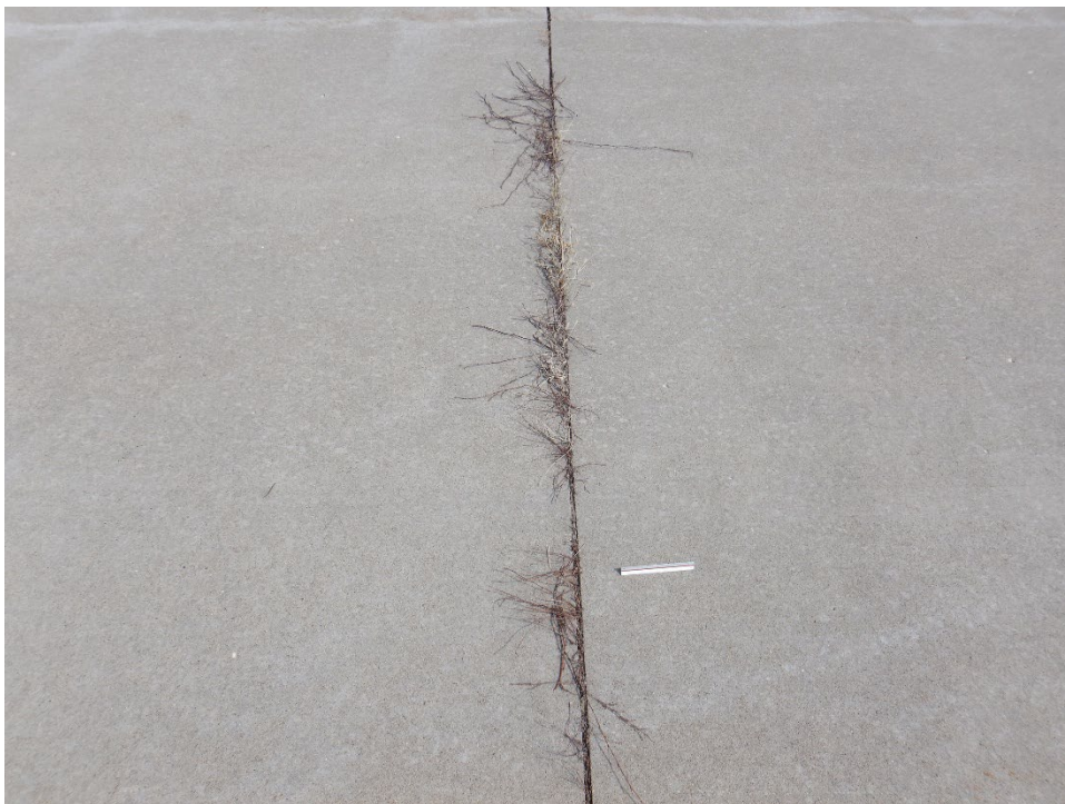
R13GL-05. Joint Seal Damage (Sample Unit No. 03).
