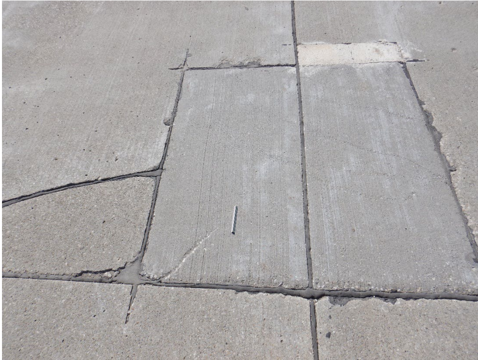
A01GL-03. Small Patching (Sample Unit No. 02).
