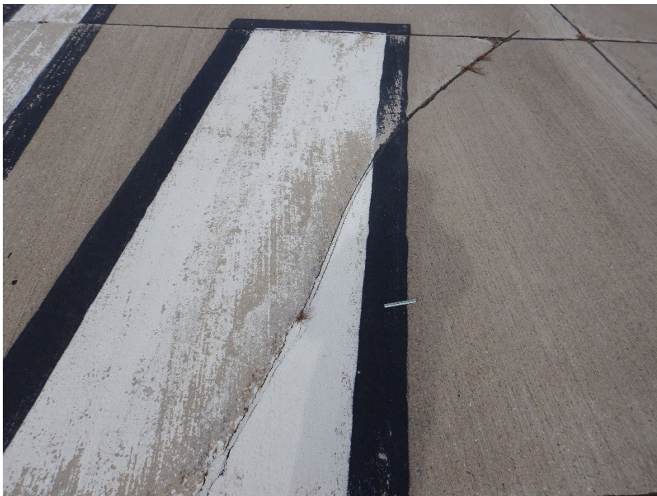
R13GL-03. LTD Cracking (Sample Unit No. 03).
