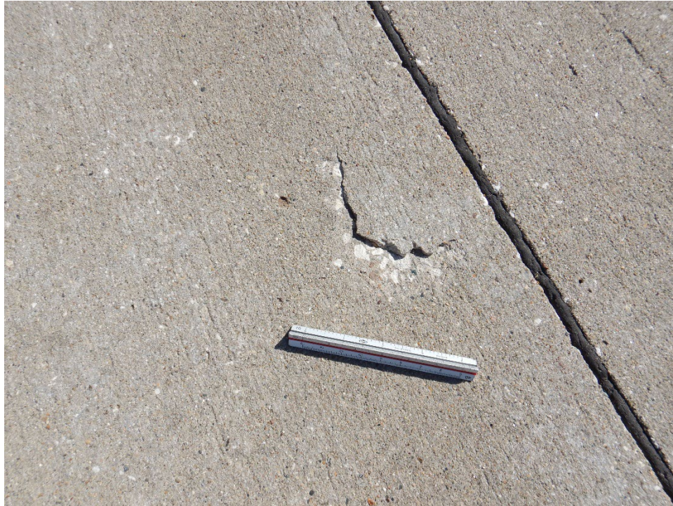
T02GL-01. Shrinkage Cracking (Sample Unit No. 01).
