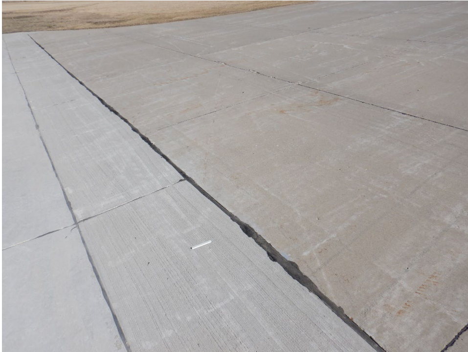
TH01GL-01. Large Patching (Sample Unit No. 01).
