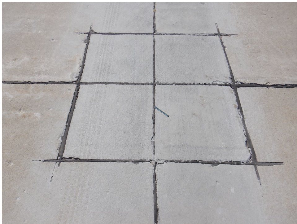
A01GL-01. Small Patching (Sample Unit No. 06).
