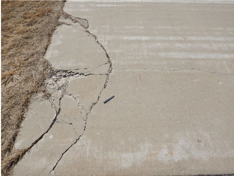
TH01GL-01. Shattered Slab (Sample Unit No. 08).
