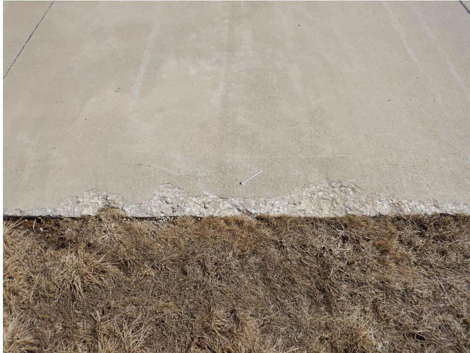
TH01GL-02. Joint Spalling (Sample Unit No. 02).
