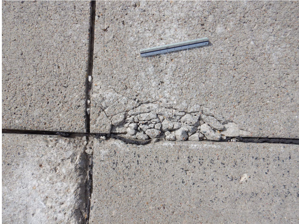
R13GL-05. Joint Spalling (Sample Unit No. 05).
