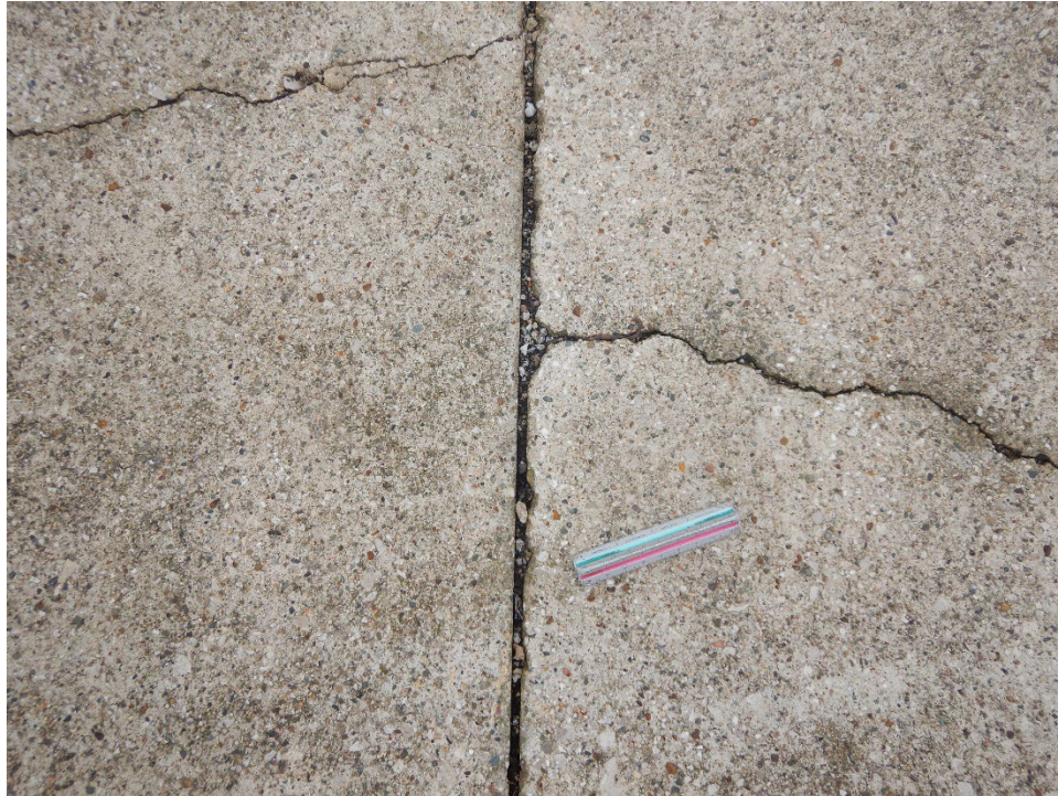
TH01GR-02. Joint Seal Damage (Sample Unit No. 01).
