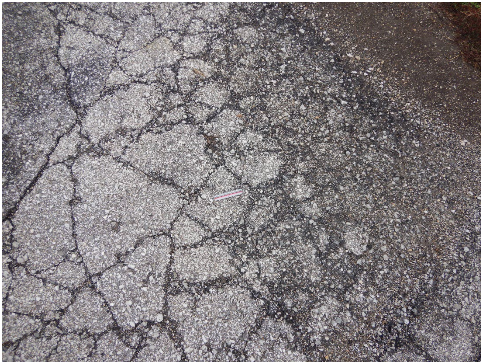
TH01GR-01. Alligator Cracking (Sample Unit No. 01).
