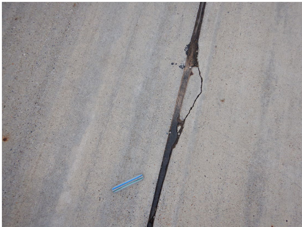
A02GR-01. Joint Spalling (Sample Unit No. 03).
