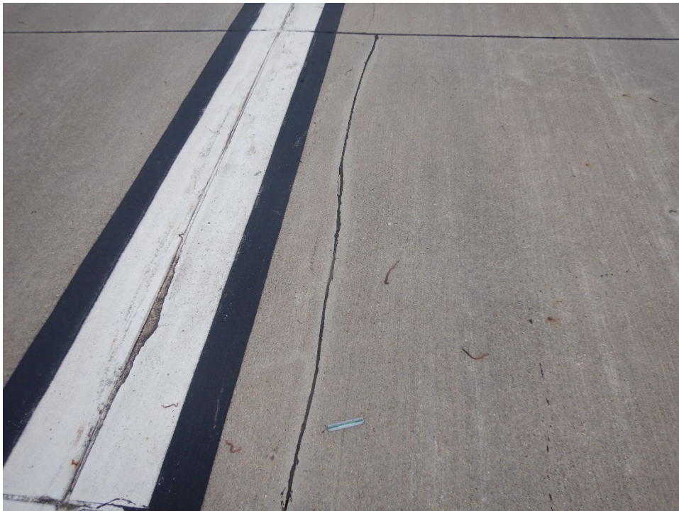
R14GR-01. LTD Cracking (Sample Unit No. 32).
