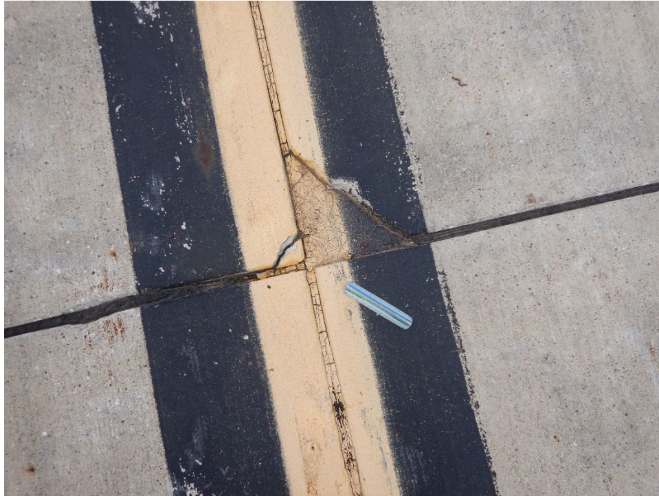
T02GR-01. Corner Spalling (Sample Unit No. 02).
