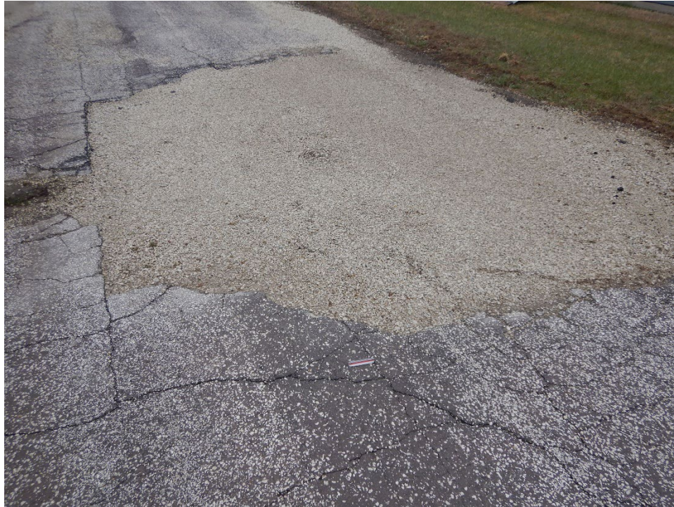
TH02GR-02. Alligator Cracking (Sample Unit No. 01) (1).
