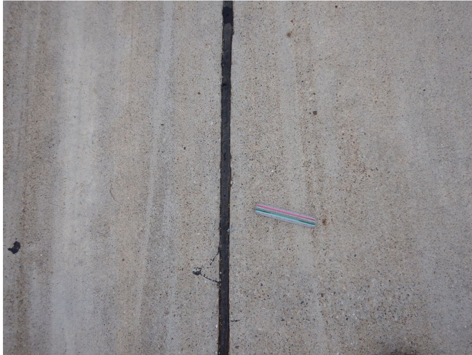
A02GR-01. Joint Seal Damage (Sample Unit No. 03).
