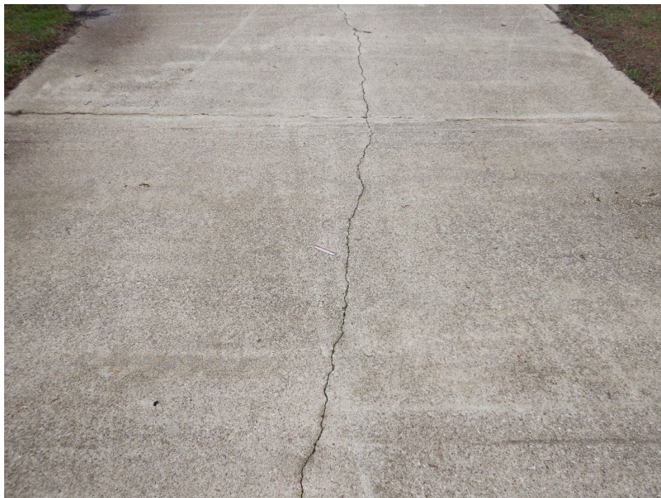
TH01GR-02. Shattered Slab (Sample Unit No. 01).
