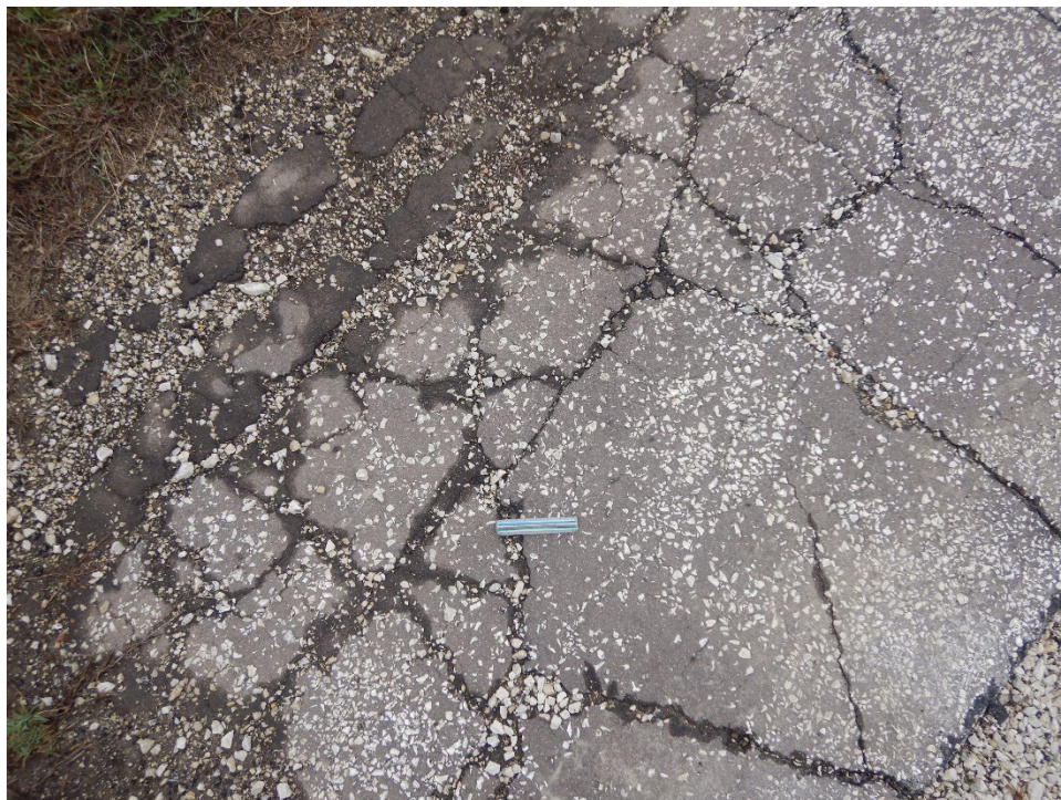
TH02GR-02. Alligator Cracking (Sample Unit No. 01) (2).
