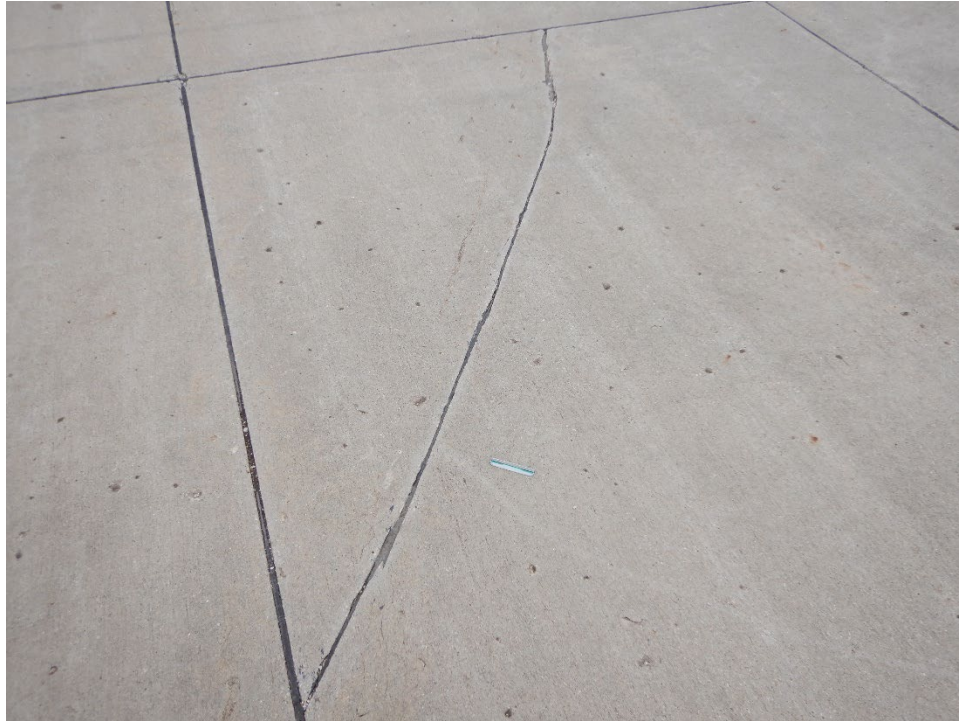
TH02GR-01. LTD Cracking (Sample Unit No. 02).
