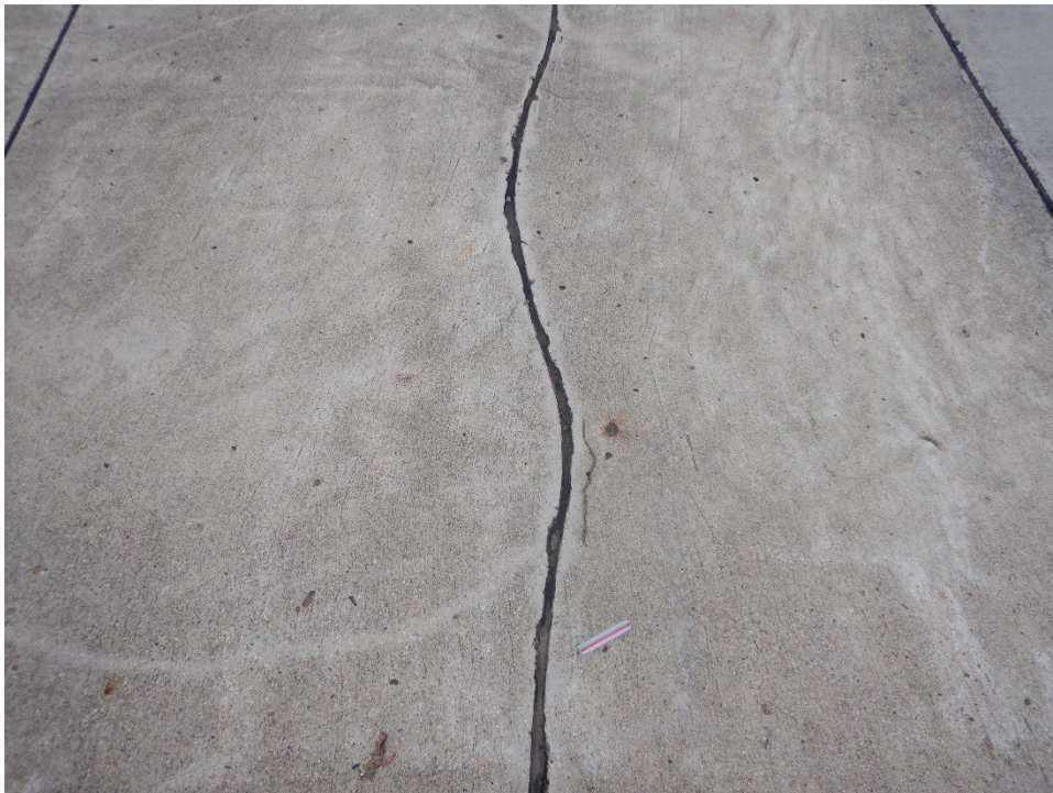
R14GR-02. LTD Cracking (Sample Unit No. 01).
