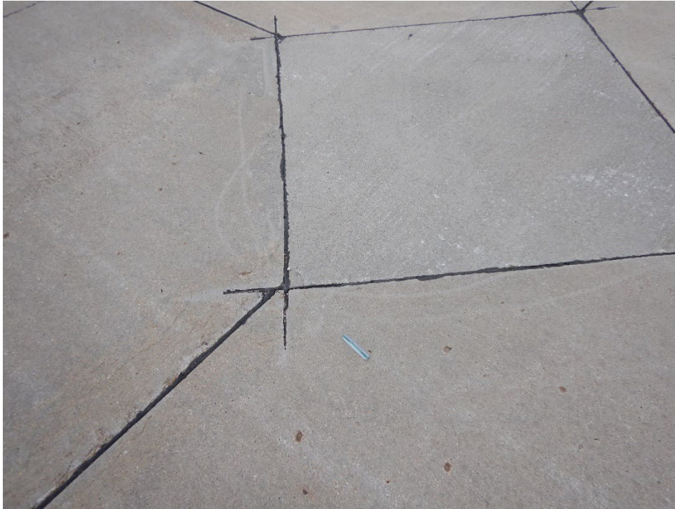
A01GR-01. Large Patching (Sample Unit No. 09).
