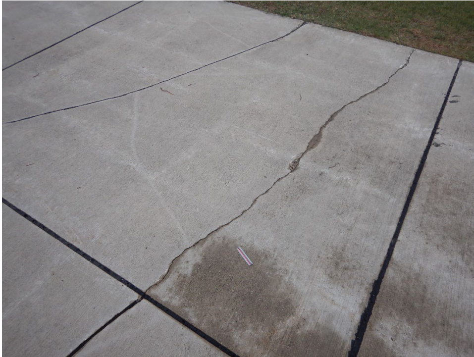
R07GR-02. LTD Cracking (Sample Unit No. 01).
