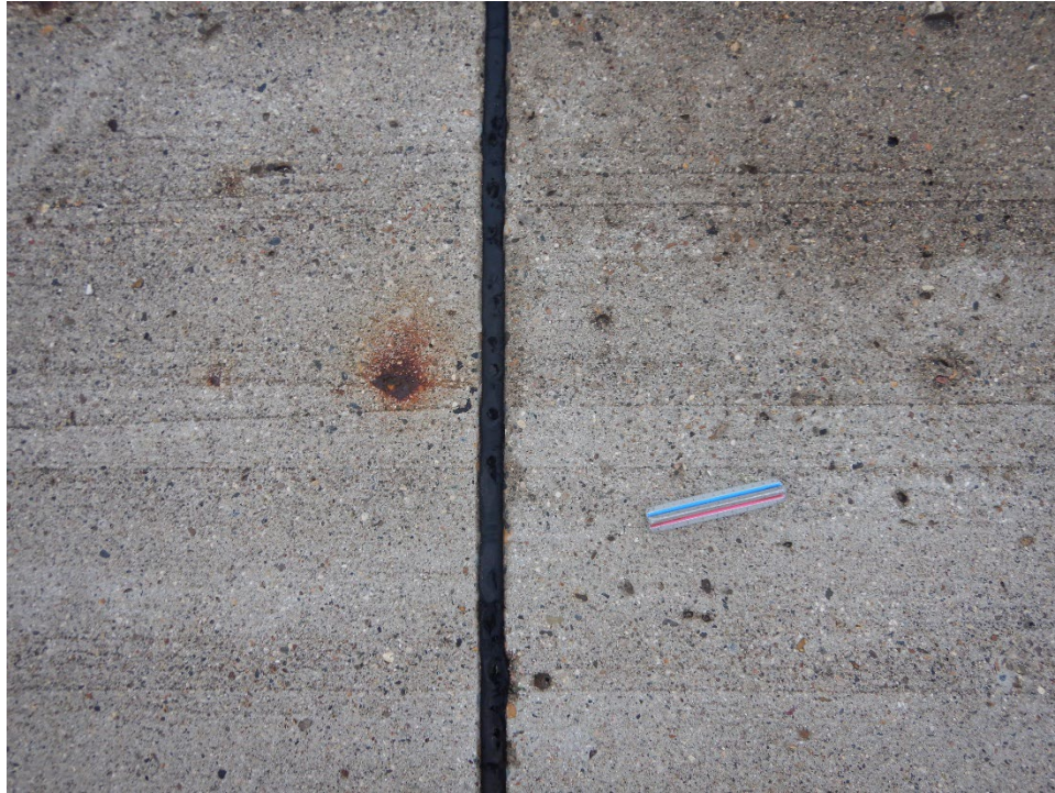
R07GR-01. Joint Seal Damage (Sample Unit No. 85).
