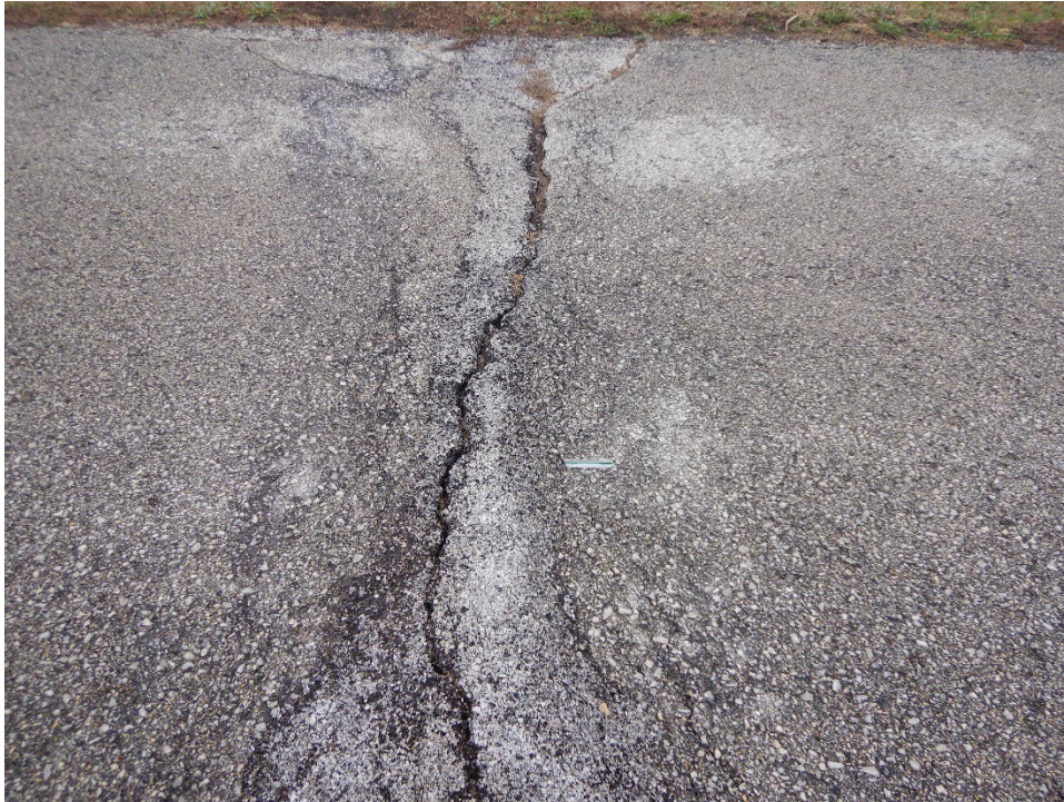
TH01GR-01. L&T Cracking (Sample Unit No. 01).
