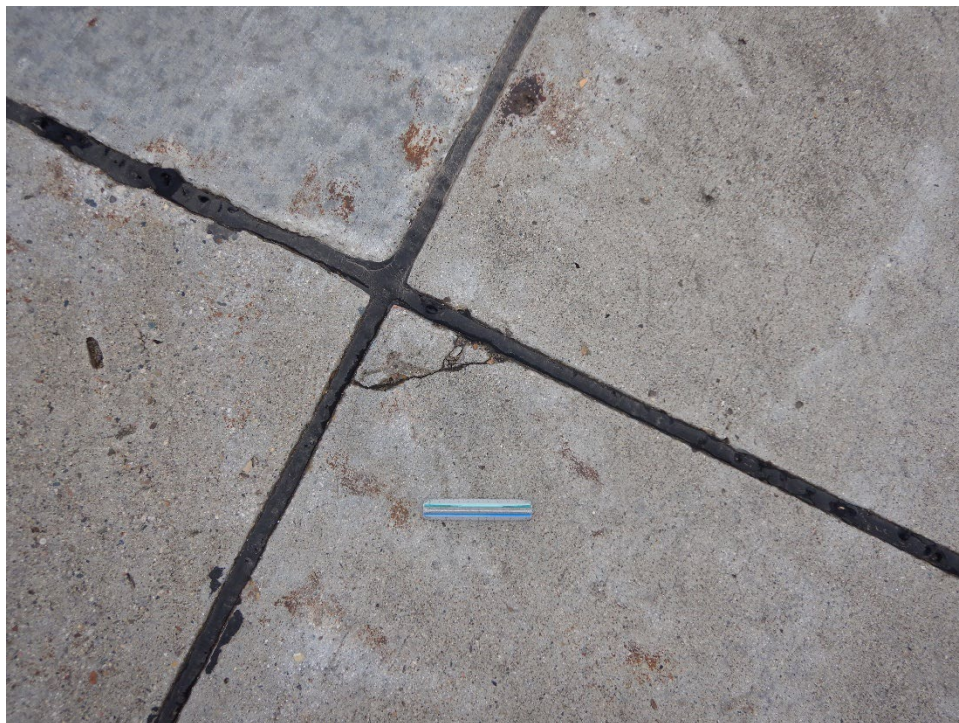
R14GR-03. Corner Spalling (Sample Unit No. 01).
