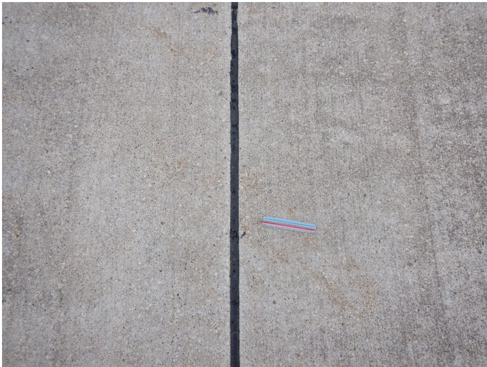
T01GR-02. Joint Seal Damage (Sample Unit No. 01).
