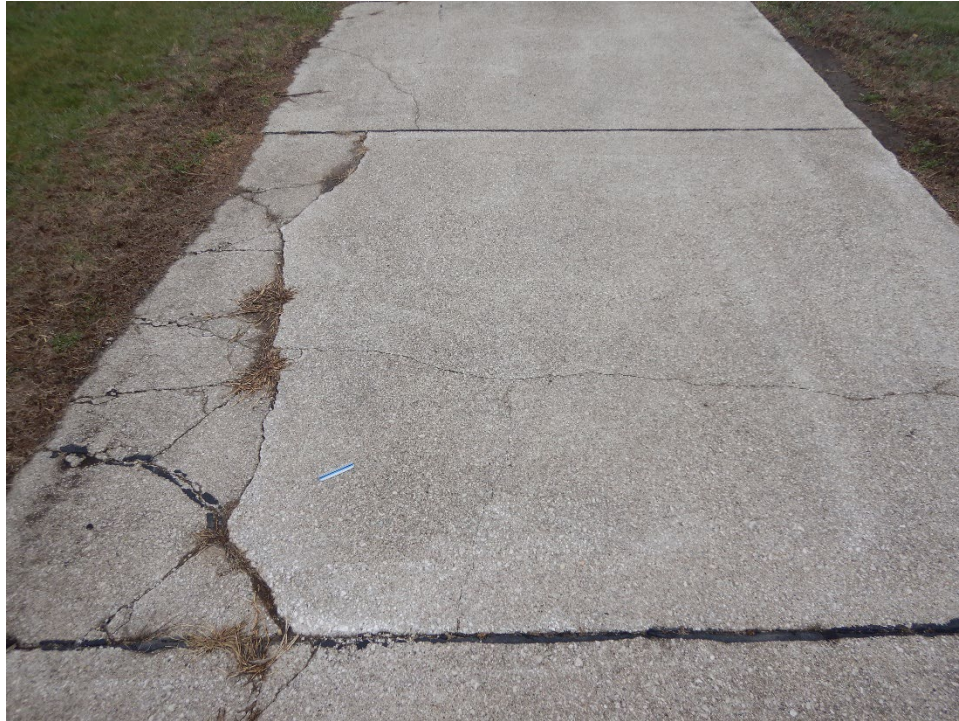
TH02GR-03. Shattered Slab (Sample Unit No. 01).
