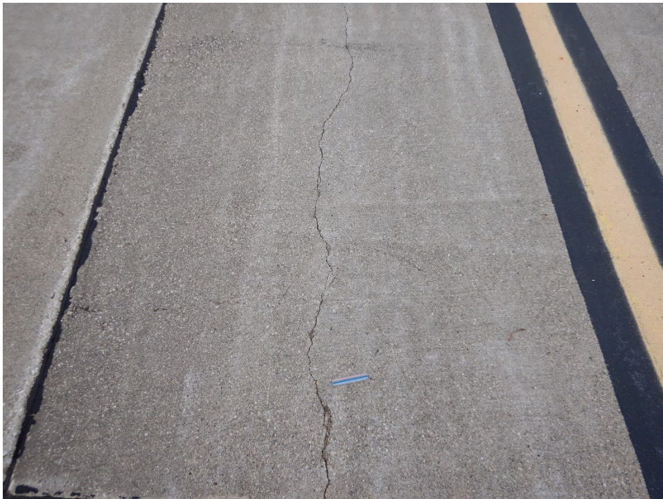
T01GR-01. LTD Cracking (Sample Unit No. 02).
