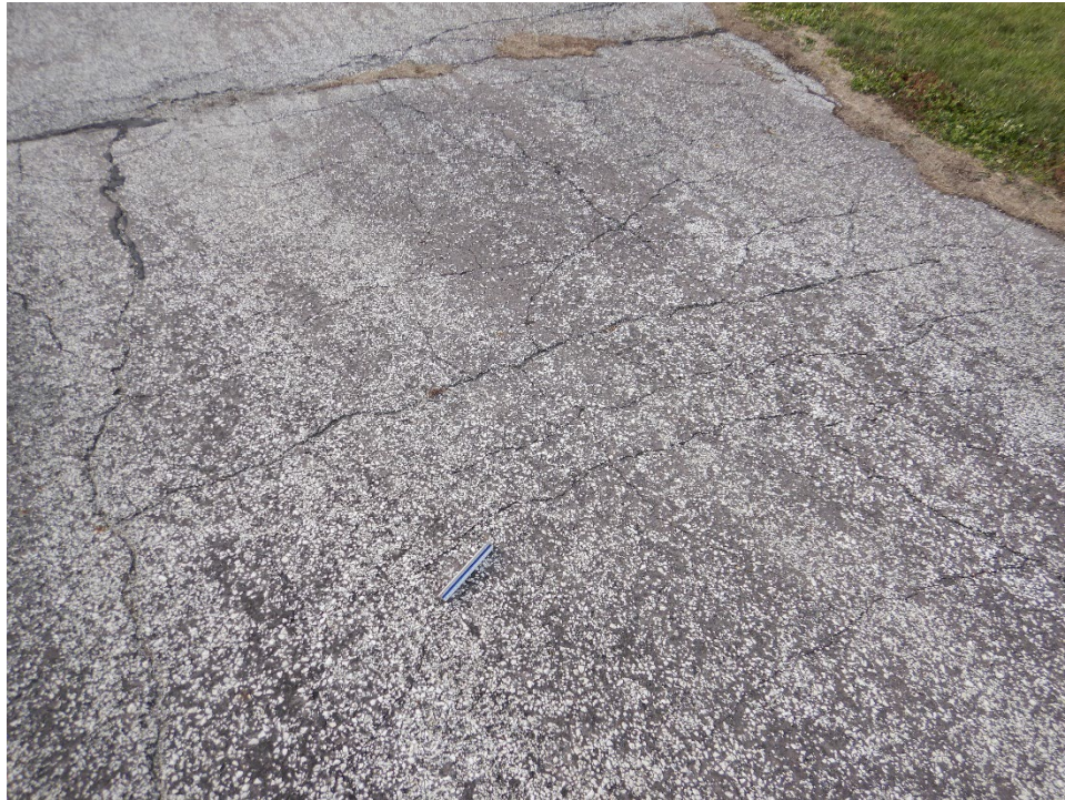
TH02GR-02. Alligator Cracking (Sample Unit No. 01).
