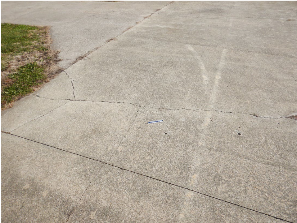
TH01GR-02. Shattered Slab (Sample Unit No. 01).
