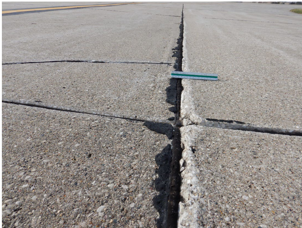
T01GR-01. Faulting (Sample Unit No. 02).
