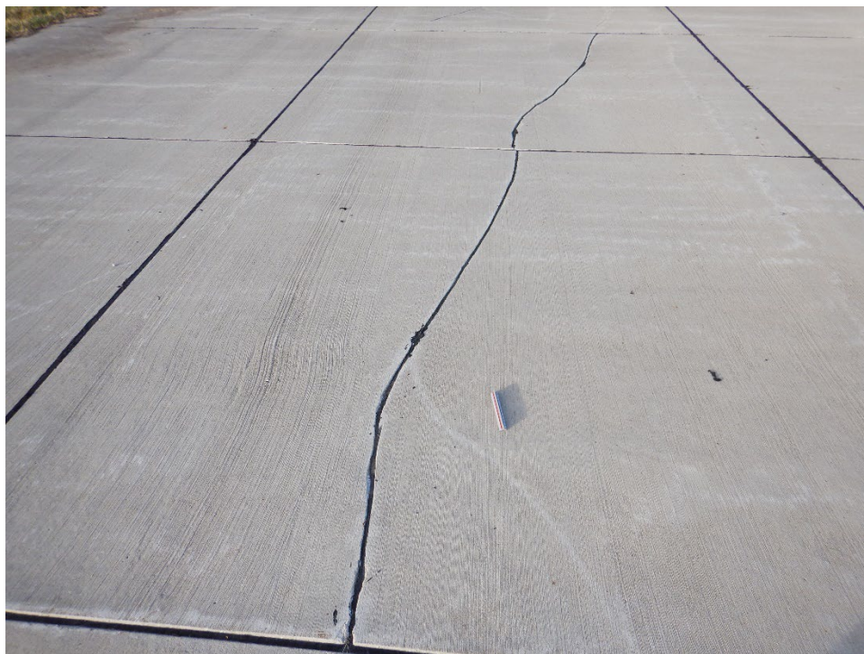
R07GR-02. LTD Cracking (Sample Unit No. 01).
