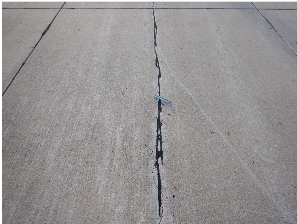
R14GR-01. LTD Cracking (Sample Unit No. 33).
