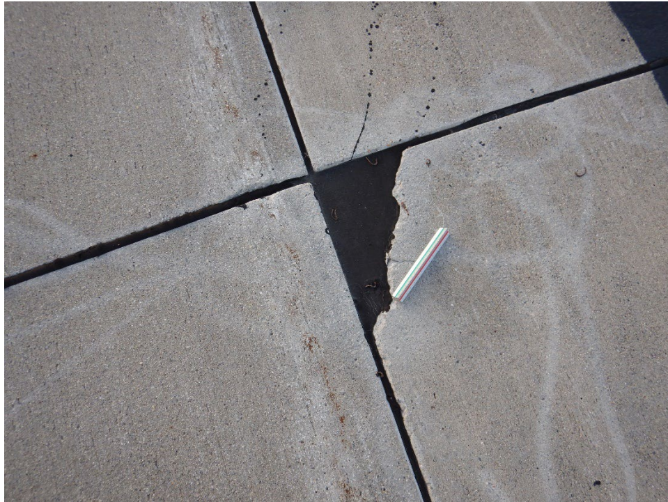
R14GR-04. Corner Spalling (Sample Unit No. 19).
