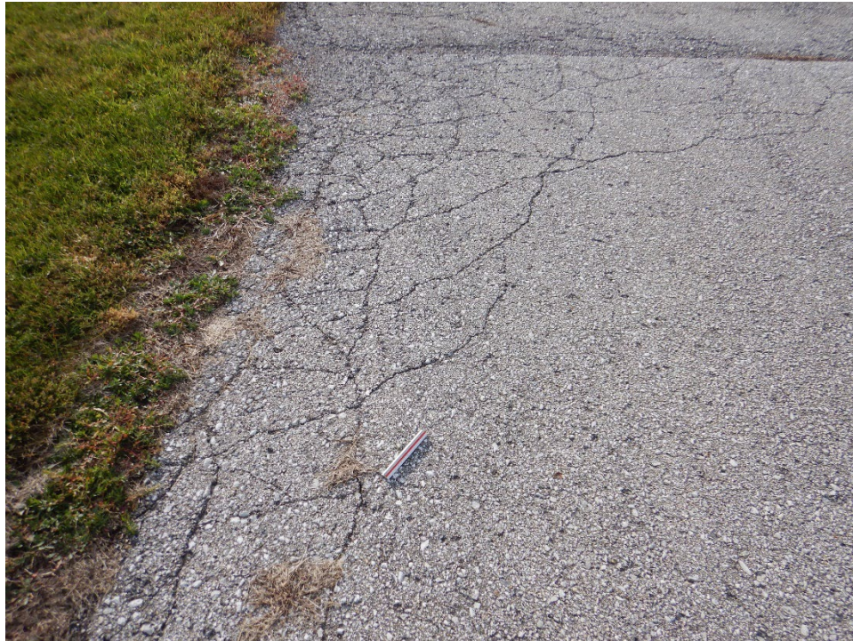
TH01GR-01. Alligator Cracking (Sample Unit No. 01).
