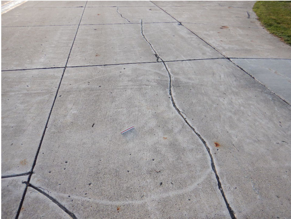
R14GR-02. LTD Cracking (Sample Unit No. 01).
