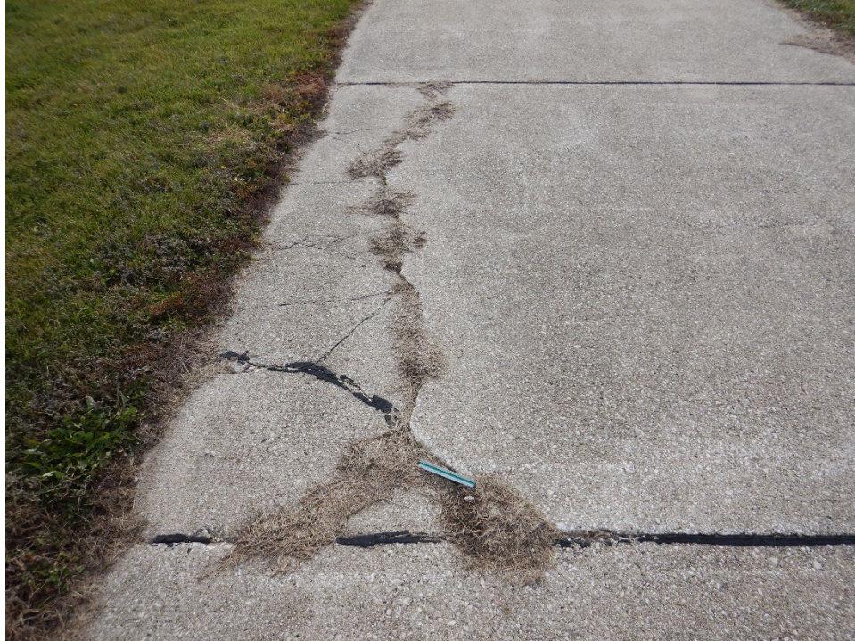
TH02GR-03. Shattered Slab (Sample Unit No. 01).
