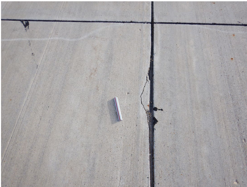
A02GR-01. Joint Spalling (Sample Unit No. 03).
