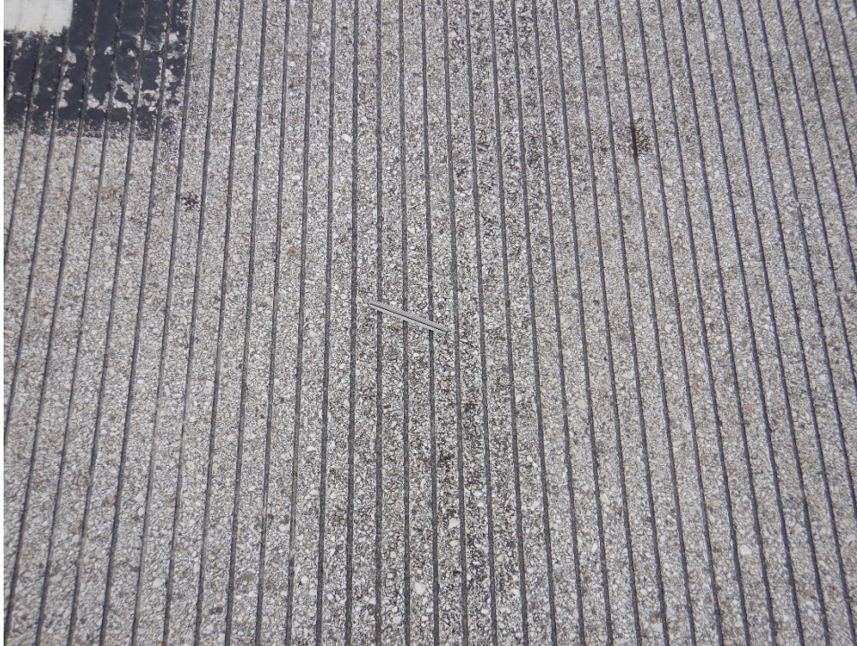
R06FD-01. Weathering (Sample Unit No. 05).
