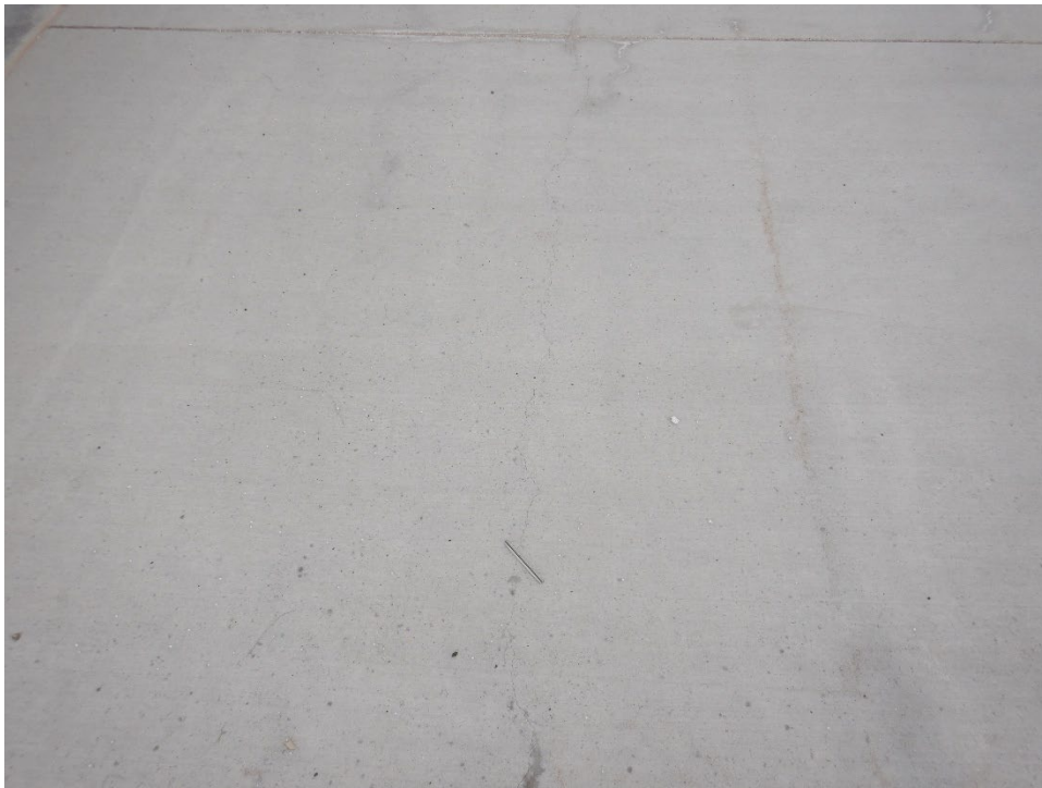
TH01FD-05. LTD Cracking (Sample Unit No. 01).
