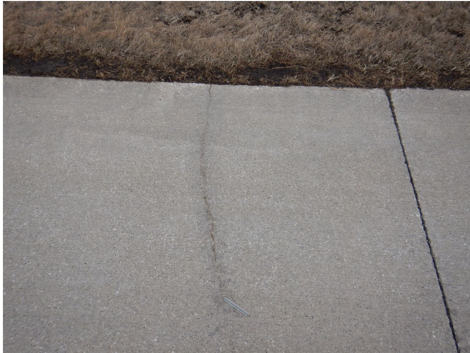
TCFD-01. Shrinkage Cracking (Sample Unit No. 02).
