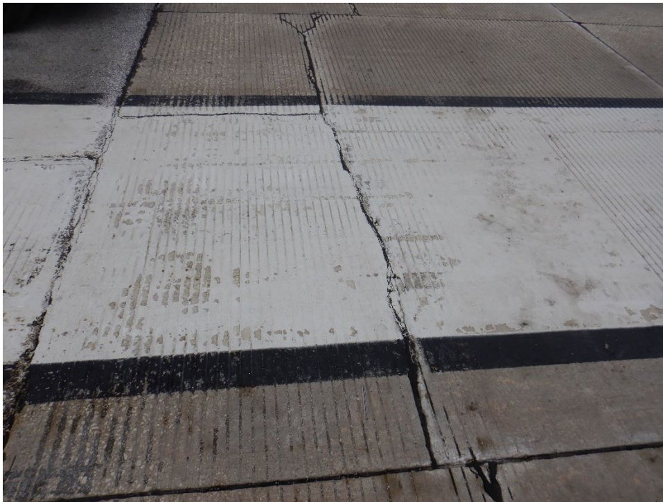
R12FD-03. LTD Cracking (Sample Unit No. 04).
