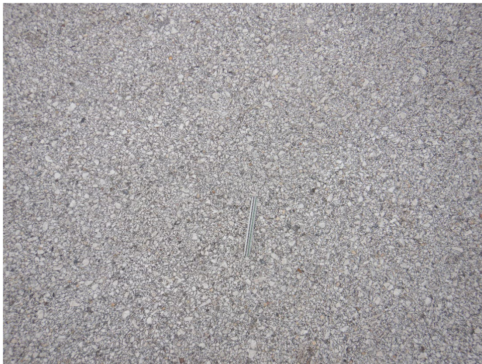
TBFD-01. Weathering (Sample Unit No. 03).
