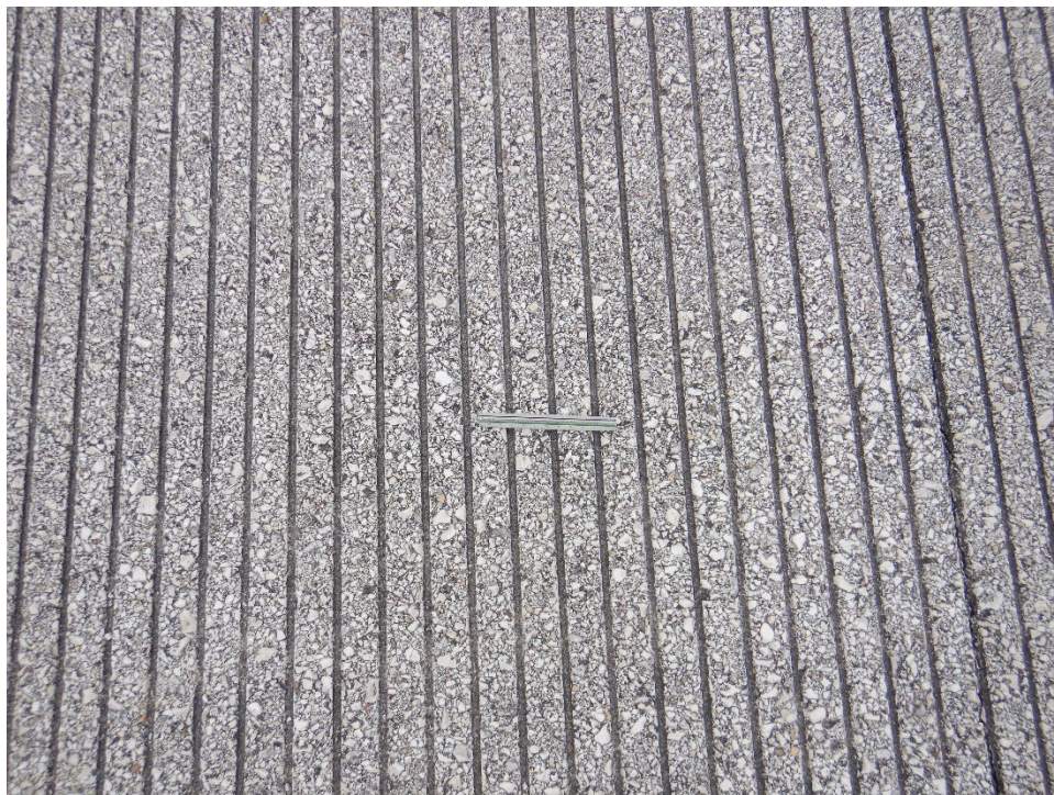
R12FD-01. Weathering (Sample Unit No. 24).
