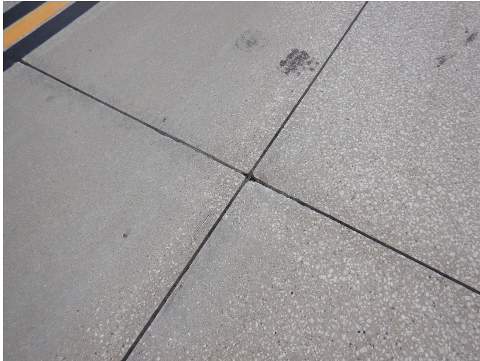
TDFD-03. Joint Seal Damage (Sample Unit No. 02).
