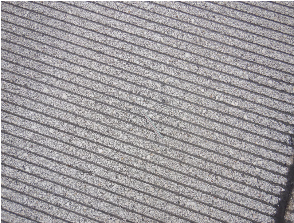
R12FD-02. Weathering (Sample Unit No. 53).
