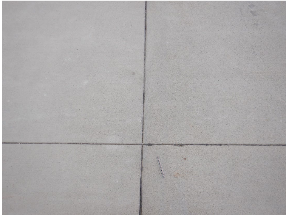
TH01FD-02. Joint Seal Damage (Sample Unit No. 01).
