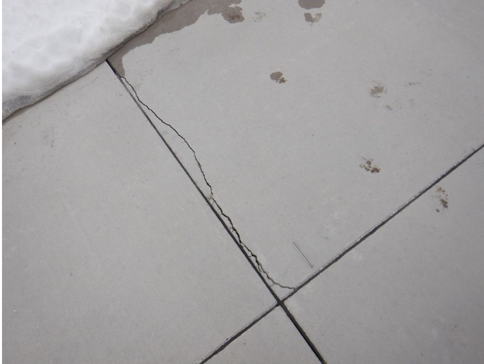
TAFD-02. Joint Spalling (Additional Sample Unit No. 05).
