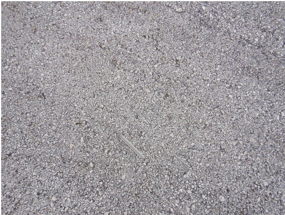
TBFD-04. Weathering (Sample Unit No. 01).
