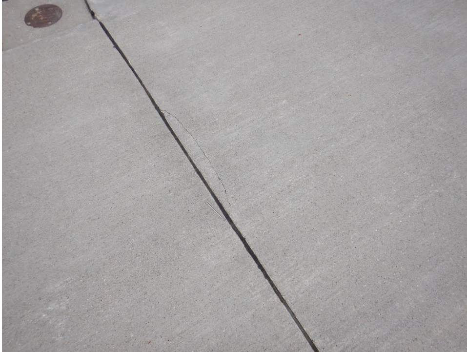
A01FD-02. Joint Spalling (Sample Unit No. 01).
