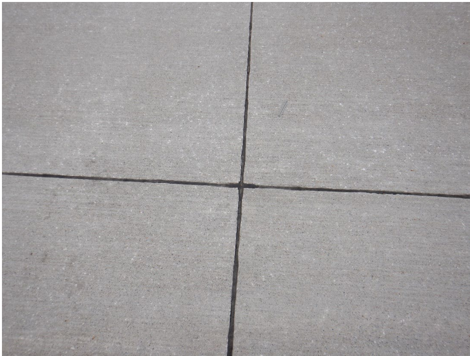
A01FD-02. Joint Seal Damage (Sample Unit No. 09).
