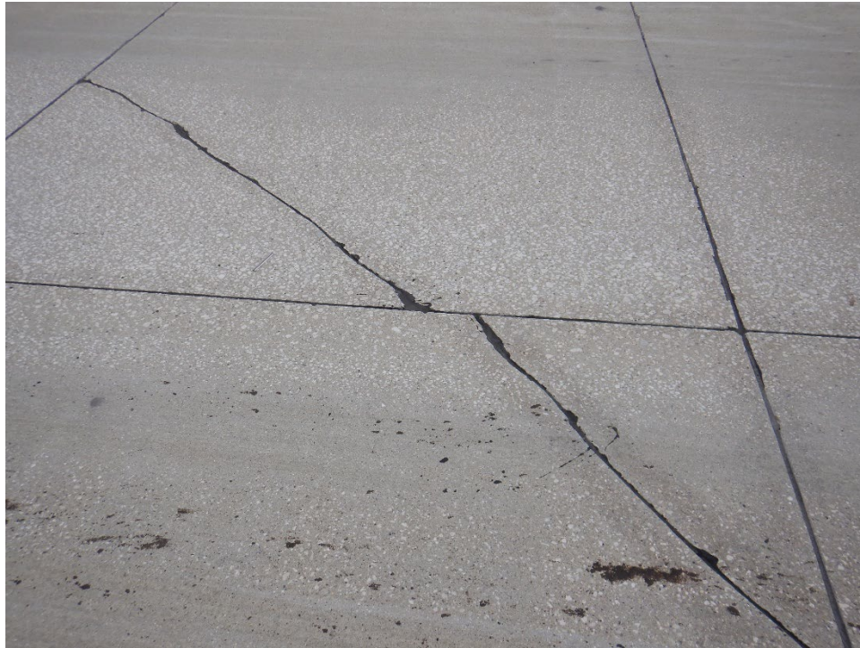
TFFD-02. LTD Cracking (Sample Unit No. 03).
