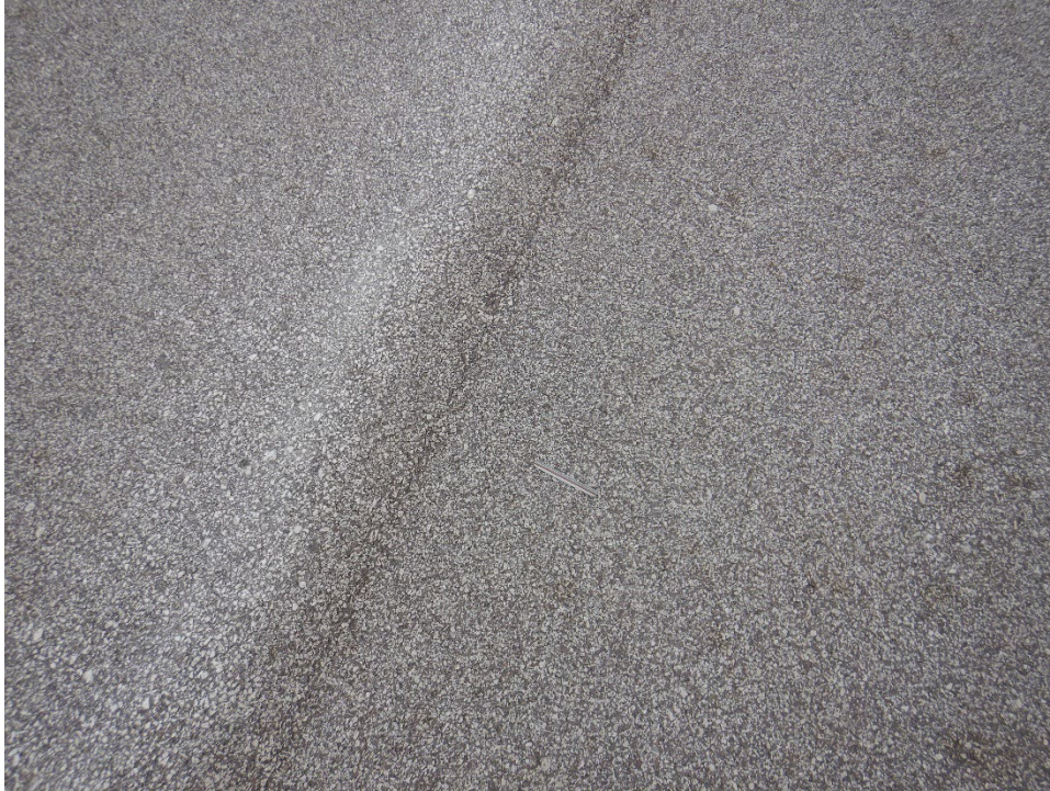
TBFD-03. Weathering (Sample Unit No. 17).
