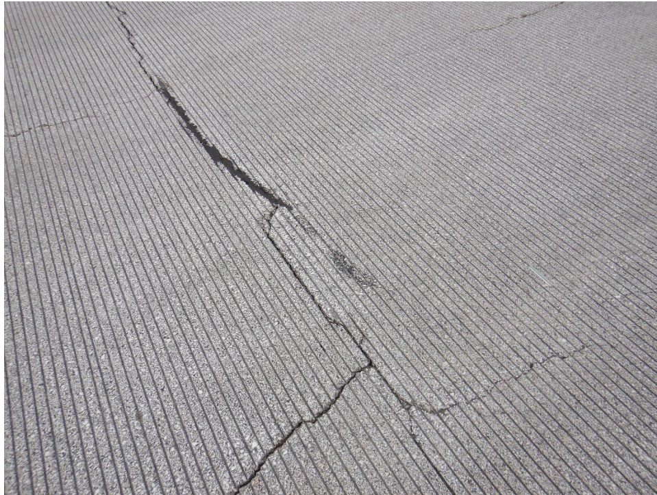
R12FD-01. L&T Cracking (Sample Unit No. 24).
