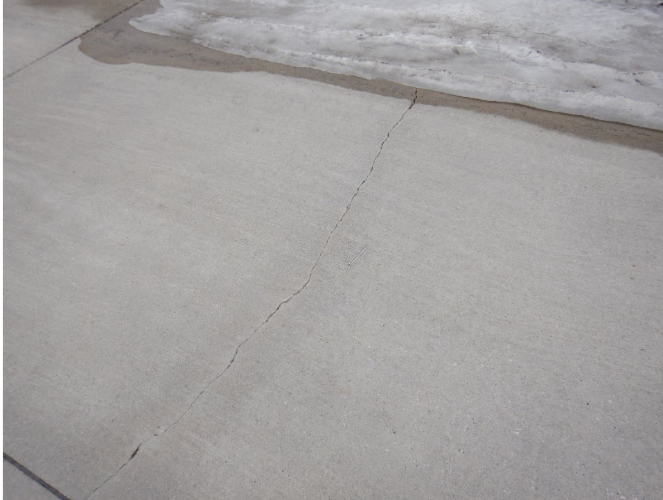
A02FD-01. LTD Cracking (Additional Sample Unit No. 14).
