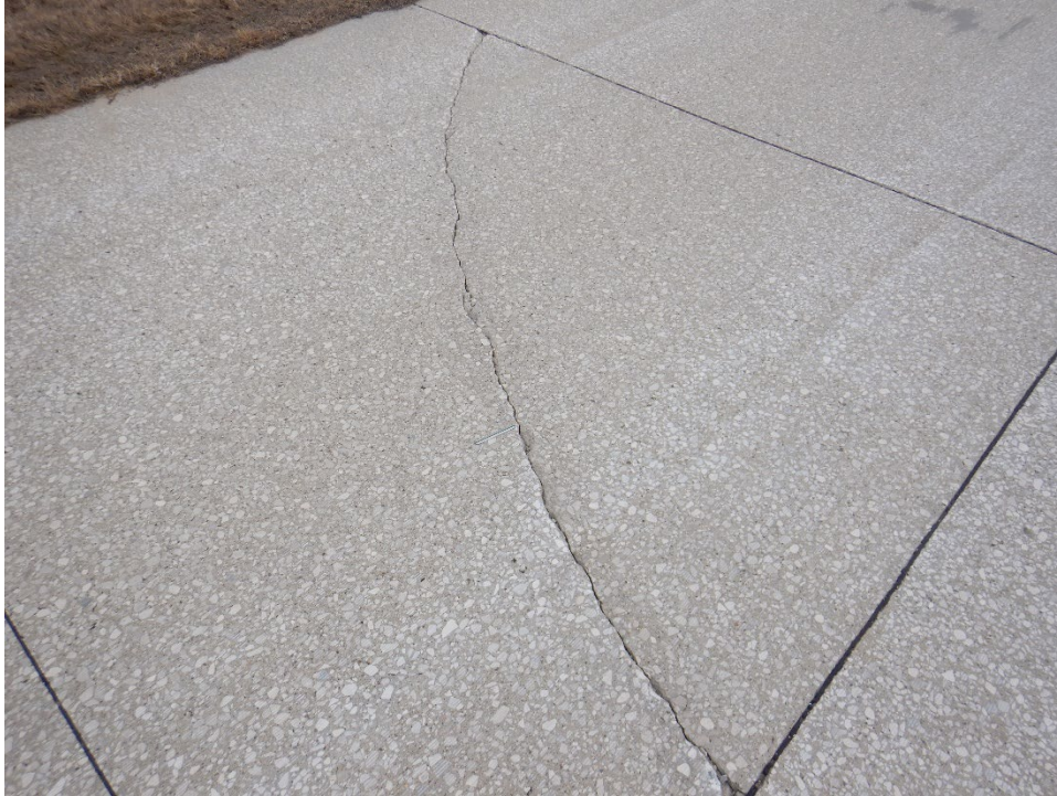
TAFD-01. LTD Cracking (Sample Unit No. 10).
