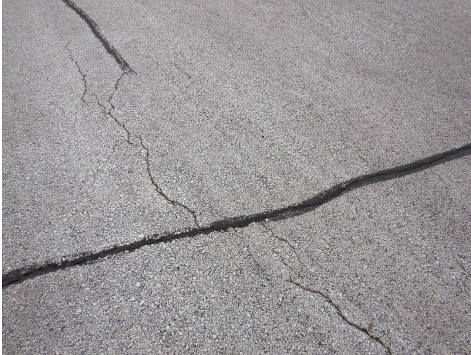
TBFD-04. L&T Cracking (Sample Unit No. 01).
