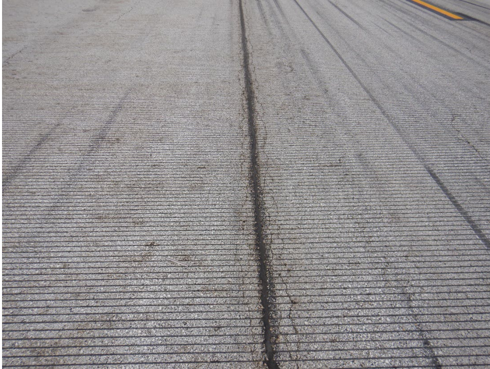
R06FD-02. Alligator Cracking (Sample Unit No. 13).
