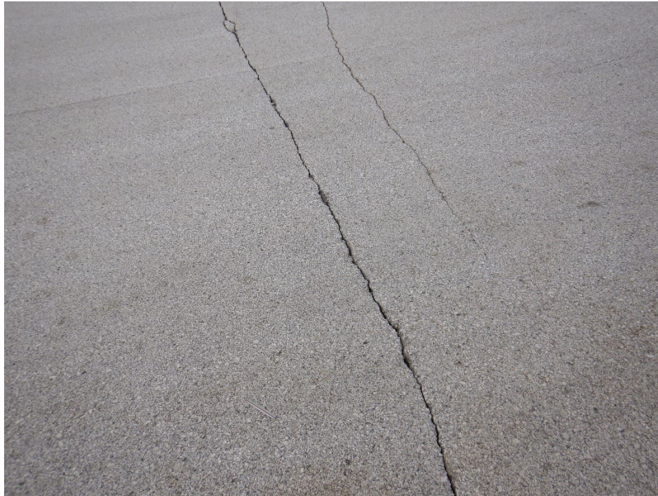
TBFD-01. L&T Cracking (Sample Unit No. 03).
