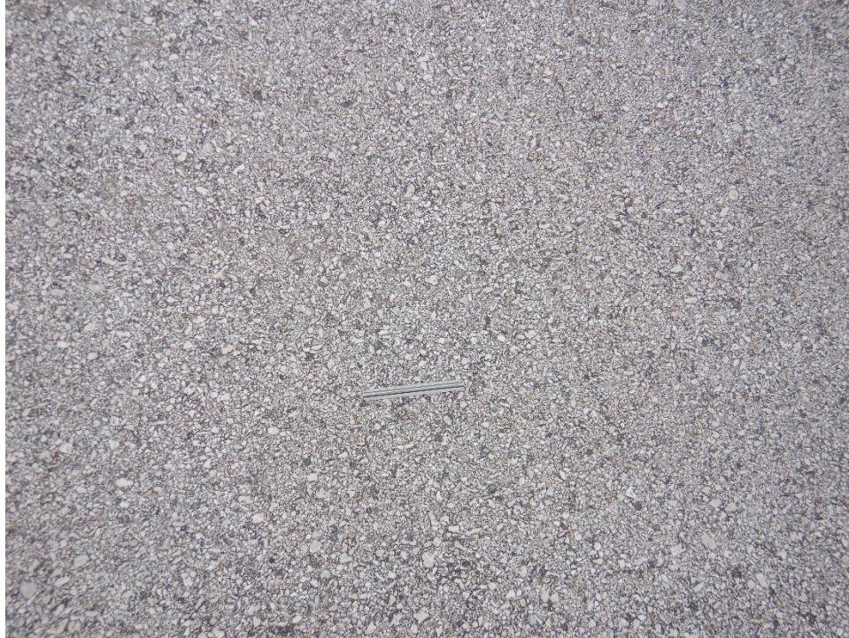
TBFD-05. Weathering (Sample Unit No. 01).
