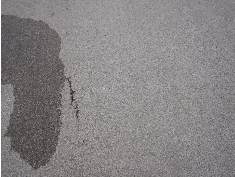
TBFD-06. L&T Cracking (Sample Unit No. 01).
