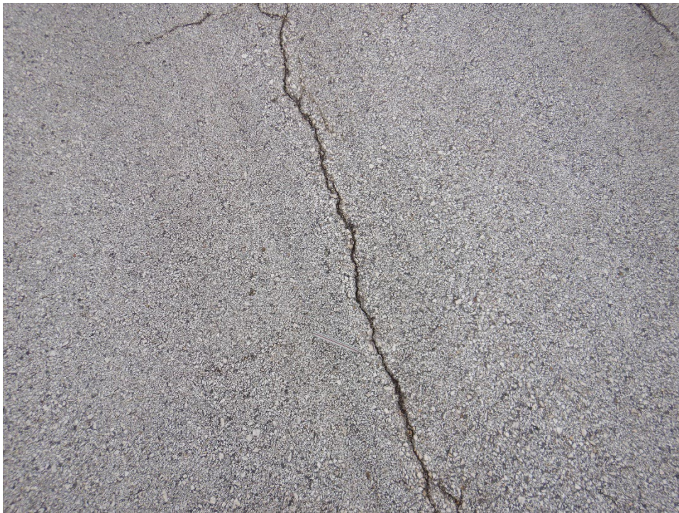
TDFD-02. L&T Cracking (Sample Unit No. 02).
