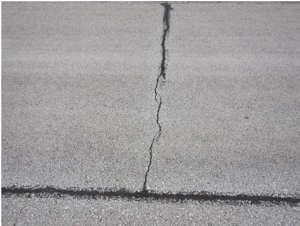
TBFD-02. L&T Cracking (Sample Unit No. 30).
