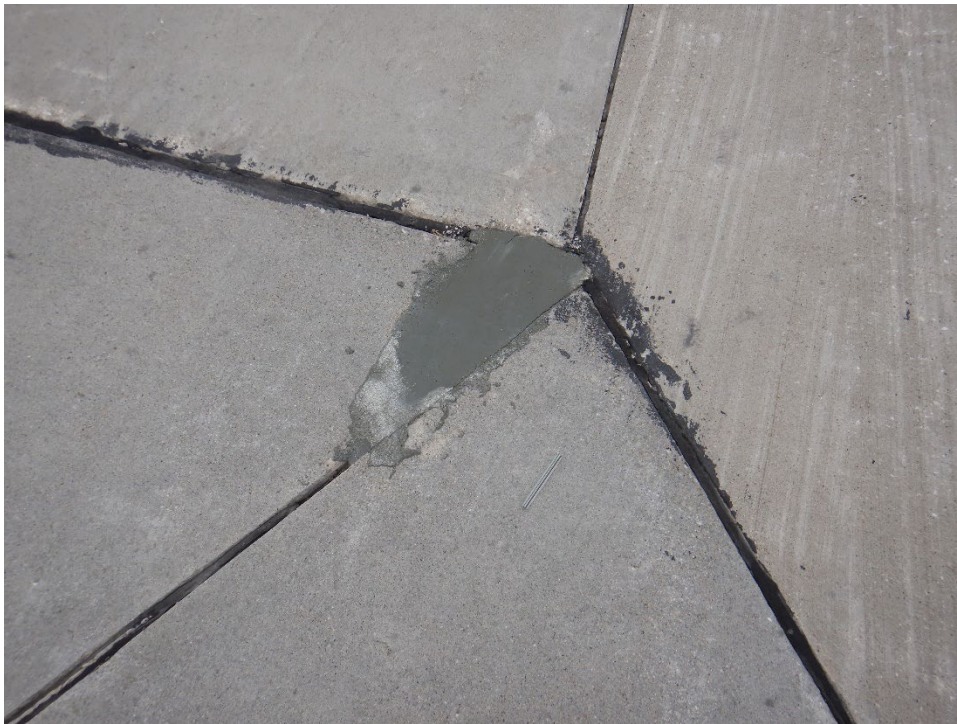
A01FD-02. Small Patching (Additional Sample Unit No. 15).
