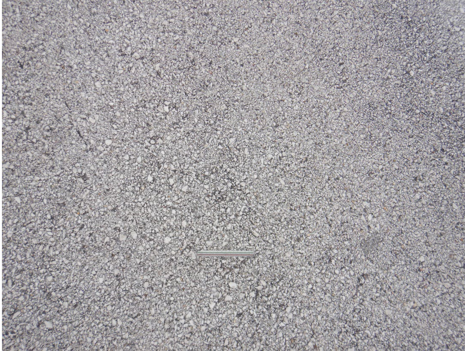
TBFD-02. Weathering (Sample Unit No. 30).
