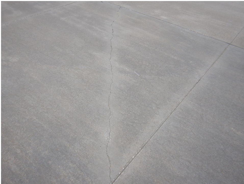
A02FD-02. LTD Cracking (Sample Unit No. 03).
