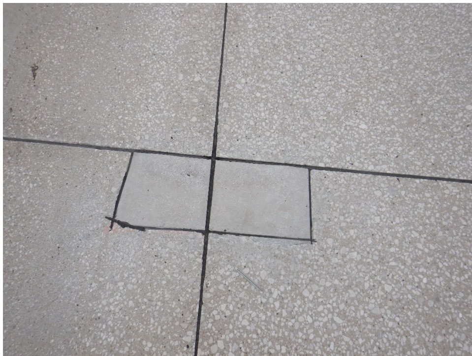
TFFD-02. Small Patching (Sample Unit No. 03).
