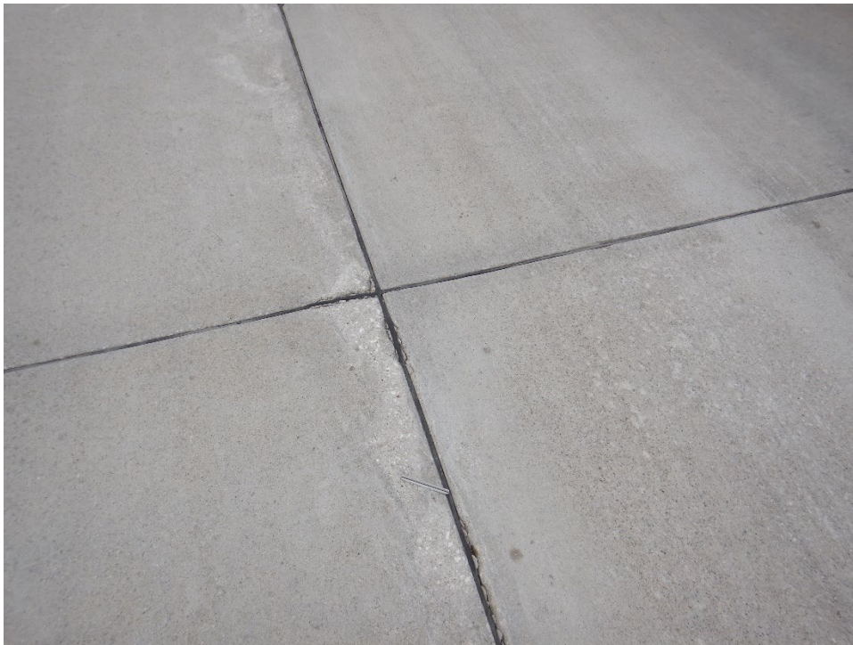
A01FD-01. Joint Seal Damage (Sample Unit No. 18).
