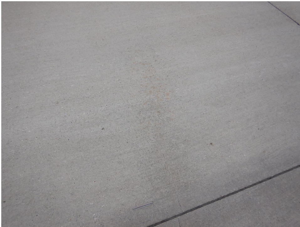
A02FD-01. Shrinkage Cracking (Additional Sample Unit No. 14).
