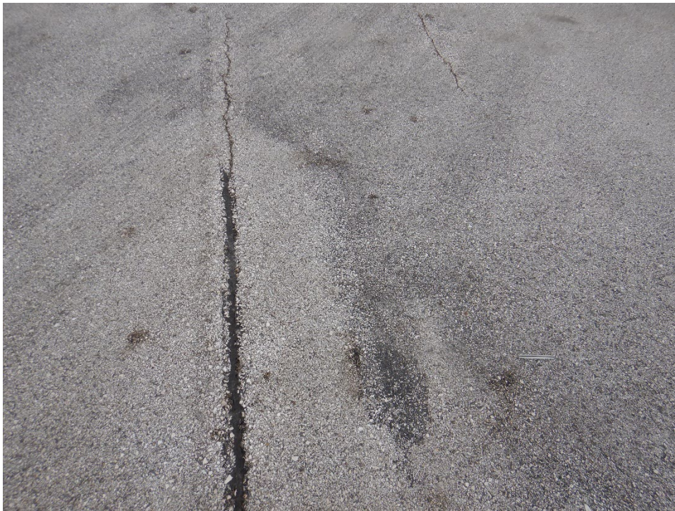
TBFD-05. L&T Cracking (Sample Unit No. 01).
