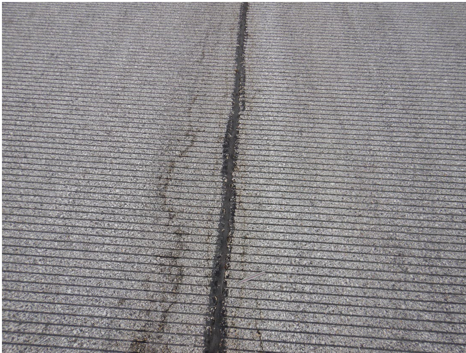
R06FD-02. L&T Cracking (Sample Unit No. 18).
