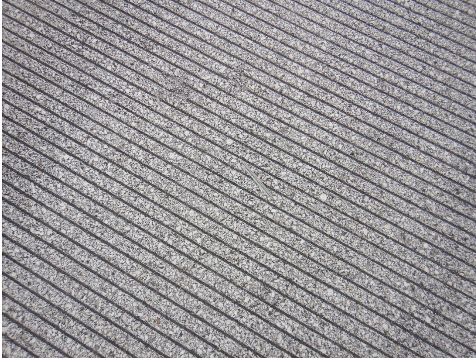
R06FD-02. Weathering (Sample Unit No. 18).
