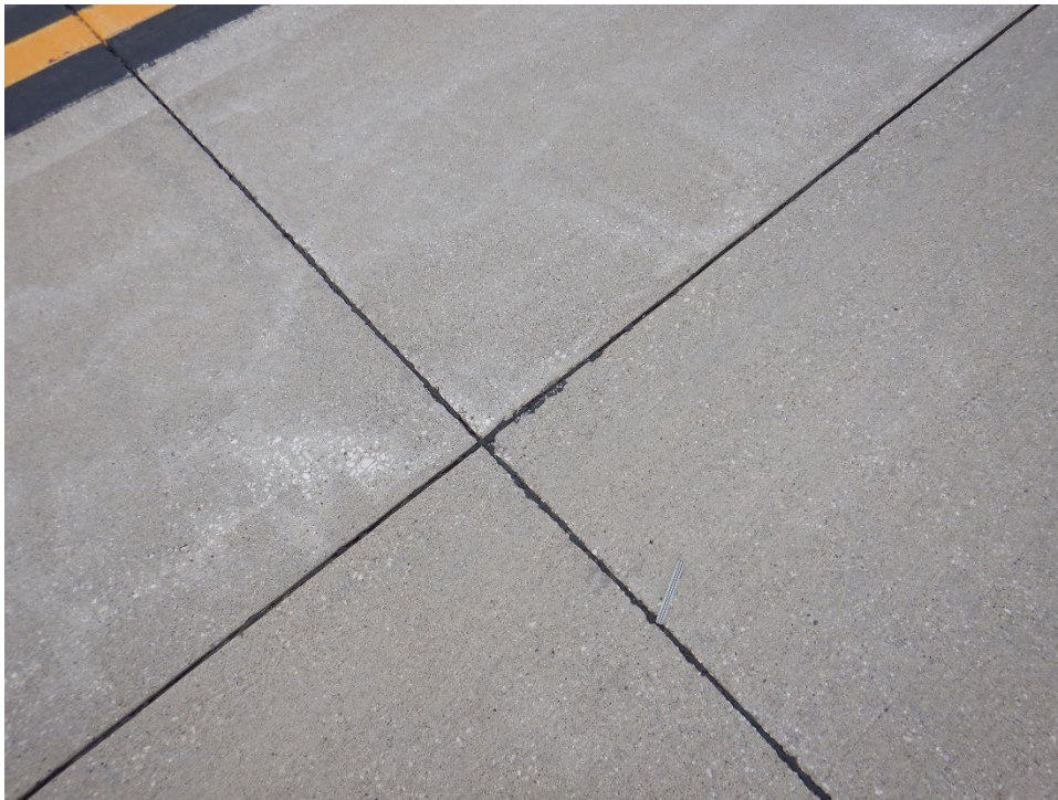
TCFD-01. Joint Seal Damage (Sample Unit No. 02).
