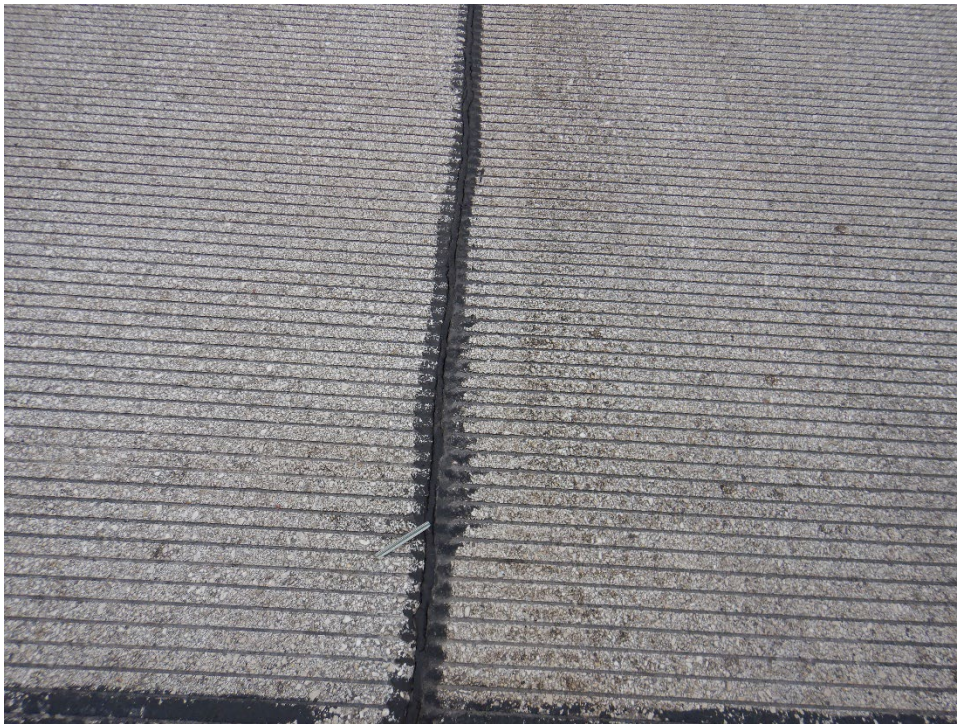
R06FD-01. L&T Cracking (Sample Unit No. 05).
