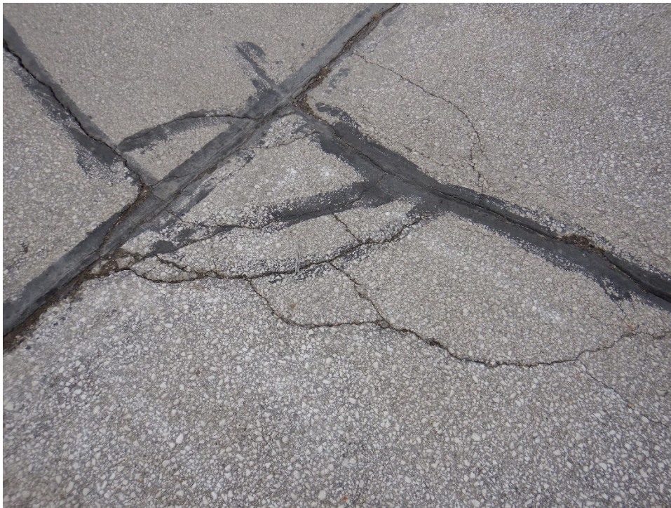
TH01FD-01. Alligator Cracking (Sample Unit No. 07).
