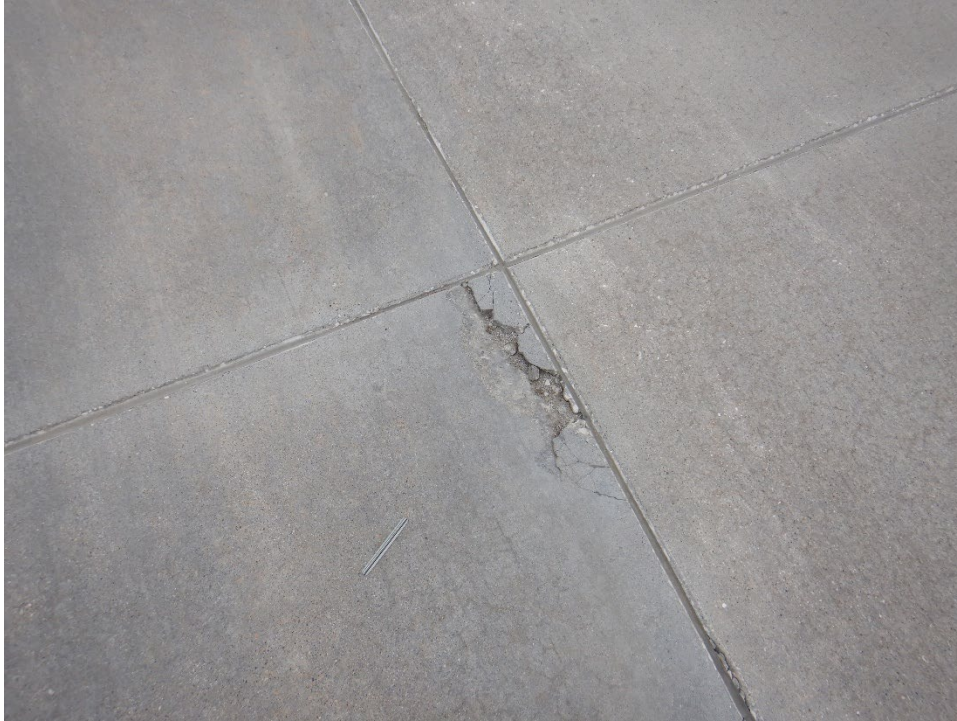
A02FD-02. Joint Spalling (Sample Unit No. 04).
