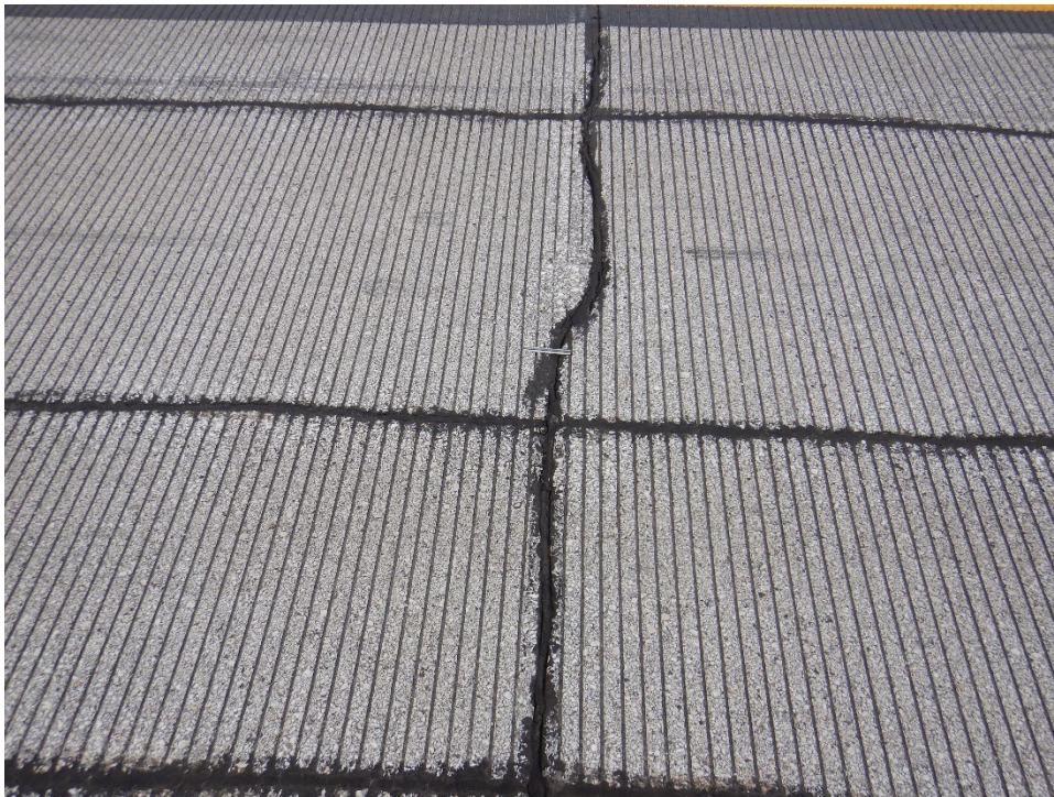
R12FD-02. L&T Cracking (Sample Unit No. 53).
