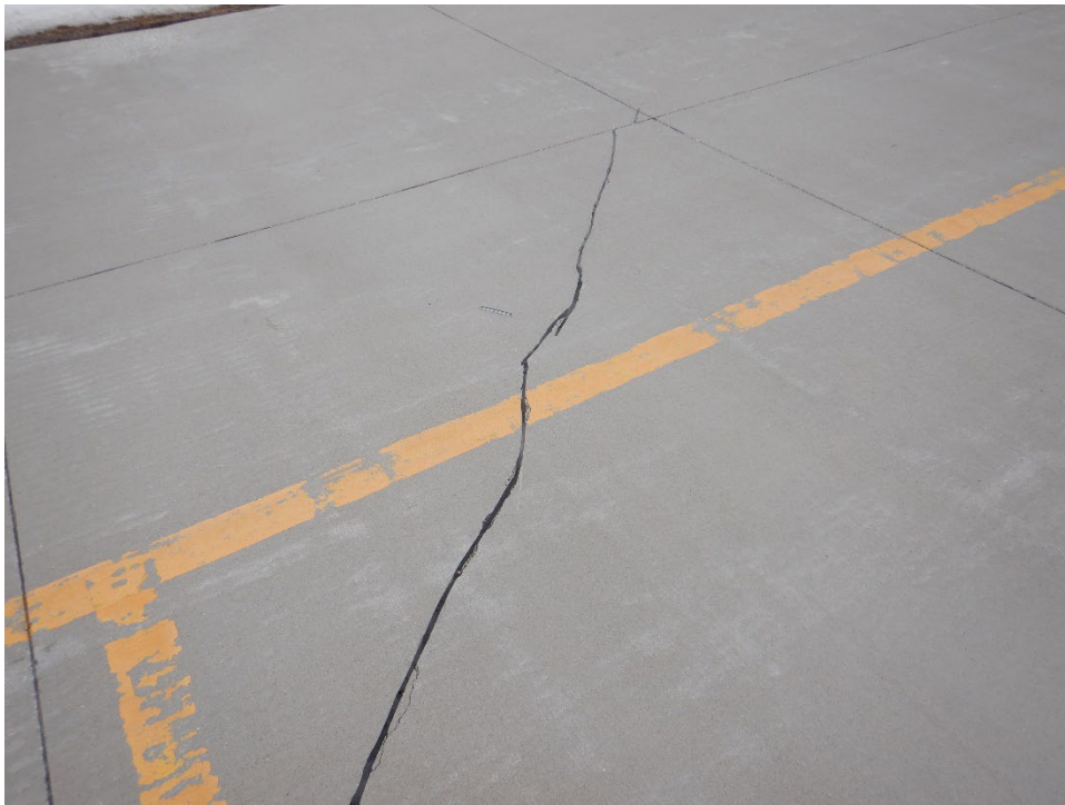
TH01FD-03. LTD Cracking (Sample Unit No. 08).
