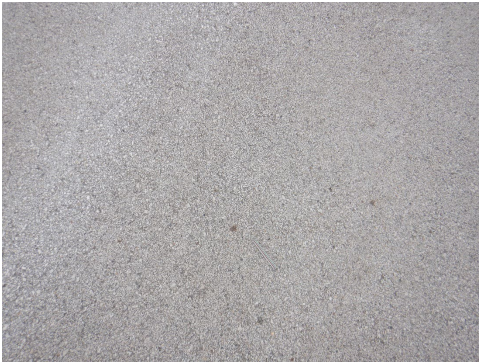
TBFD-06. Weathering (Sample Unit No. 01).
