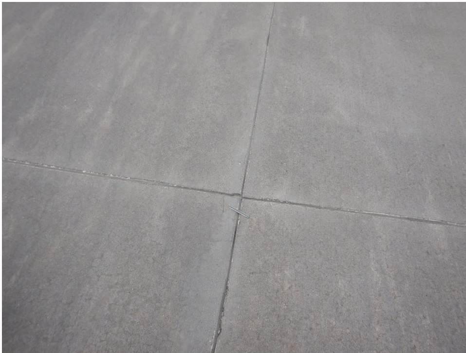
A02FD-02. Joint Seal Damage (Sample Unit No. 04).
