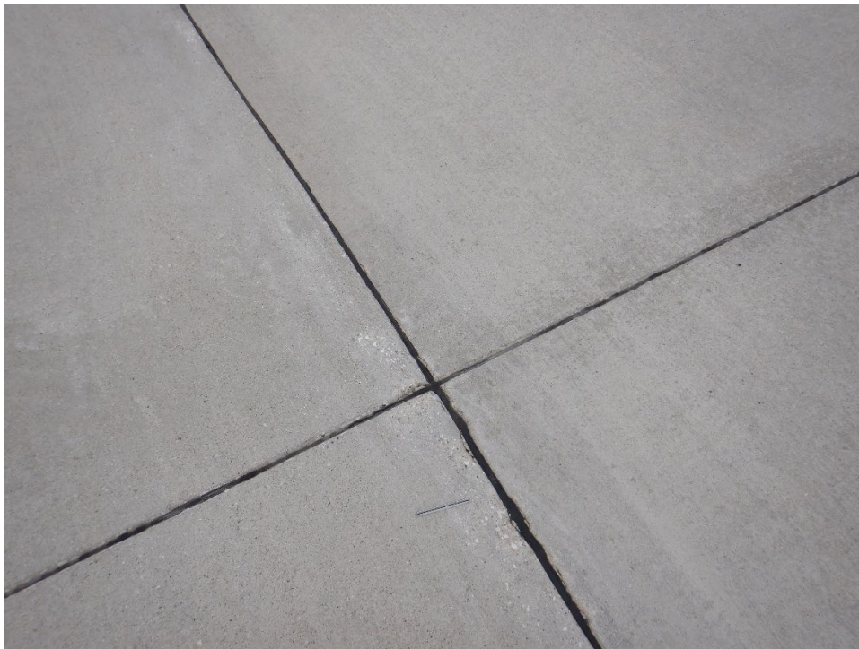
A02FD-01. Joint Seal Damage (Sample Unit No. 01).
