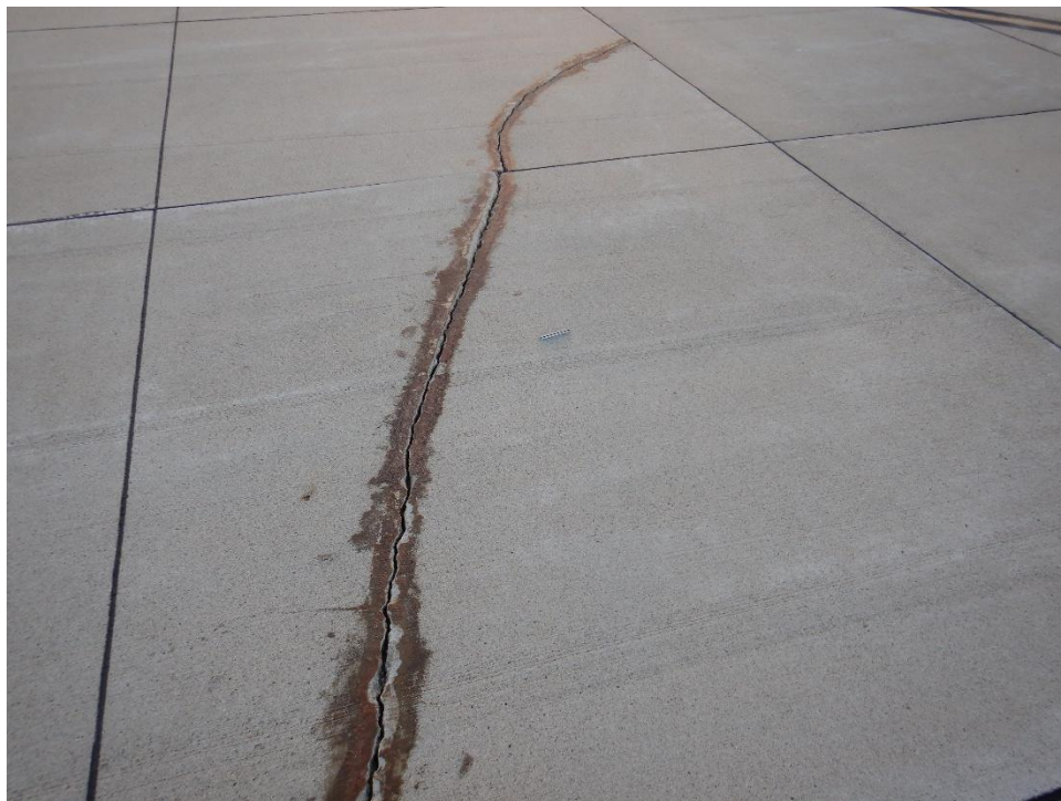
A01FC-02. LTD Cracking (Sample Unit No. 16).
