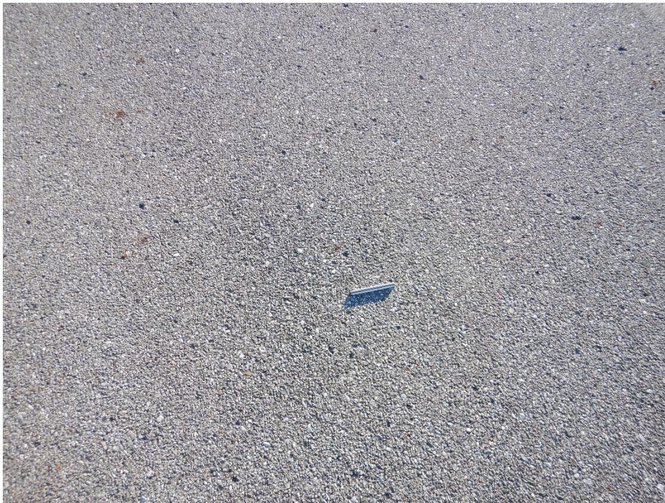
T02FC-03. Weathering and Raveling (Sample Unit No. 01).
