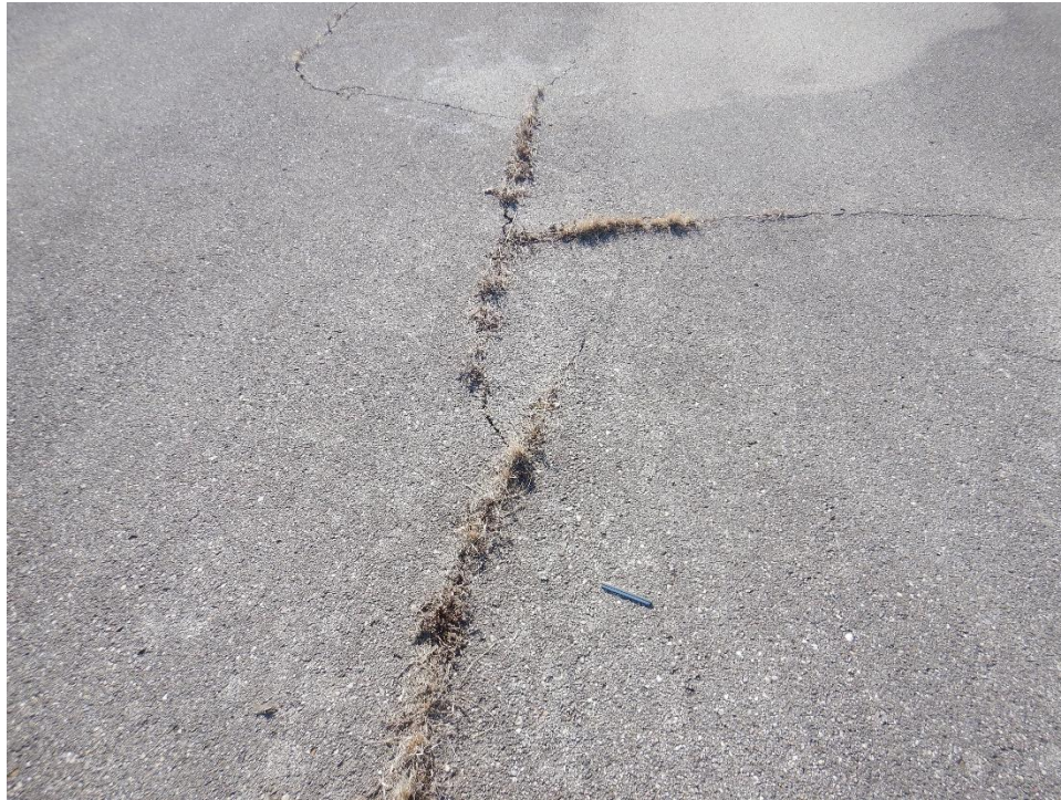
R15FC-03. L&T Cracking (Sample Unit No. 01).
