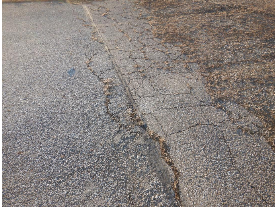
TH01FC-03. Alligator Cracking (Sample Unit No. 01).
