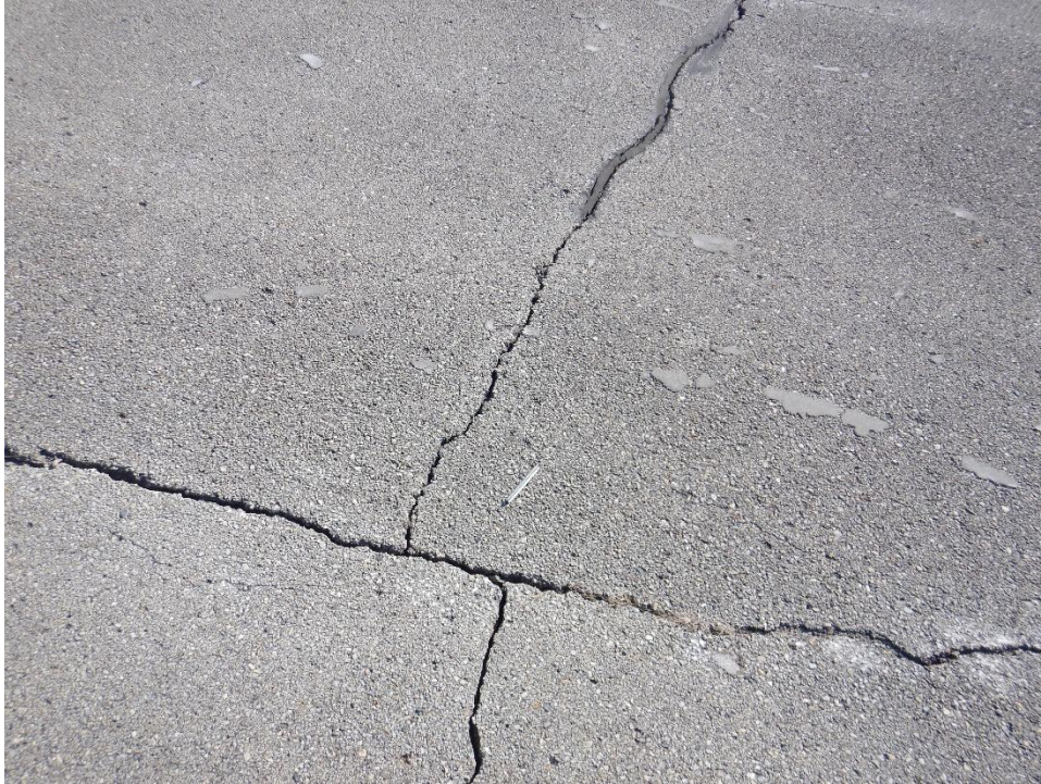
R09FC-04. L&T Cracking (Sample Unit No. 04).
