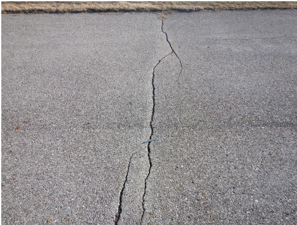
T01FC-02. L&T Cracking (Sample Unit No. 01).
