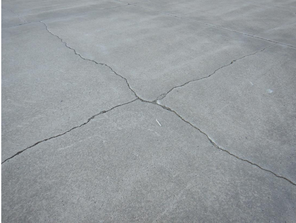
TH01FC-02. Shattered Slab (Sample Unit No. 01).
