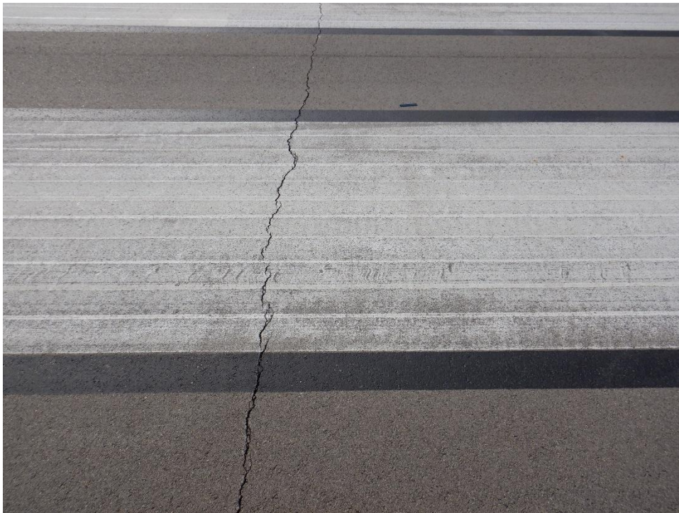
R15FC-02. L&T Cracking (Sample Unit No. 047) (1).
