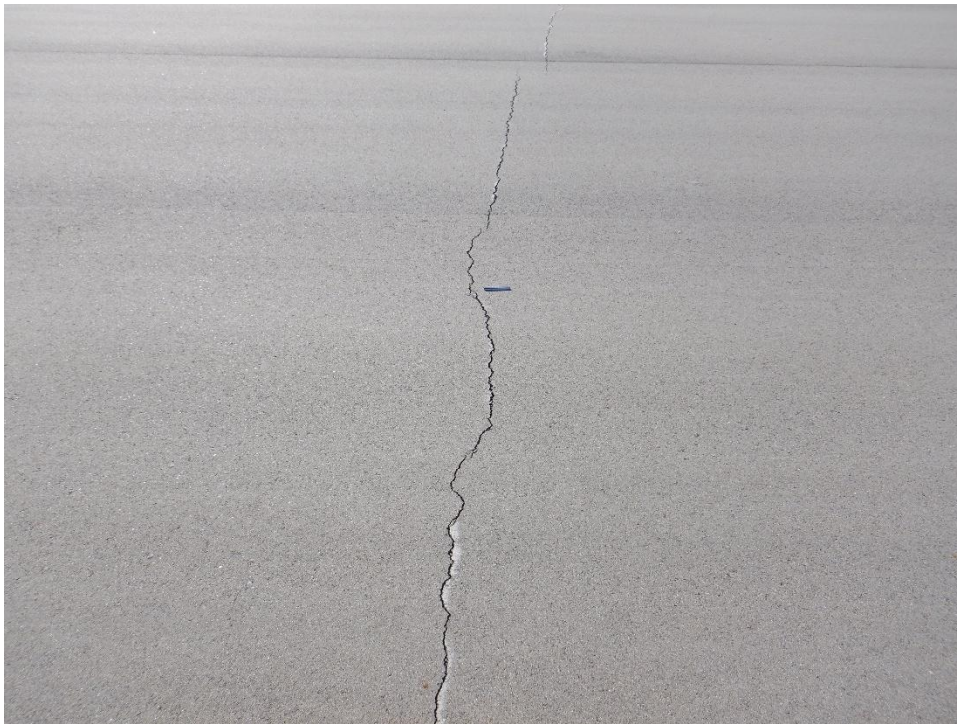
R15FC-01. L&T Cracking (Sample Unit No. 23).
