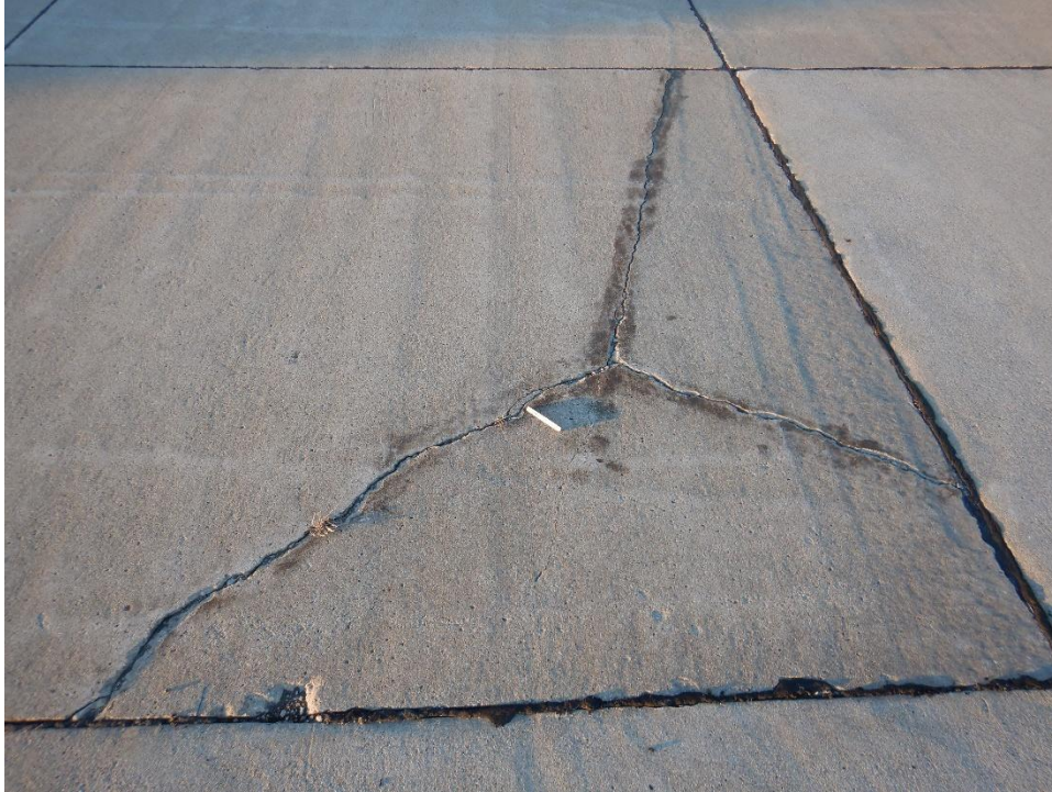
A01FC-01. LTD Cracking (Sample Unit No. 10).
