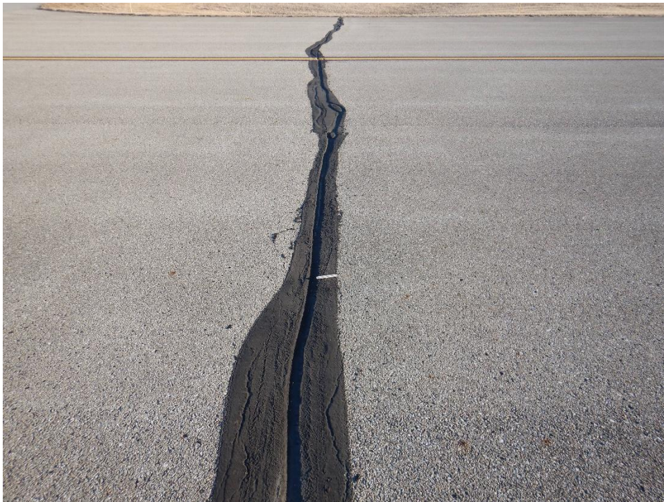
T02FC-02. L&T Cracking (Sample Unit No. 01).
