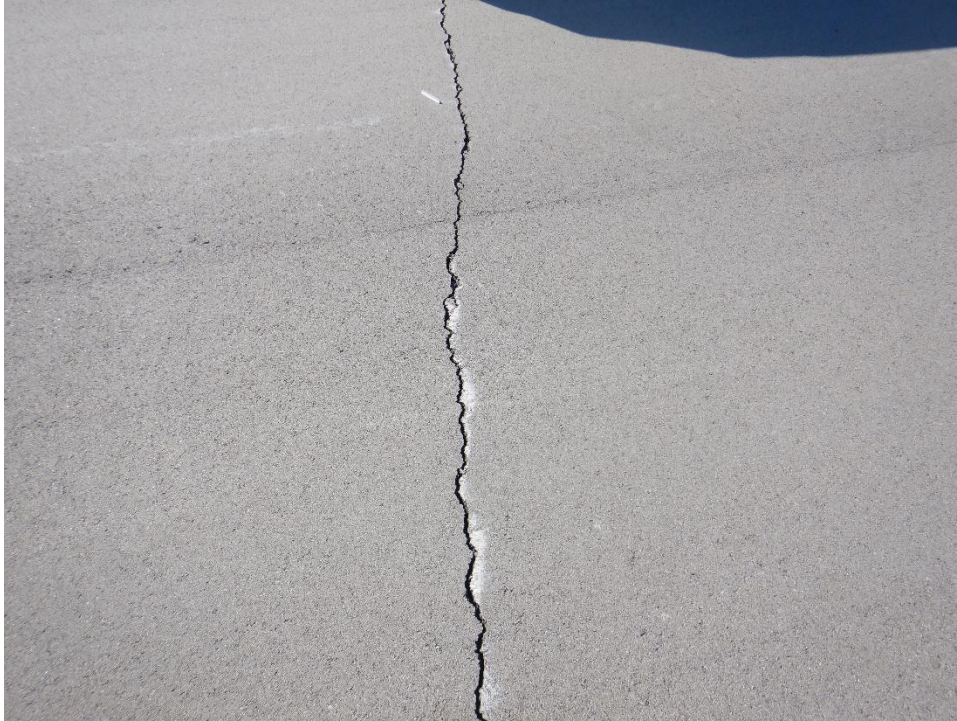
R15FC-02. L&T Cracking (Sample Unit No. 047) (2).
