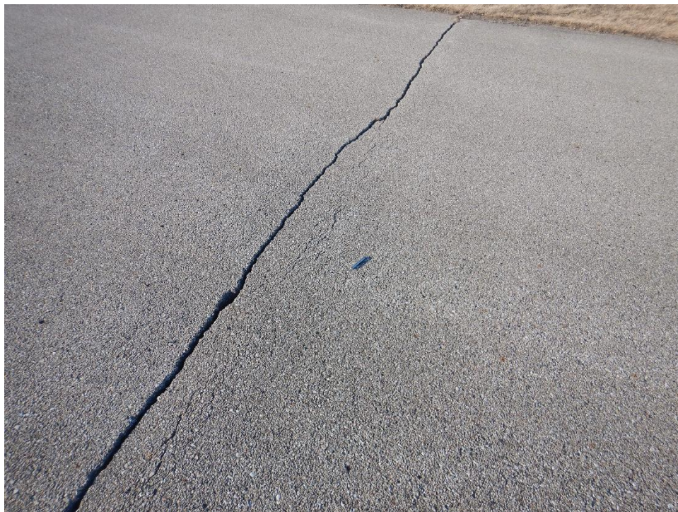
T01FC-01. L&T Cracking (Sample Unit No. 01).
