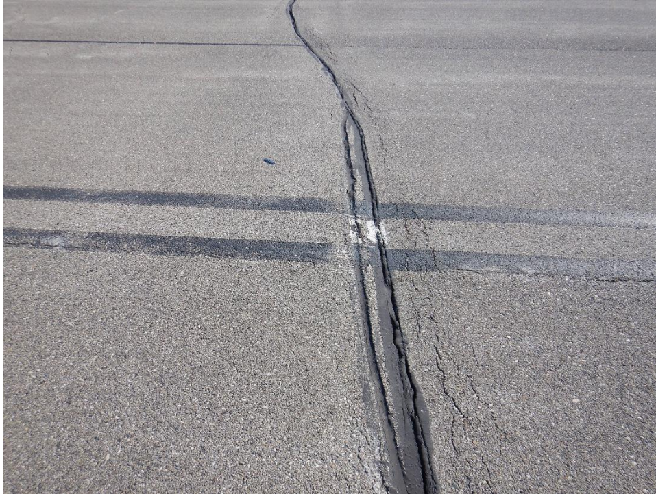
R09FC-02. L&T Cracking (Sample Unit No. 08).
