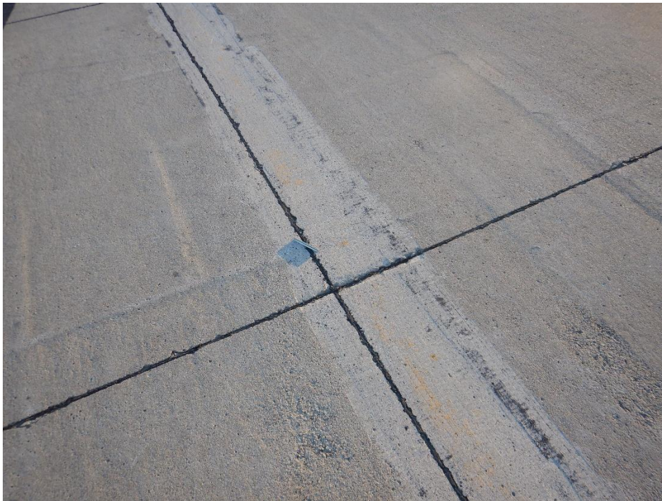
TH01FC-01. Joint Seal Damage (Sample Unit No. 01).
