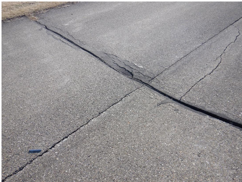
R09FC-01. L&T Cracking (Sample Unit No. 11).
