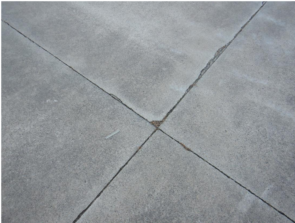
TH01FC-02. Joint Seal Damage (Sample Unit No. 01).
