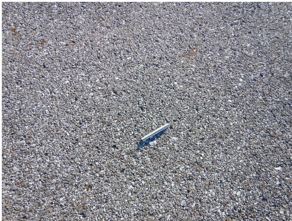
T01FC-02. Weathering and Raveling (Sample Unit No. 01).
