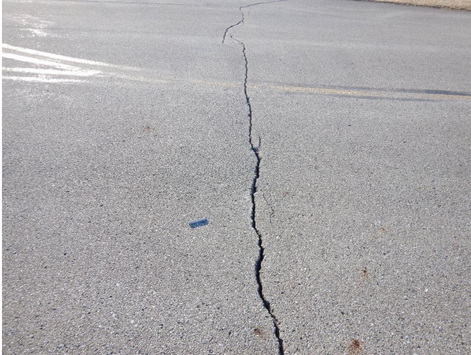
T02FC-03. L&T Cracking (Sample Unit No. 01).
