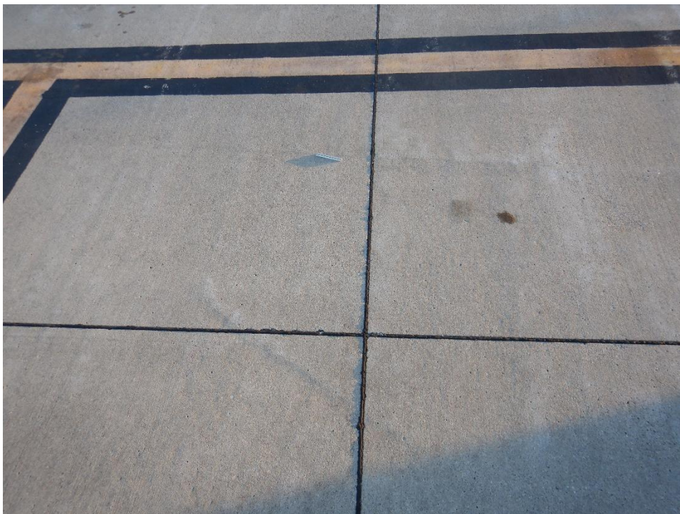
A01FC-01. Joint Seal Damage (Sample Unit No. 01).
