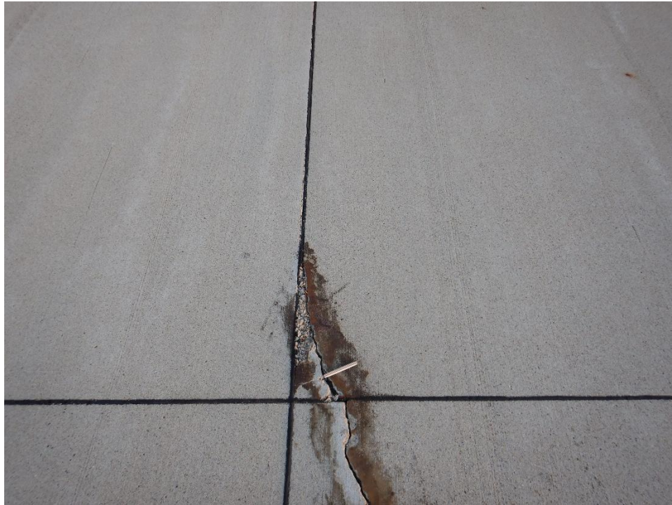
A01FC-02. Joint Spalling (Sample Unit No. 16).
