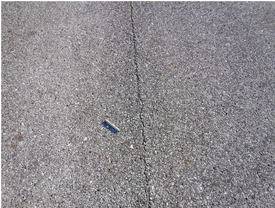
T02FC-01. L&T Cracking (Sample Unit No. 02).
