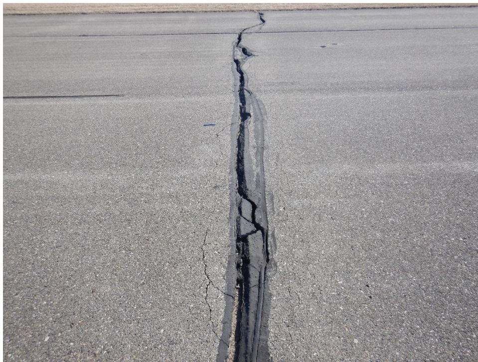
R09FC-03. L&T Cracking (Sample Unit No. 03).
