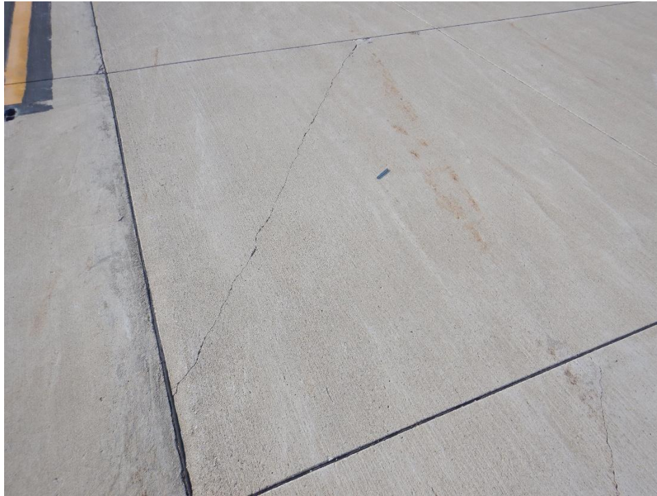
A01ES-01. LTD Cracking (Sample Unit No. 12).
