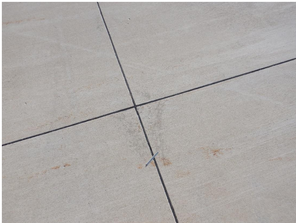
A01ES-01. Joint Seal Damage (Sample Unit No. 12).
