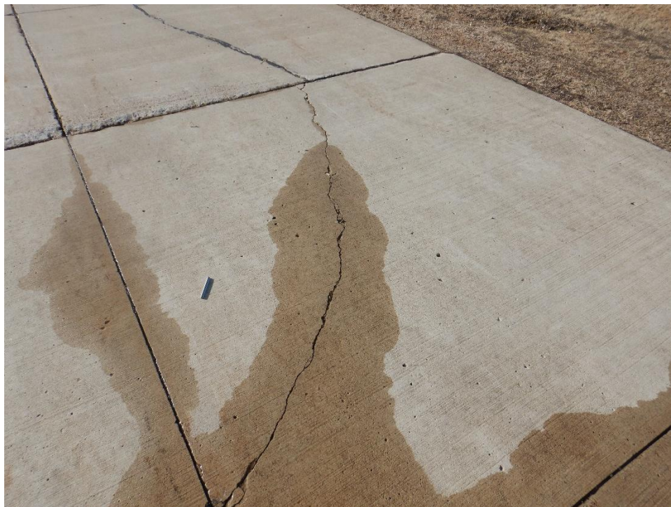
TH01ES-01. LTD Cracking (Sample Unit No. 05).
