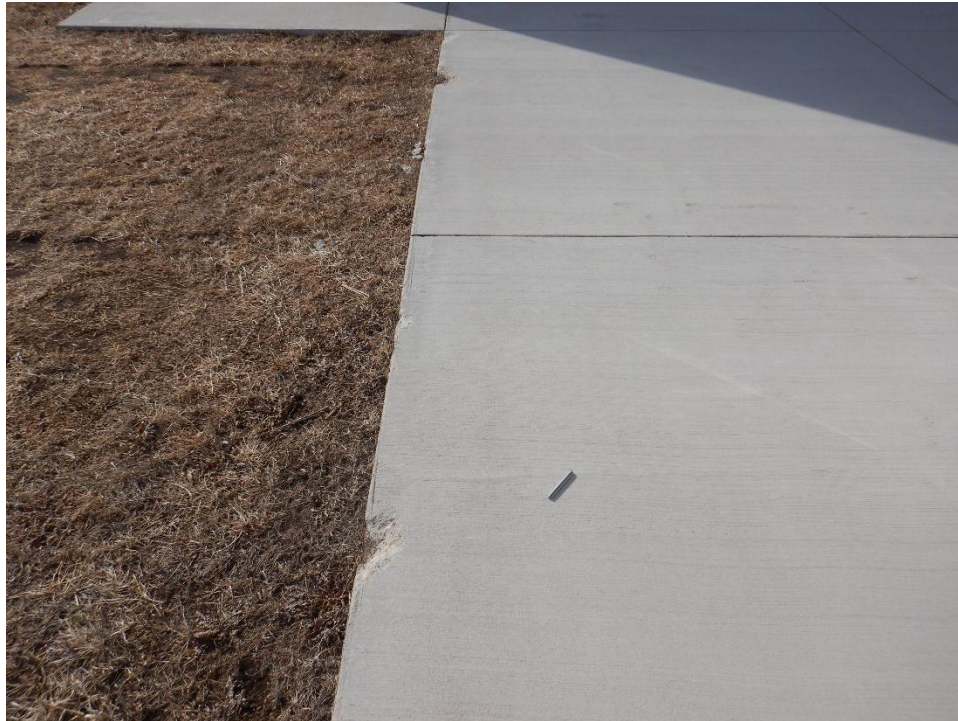
A01ES-03. Joint Spalling (Sample Unit No. 03).
