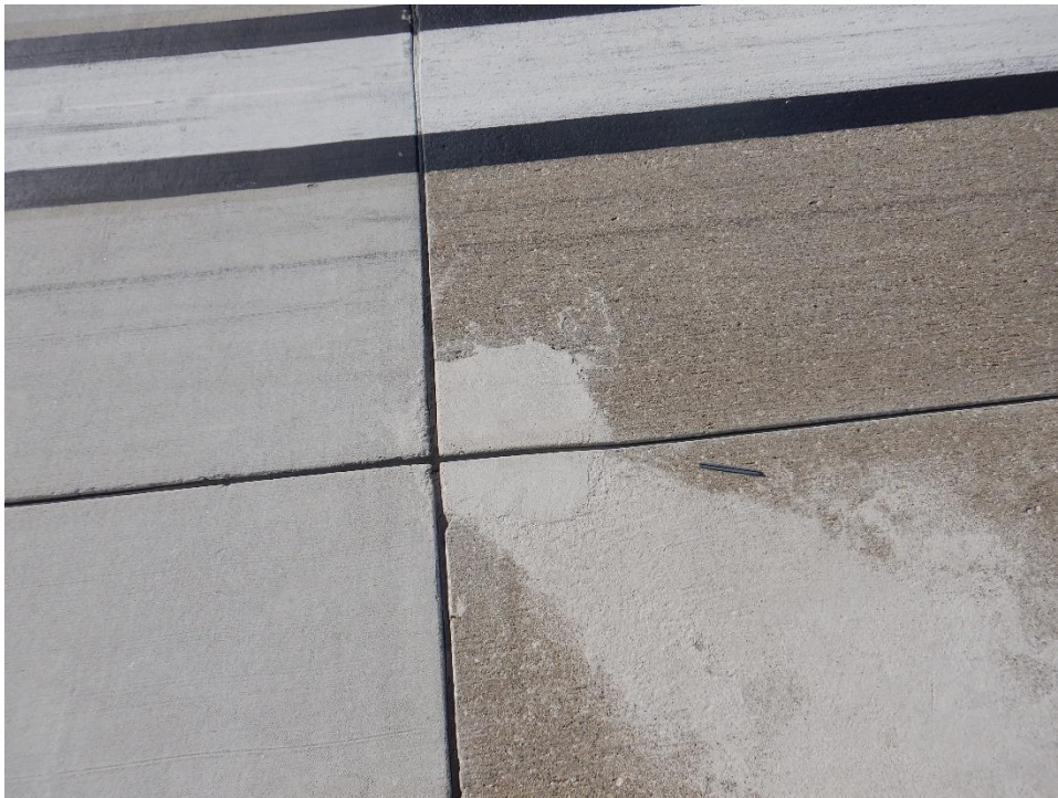
R16ES-01. Small Patching (Sample Unit No. 150).
