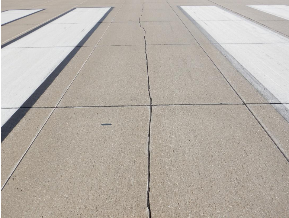
R16ES-01. LTD Cracking (Sample Unit No. 160).
