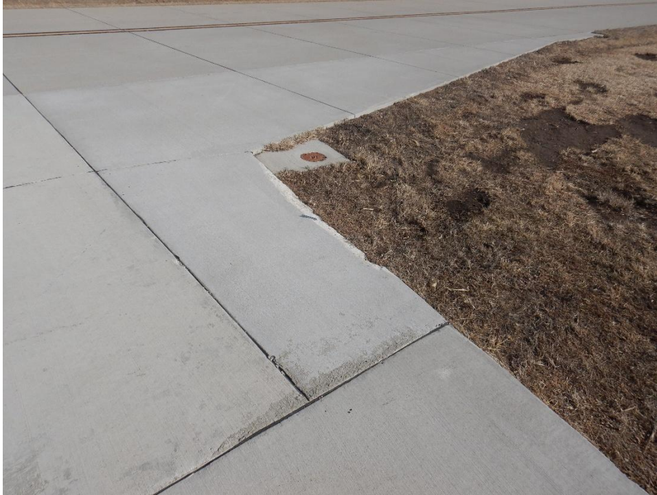
A01ES-02. Joint Spalling (Sample Unit No. 05).
