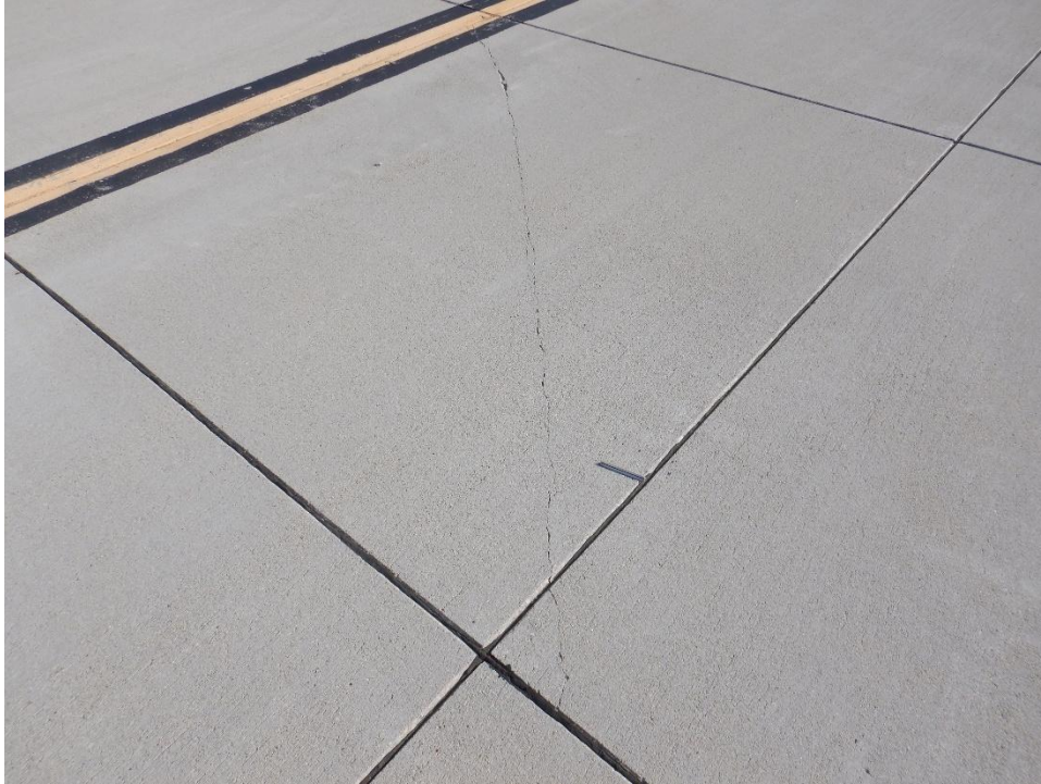
T01ES-02. LTD Cracking (Sample Unit No. 17).
