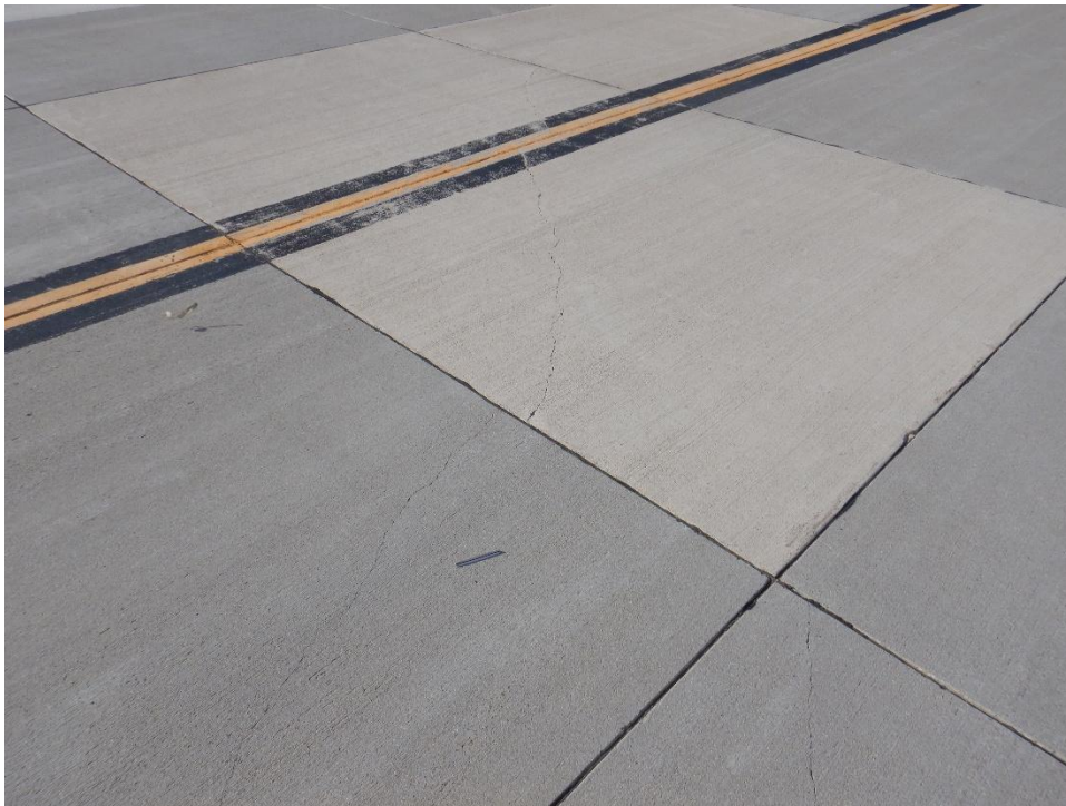
T01ES-02. LTD Cracking (Sample Unit No. 05).
