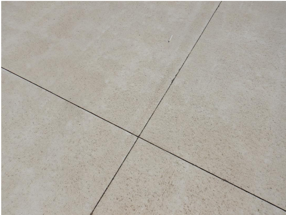
A01EM-02. Joint Seal Damage (Sample Unit No. 03).
