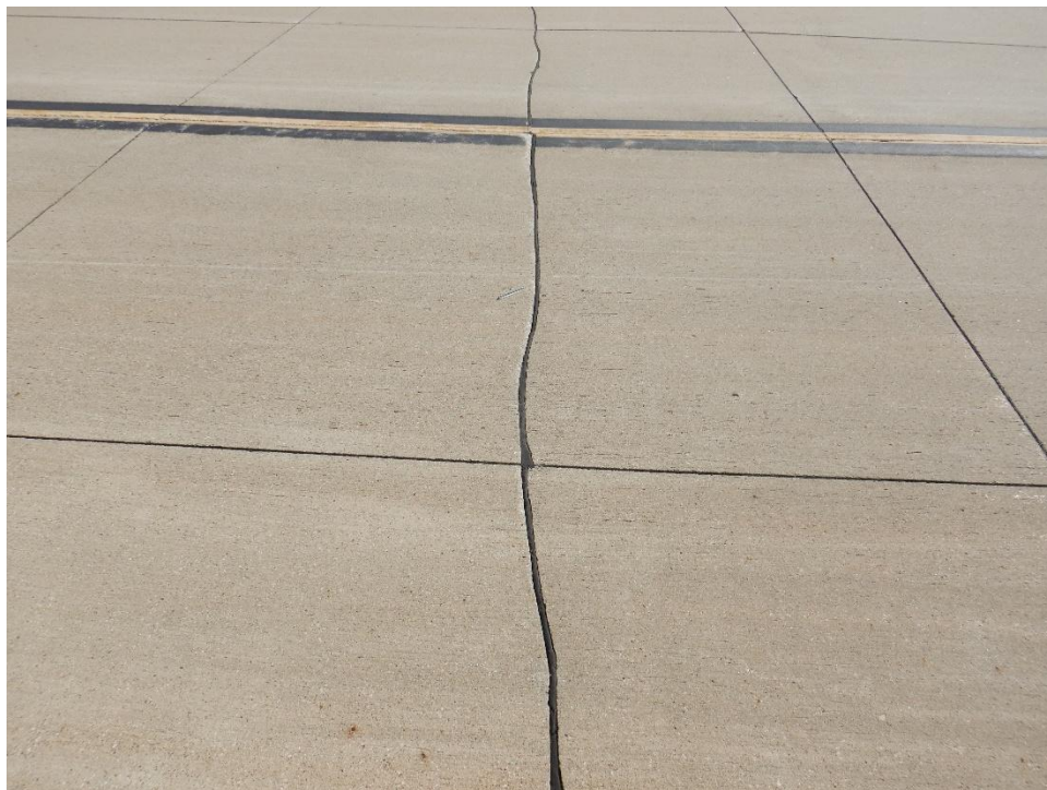
T01EM-01. LTD Cracking (Sample Unit No. 02).
