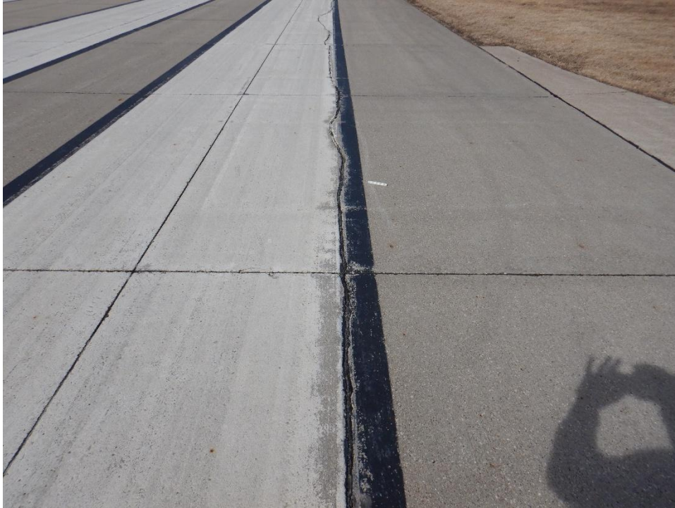
R13EM-01. LTD Cracking (Sample Unit No. 03).
