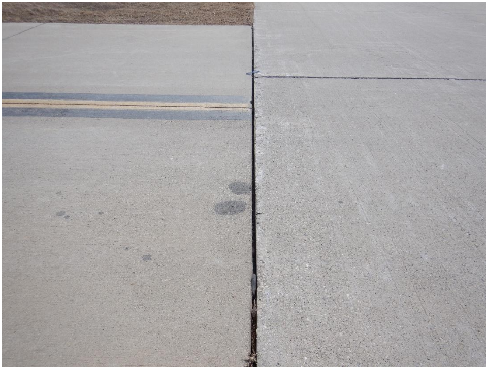
TH01EM-01. Faulting (Sample Unit No. 01).
