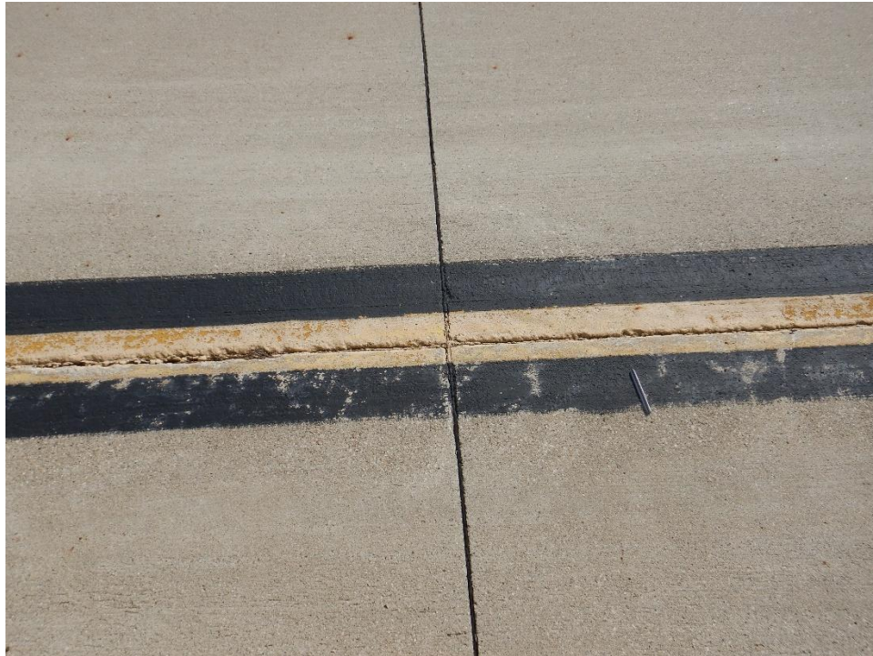
T01EM-01. Joint Seal Damage (Sample Unit No. 02).
