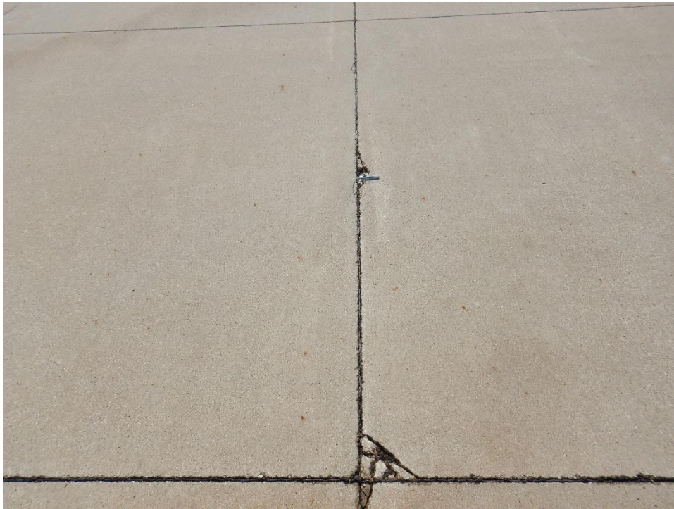
A01EM-01. Corner Spalling (Sample Unit No. 16).
