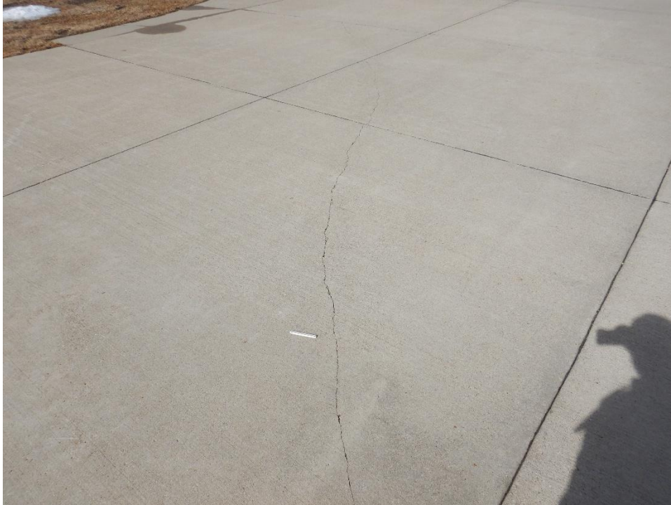
A01EM-01. LTD Cracking (Sample Unit No. 21).
