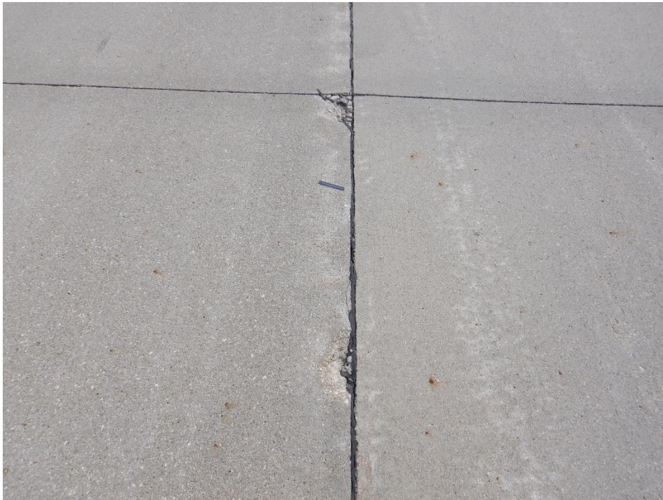
R13EM-01. Joint and Corner Spalling (Sample Unit No. 72).
