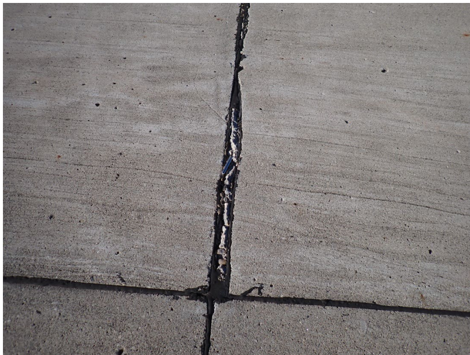
R13EG-01. Joint Spalling (Sample Unit No. 07).
