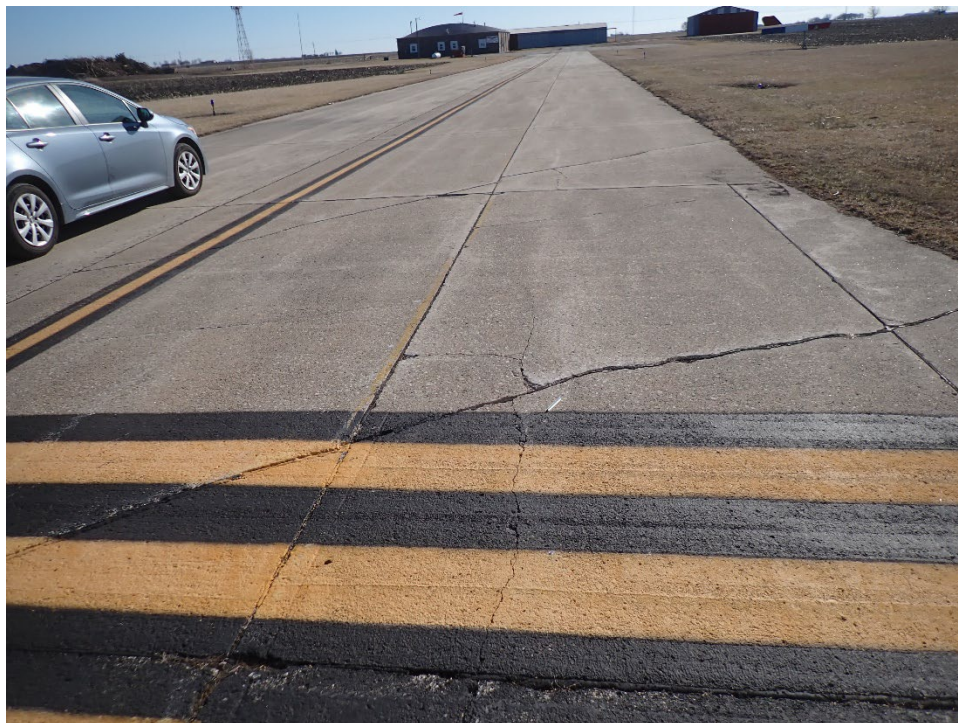
T01EG-01. Shattered Slab (Sample Unit No. 02).
