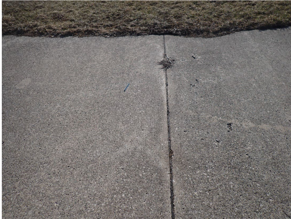
T01EG-02. Joint Seal Damage (Sample Unit No. 04).
