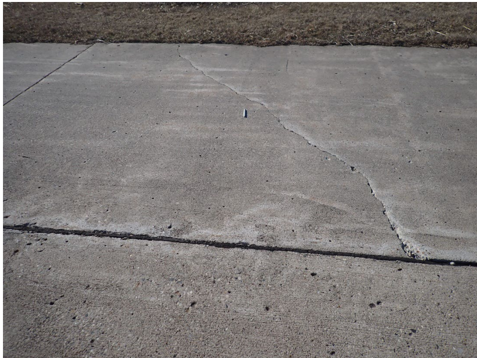
T01EG-02. LTD Cracking (Sample Unit No. 02).
