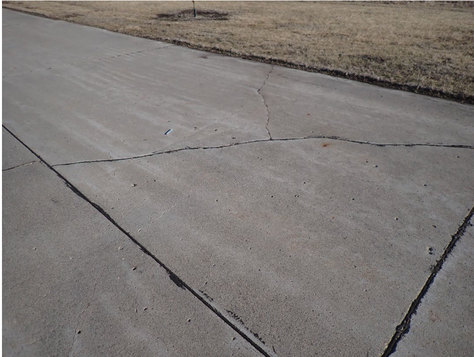
R13EG-01. Shattered Slab (Sample Unit No. 07).
