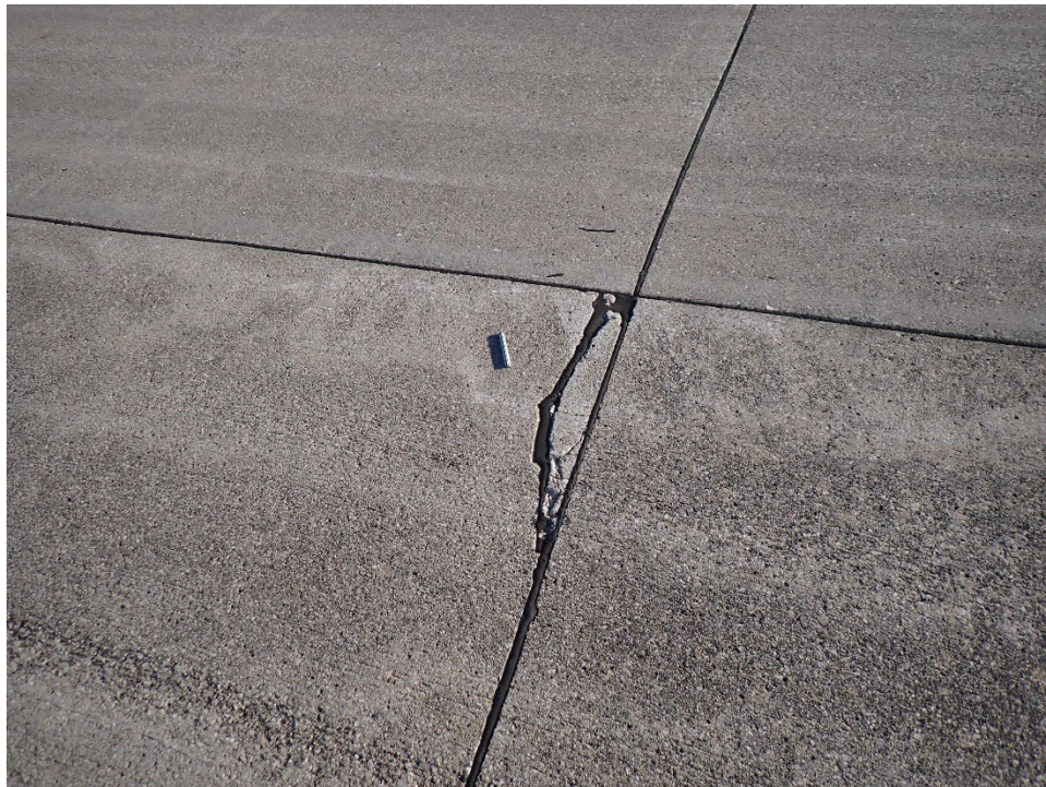
R13EG-02. Joint Spalling (Sample Unit No. 34).
