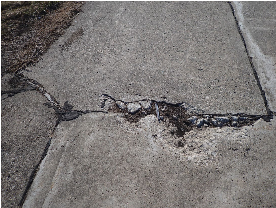
T01EG-01. Joint Spalling (Sample Unit No. 01) (1).
