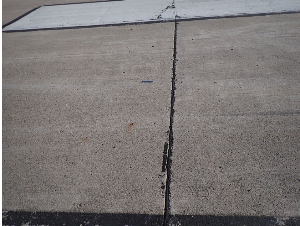
R13EG-01. Joint Seal Damage (Sample Unit No. 05).
