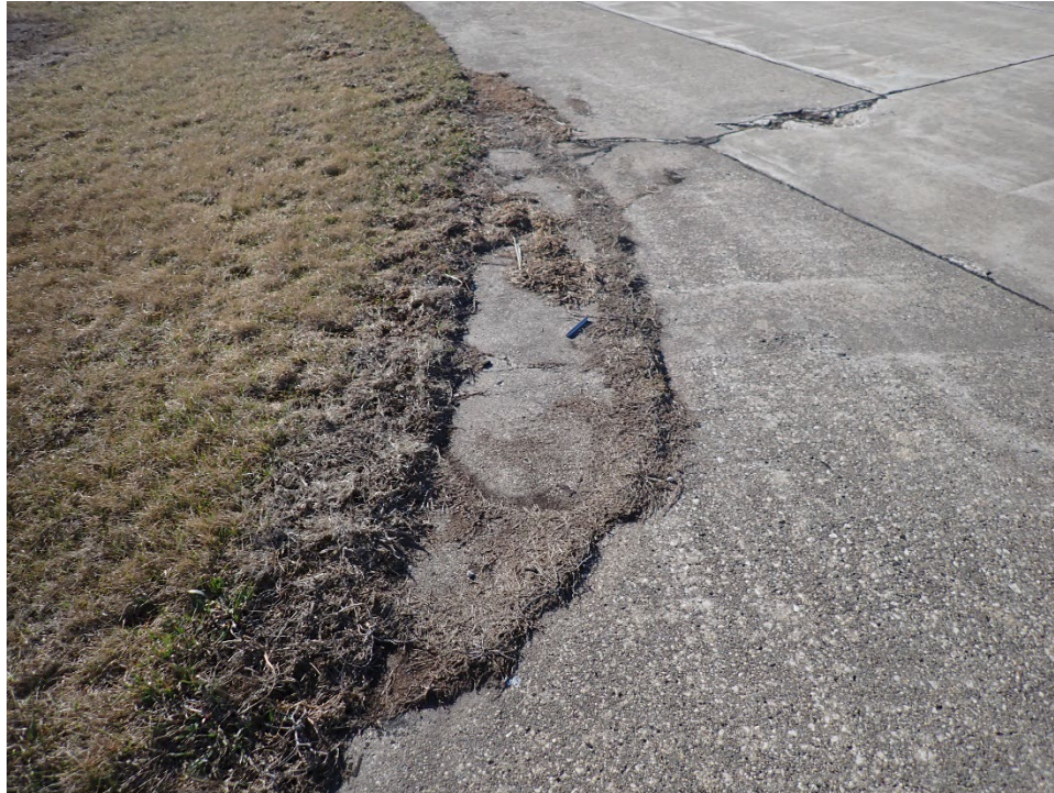
T01EG-01. Joint Spalling (Sample Unit No. 01) (2).
