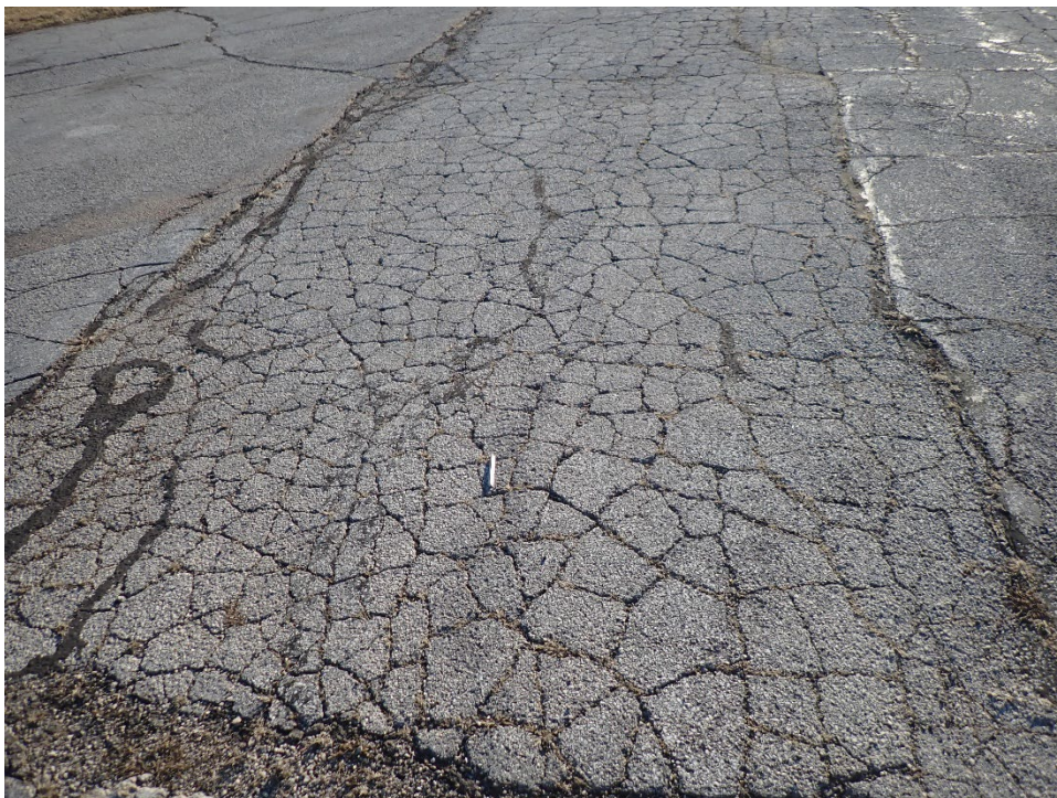
A01EG-01. Alligator Cracking (Sample Unit No. 02).
