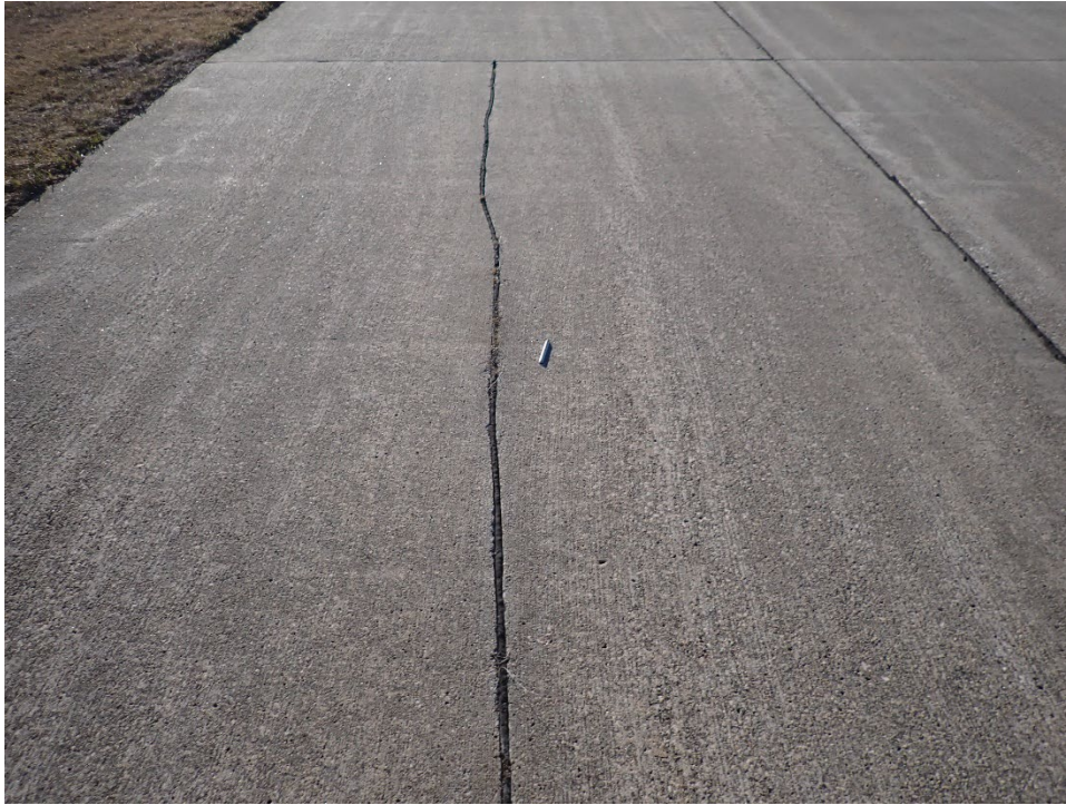
R13EG-02. LTD Cracking (Sample Unit No. 34).
