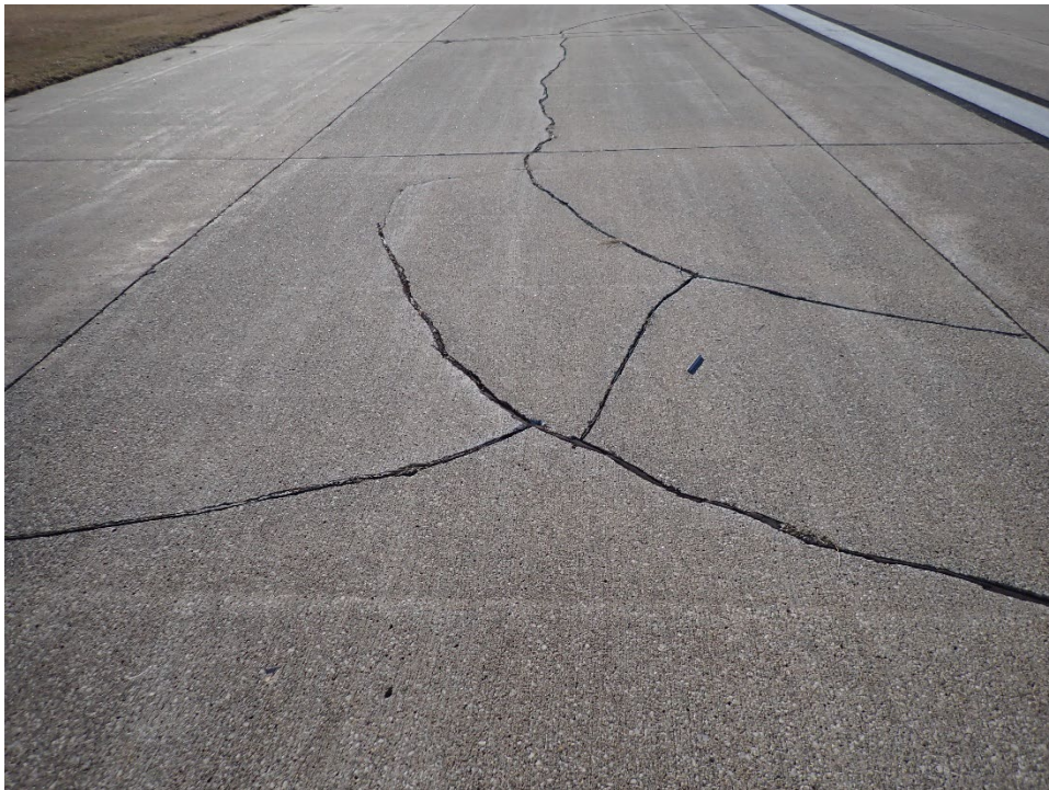
R13EG-02. Shattered Slab (Sample Unit No. 17).
