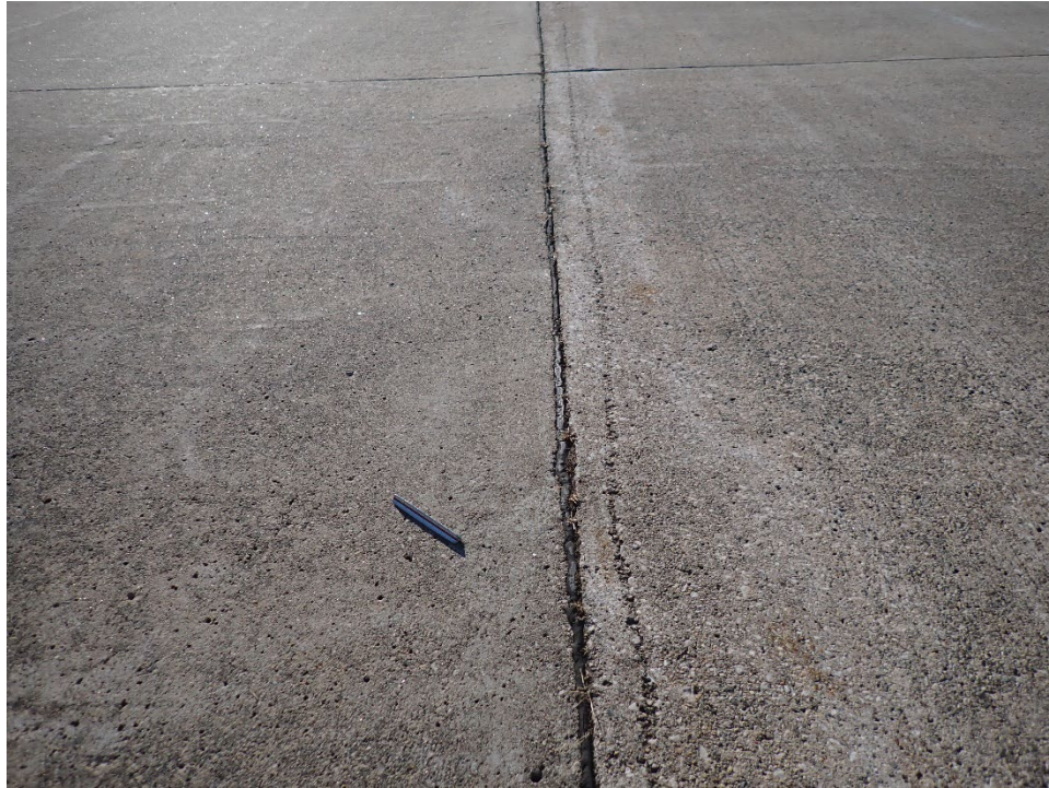
R13EG-02. Joint Seal Damage (Sample Unit No. 03).
