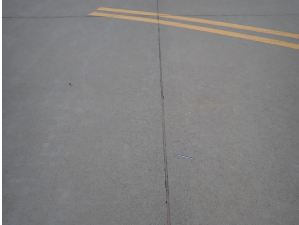
A01DN-02. Joint Seal Damage (Sample Unit No. 08).
