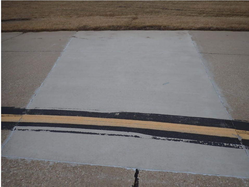
R12DN-04. Large Patching (Sample Unit No. 02).
