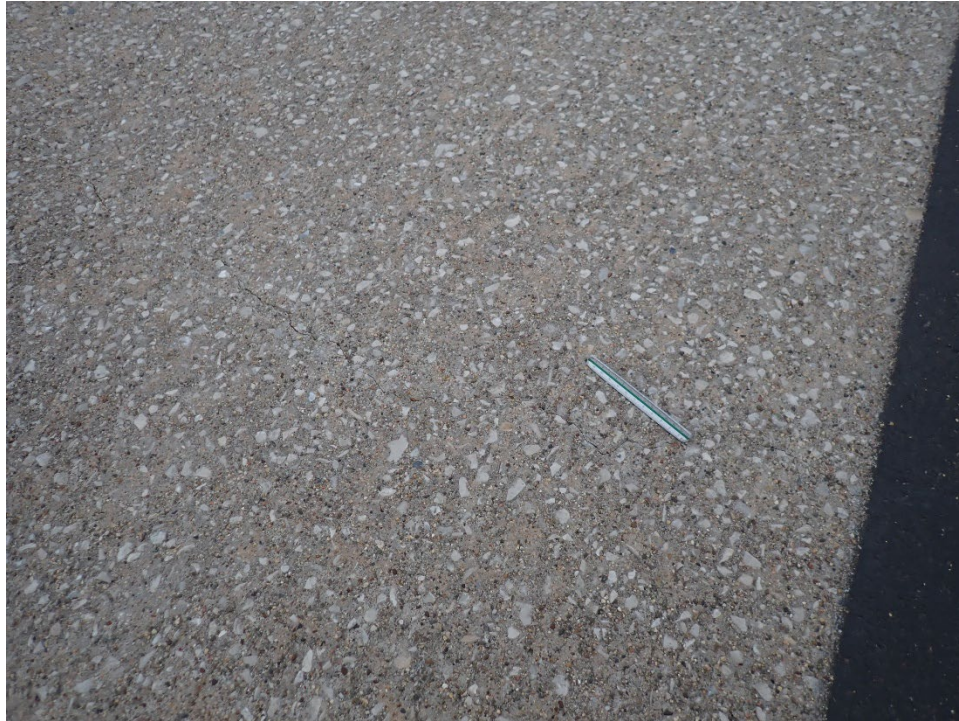
T01DN-05. Shrinkage Cracking (Sample Unit No. 01).
