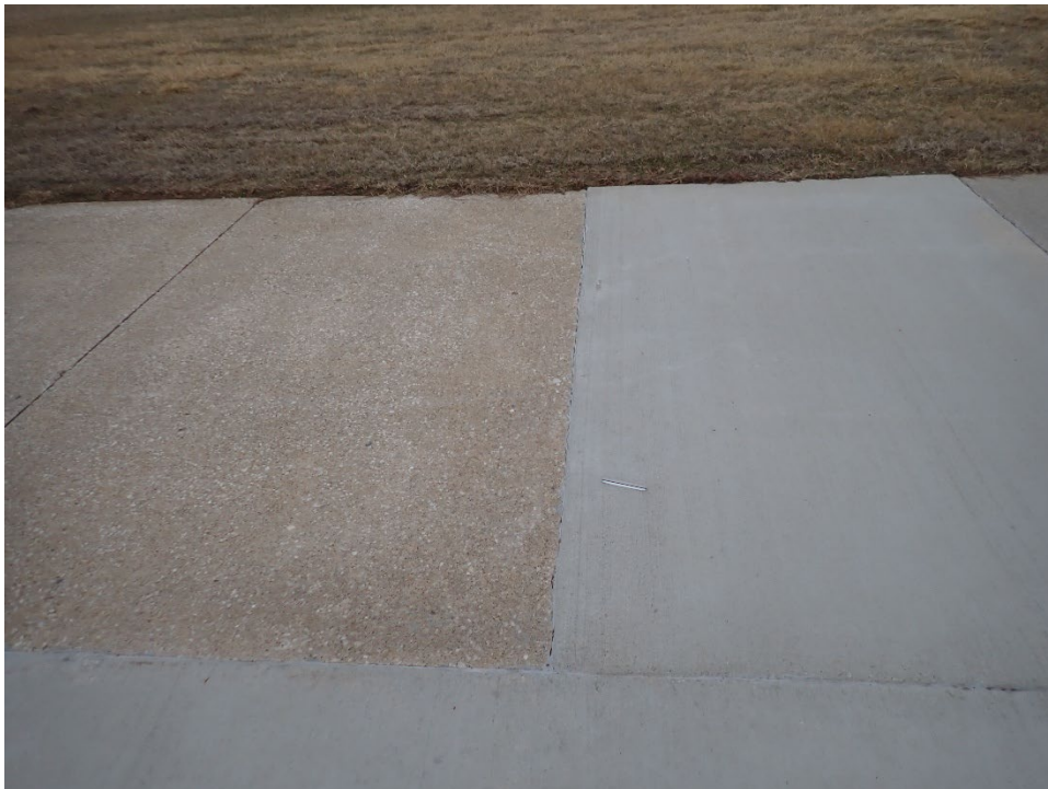
T01DN-03. Large Patching (Sample Unit No. 02).
