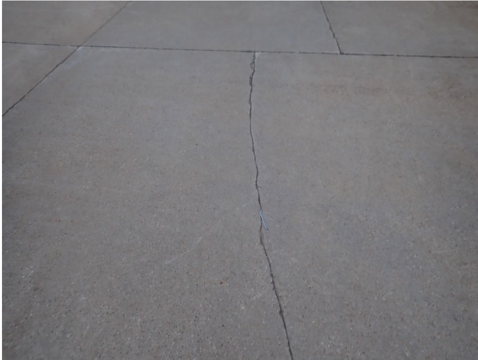
TH01DN-01. LTD Cracking (Sample Unit No. 01).
