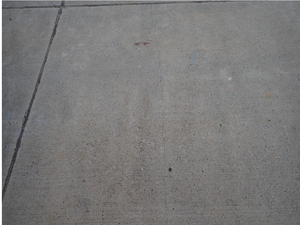
A01DN-02. LTD Cracking (Sample Unit No. 03).
