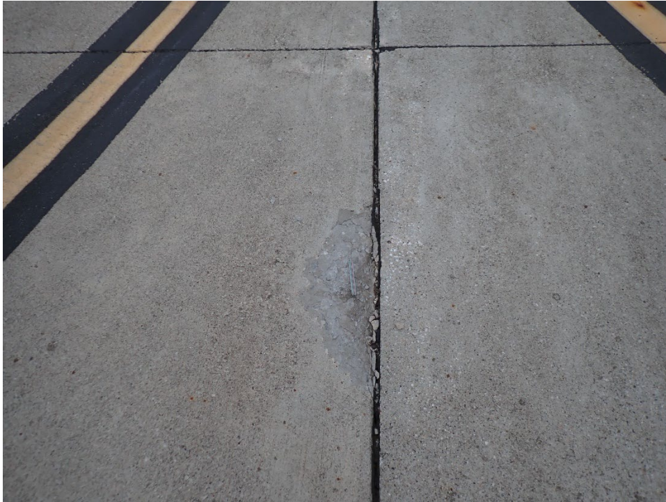
R12DN-07. Joint Spalling (Sample Unit No. 01).
