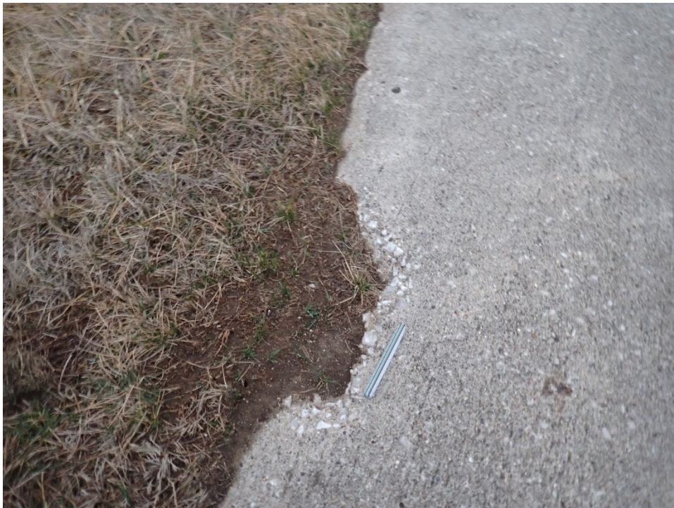
R12DN-06. Joint Spalling (Sample Unit No. 01).
