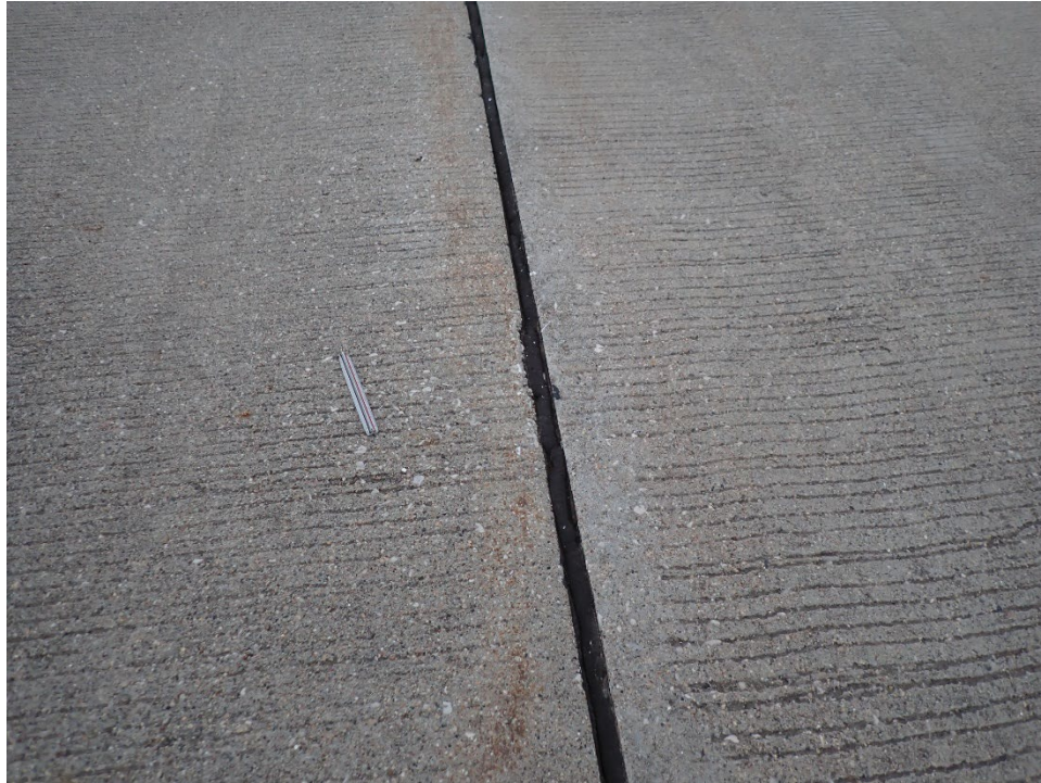
R12DN-02. Joint Seal Damage (Sample Unit No. 09).
