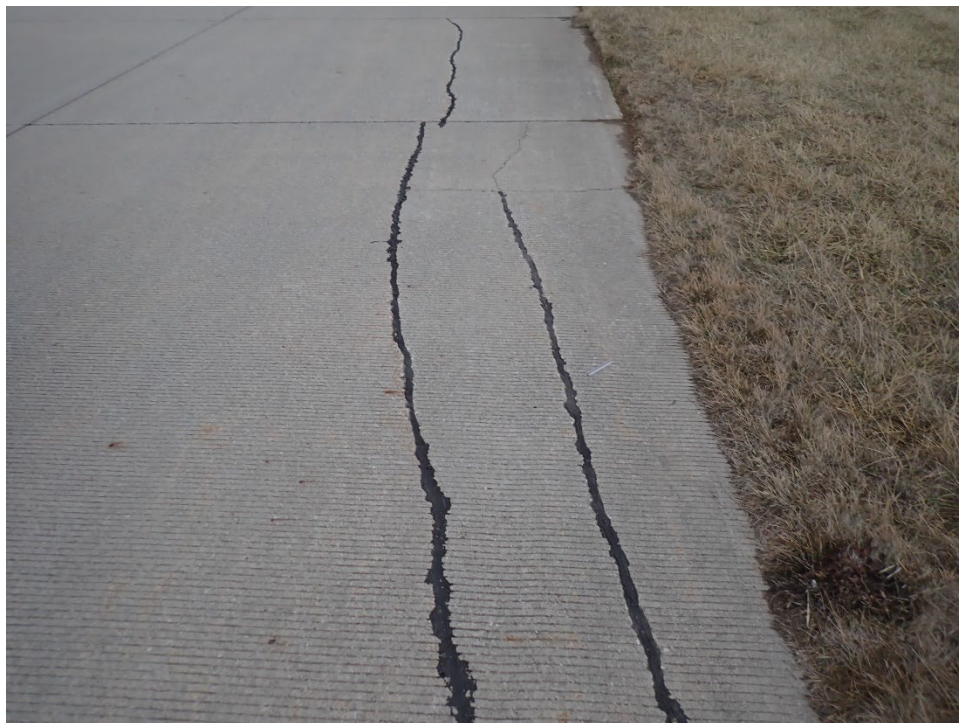
R12DN-01. Shattered Slab (Additional Sample Unit No. 36).
