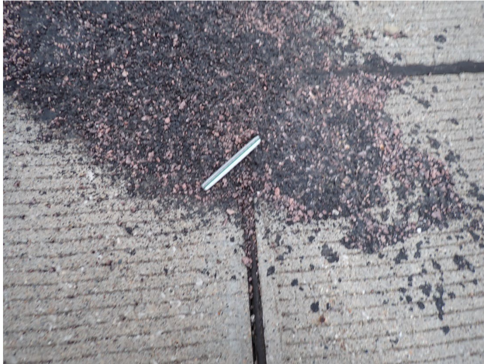
R12DN-01. Small Patching (Sample Unit No. 35).
