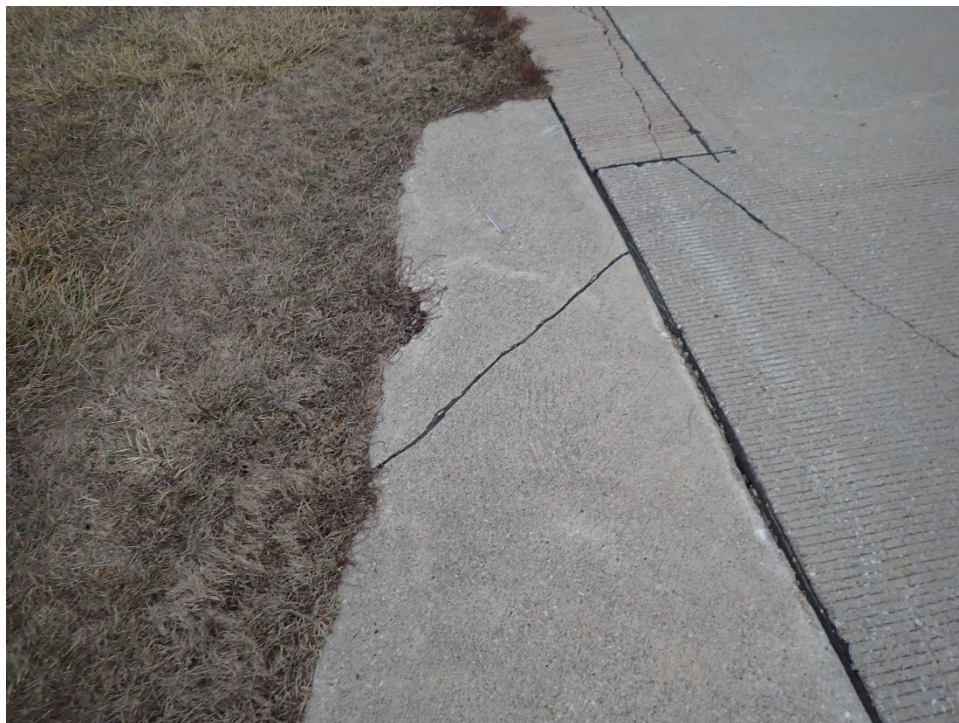
T01DN-06. LTD Cracking (Sample Unit No. 01).
