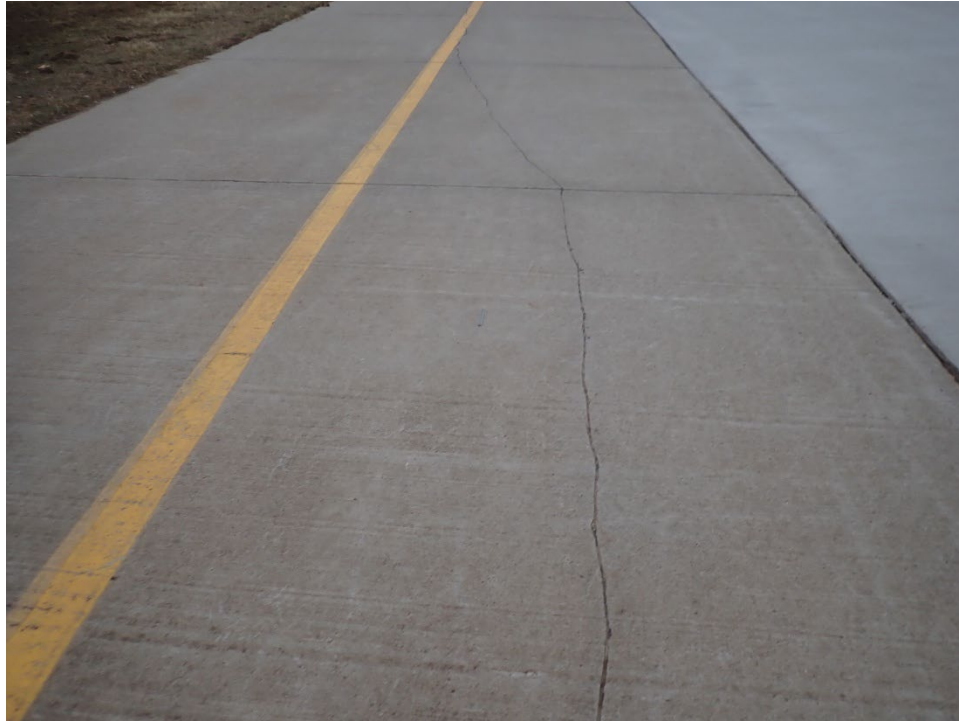
TH01DN-02. LTD Cracking (Sample Unit No. 01).
