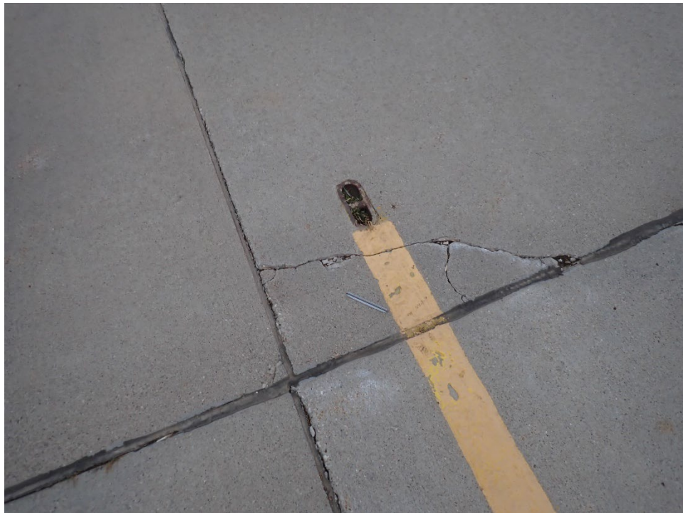
A01DN-02. Joint Spalling (Sample Unit No. 06).
