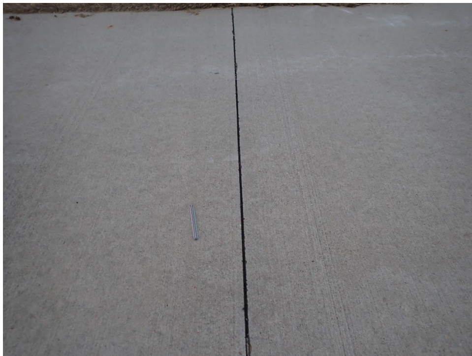
TH01DN-02. Joint Seal Damage (Sample Unit No. 02) (2).
