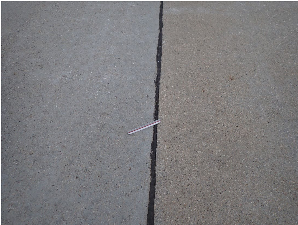
T01DN-01. Joint Seal Damage (Sample Unit No. 02).
