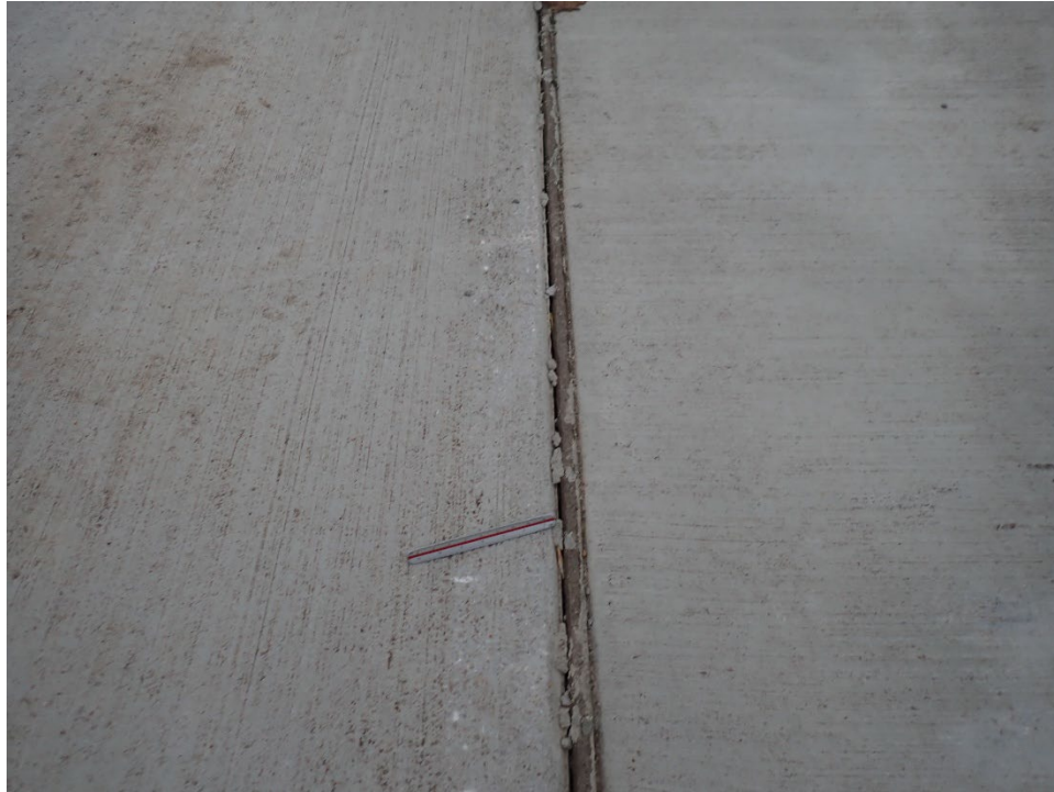
TH01DN-04. Joint Seal Damage (Sample Unit No. 01).
