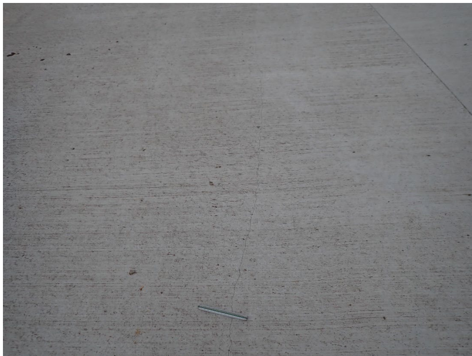
TH01DN-04. Shrinkage Cracking (Sample Unit No. 01).
