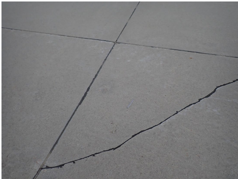
A01DN-02. LTD Cracking (Sample Unit No. 08).
