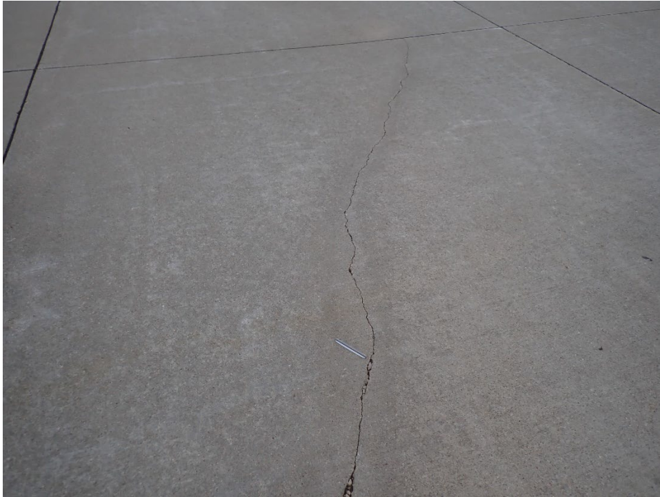
A01DN-01. LTD Cracking (Sample Unit No. 04).
