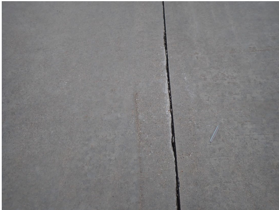
T01DN-04. Joint Seal Damage (Sample Unit No. 01).
