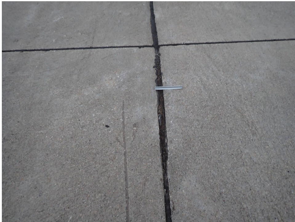
R12DN-05. Joint Seal Damage (Sample Unit No. 02).
