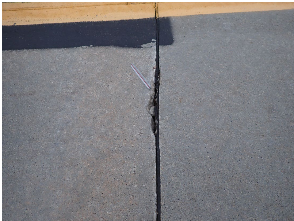
T01DN-02. Joint Seal Damage (Sample Unit No. 01).
