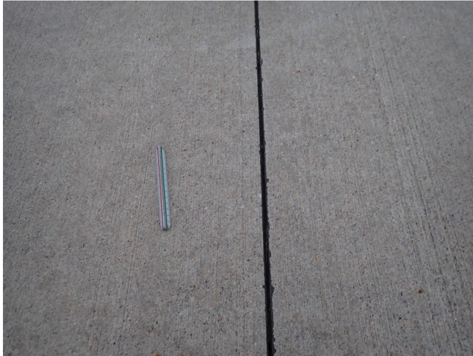
TH01DN-02. Joint Seal Damage (Sample Unit No. 02) (1).
