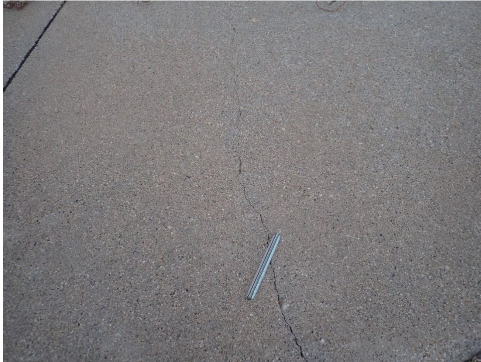
T01DN-01. LTD Cracking (Sample Unit No. 02).
