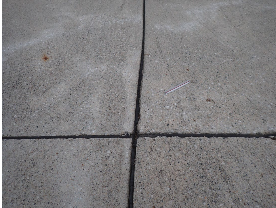
T01DN-06. Joint Seal Damage (Sample Unit No. 01).
