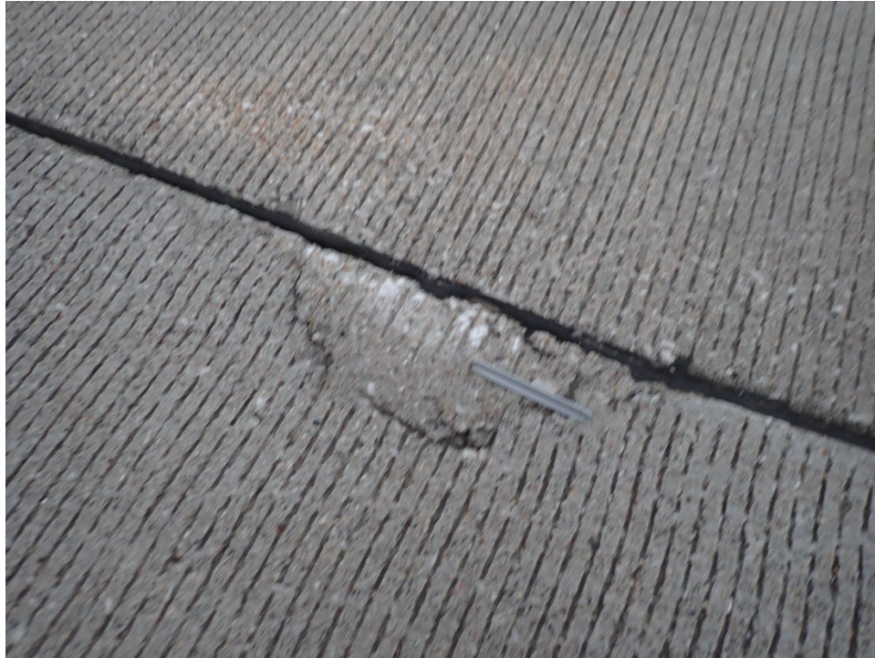
R12DN-01. Joint Spalling (Sample Unit No. 13).
