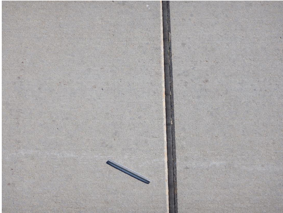
TADA-06. Joint Seal Damage (Sample Unit No. 06).
