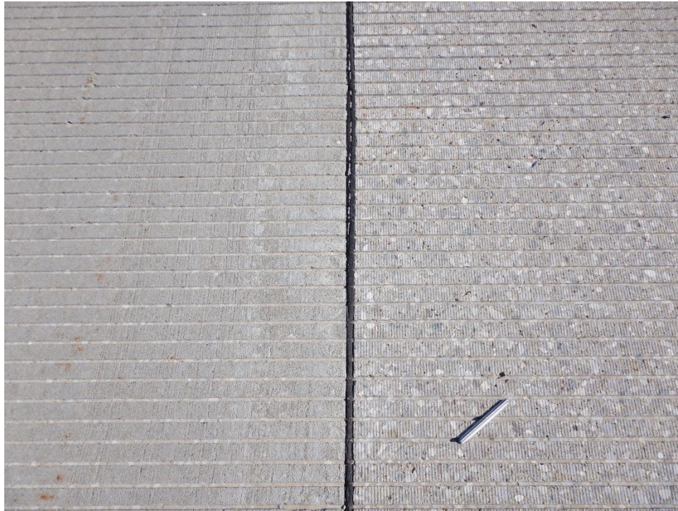
R03DA-01. Joint Seal Damage (Sample Unit No. 99).
