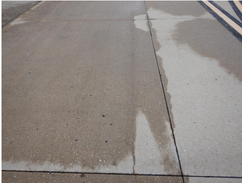
T06DA-01. LTD Cracking (Sample Unit No. 02).
