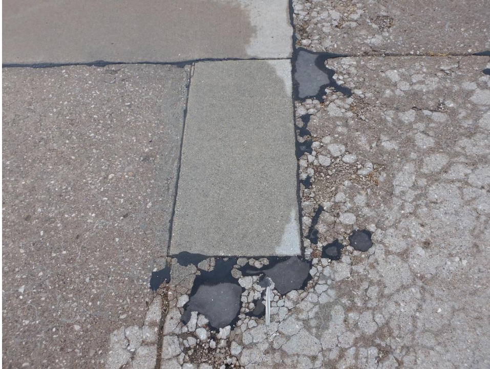
T04DA-01. Small Patching (Sample Unit No. 02).
