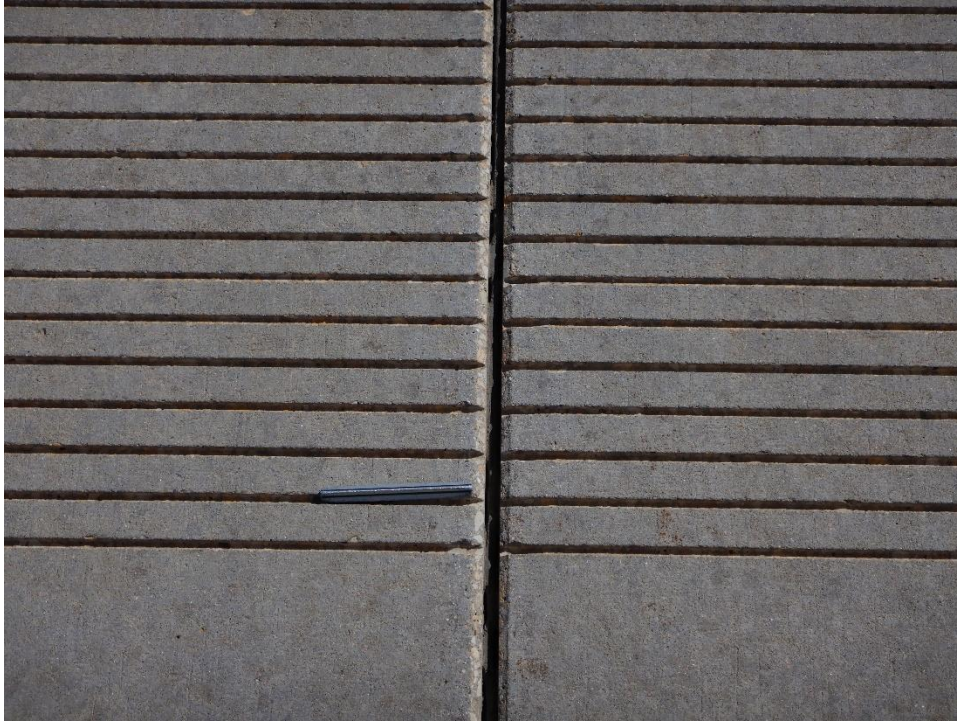
R15DA-01. Joint Seal Damage (Sample Unit No. 61).
