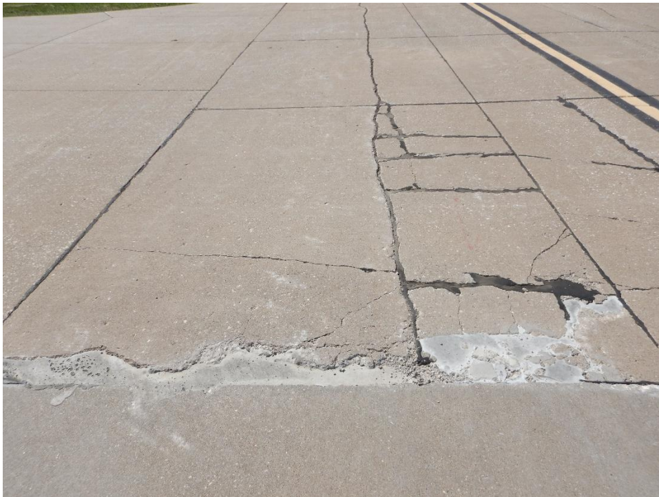
TBDA-01. Shattered Slab (Sample Unit No. 17).
