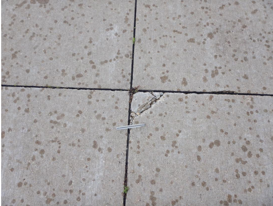
TH01DA-04. Corner Spalling (Sample Unit No. 05).
