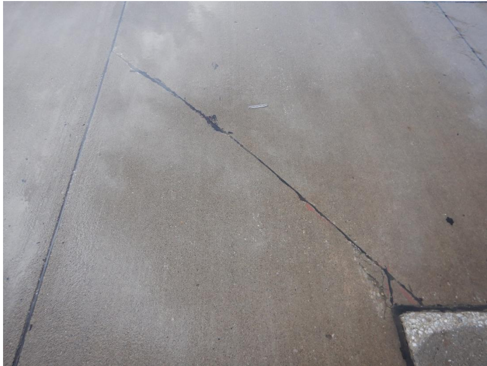
TH01DA-03. LTD Cracking (Sample Unit No. 07).
