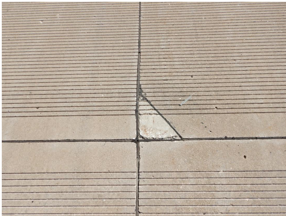
R15DA-02. Small Patching (Sample Unit No. 24).
