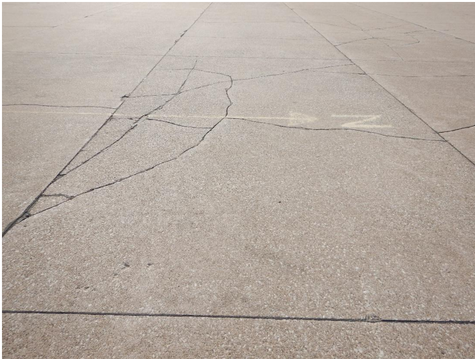
A03DA-01. Shattered Slab (Sample Unit No. 03).
