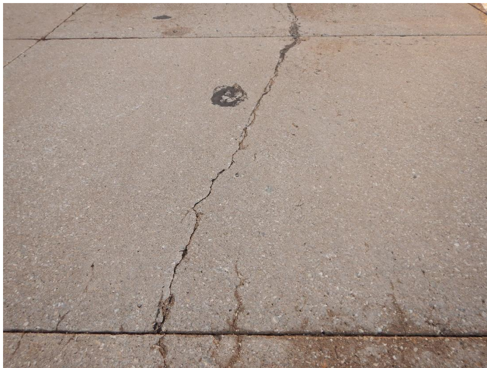
T05DA-01. LTD Cracking (Sample Unit No. 02).
