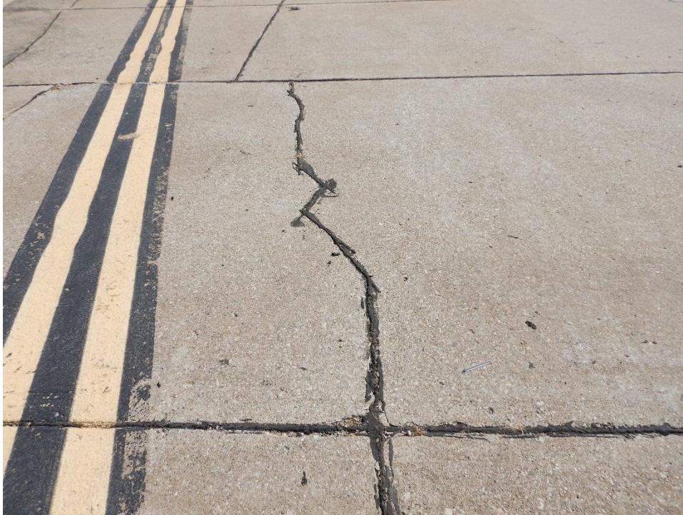
TADA-03. LTD Cracking (Sample Unit No. 03).
