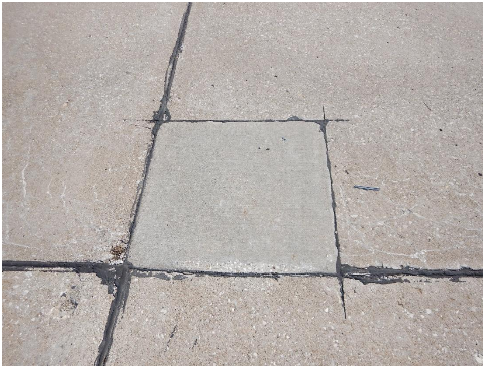
TADA-03. Large Patching (Sample Unit No. 01).
