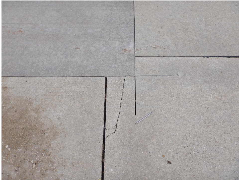
A02DA-02. Corner Spalling (Sample Unit No. 04).
