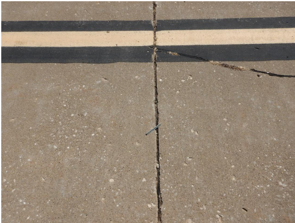
TBDA-01. Joint Seal Damage (Sample Unit No. 02).
