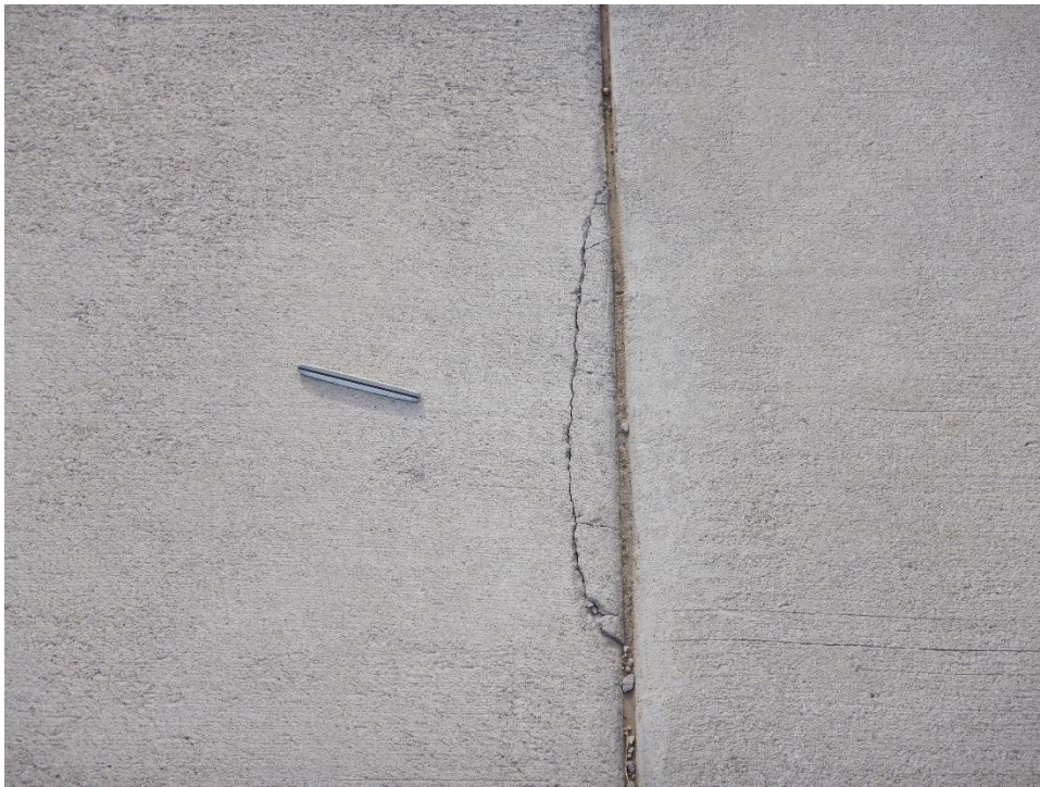
A04DA-01. Joint Spalling (Sample Unit No. 14).
