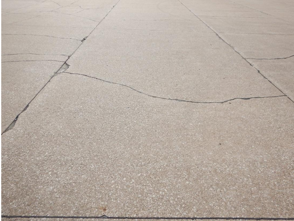
A03DA-01. LTD Cracking (Sample Unit No. 04).
