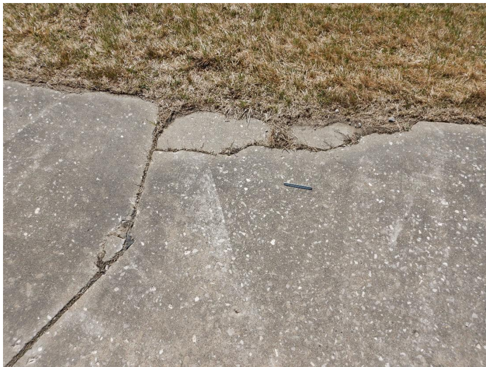
TB1DA-02. Corner Break (Sample Unit No. 04).
