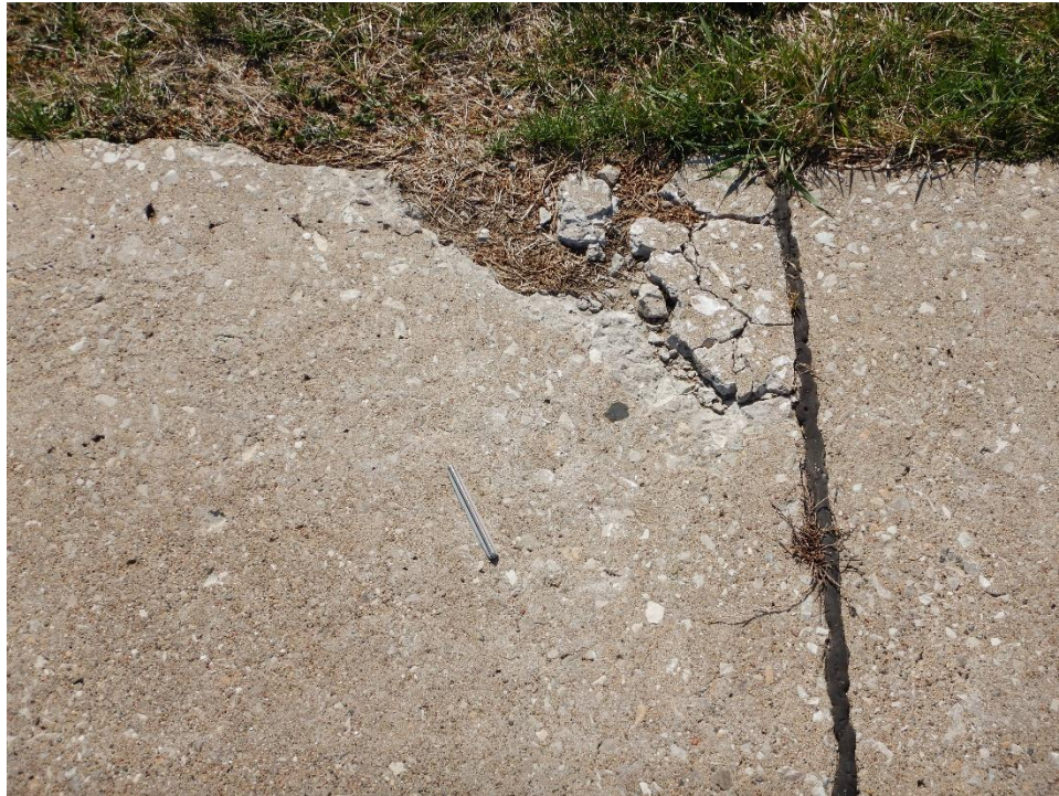
TADA-02. Corner Spalling (Sample Unit No. 04).
