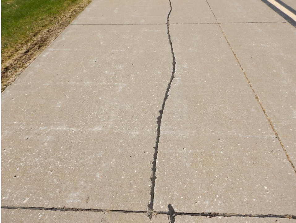
TBDA-01. LTD Cracking (Sample Unit No. 02) (1).
