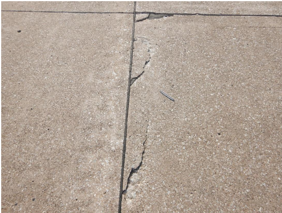
TCDA-01. Joint Spalling (Sample Unit No. 10).
