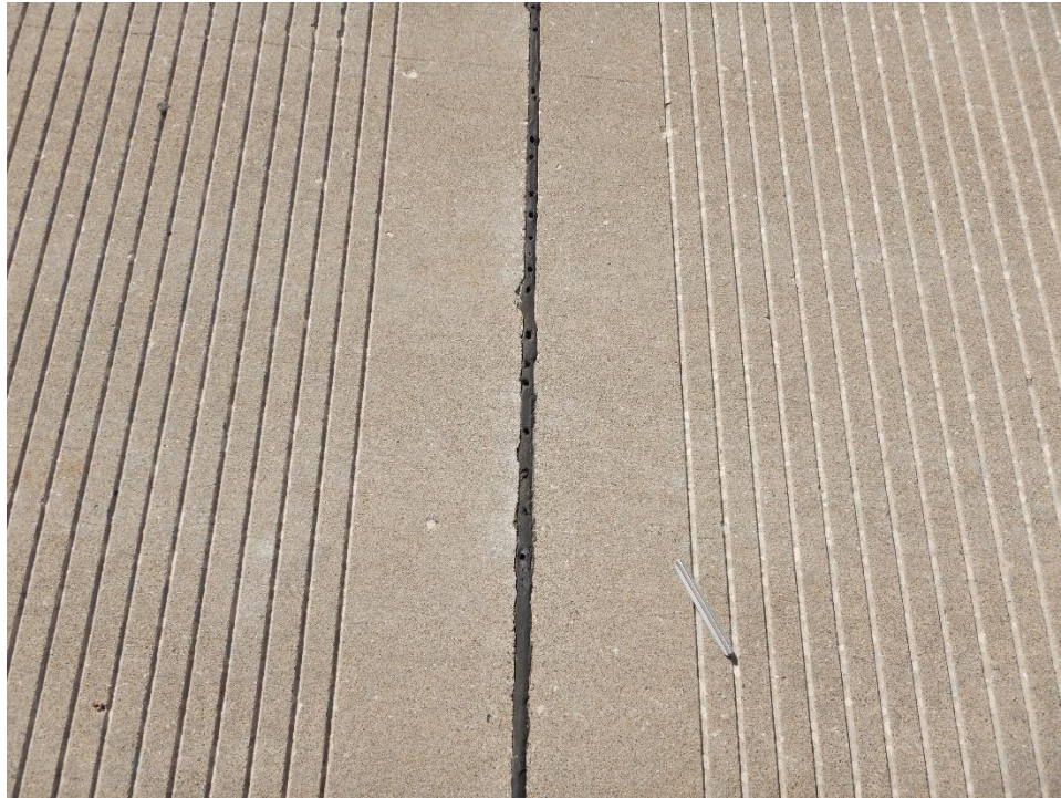
R15DA-02. Joint Seal Damage (Sample Unit No. 15).
