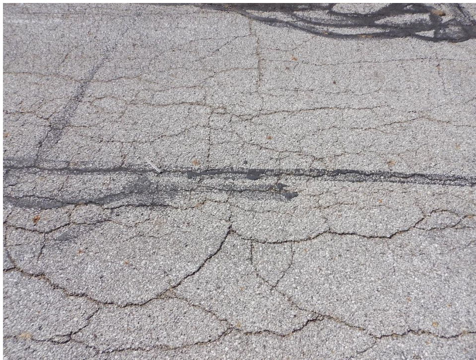
TH01DA-02. Alligator Cracking (Sample Unit No. 05).
