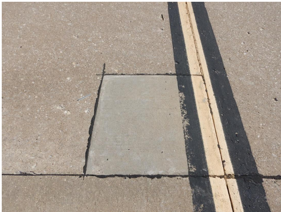
TADA-02. Large Patching (Sample Unit No. 02).
