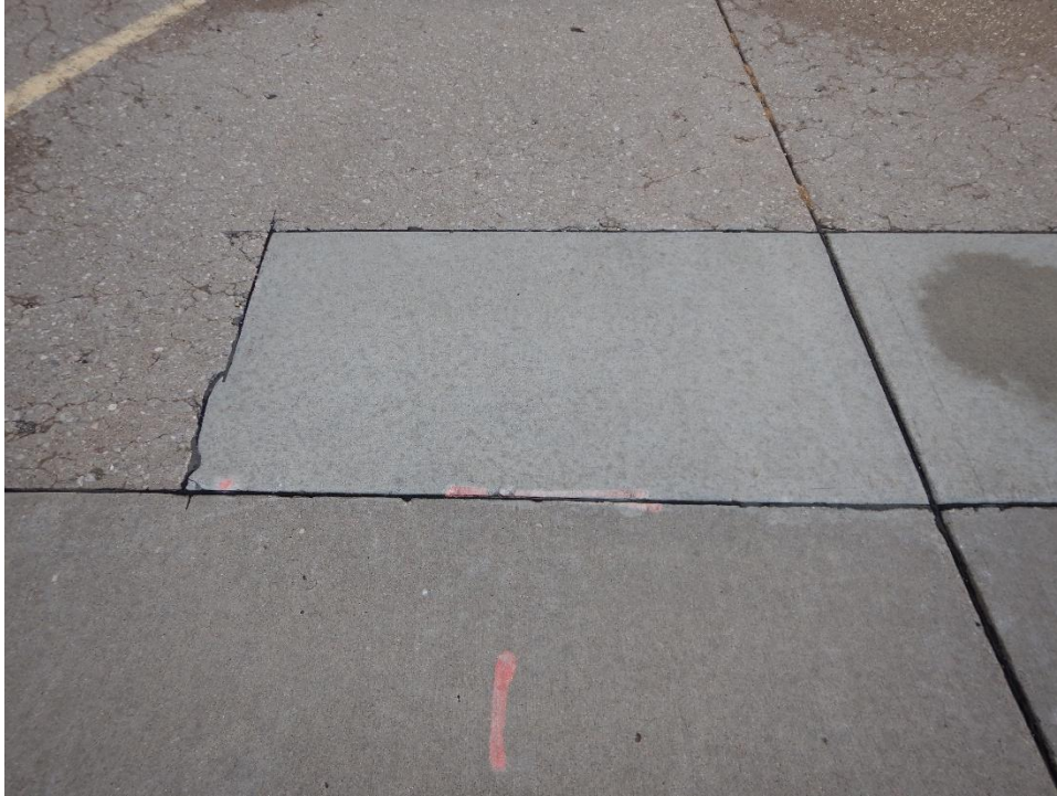
T05DA-01. Large Patching (Sample Unit No. 01).
