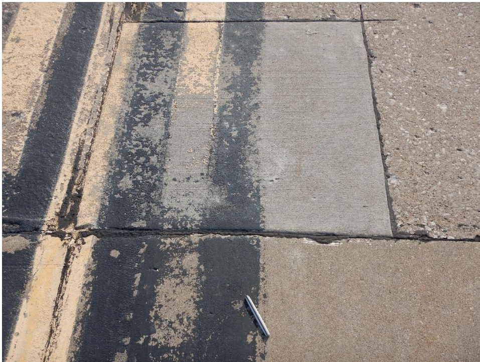
TCDA-02. Large Patching (Sample Unit No. 04).
