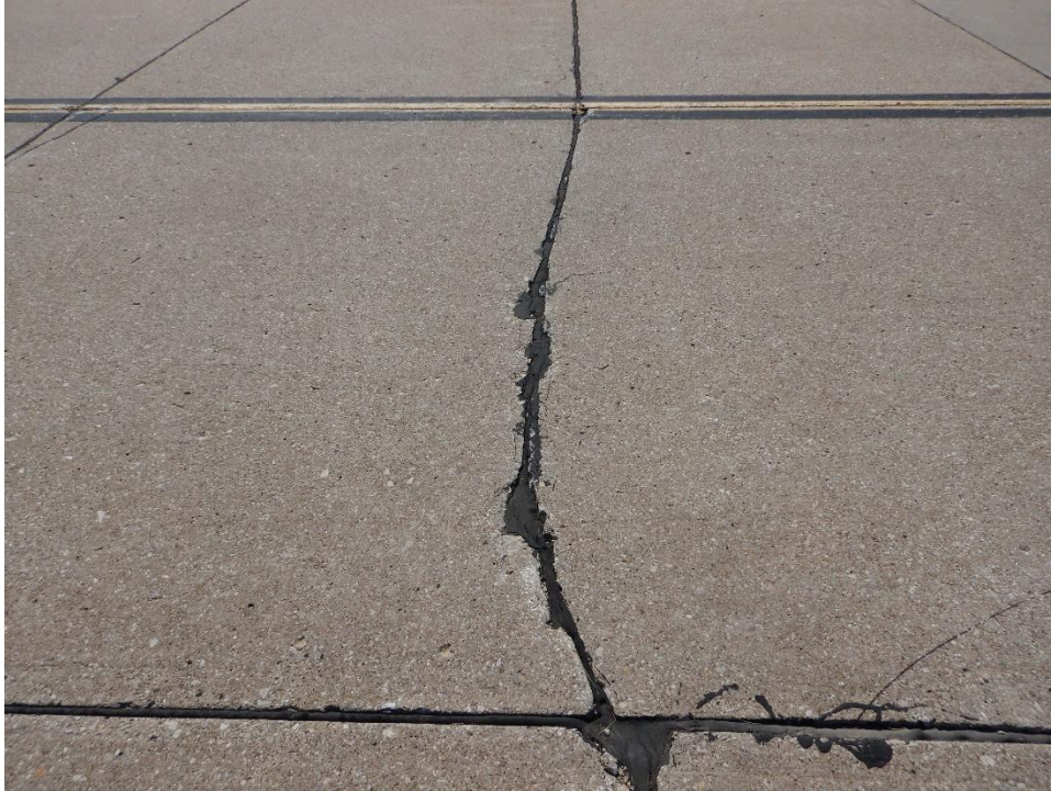
TADA-01. LTD Cracking (Additional Sample Unit No. 04).
