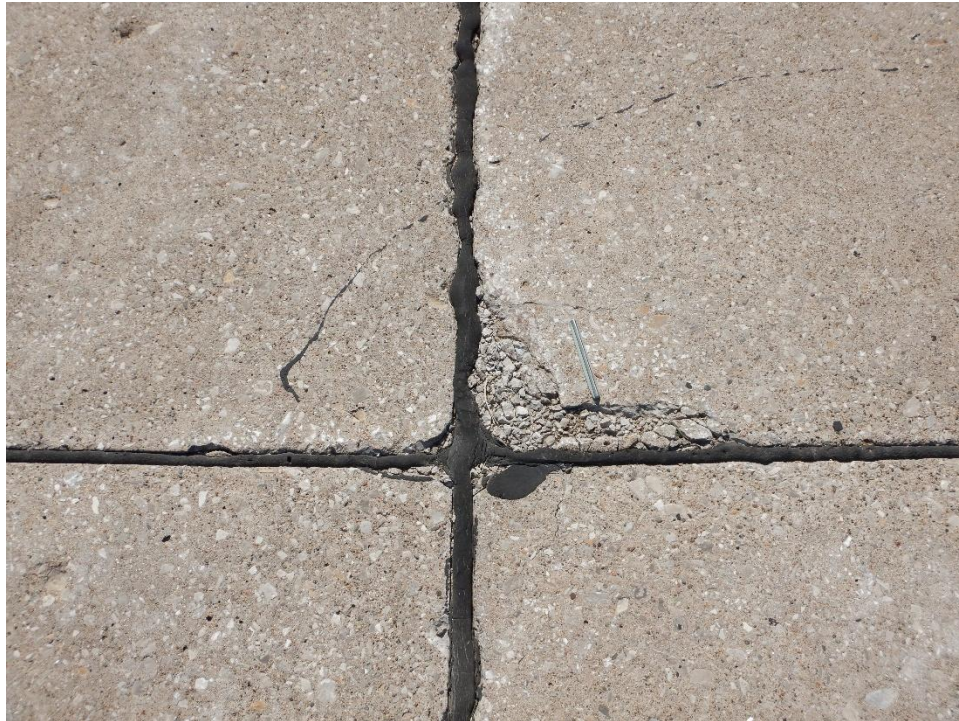
TADA-01. ASR (Additional Sample Unit No. 04).
