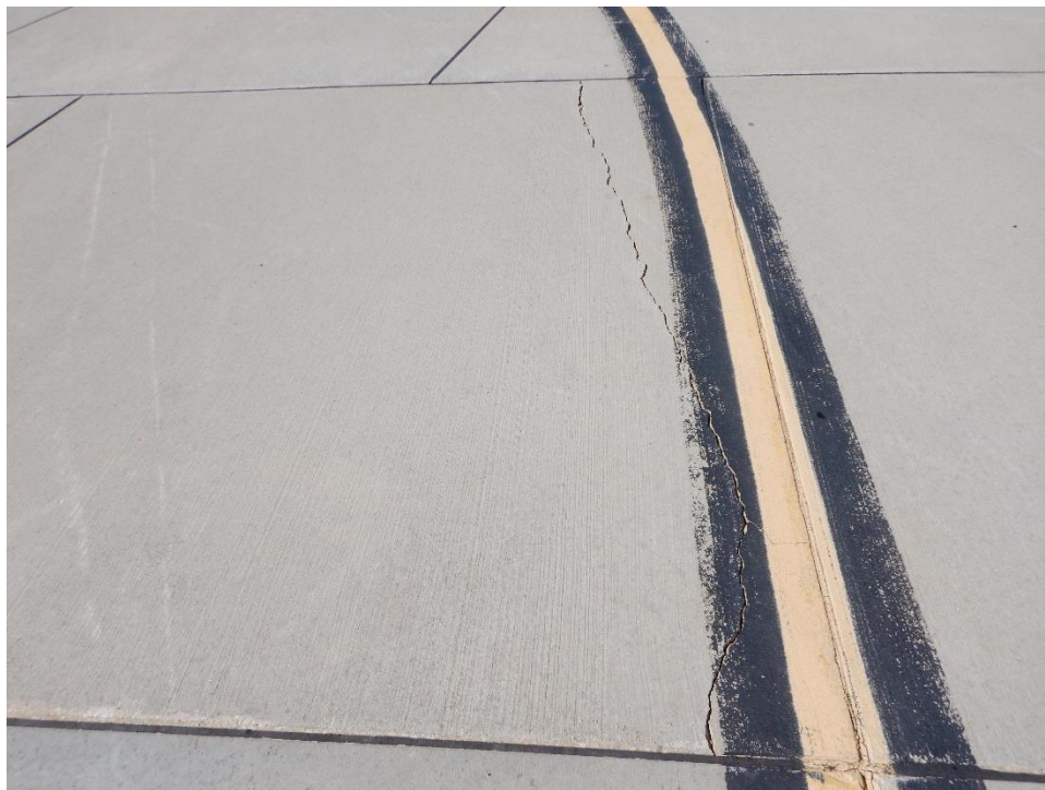
TADA-06. LTD Cracking (Additional Sample Unit No. 08).
