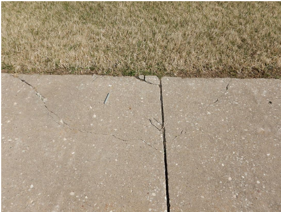
TB1DA-01. Corner Break (Sample Unit No. 01).
