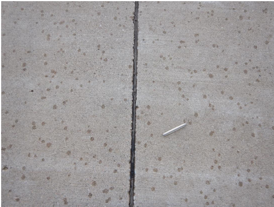
TH01DA-03. Joint Seal Damage (Sample Unit No. 02).
