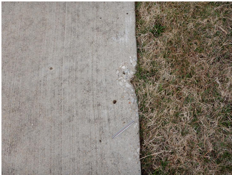
T06DA-01. Joint Spalling (Sample Unit No. 01).
