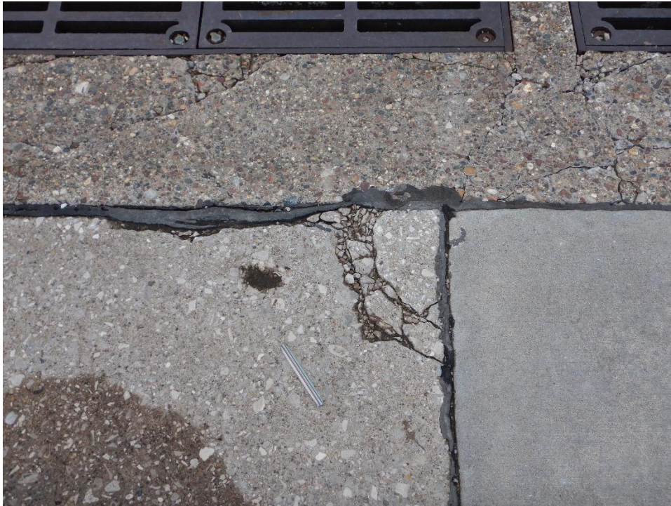
A02DA-01. Corner Spalling (Sample Unit No. 09).
