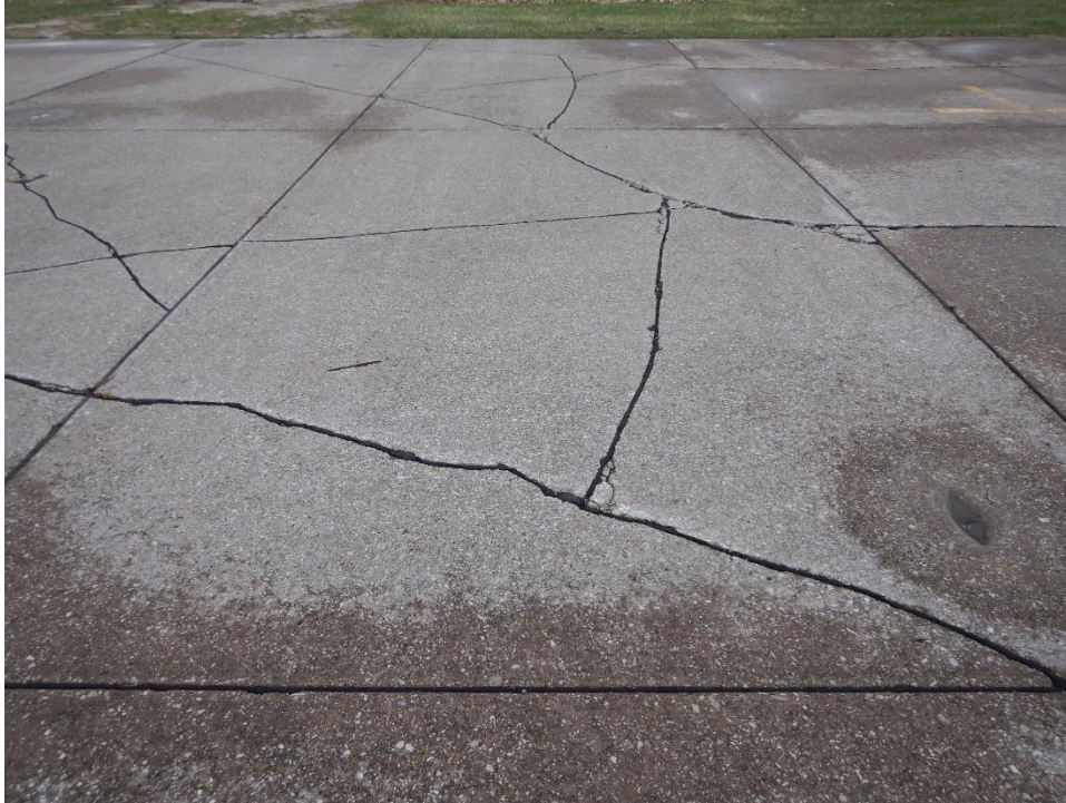
A02DA-01. Shattered Slab (Sample Unit No. 07).
