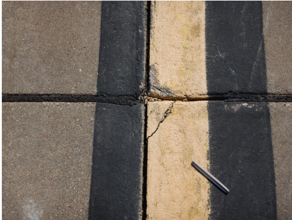
TB1DA-02. Corner Spalling (Sample Unit No. 01).
