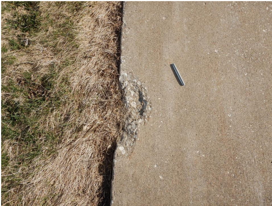
TADA-07. Joint Spalling (Sample Unit No. 17) (1).
