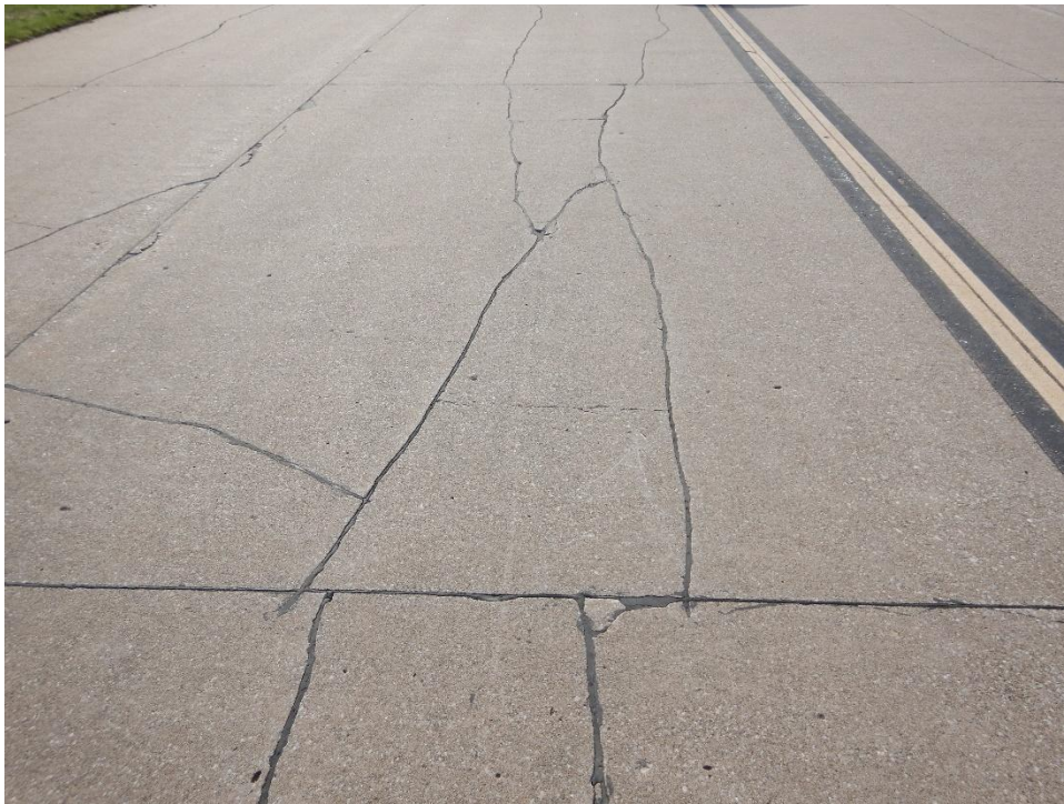
TCDA-01. Shattered Slab (Sample Unit No. 10).
