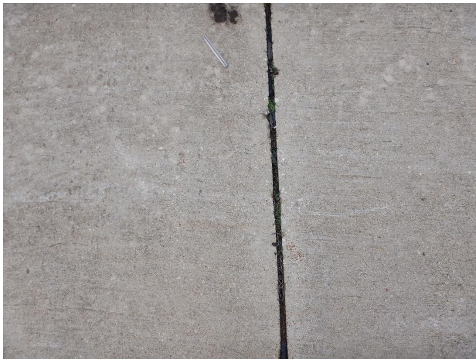
A02DA-02. Joint Seal Damage (Sample Unit No. 04).
