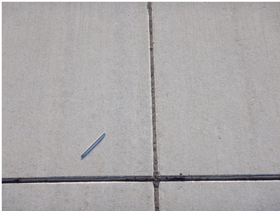
TCDA-03. Joint Seal Damage (Sample Unit No. 03).
