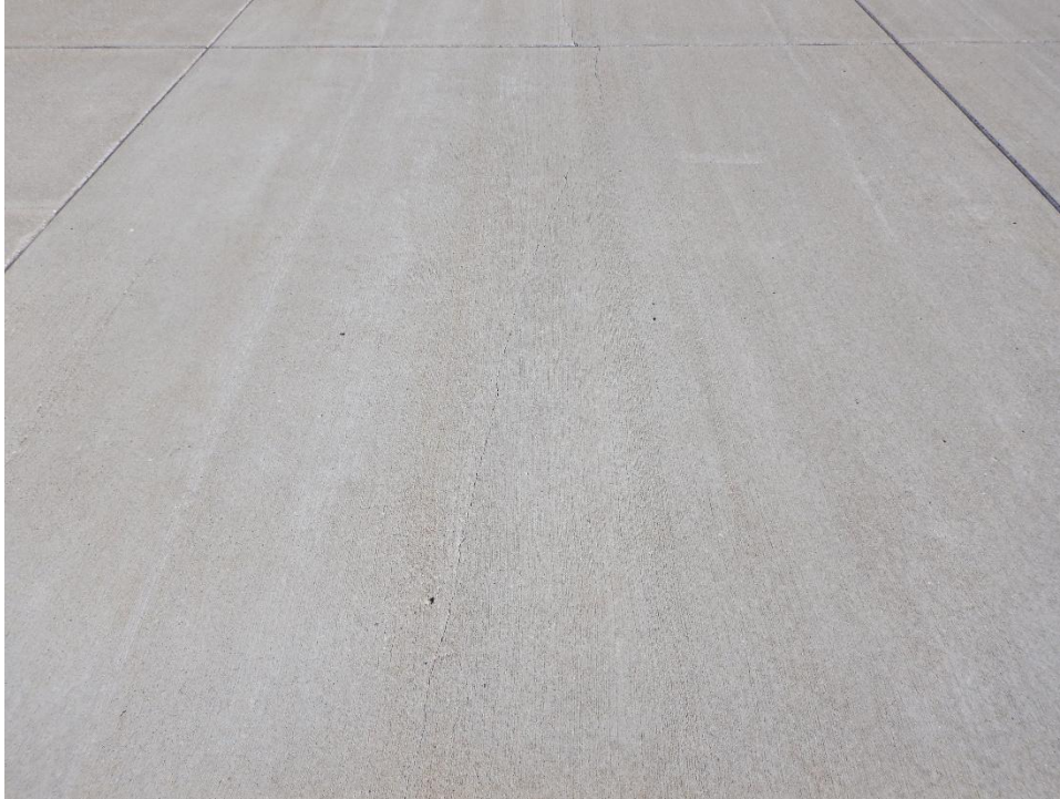
TADA-05. LTD Cracking (Sample Unit No. 01).
