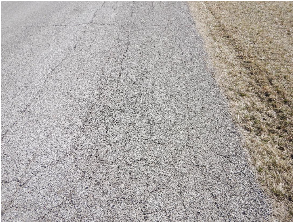
TH01DA-01. Alligator Cracking (Sample Unit No. 02).
