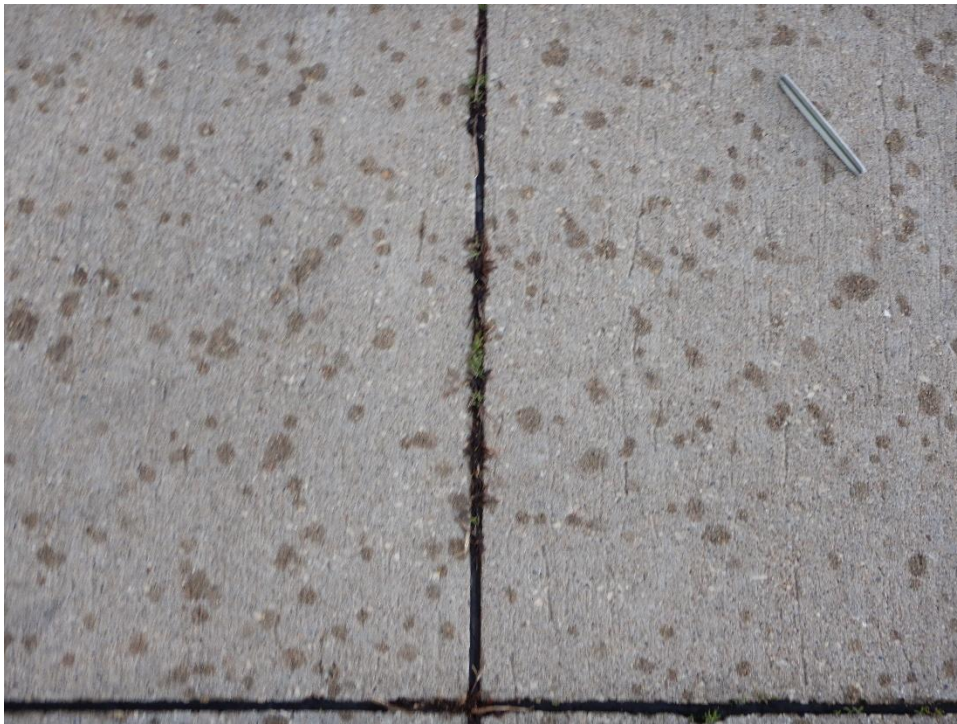
TH01DA-04. Joint Seal Damage (Sample Unit No. 05).
