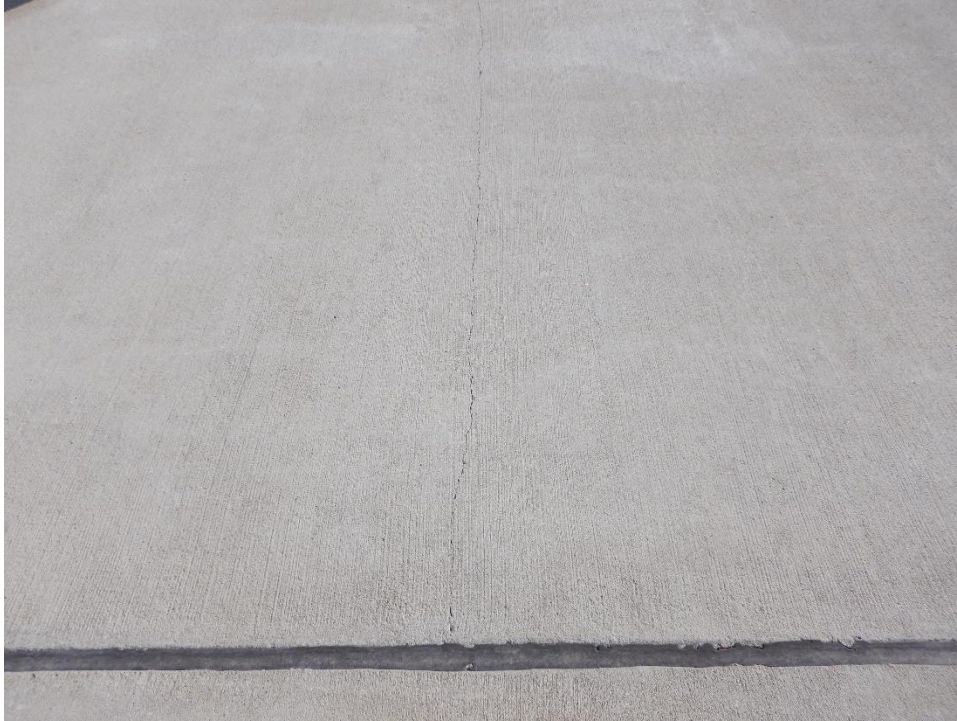
A04DA-01. LTD Cracking (Sample Unit No. 12).
