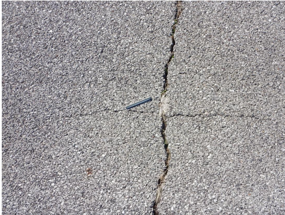
TH01DA-01. L&T Cracking (Sample Unit No. 02).
