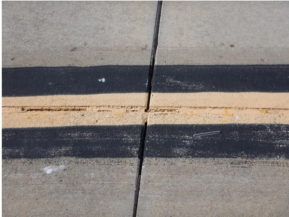
TB1DA-03. Joint Seal Damage (Sample Unit No. 04).
