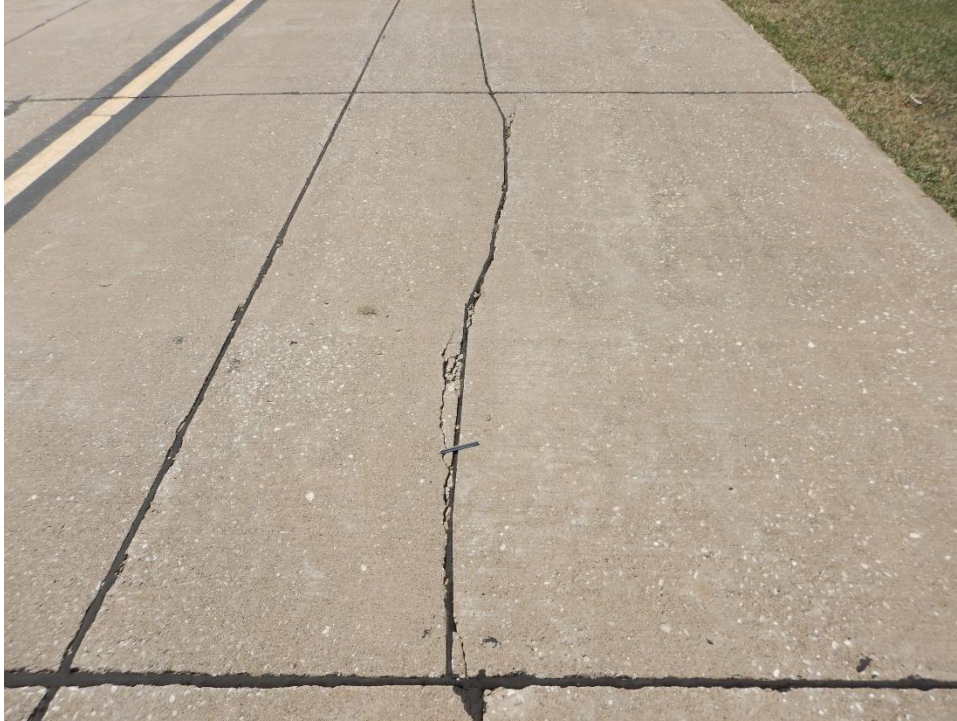
TBDA-01. LTD Cracking (Sample Unit No. 17).
