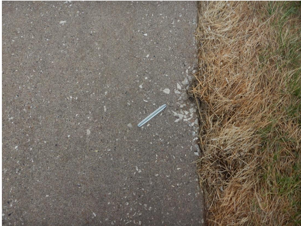
TADA-07. Joint Spalling (Sample Unit No. 17) (2).
