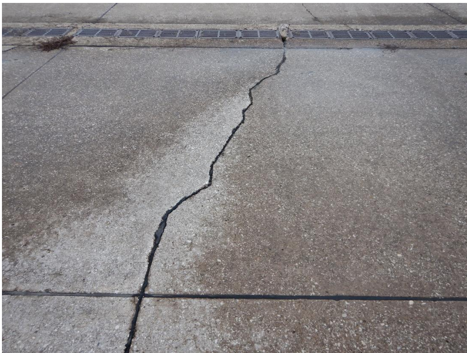
A02DA-01. LTD Cracking (Sample Unit No. 07).
