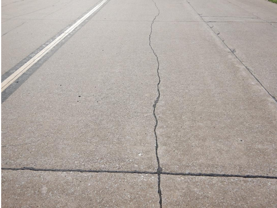
TCDA-01. LTD Cracking (Sample Unit No. 10).
