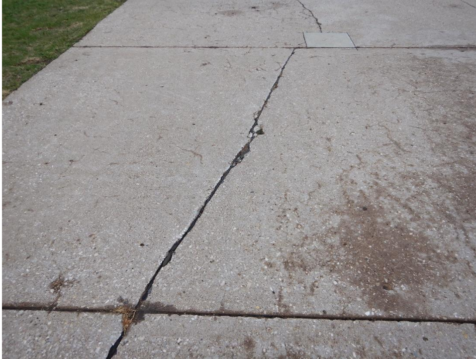
A01DA-01. LTD Cracking (Sample Unit No. 07).
