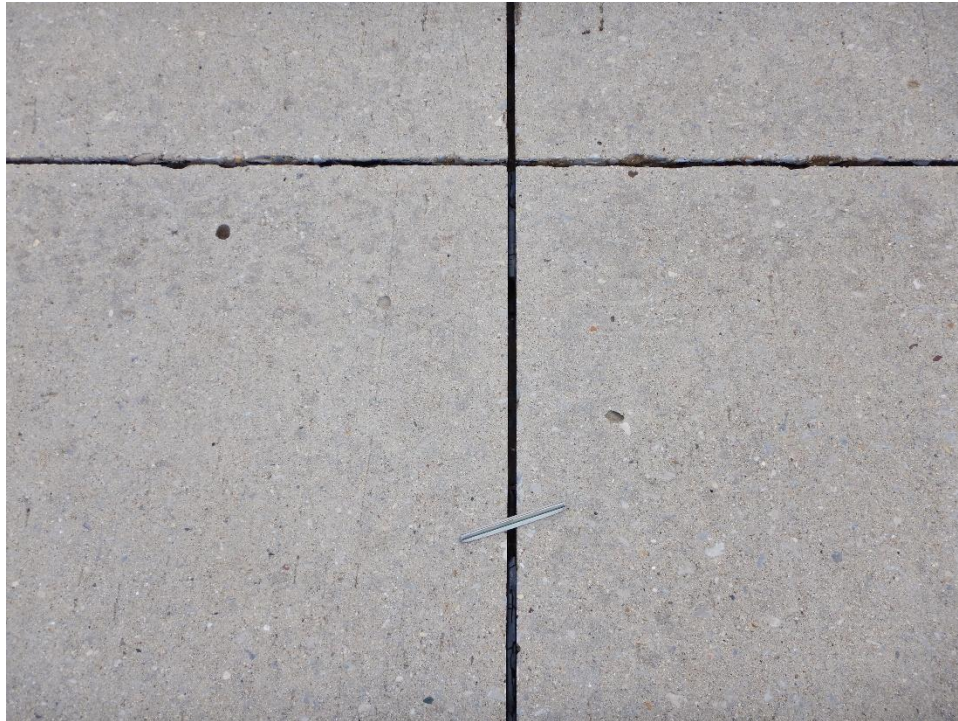
T06DA-01. Joint Seal Damage (Sample Unit No. 01).
