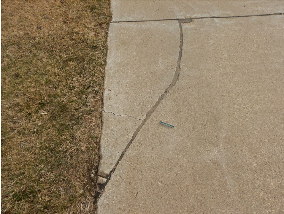
A01CT-01. LTD Cracking (Sample Unit No. 006).
