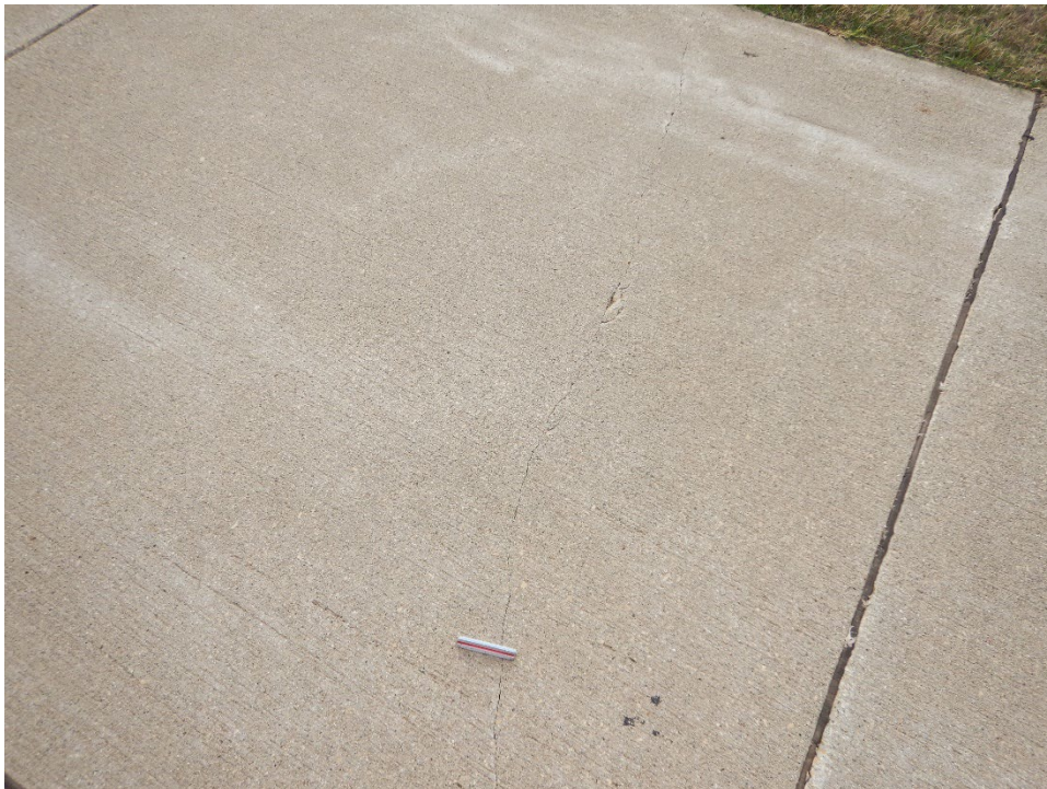
A01CT-01. LTD Cracking (Sample Unit No. 029).
