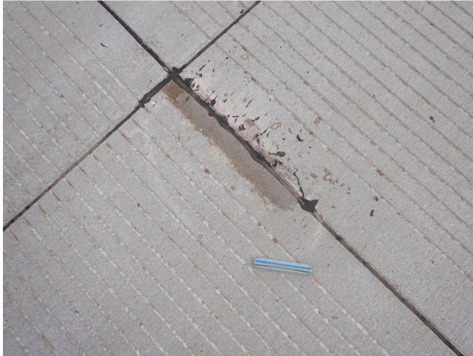
R16CT-02. Small Patching (Sample Unit No. 067).
