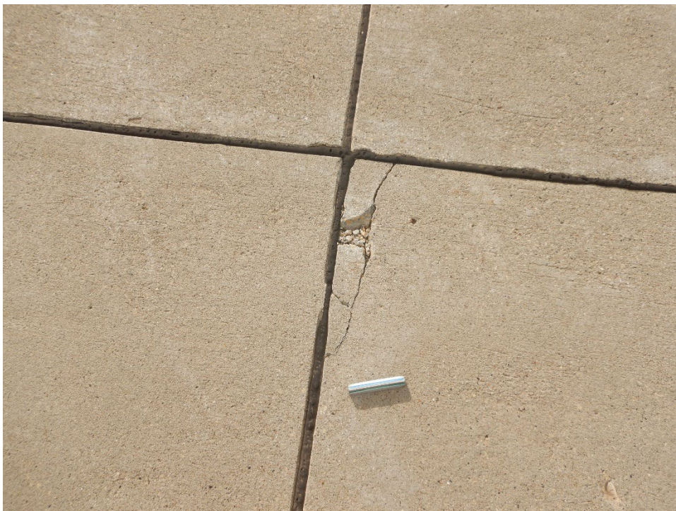
A01CT-01. Joint Spalling (Sample Unit No. 006).
