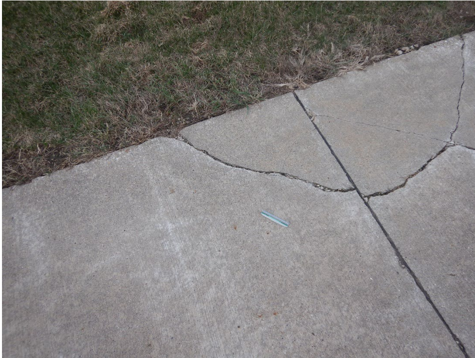
TH01CT-01. Corner Break (Sample Unit No. 03).
