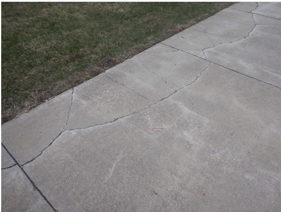
TH01CT-01. Shattered Slab (Sample Unit No. 03).
