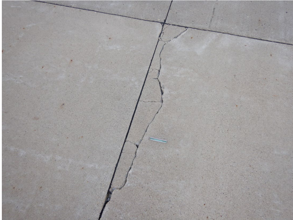
TH01CT-02. Joint Spalling (Sample Unit No. 04).
