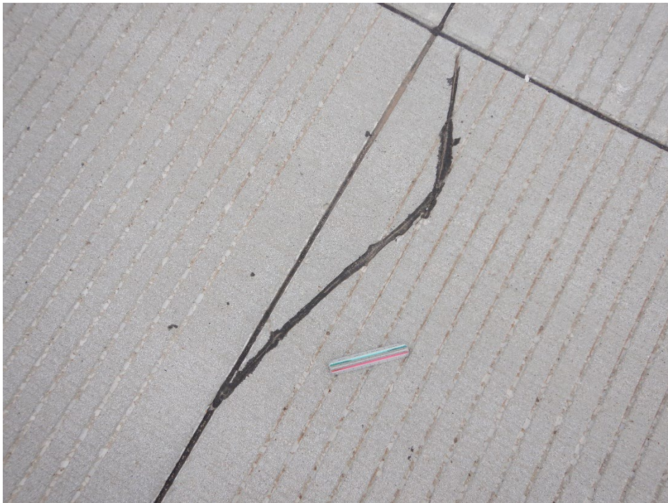
R16CT-02. Joint Spalling (Sample Unit No. 027).
