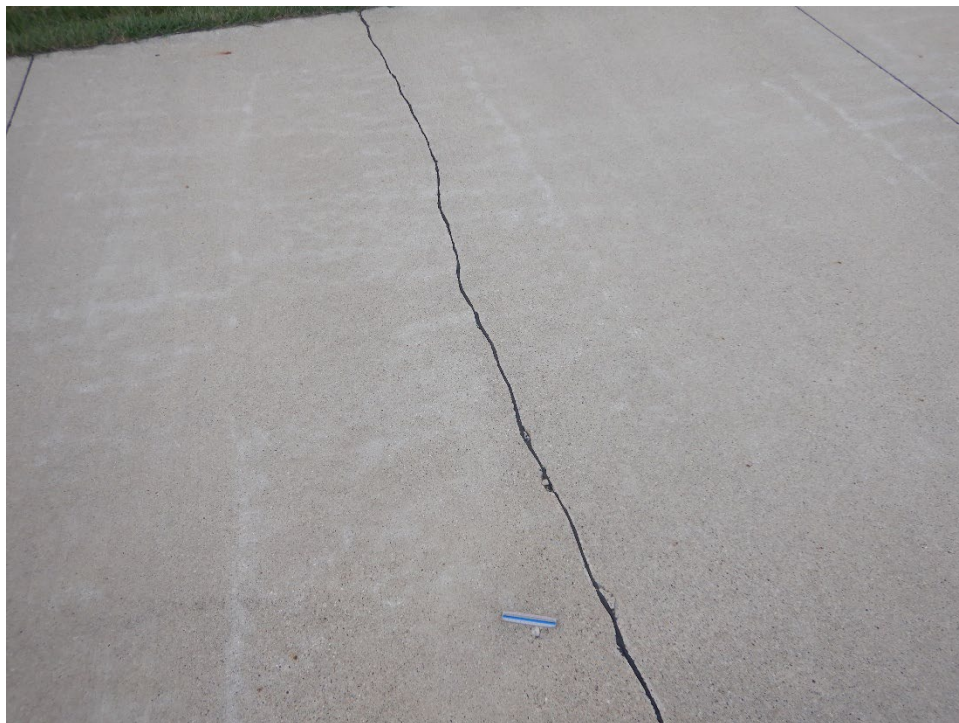
TH01CT-02. LTD Cracking (Sample Unit No. 05).
