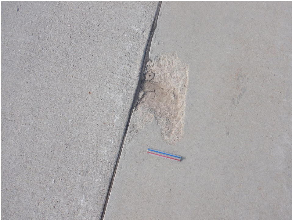
R16CT-01. Joint Spalling (Sample Unit No. 10).
