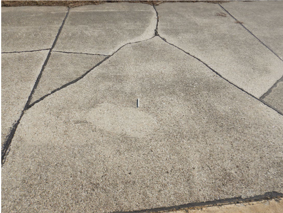
A01CR-03. Shattered Slab (Sample Unit No. 02).
