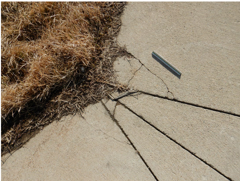
T04CR-01. Corner Spalling (Sample Unit No. 02).
