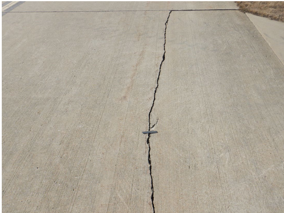
T03CR-01. LTD Cracking (Sample Unit No. 03).
