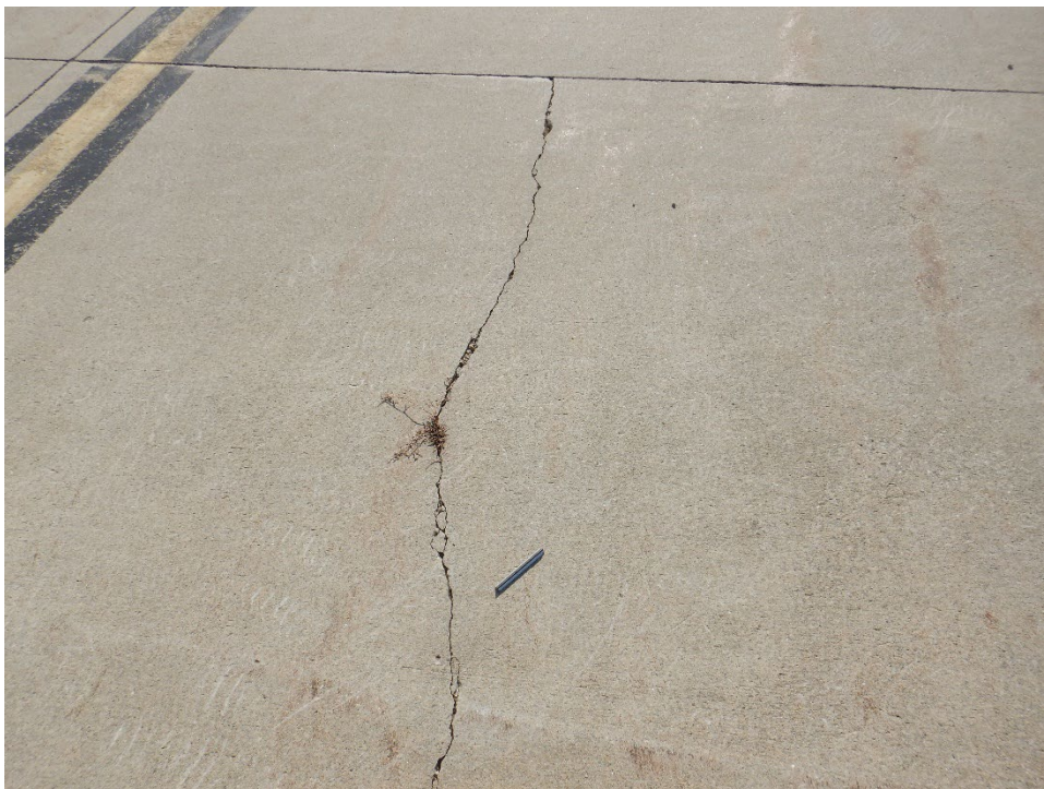
T01CR-01. LTD Cracking (Sample Unit No. 01).
