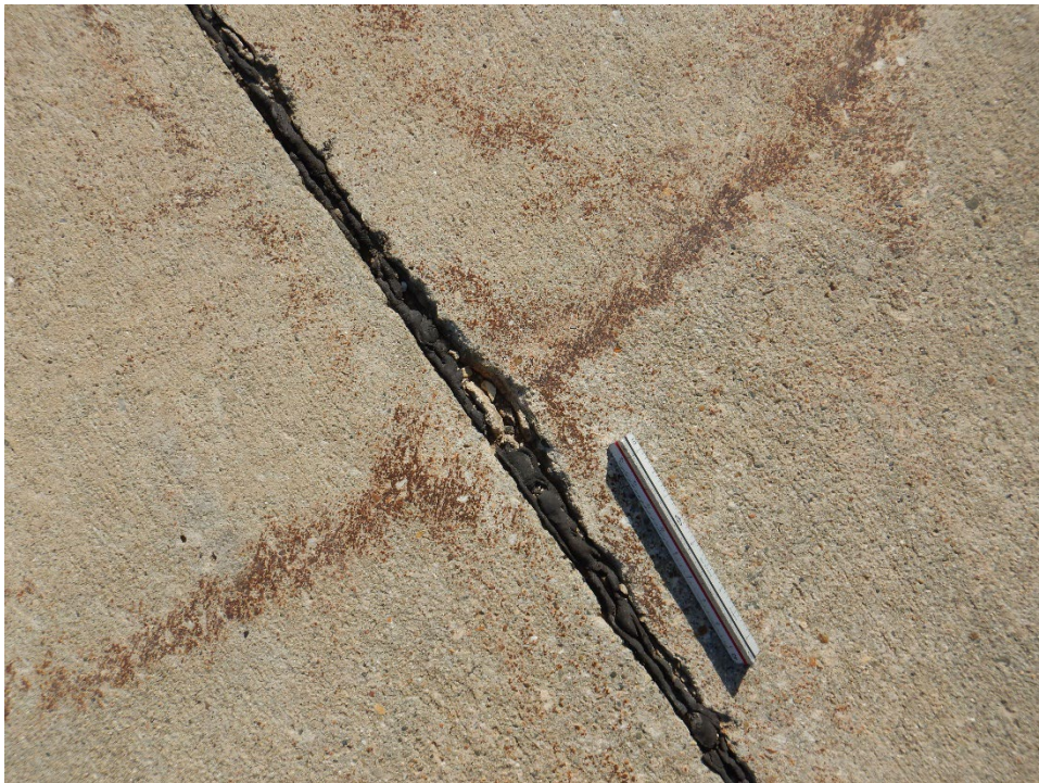
A01CR-01. Joint Seal Damage (Sample Unit No. 01).
