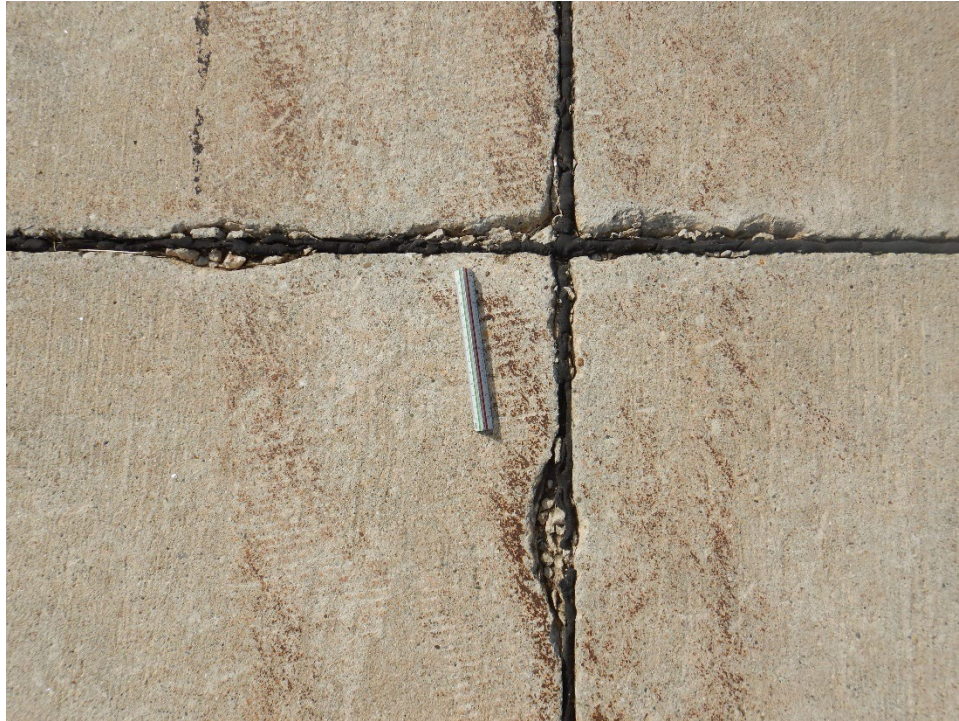
T03CR-01. Joint Seal Damage (Sample Unit No. 07).
