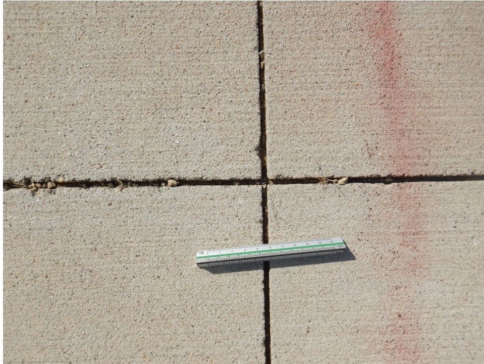
T04CR-01. Joint Seal Damage (Sample Unit No. 02).
