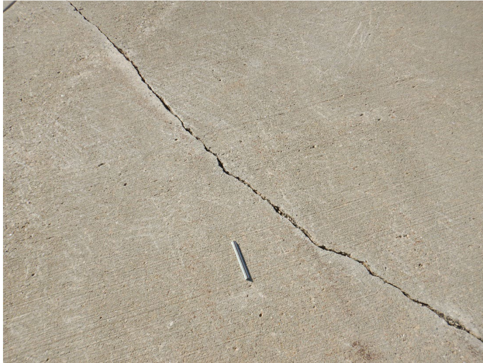
A02CR-01. LTD Cracking (Sample Unit No. 02) (2).
