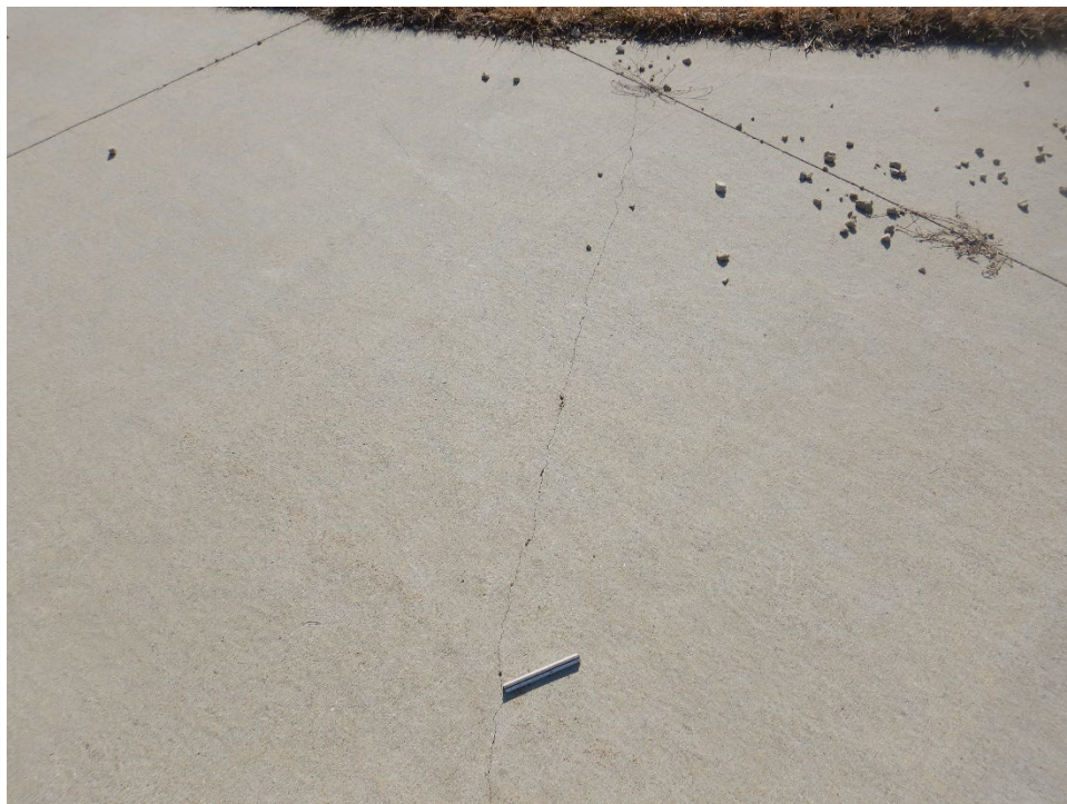
A02CR-01. LTD Cracking (Sample unit No. 02) (1).
