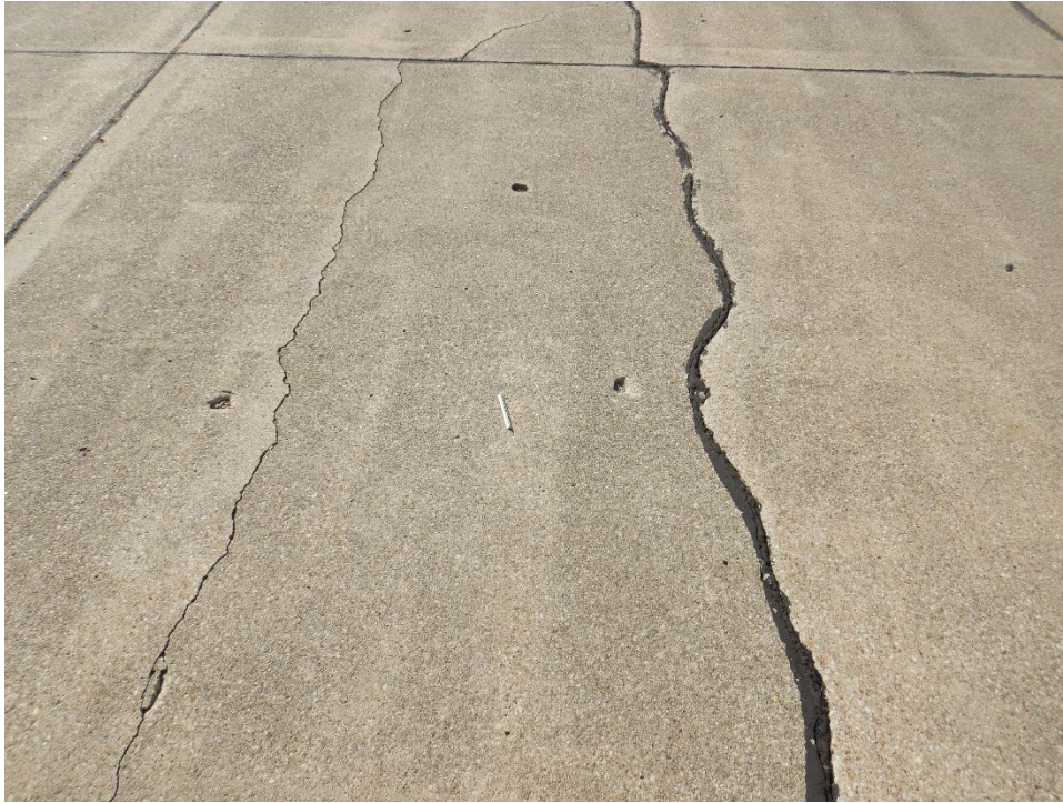
A01CR-02. LTD Cracking (Sample Unit No. 01).
