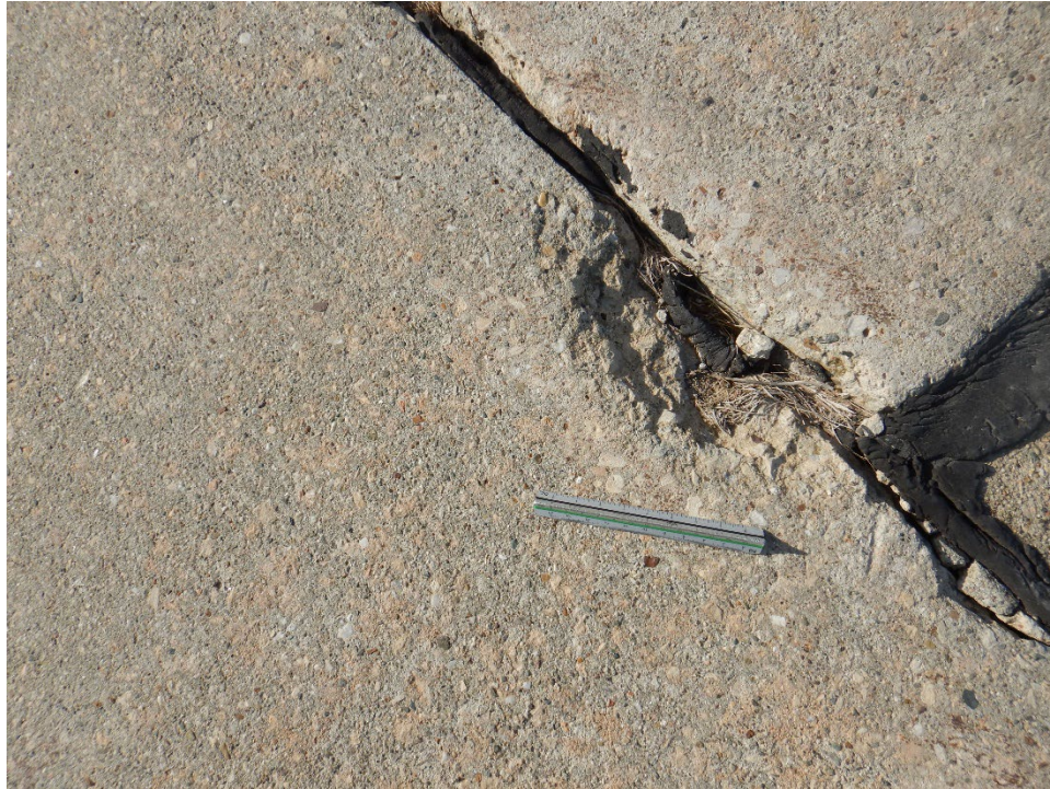
A01CR-01. Joint Spalling (Sample Unit No. 01).
