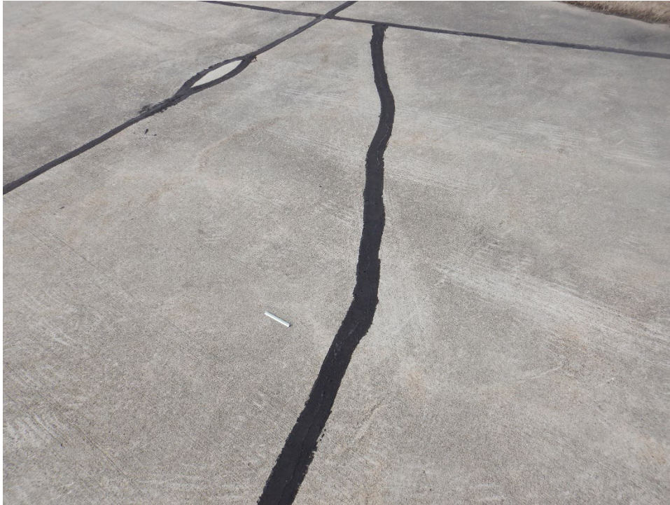
R15CR-02. LTD Cracking (Sample Unit No. 01).
