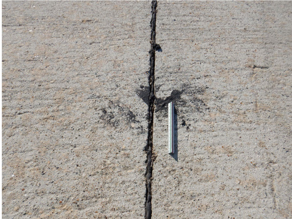
T02CR-01. Joint Seal Damage (Sample Unit No. 01).
