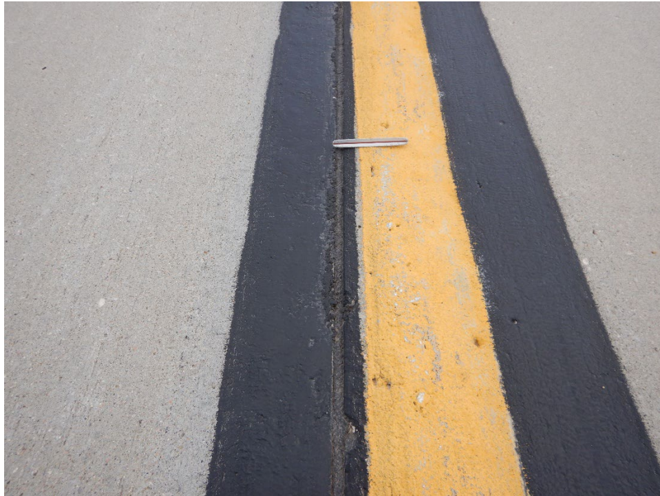
TACB-01. Faulting (Sample Unit No. 12).
