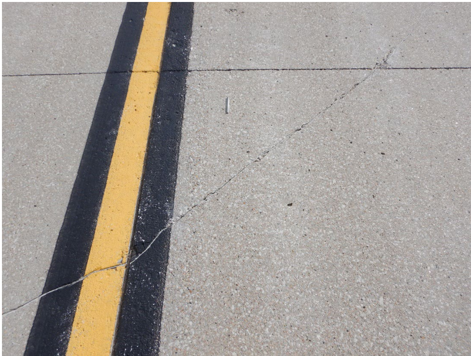
TBCB-04. Corner Break (Sample Unit No. 55).
