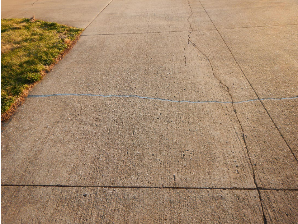
TH01CB-03. Shattered Slab (Sample Unit No. 04).
