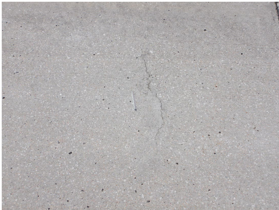
TBCB-04. Shrinkage Cracking (Sample Unit No. 19).
