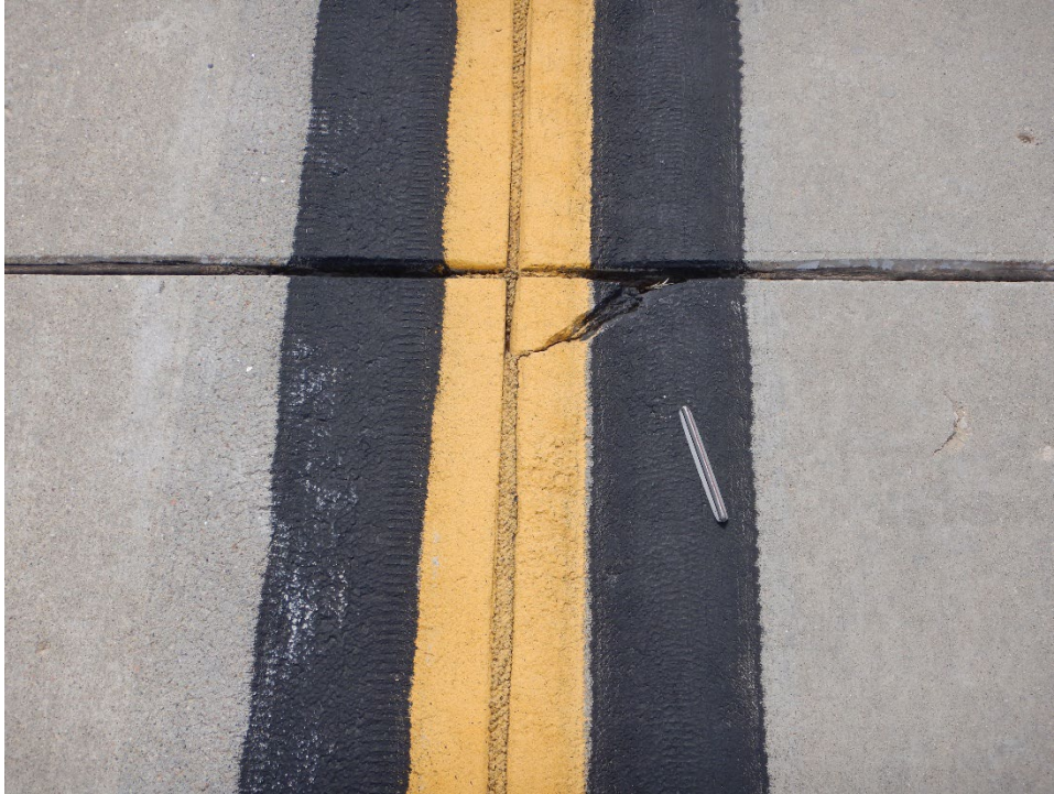
TBCB-01. Corner Spalling (Sample Unit No. 05).
