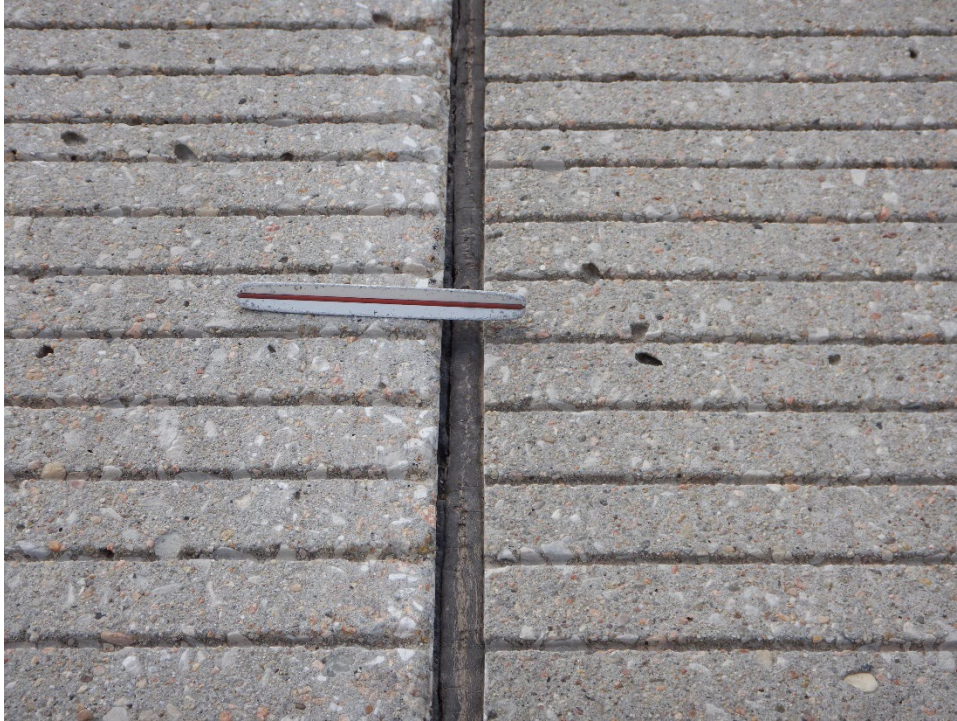
R18CB-01. Faulting (Sample Unit No. 11).
