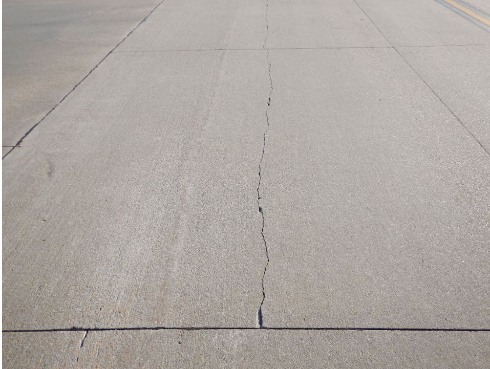
TH01CB-01. LTD Cracking (Sample Unit No. 03).
