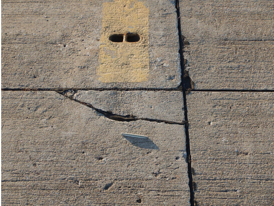
A02CB-01. Corner Spalling (Sample Unit No. 06).
