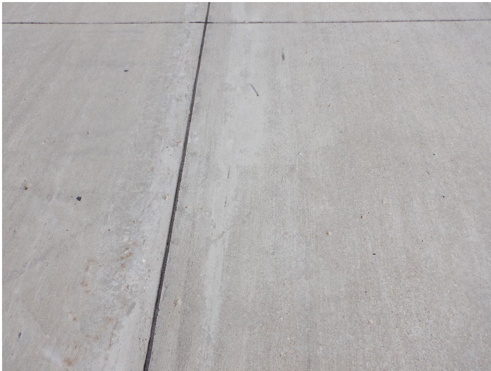
R14CB-01. LTD Cracking (Sample Unit No. 59).
