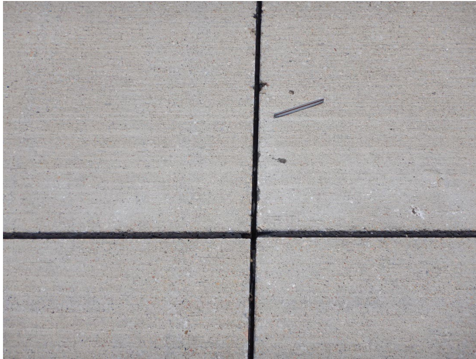
TDCB-01. Joint Seal Damage (Sample Unit No. 21).
