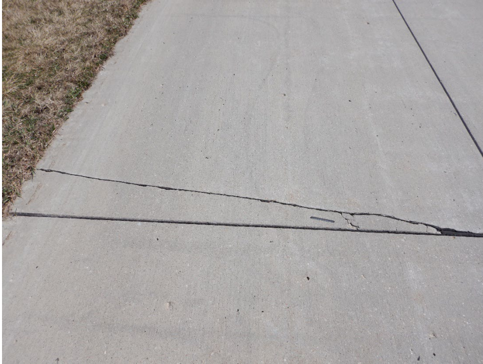
TBCB-03. LTD Cracking (Sample Unit No. 19).
