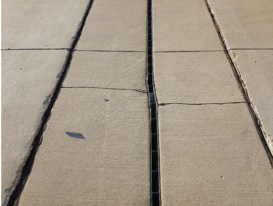
A01CB-01. LTD Cracking (Sample Unit No. 61).
