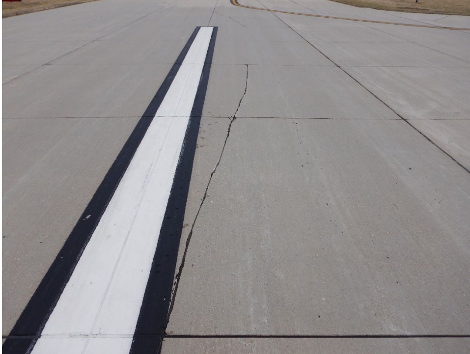
R14CB-02. LTD Cracking (Sample Unit No. 08).
