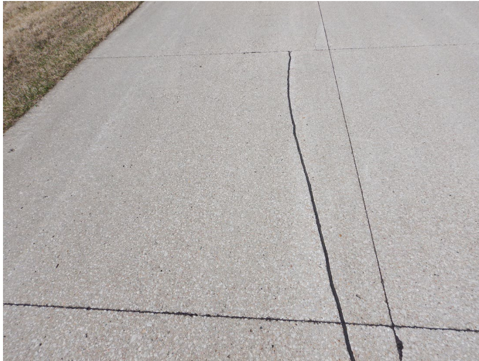
TBCB-04. LTD Cracking (Sample Unit No. 55).
