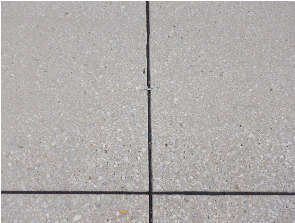
TCCB-02. Joint Seal Damage (Sample Unit No. 16).
