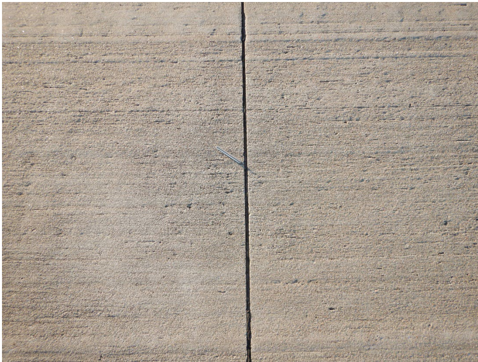
A02CB-01. Joint Seal Damage (Sample Unit No. 13).
