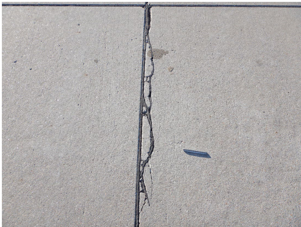
TH01CB-02. Joint Spalling (Sample Unit No. 15).
