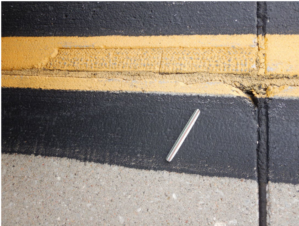
TBCB-03. Small Patching (Sample Unit No. 11).
