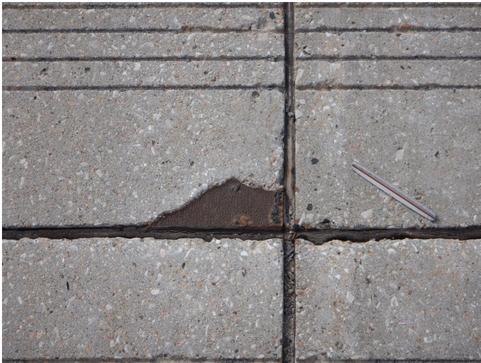
R18CB-01. Small Patching (Sample Unit No. 03).
