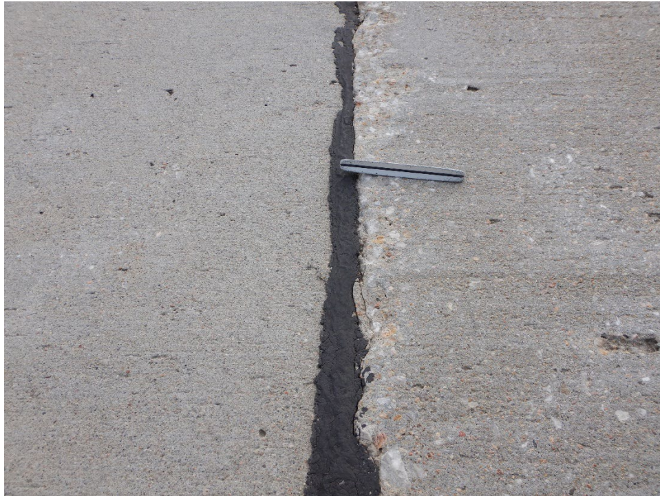
TACB-03. Faulting (Sample Unit No. 01).
