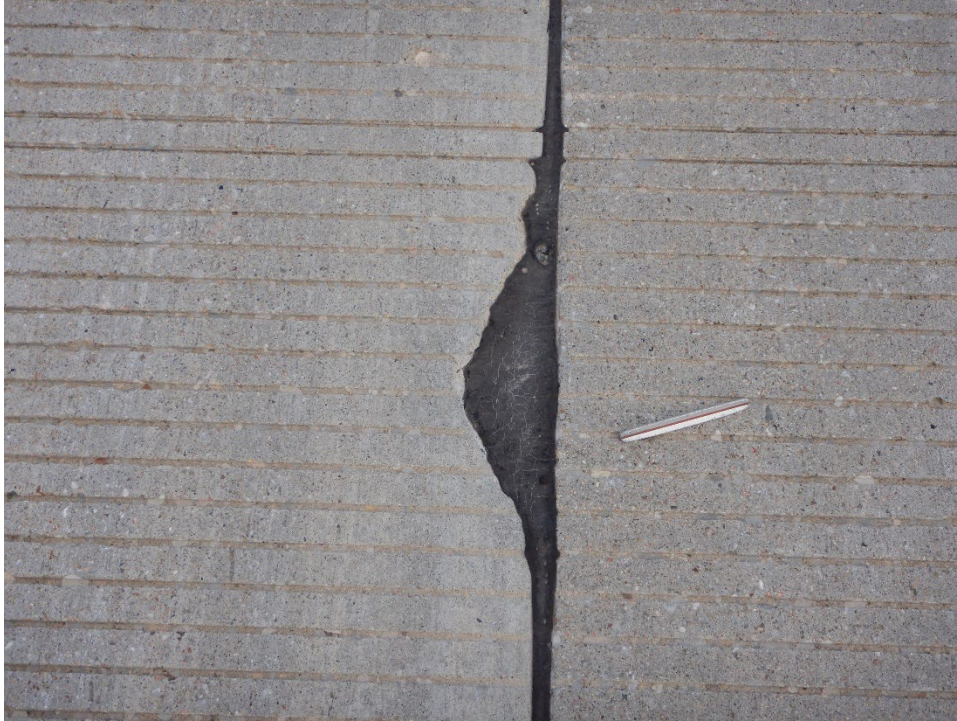
R18CB-02. Joint Spalling (Sample Unit No. 18).
