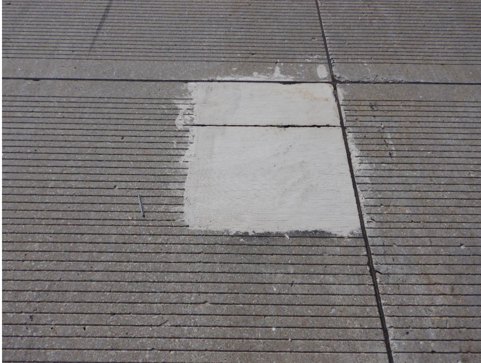
R18CB-01. Small Patching (Sample Unit No. 119).
