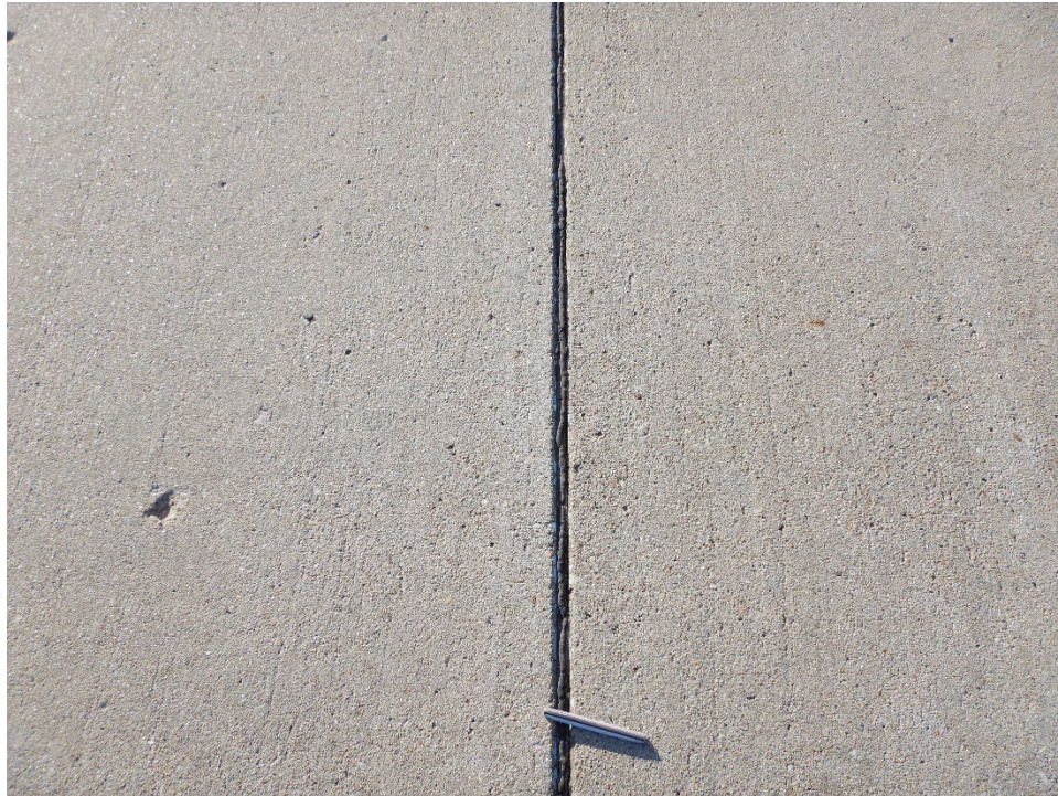
TH01CB-02. Joint Seal Damage (Sample Unit No. 15).
