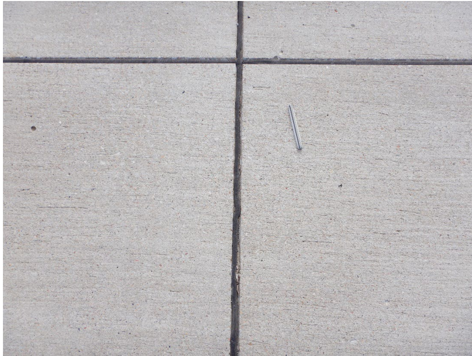
TACB-02. Joint Seal Damage (Sample Unit No. 02).
