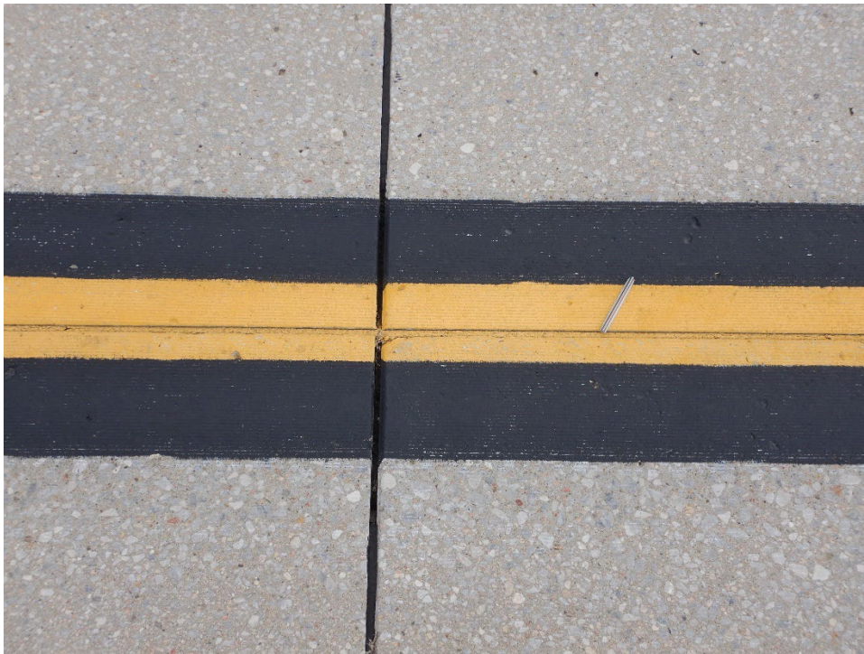
TCCB-01. Joint Seal Damage (Sample Unit No. 04).
