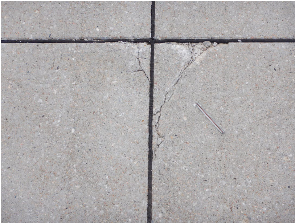
TBCB-02. Corner Spalling (Sample Unit No. 09).
