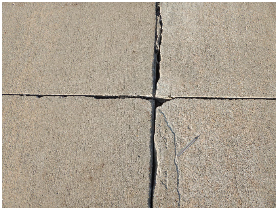
TH01CB-01. Joint Spalling (Sample Unit No. 03).
