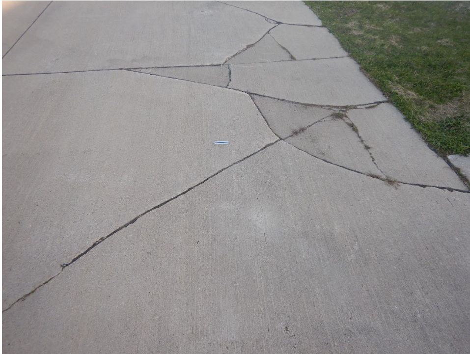
A01CO-01. Shattered Slab (Additional Sample Unit No. 004).
