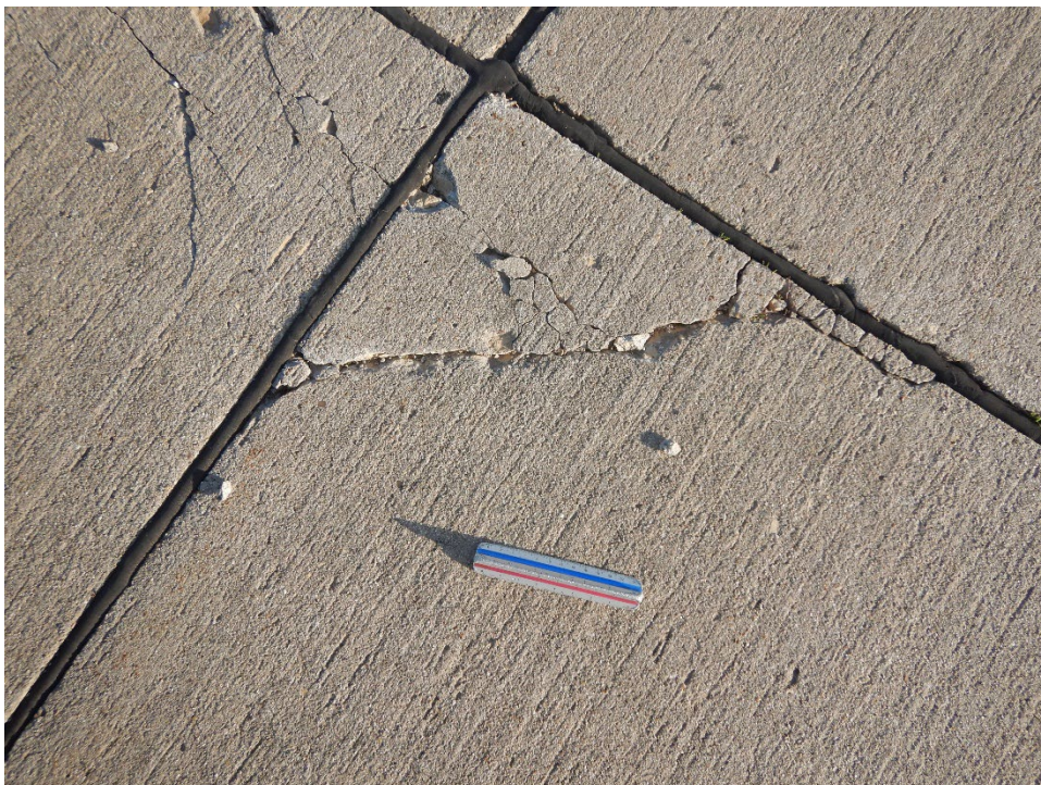
A01CO-01. Corner Spalling (Sample Unit No. 005).
