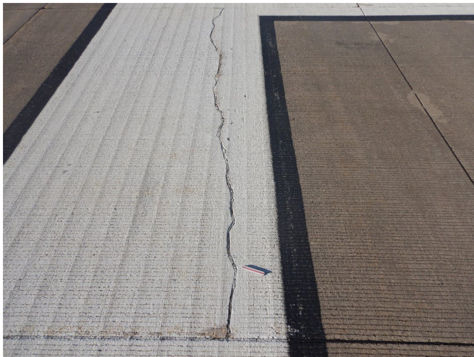
R18CO-01. LTD Cracking (Sample Unit No. 040).
