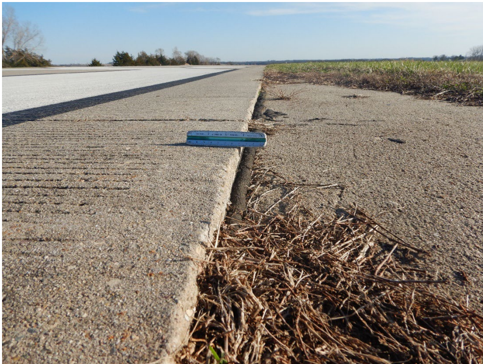
T01CO-01. Faulting (Sample Unit No. 003).
