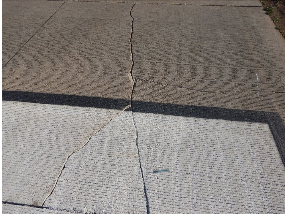
R18CO-01. Shattered Slab (Additional Sample Unit No. 005).
