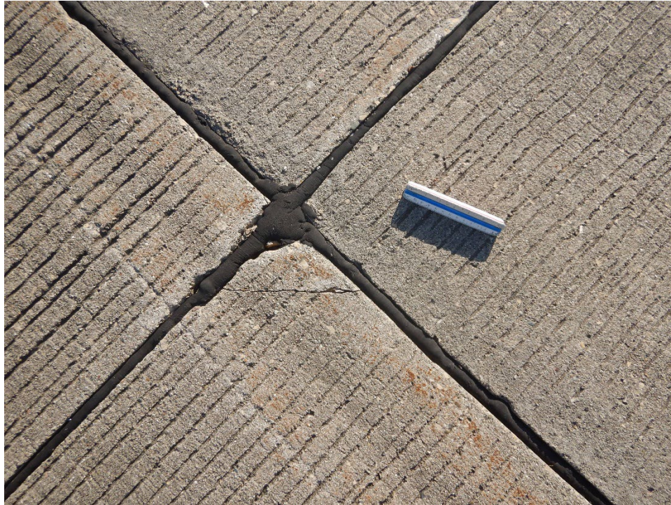
R18CO-01. Corner Spalling (Sample Unit No. 040).
