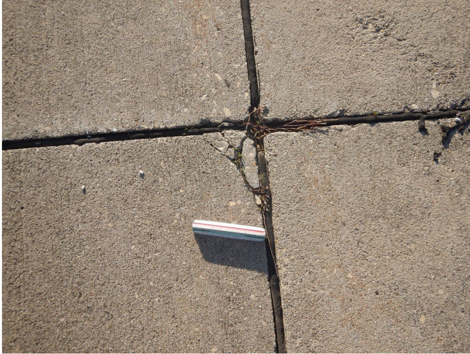
T01CO-01. Corner Spalling (Sample Unit No. 003).
