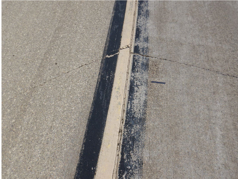
TACN-01. LTD Cracking (Sample Unit No. 01).
