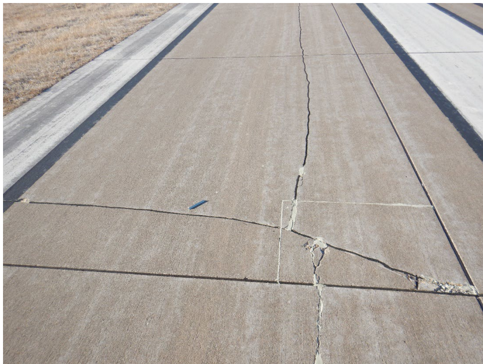
R03CN-01. Shattered Slab (Sample Unit No. 44).
