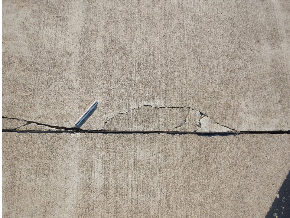
TA1CN-01. Joint Spalling (Sample Unit No. 04).
