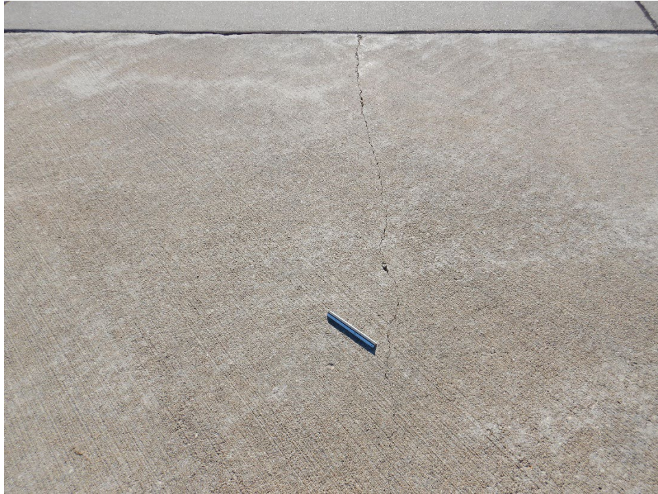
TCCN-01. LTD Cracking (Sample Unit No. 05).
