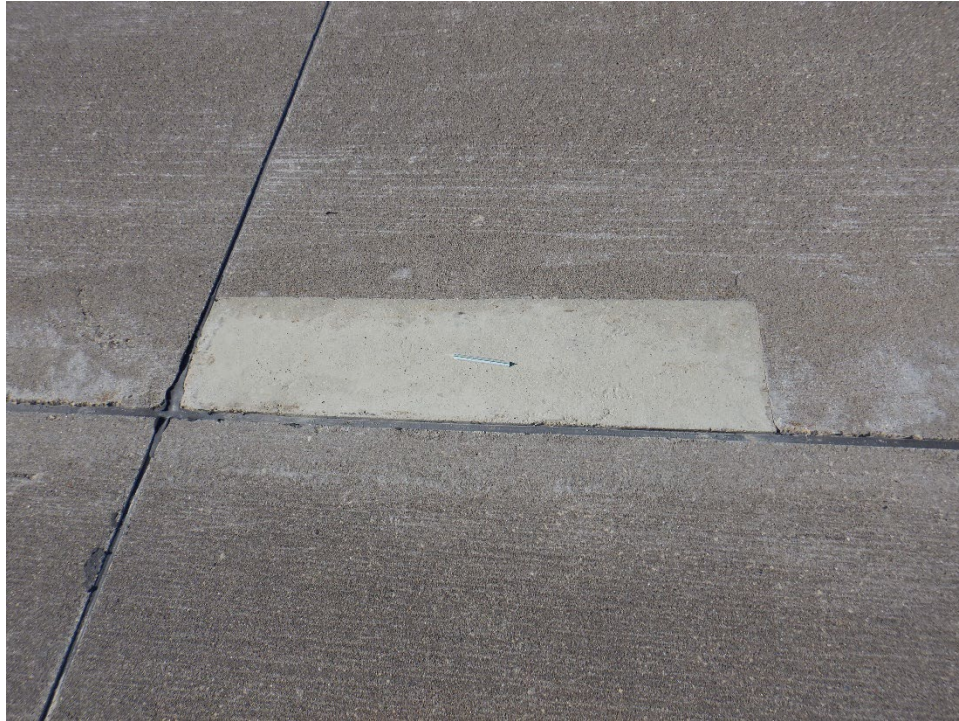
R14CN-01. Large Patching (Sample Unit No. 53).
