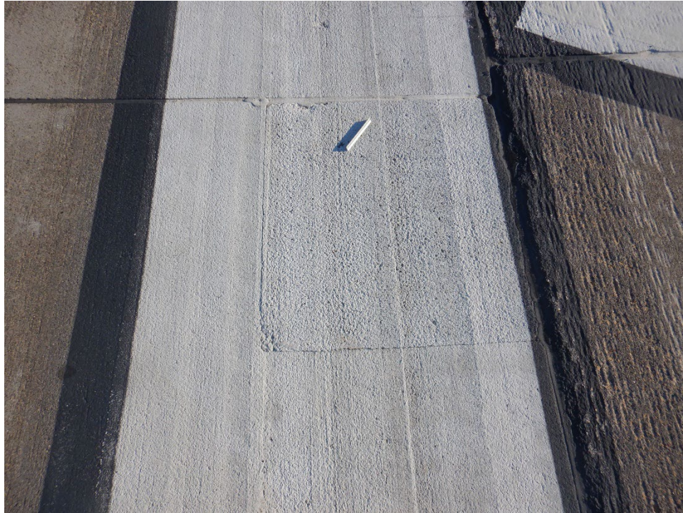
R03CN-02. Small Patching (Sample Unit No. 04).
