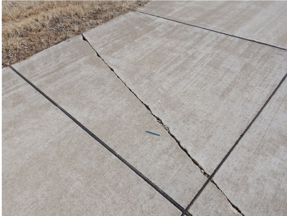
TACN-04. LTD Cracking (Sample Unit No. 05).
