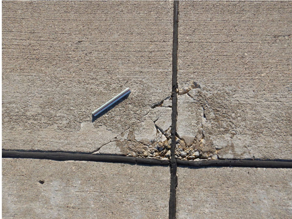
R03CN-01. Corner Spalling (Additional Sample Unit No. 110).
