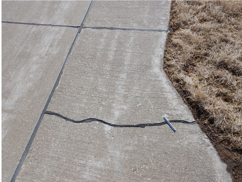
TCCN-02. LTD Cracking (Sample Unit No. 01).
