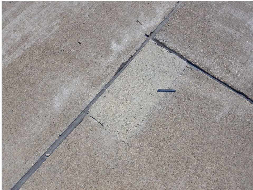
TCCN-02. Small Patching (Sample Unit No. 01).
