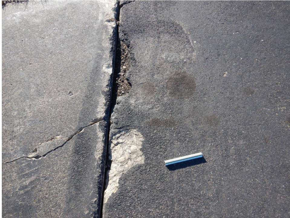
A02CN-01. Joint Spalling (Sample Unit No. 01).
