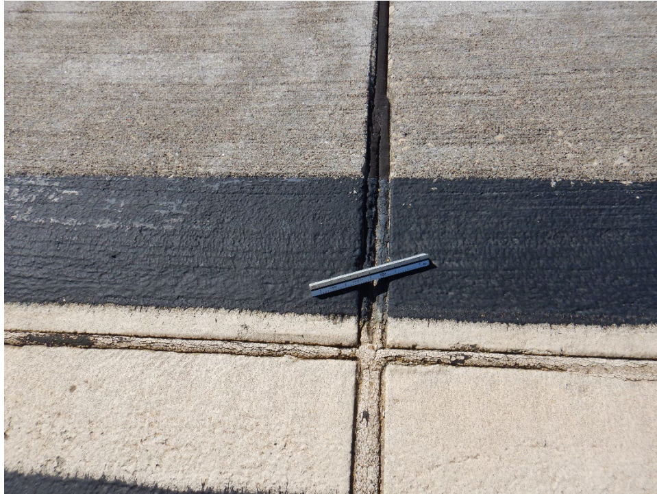
TBCN-02. Joint Seal Damage (Sample Unit No. 01).
