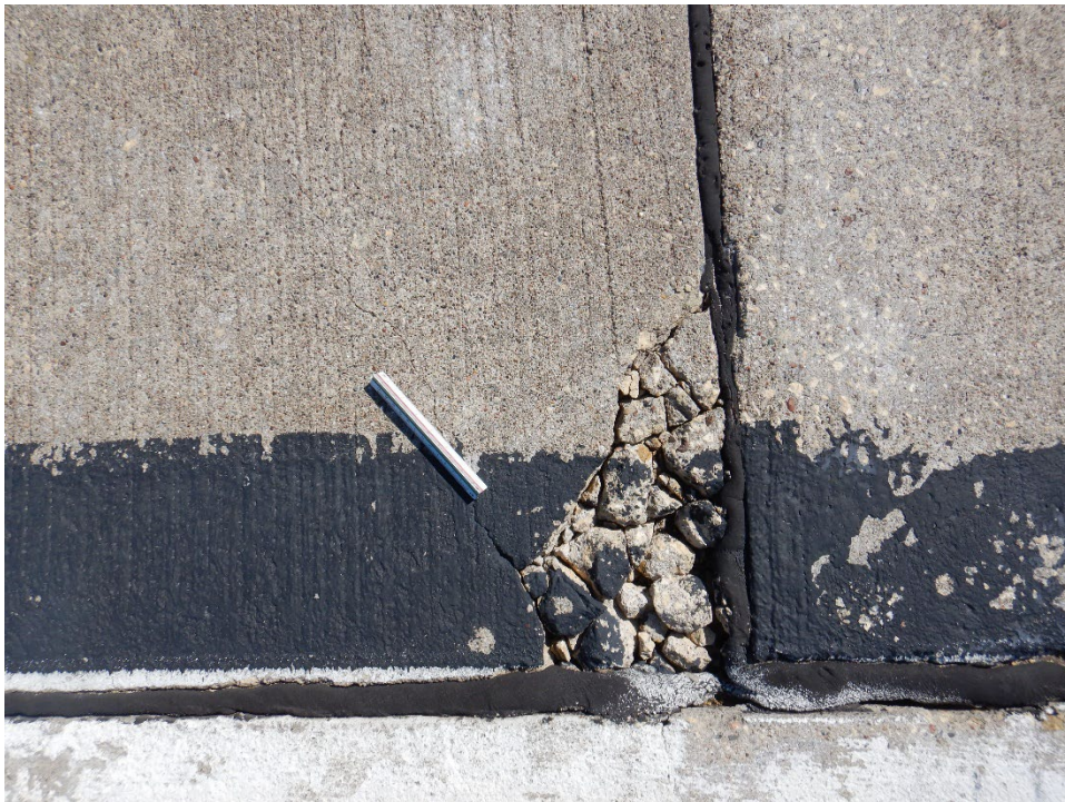
TACN-01. Corner Spalling (Sample Unit No. 01).
