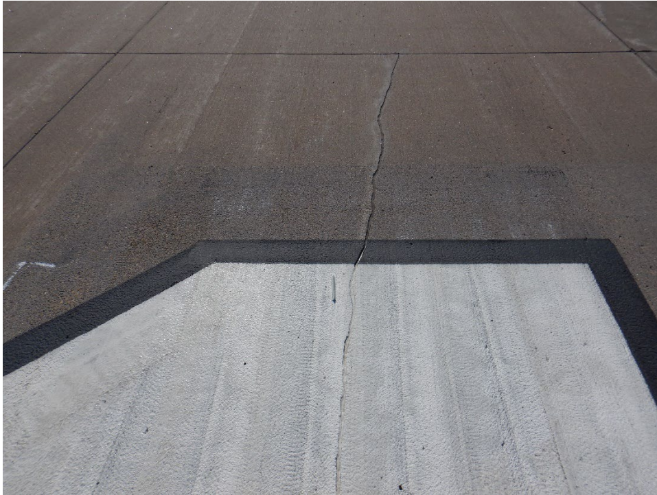
R14CN-01. LTD Cracking (Sample Unit No. 06).
