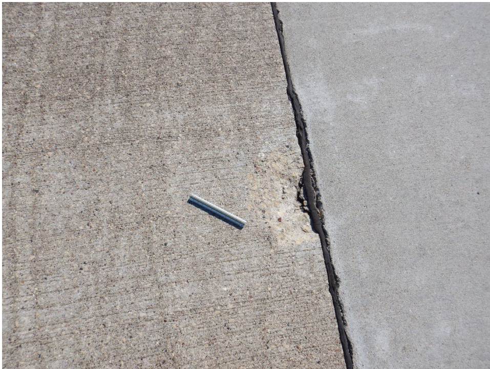
TACN-03. Joint Spalling (Sample Unit No. 42).
