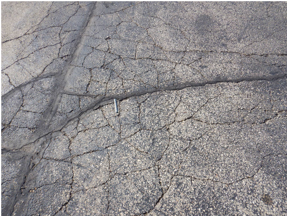
A01CN-03. Alligator Cracking (Sample Unit No. 01).
