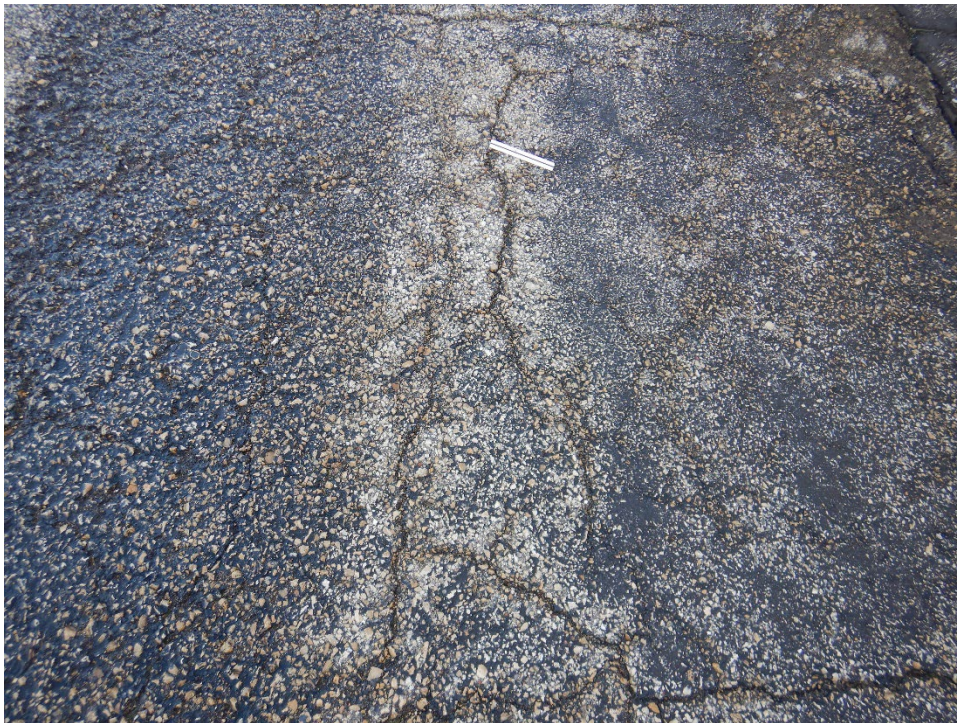
T04CN-01. L&T Cracking (Sample Unit No. 01).
