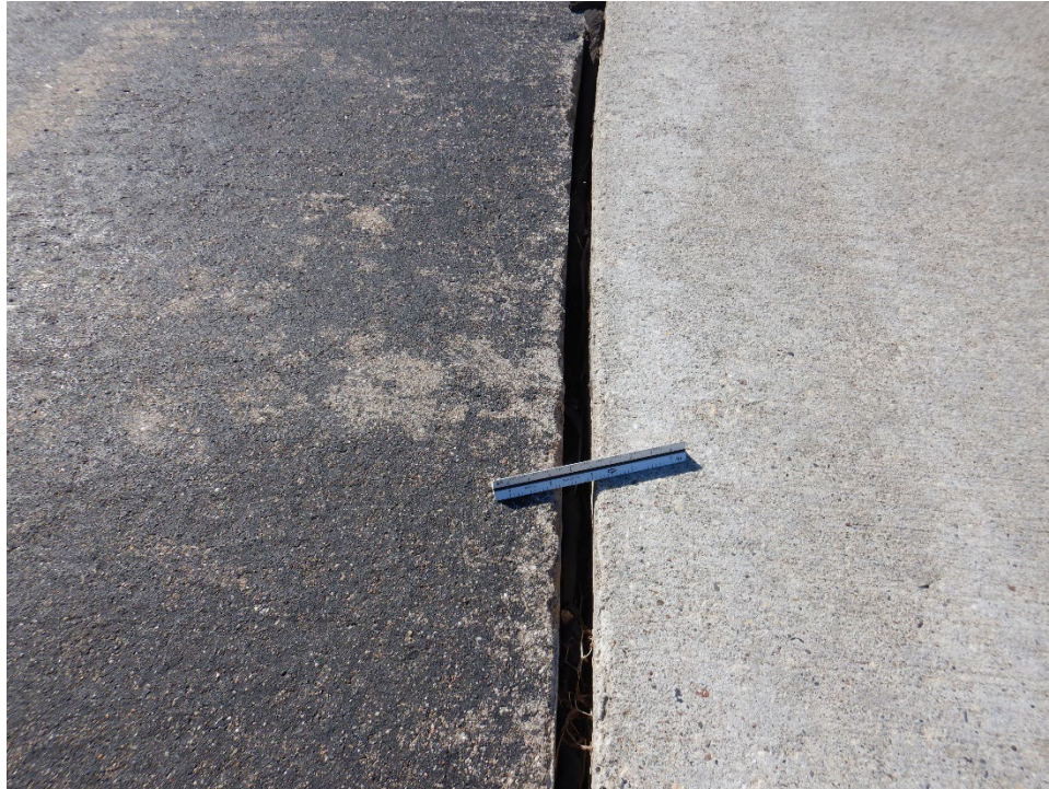
A01CN-01. Joint Seal Damage (Sample Unit No. 08).
