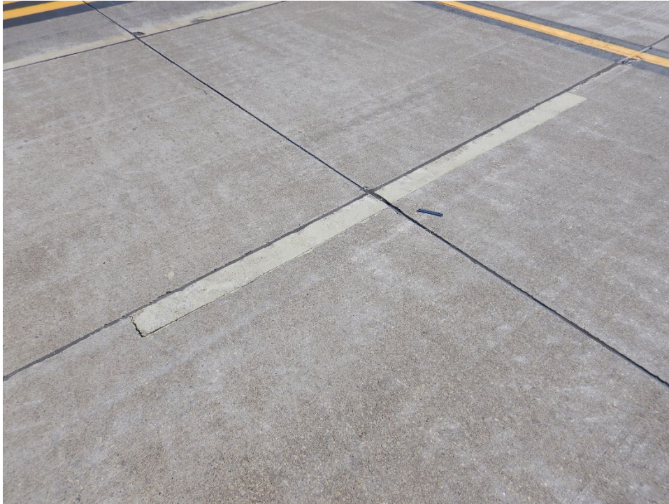
T07CN-01. Small Patching (Sample Unit No. 04).
