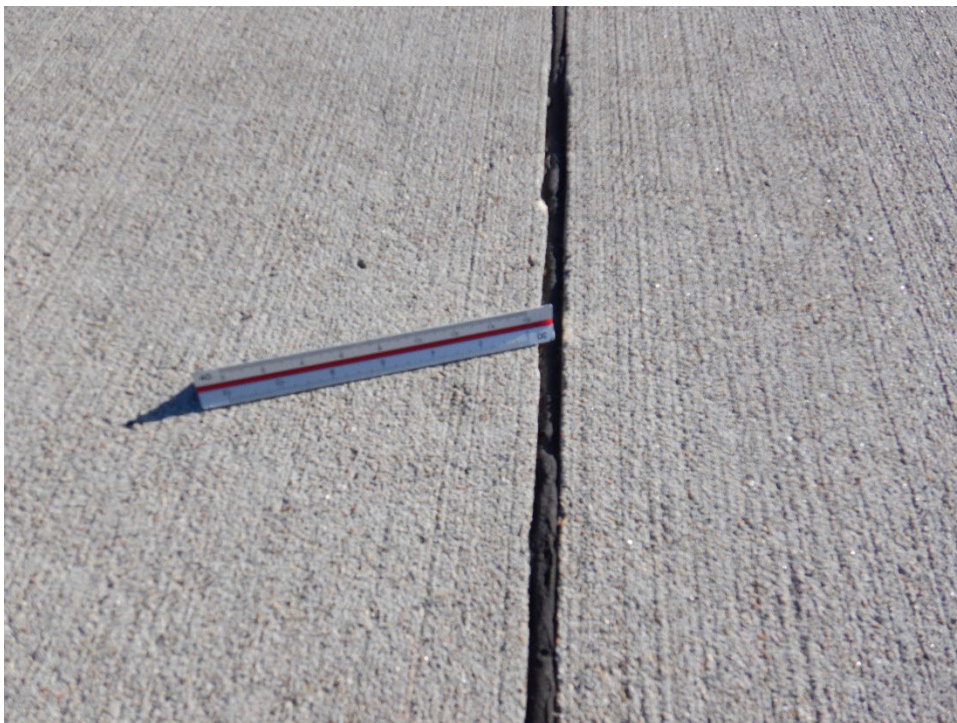
A02CN-02. Joint Seal Damage (Sample Unit No. 17).
