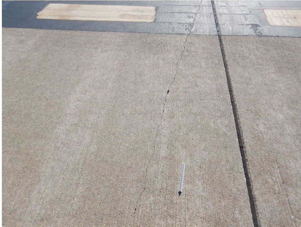
TA1CN-02. LTD Cracking (Sample Unit No. 05).
