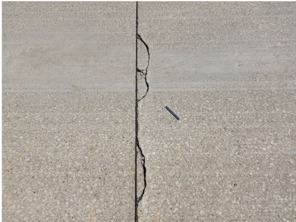
TACN-02. Joint Spalling (Sample Unit No. 10).
