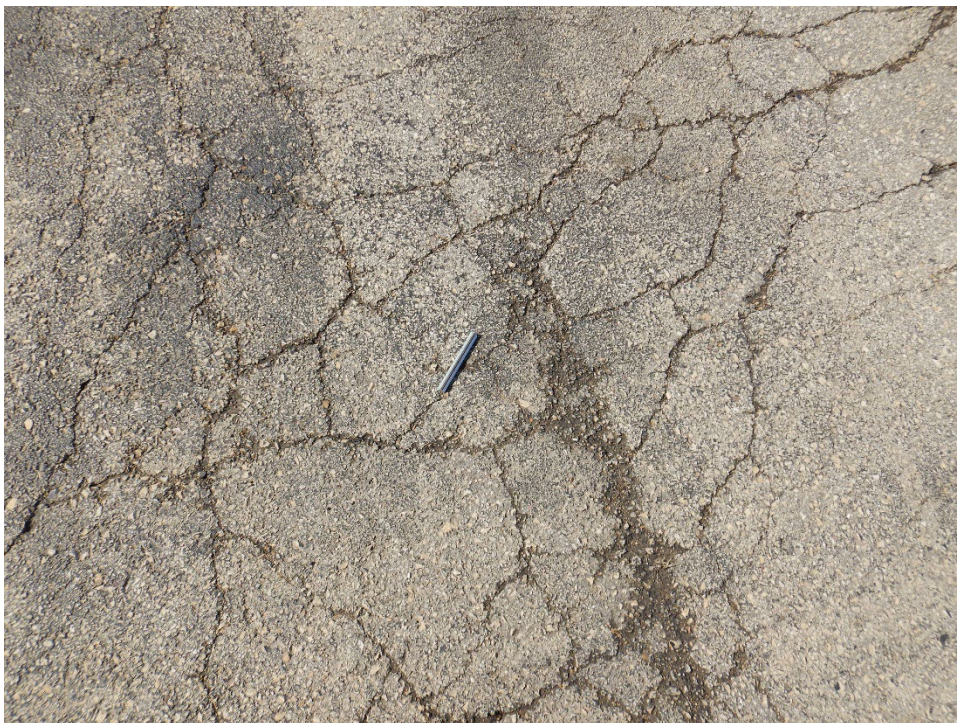
TH01CN-03. Alligator Cracking (Sample Unit No. 01).
