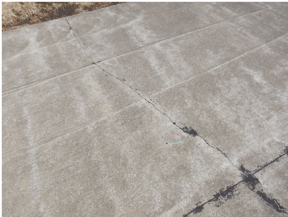
TH01CN-01. LTD Cracking (Sample Unit No. 04).
