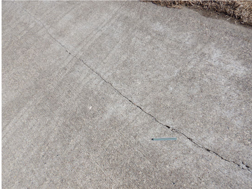
TACN-03. LTD Cracking (Sample Unit No. 42).
