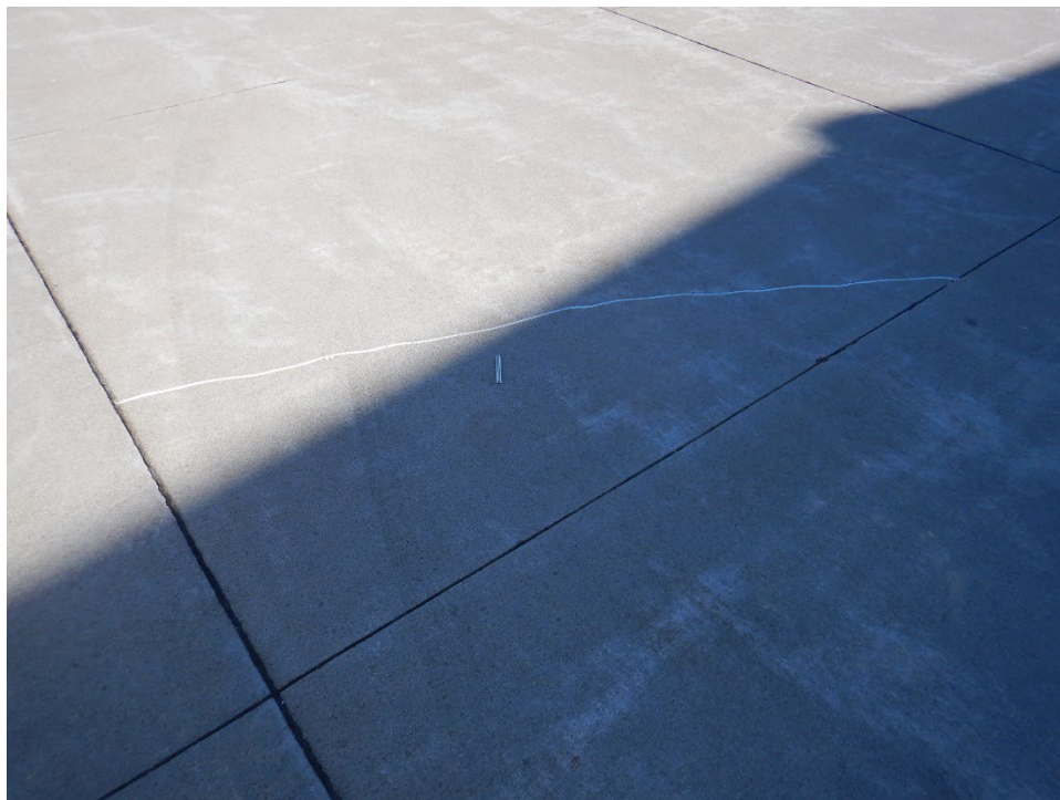
A01CN-02. LTD Cracking (Sample Unit No. 01).
