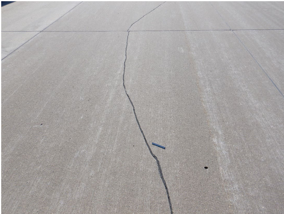
R14CN-01. LTD Cracking (Sample Unit No. 26).
