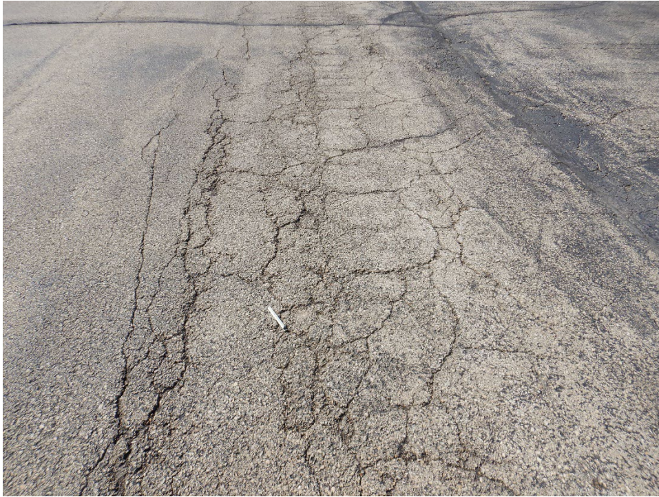
T04CN-01. Alligator Cracking (Sample Unit No. 02).
