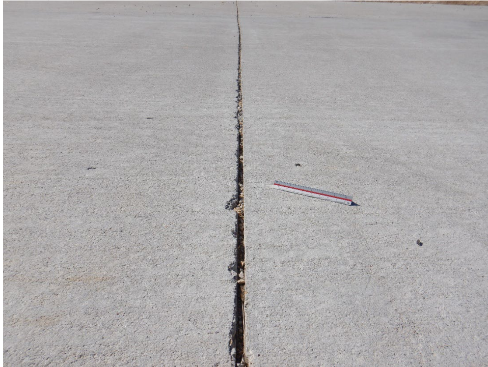
T04CN-02. Joint Seal Damage (Sample Unit No. 07).
