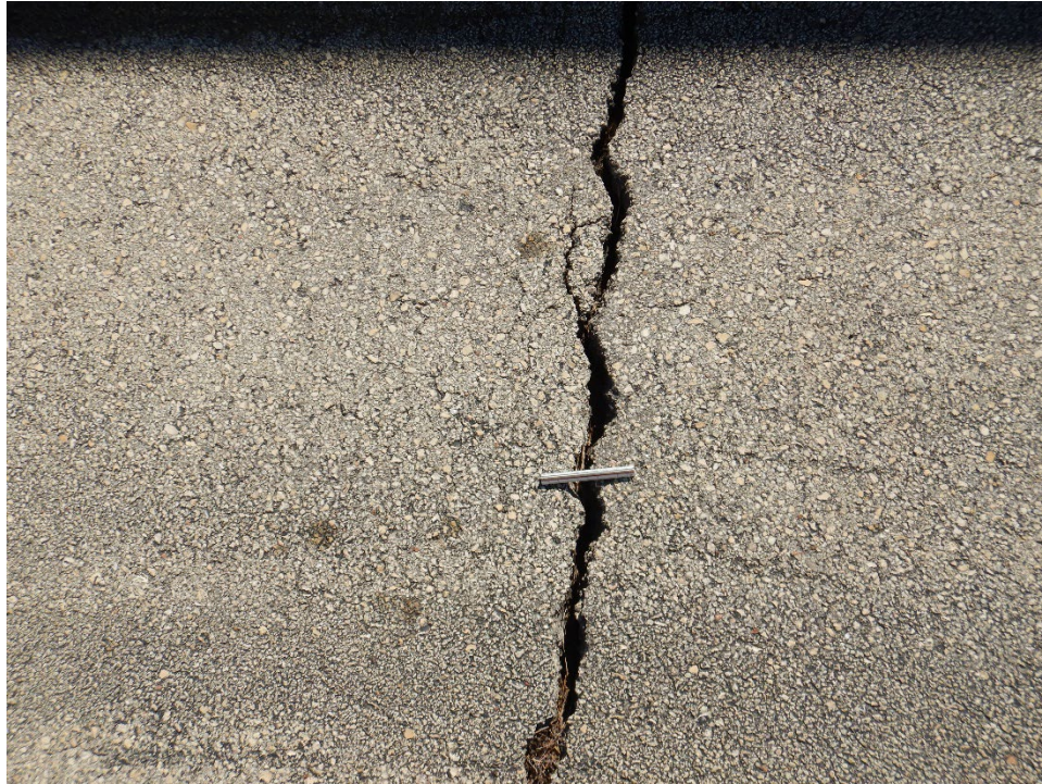
TH01CN-03. L&T Cracking (Sample Unit No. 01).
