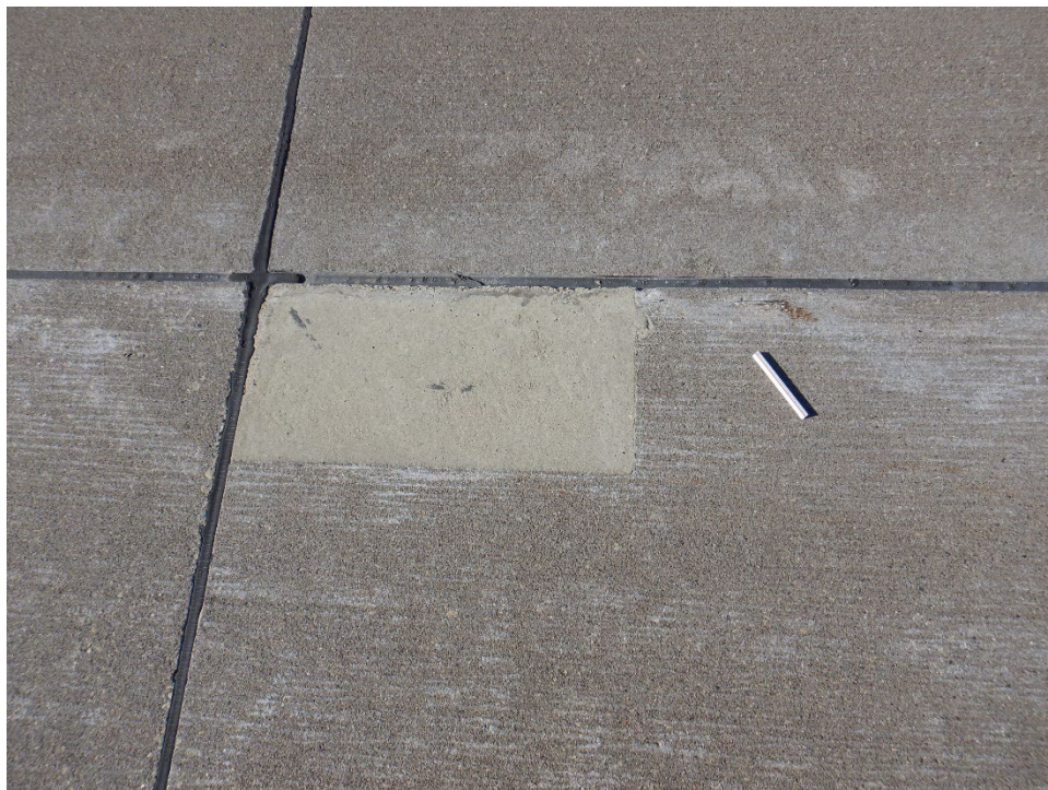
R14CN-01. Small Patching (Sample Unit No. 06).
