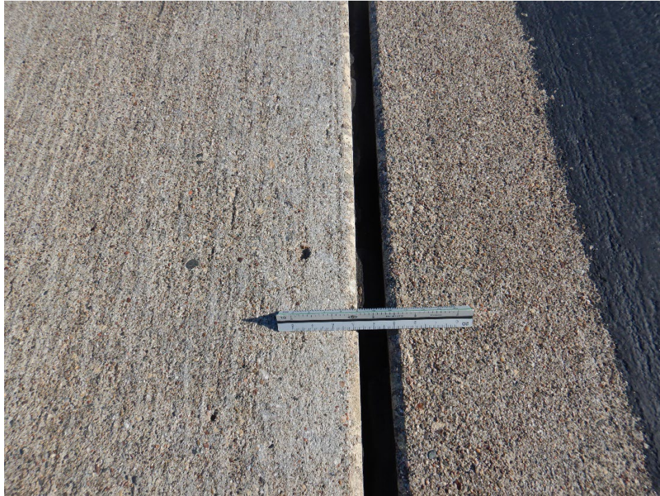
R03CN-01. Joint Seal Damage (Sample Unit No. 153).
