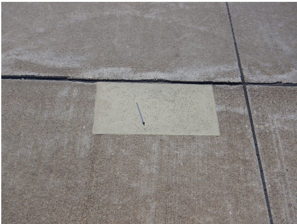
T02CN-01. Small Patching (Sample Unit No. 07).
