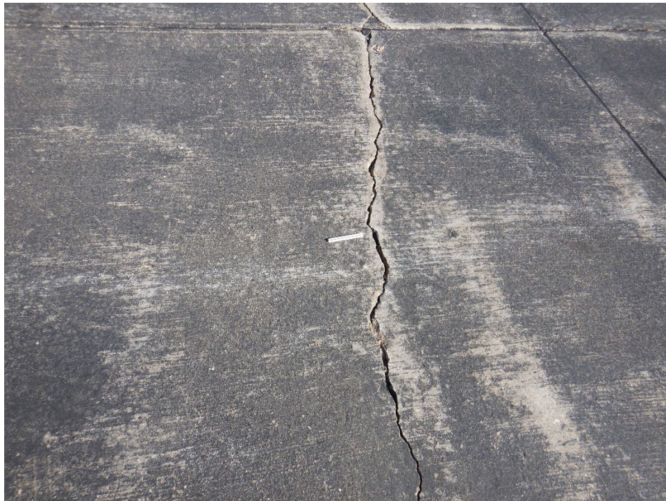
A01CN-01. LTD Cracking (Sample Unit No. 05).
