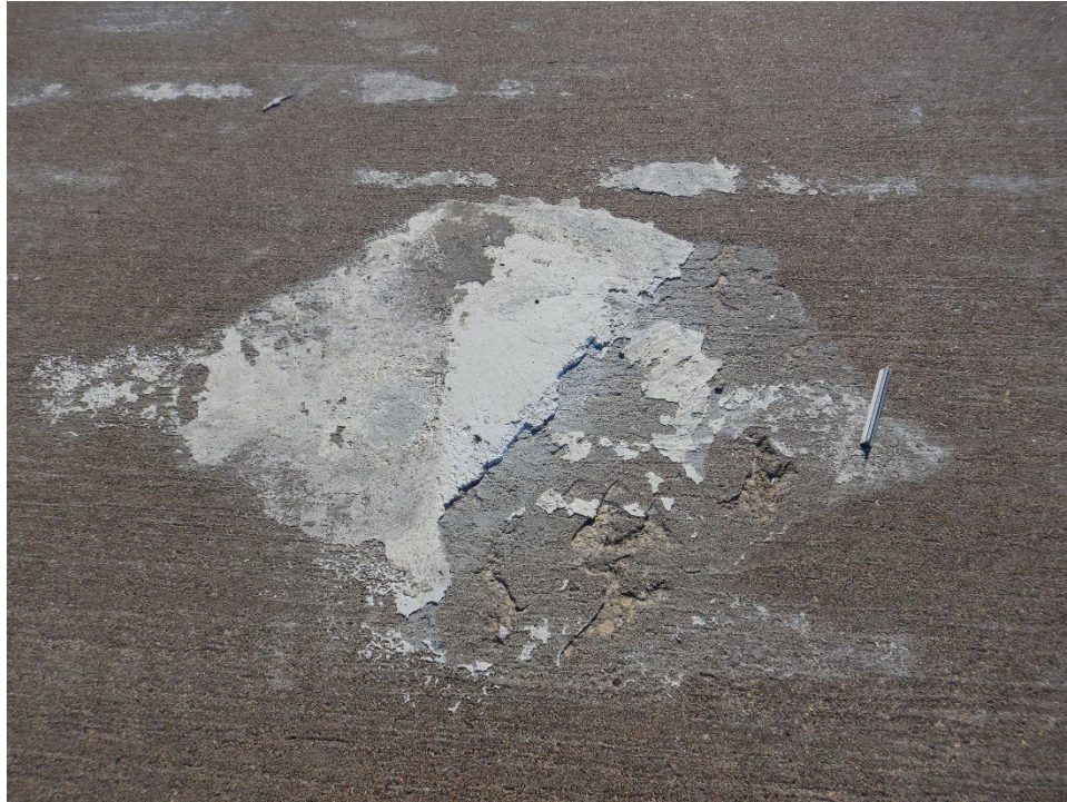
R03CN-01. Scaling (Additional Sample Unit No. 110).
