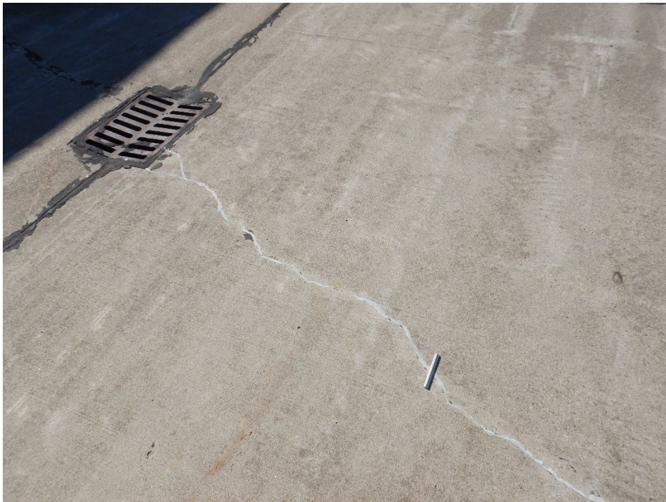
TH01CN-02. LTD Cracking (Sample Unit No. 01).
