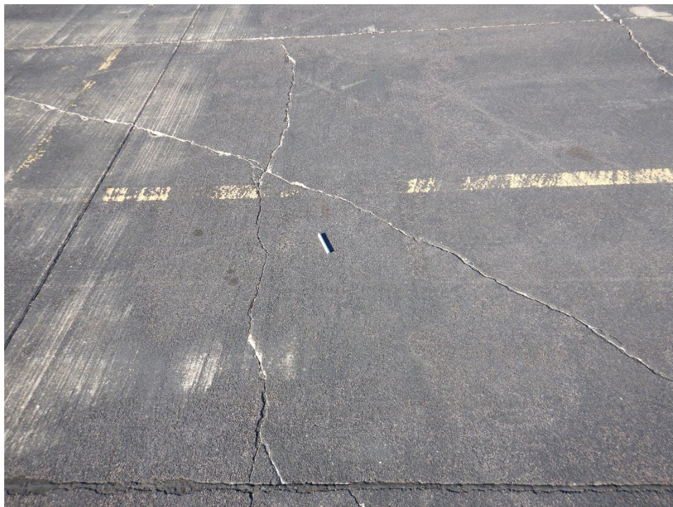
A02CN-01. Shattered Slab (Sample Unit No. 01).
