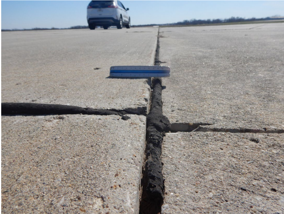
R13CD-01. Faulting (Sample Unit No. 01).
