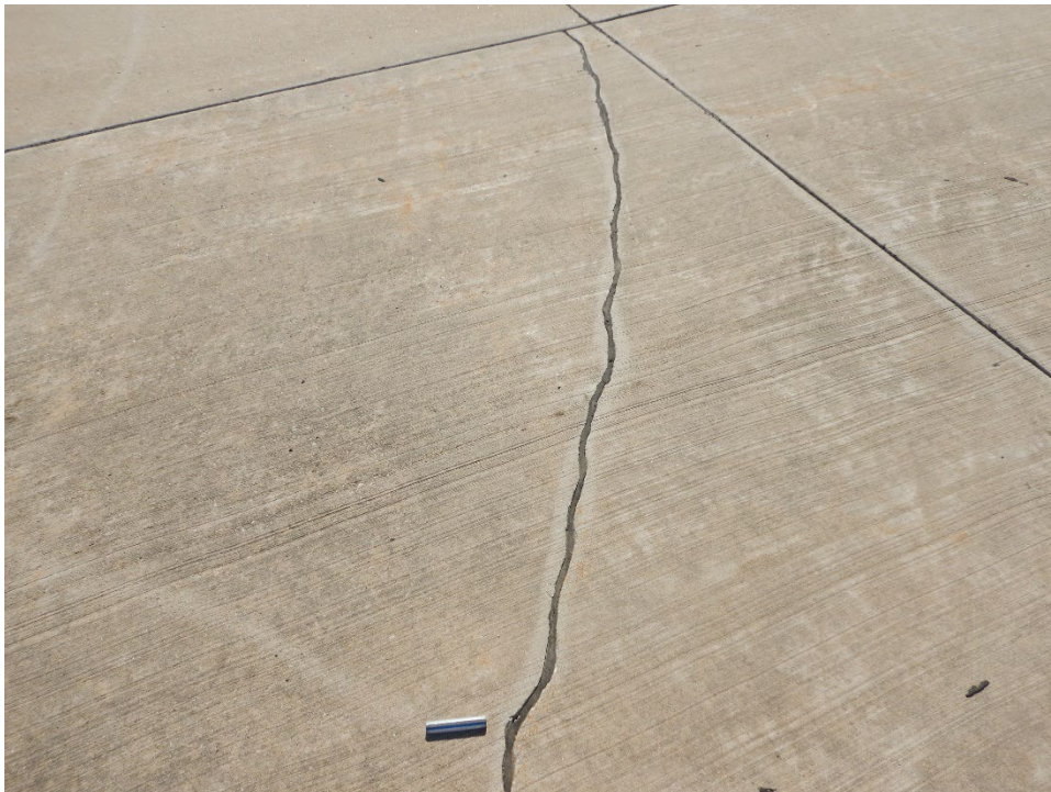
T01CD-01. LTD Cracking (Sample Unit No. 07).
