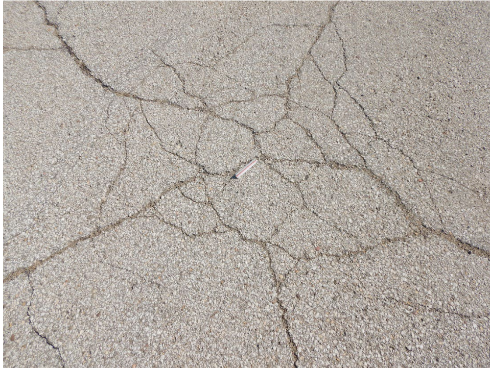
TH01CD-01. Alligator Cracking (Sample Unit No. 01).
