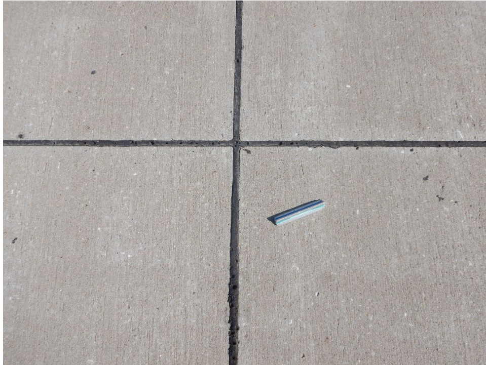
T03CD-01. Joint Seal Damage (Sample Unit No. 02).
