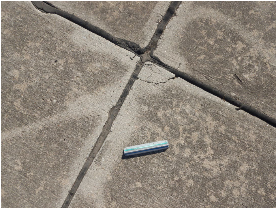
R13CD-01. Corner Spalling (Sample Unit No. 01).
