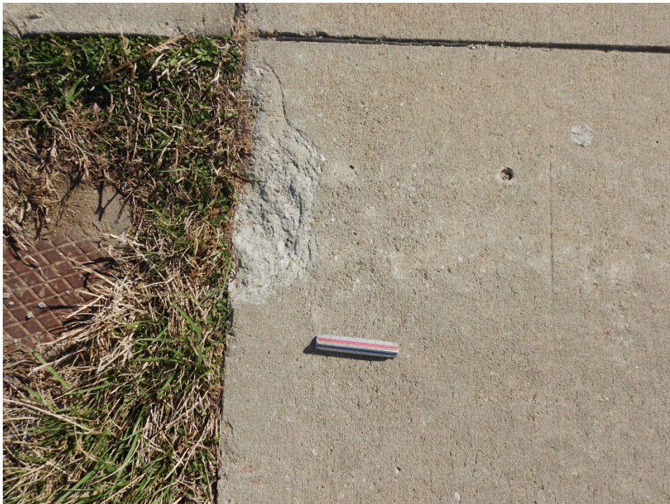
TH01CD-02. Joint Spalling (Sample Unit No. 05).
