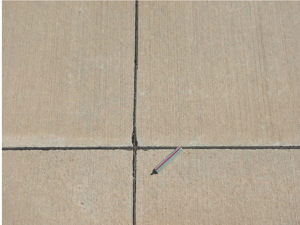
TH01CD-03. Joint Seal Damage (Sample Unit No. 03).
