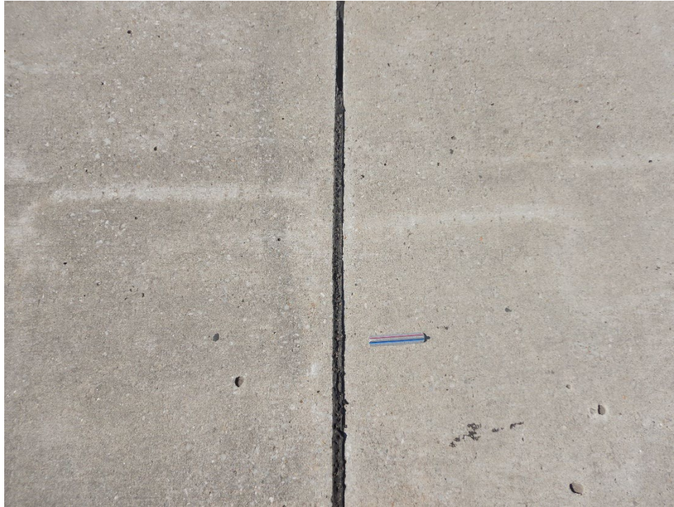
T02CD-01. Joint Seal Damage (Sample Unit No. 06).
