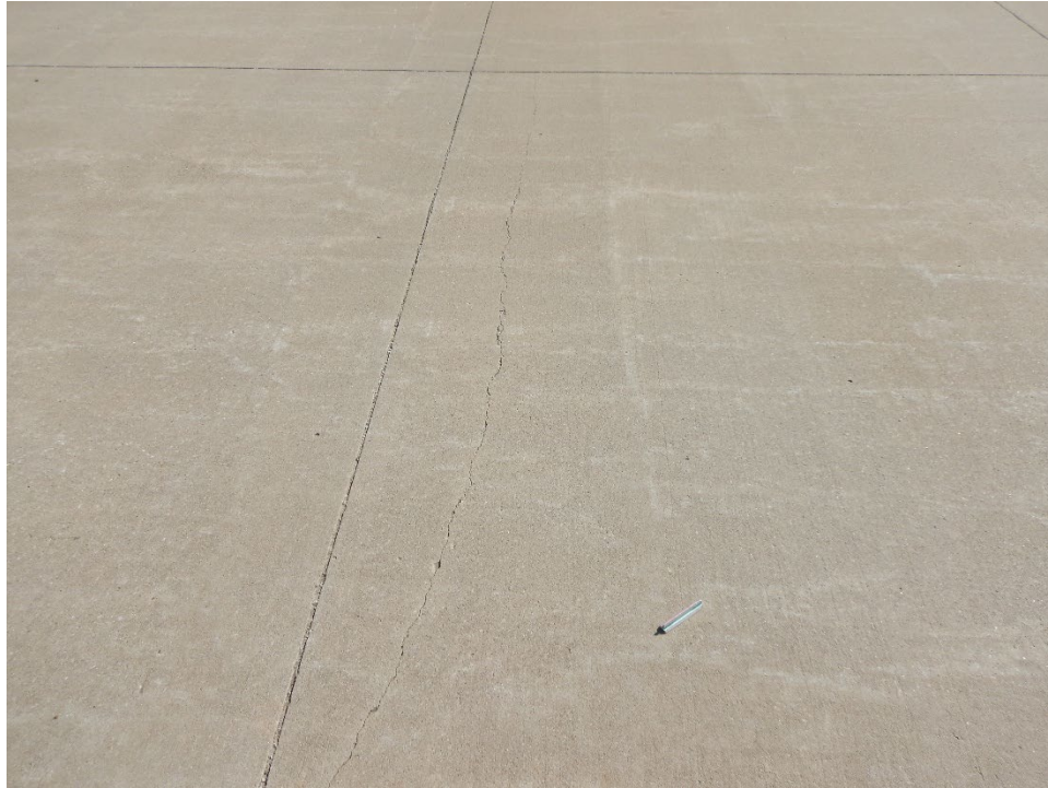
TH01CD-02. LTD Cracking (Sample Unit No. 06).
