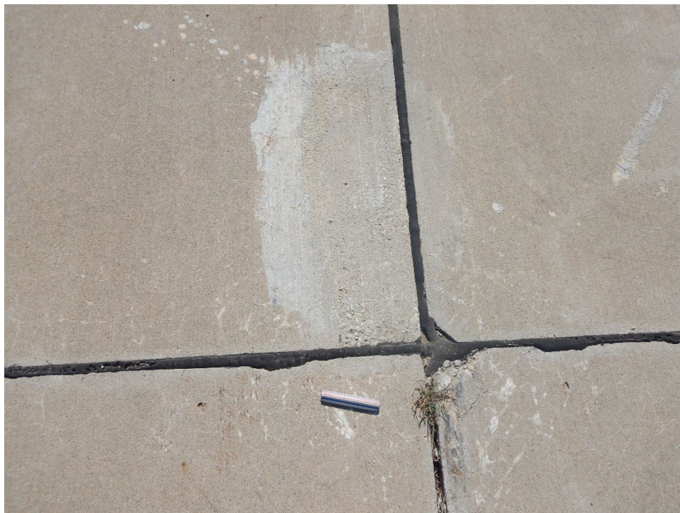
R02CD-02. Small Patching (Sample Unit No. 07).
