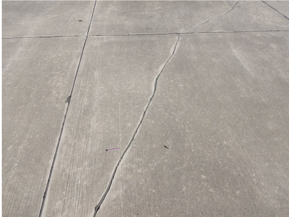
R13CD-02. LTD Cracking (Sample Unit No. 02).
