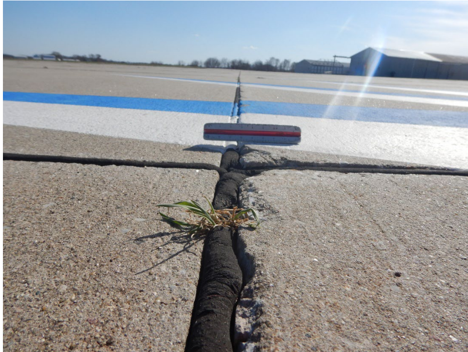
A01CD-01. Faulting (Sample Unit No. 13).
