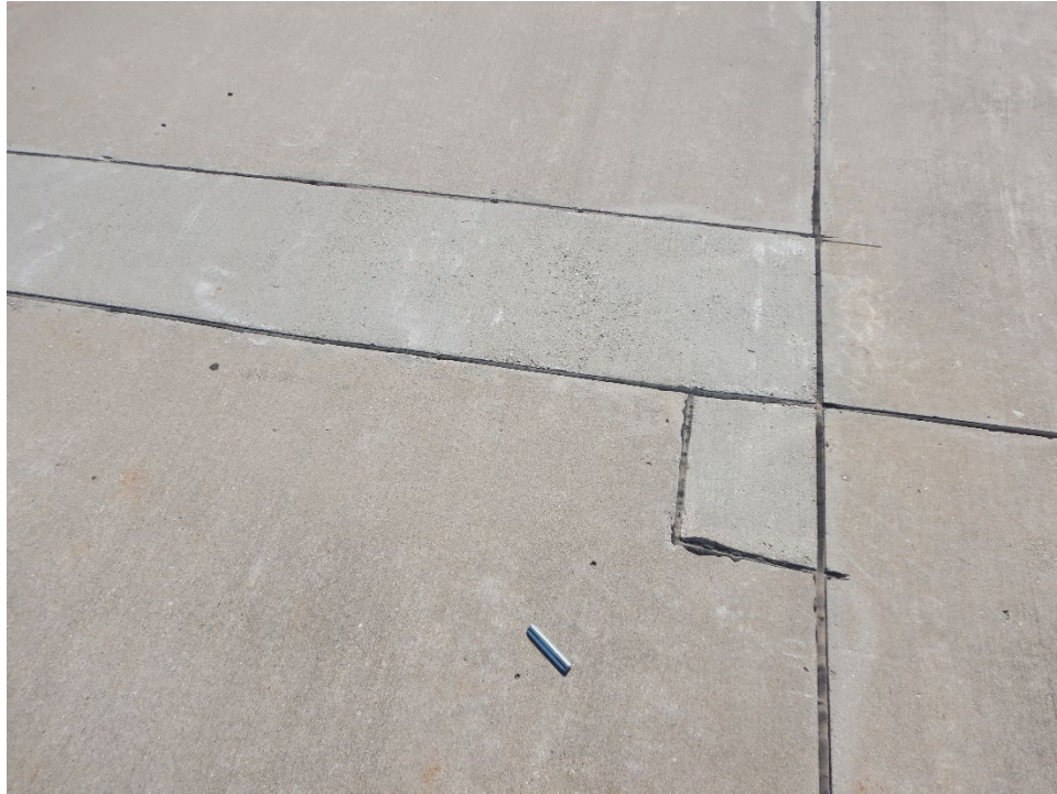
R02CD-01. Small Patching (Sample Unit No. 80).
