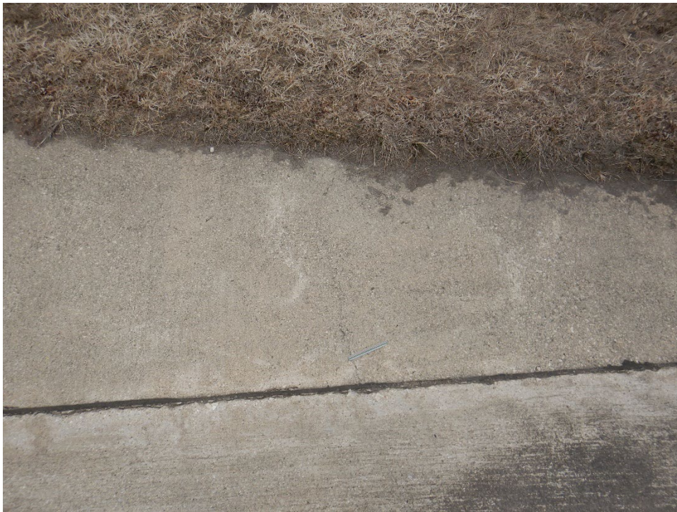
T01CK-01. LTD Cracking (Sample Unit No. 02).
