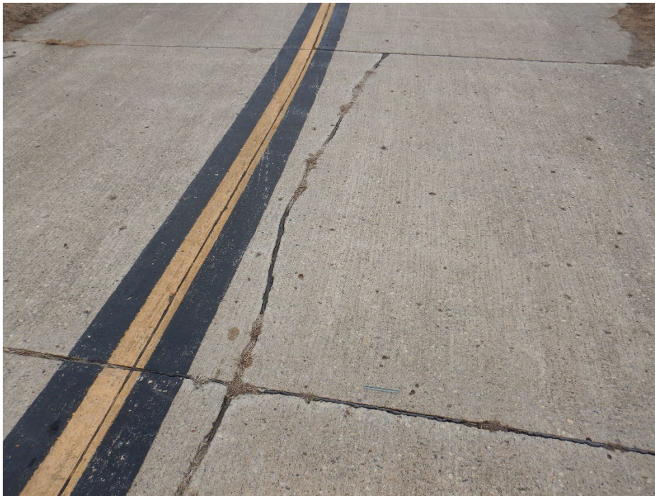
TH02CK-02. LTD Cracking (Sample Unit No. 01).
