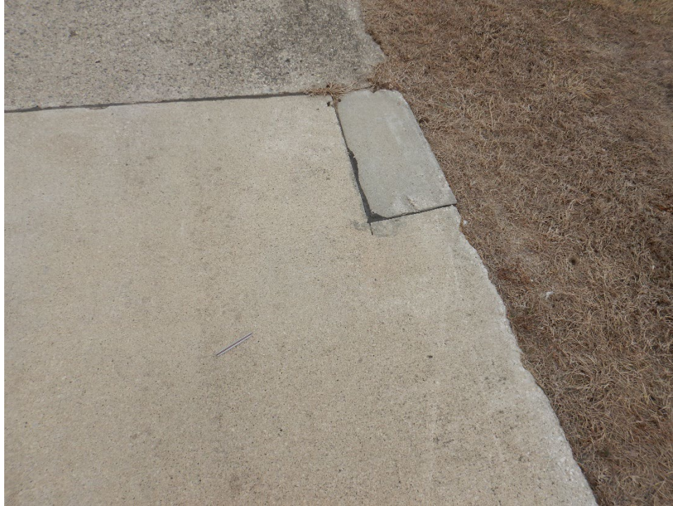
TH01CK-01. Small Patching (Sample Unit No. 01).
