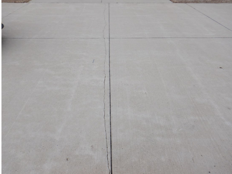
TH02CK-03. Joint Spalling (Sample Unit No. 02).
