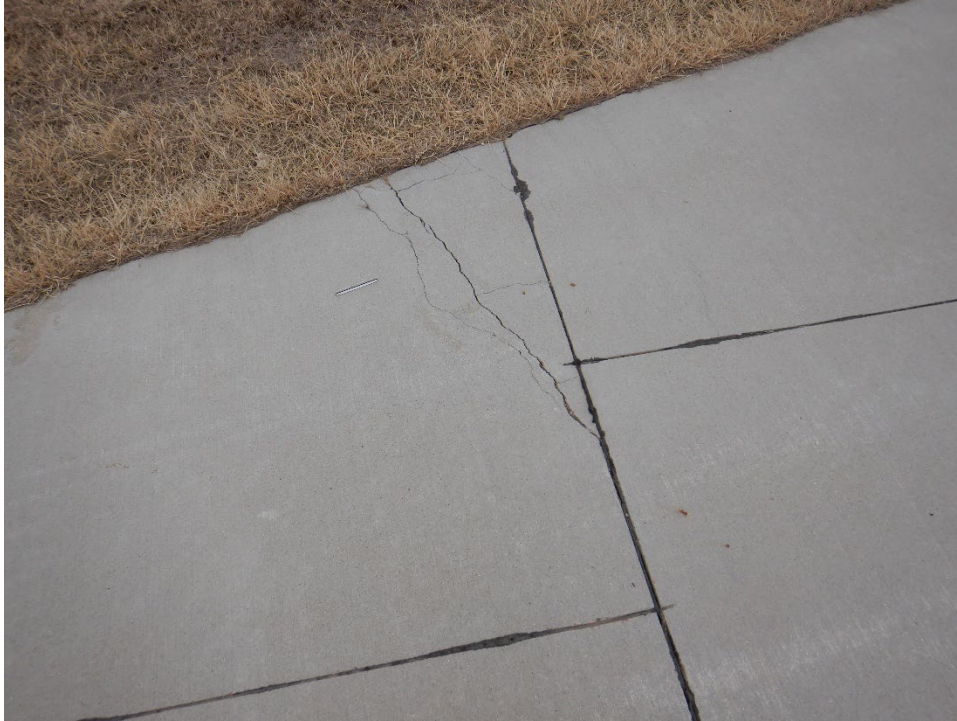
T02CK-01. Corner Break (Additional Sample Unit No. 04).
