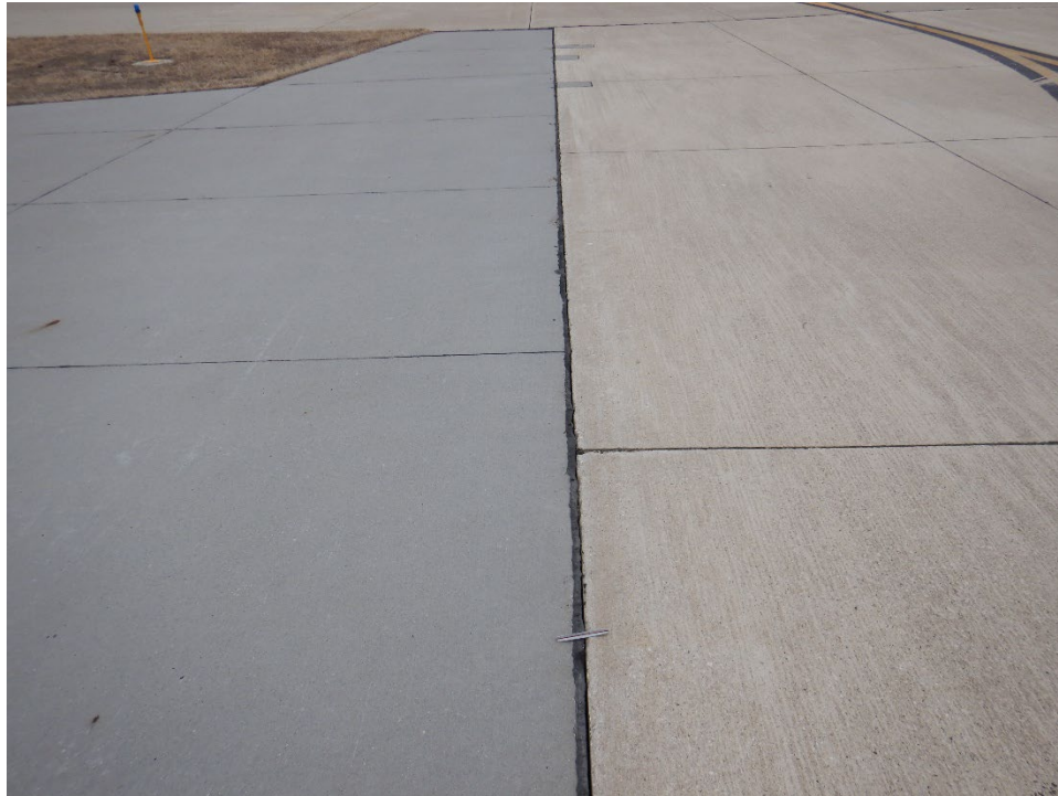
T02CK-01. Faulting (Additional Sample Unit No. 02).
