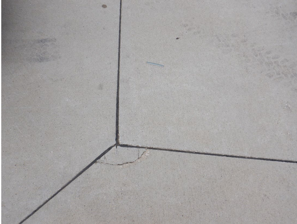
TH02CK-03. Corner Spalling (Sample Unit No. 04).
