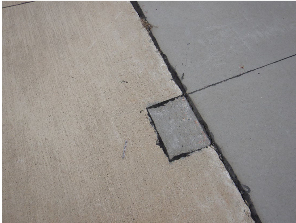
T01CK-01. Small Patching (Sample Unit No. 05).
