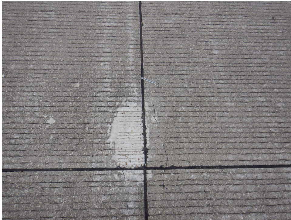
R18CK-01. Small Patching (Sample Unit No. 65).
