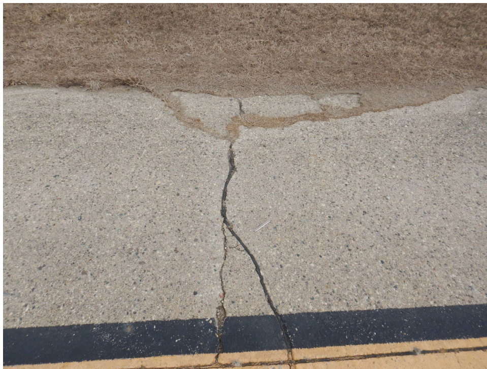
TH01CK-02. Shattered Slab (Sample Unit No. 01).
