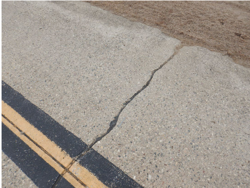
TH01CK-02. LTD Cracking (Sample Unit No. 01).
