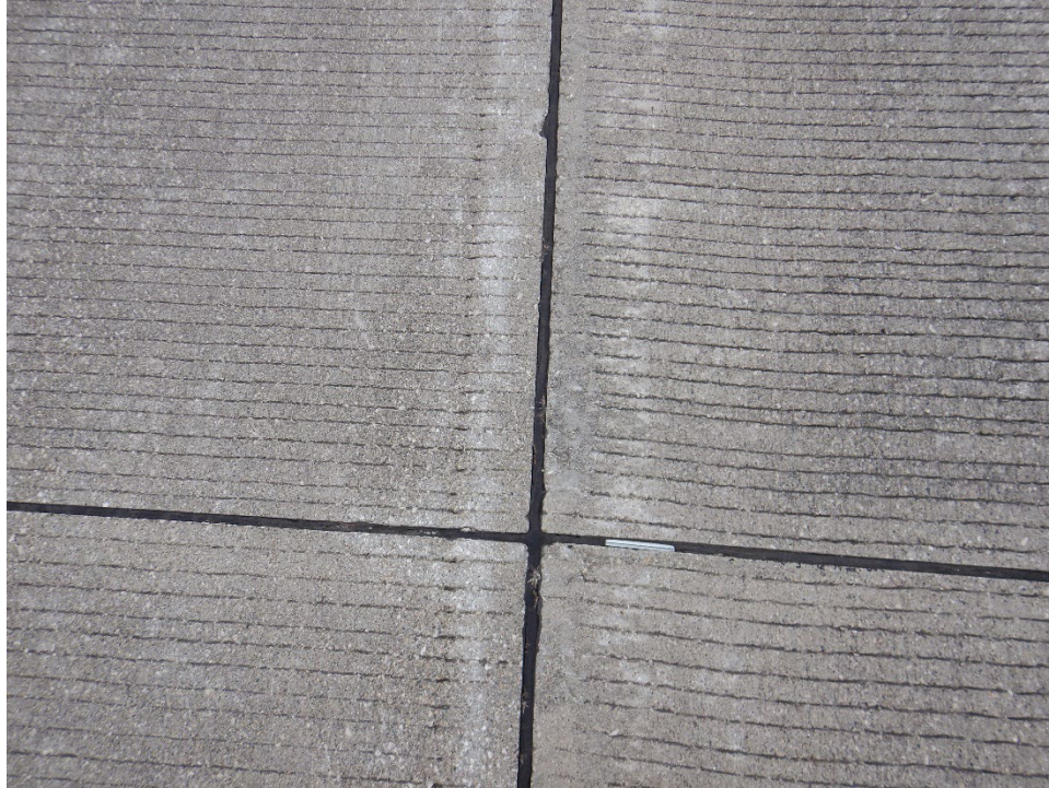
R18CK-01. Joint Seal Damage (Sample Unit No. 74).
