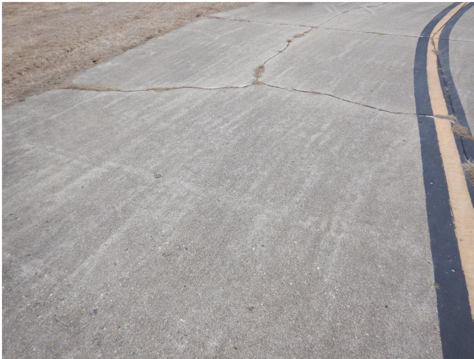
TH01CK-03. LTD Cracking (Sample Unit No. 04).
