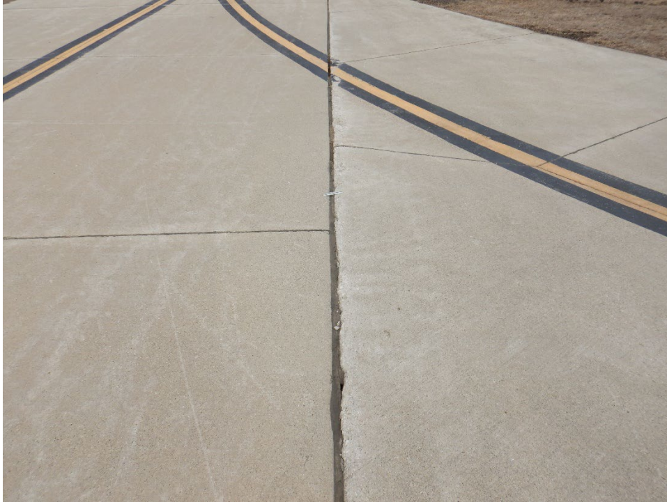
TH02CK-01. Faulting (Sample Unit No. 02).
