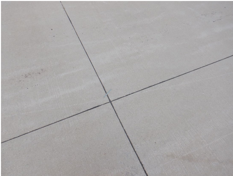
TH02CK-03. Joint Seal Damage (Sample Unit No. 04).
