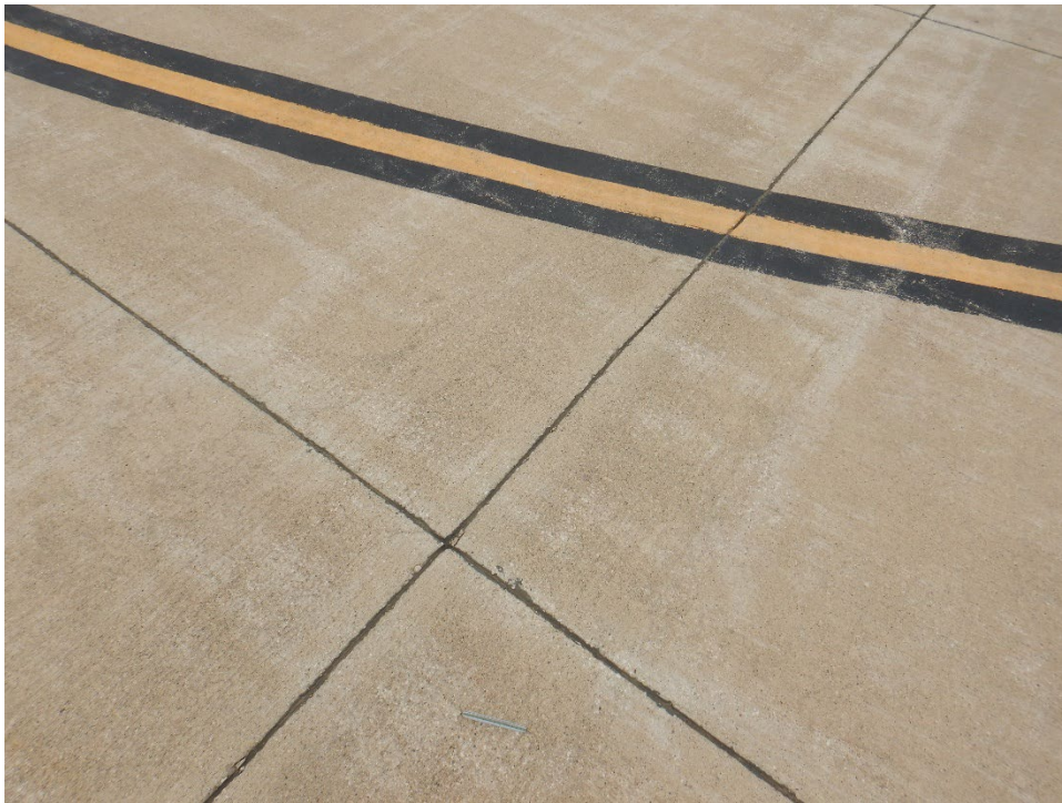
TH01CK-01. Joint Seal Damage (Sample Unit No. 01).
