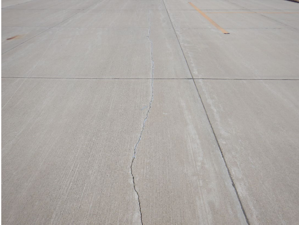
A01CK-01. LTD Cracking (Sample Unit No. 03).
