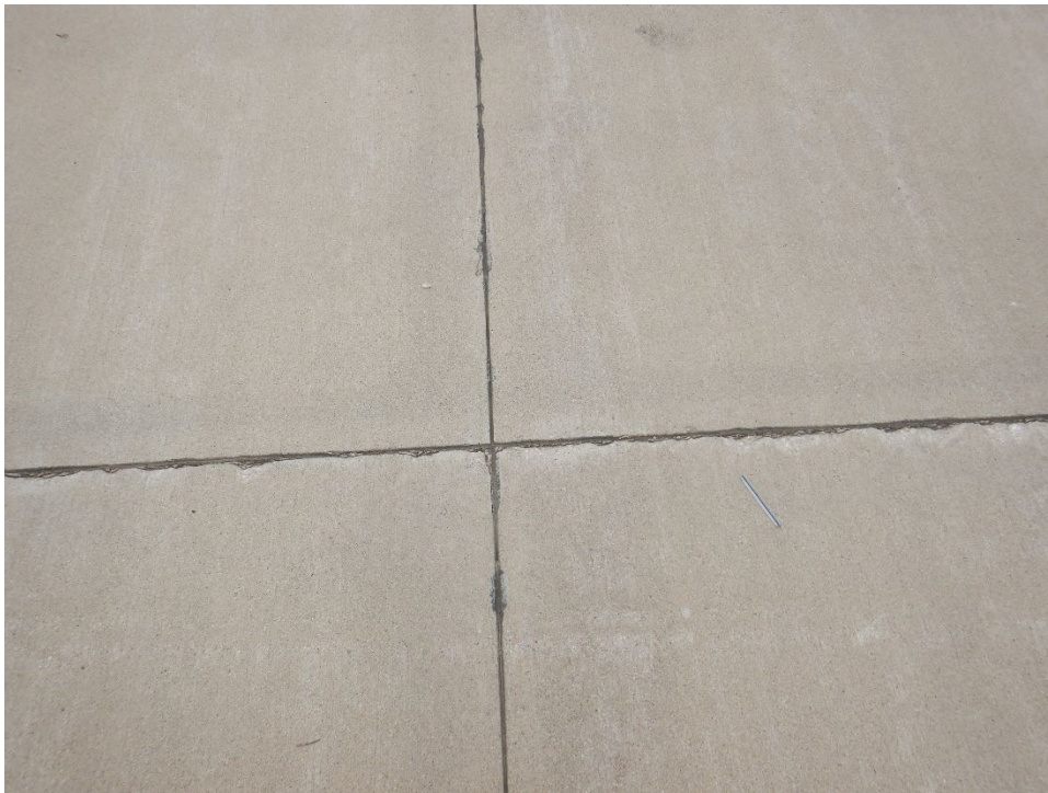
A01CK-01. Joint Seal Damage (Sample Unit No. 03).
