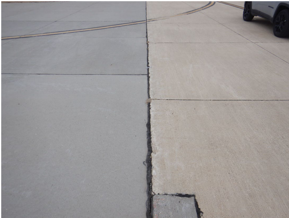
T02CK-01. Faulting (Additional Sample Unit No. 01).
