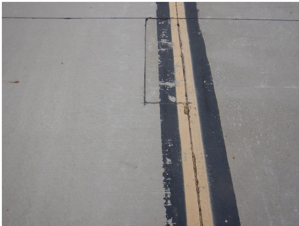
T02CK-01. Small Patching (Sample Unit No. 03).
