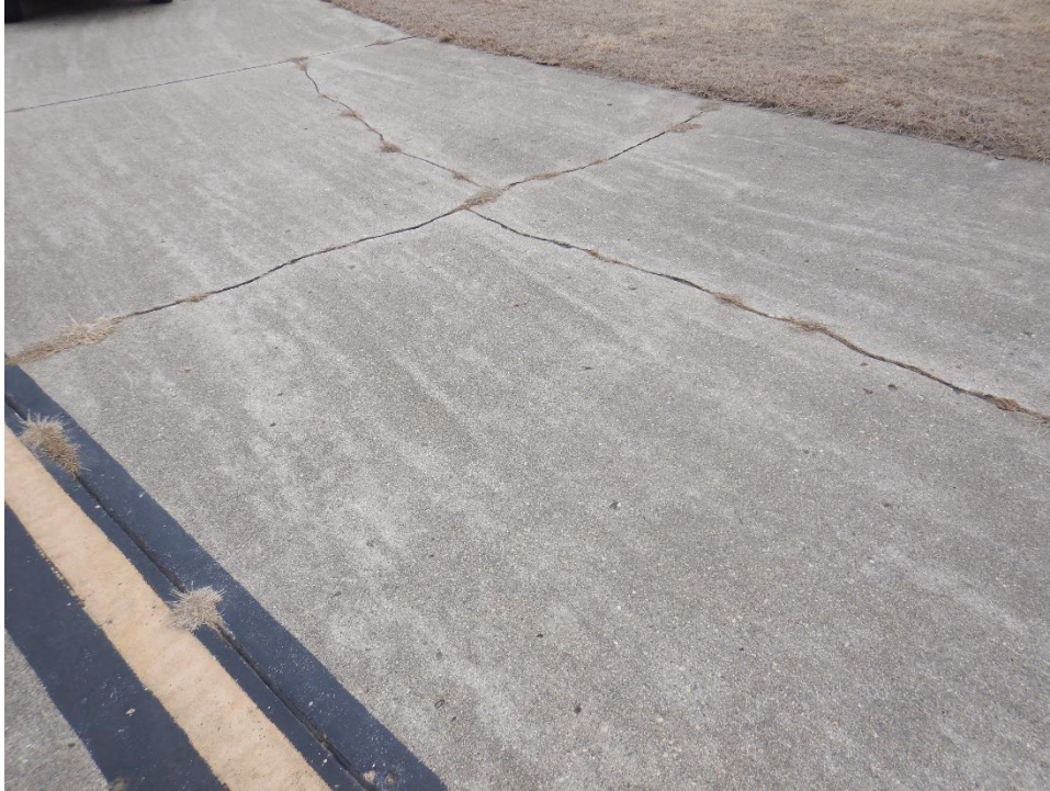
TH01CK-03. Shattered Slab (Sample Unit No. 04).
