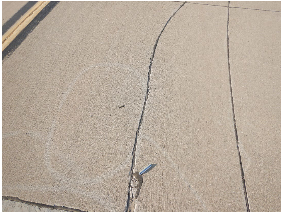
T02CH-01. LTD Cracking (Sample Unit No. 003).
