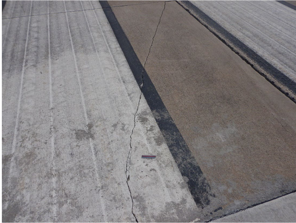
R17CH-01. LTD Cracking (Sample Unit No. 05).
