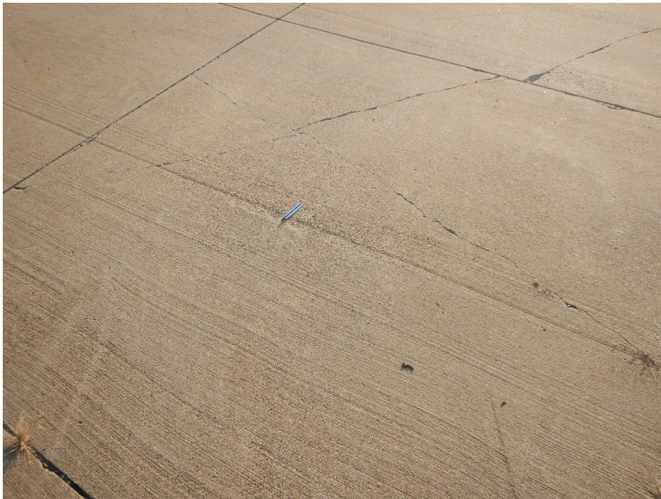
A01CH-01. Shattered Slab (Additional Sample Unit No. 13).
