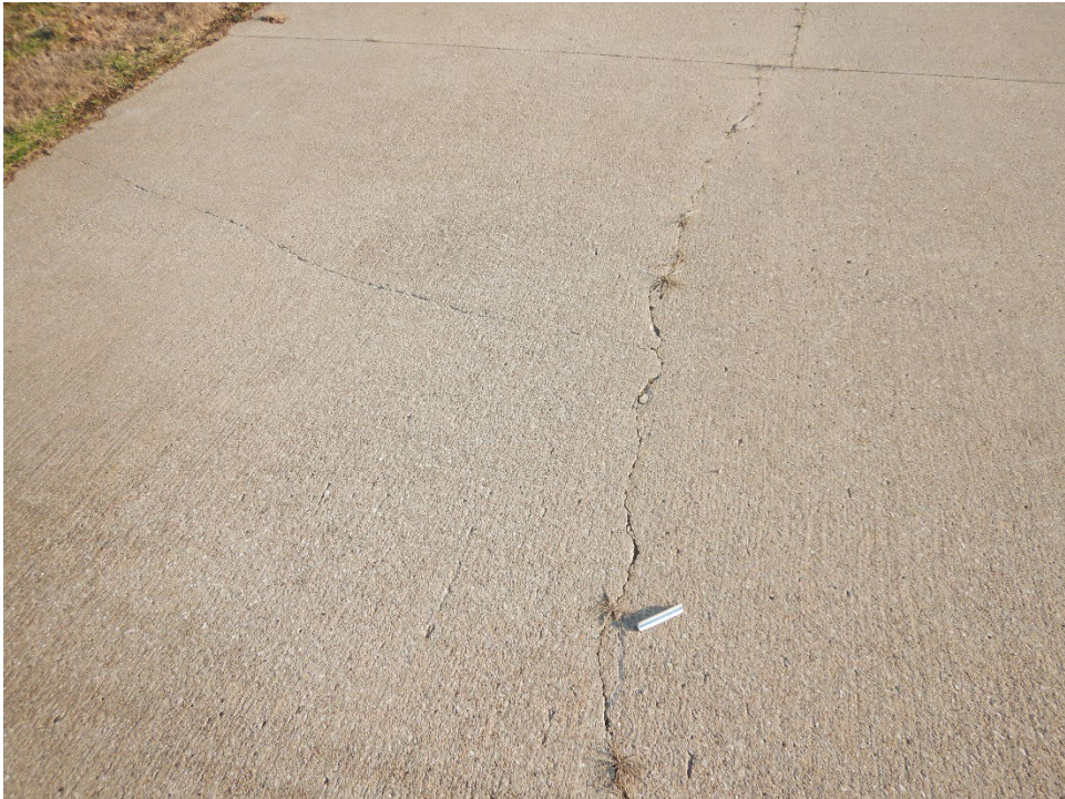
TH01CH-03. LTD Cracking (Sample Unit No. 01) (2).
