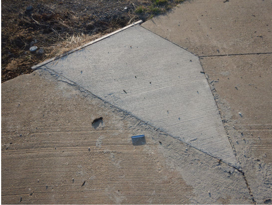
A01CH-01. Large Patching (Additional Sample Unit No. 13).
