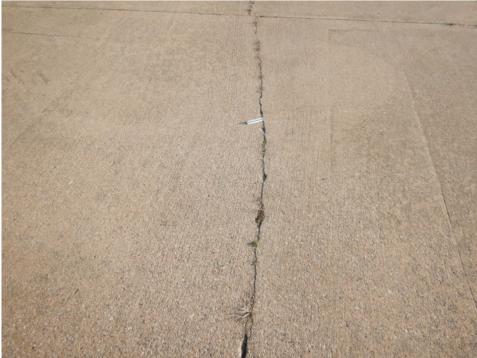
TH01CH-03. LTD Cracking (Sample Unit No. 01) (1).
