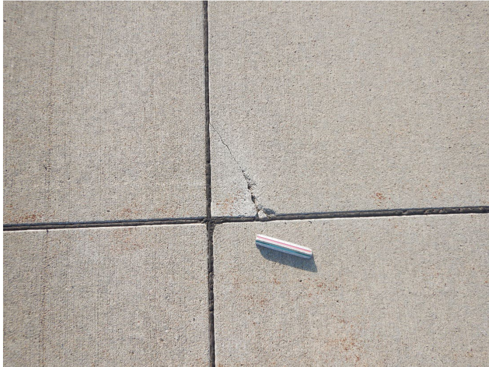
T04CH-01. Corner Spalling (Sample Unit No. 007).
