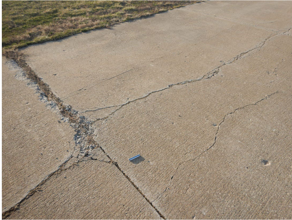
TH01CH-02. Shattered Slab (Sample Unit No. 01) (2).
