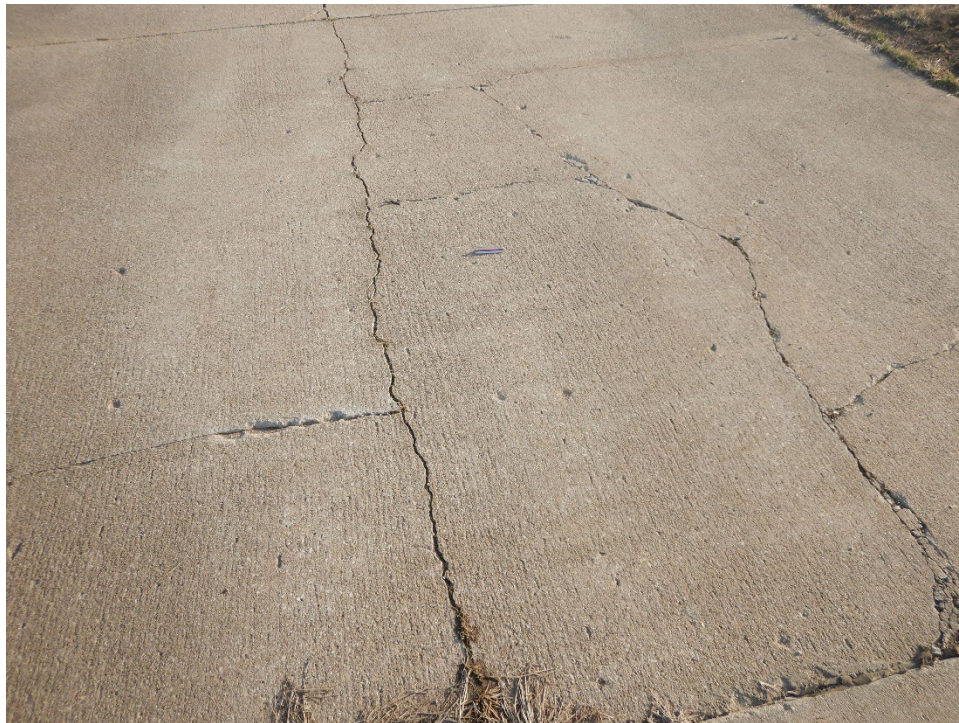
TH01CH-02. Shattered Slab (Sample Unit No. 01) (1).
