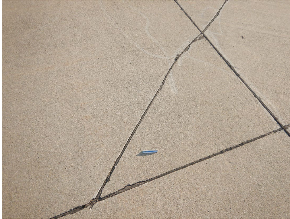
A01CH-01. Corner Break (Additional Sample Unit No. 11).
