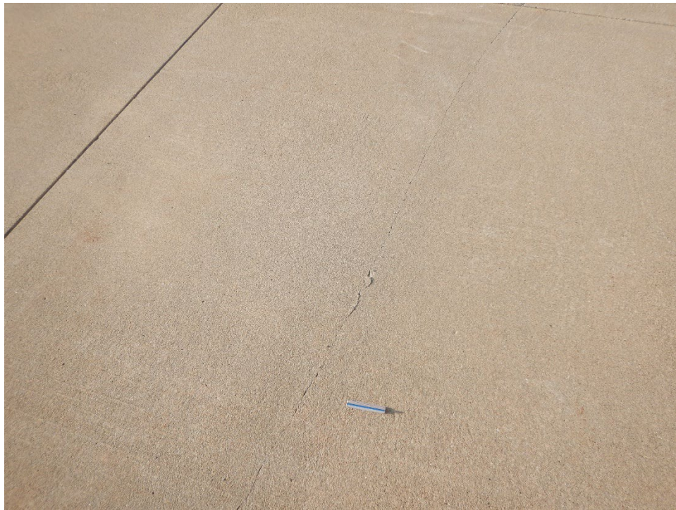
A01CH-01. LTD Cracking (Sample Unit No. 03).
