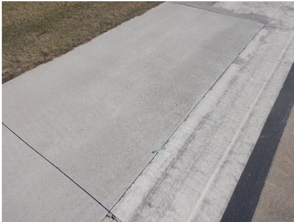
R17CH-01. Large Patching (Sample Unit No. 05).
