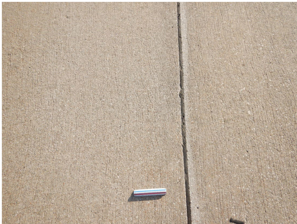
T03CH-01. Joint Seal Damage (Sample Unit No. 020).
