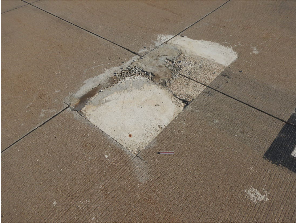
R10CH-01. Large Patching (Sample Unit No. 39).
