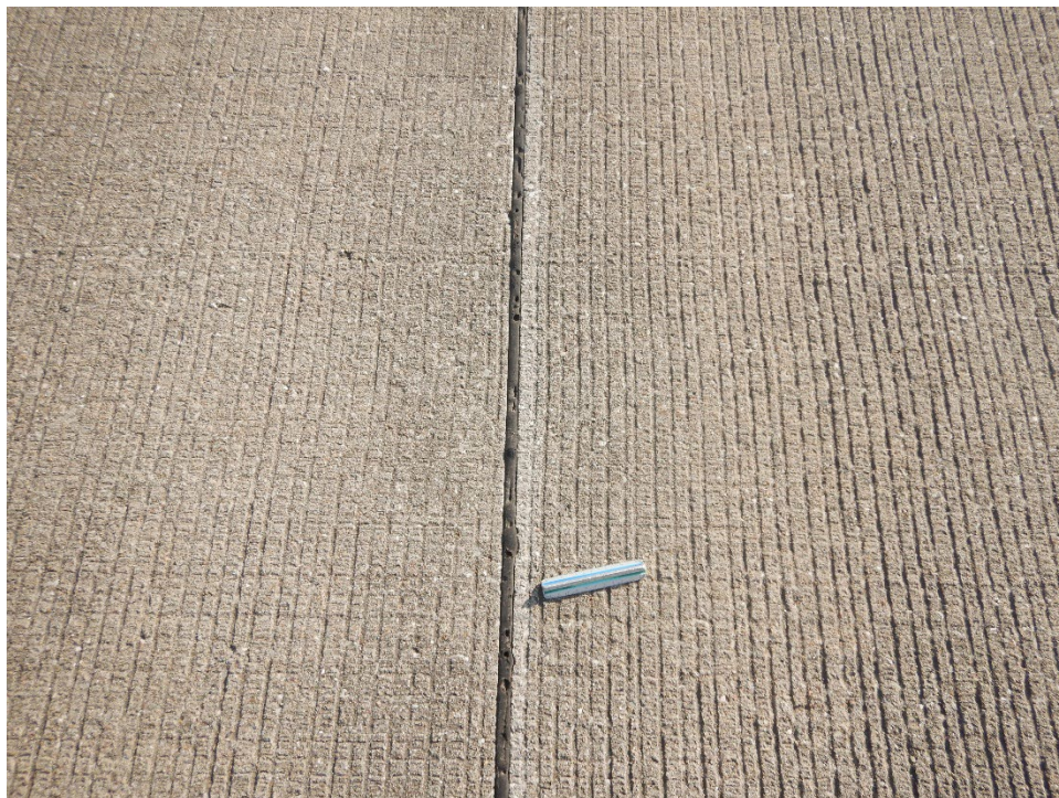
R10CH-01. Joint Seal Damage (Sample Unit No. 019).
