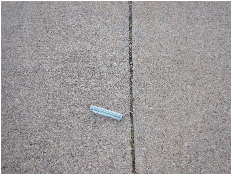
TH01CH-01. Joint Seal Damage (Sample Unit No. 01).
