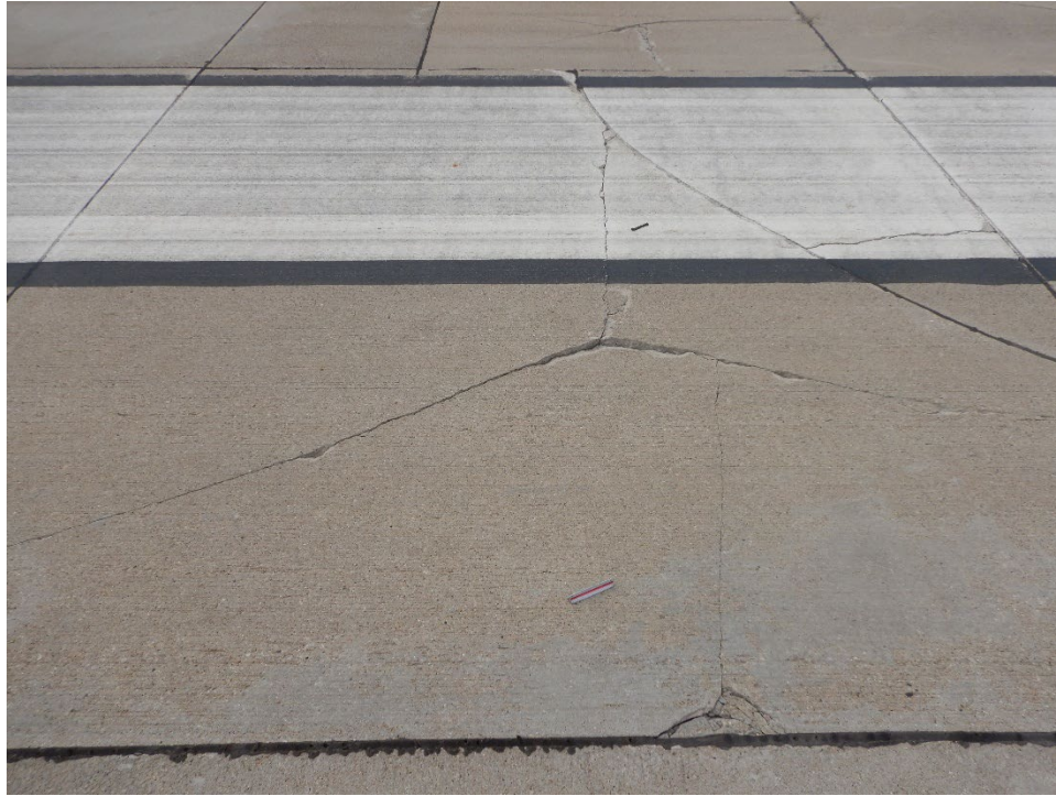
R17CH-01. Shattered Slab (Sample Unit No. 57).
