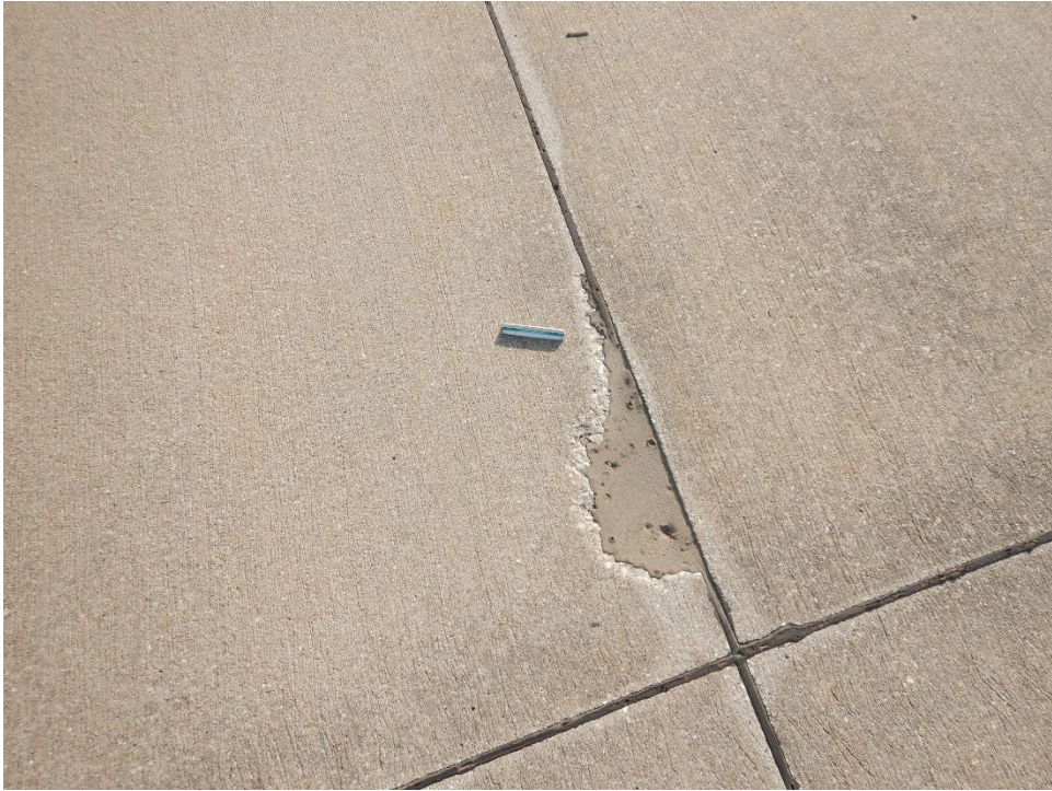
T03CH-01. Joint Spalling (Sample Unit No. 020).
