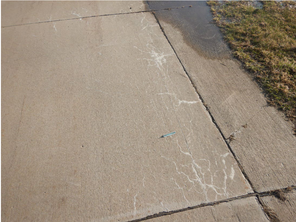
T02CH-01. ASR (Sample Unit No. 001).
