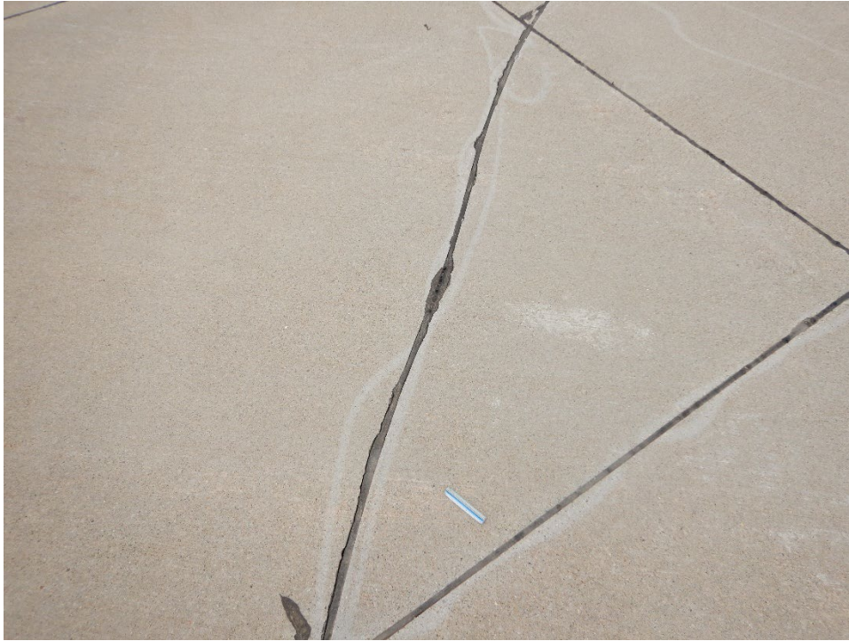
T01CH-01. LTD Cracking (Sample Unit No. 04).
