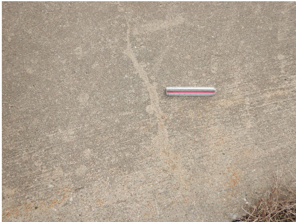
T01CH-02. ASR (Sample Unit No. 002).
