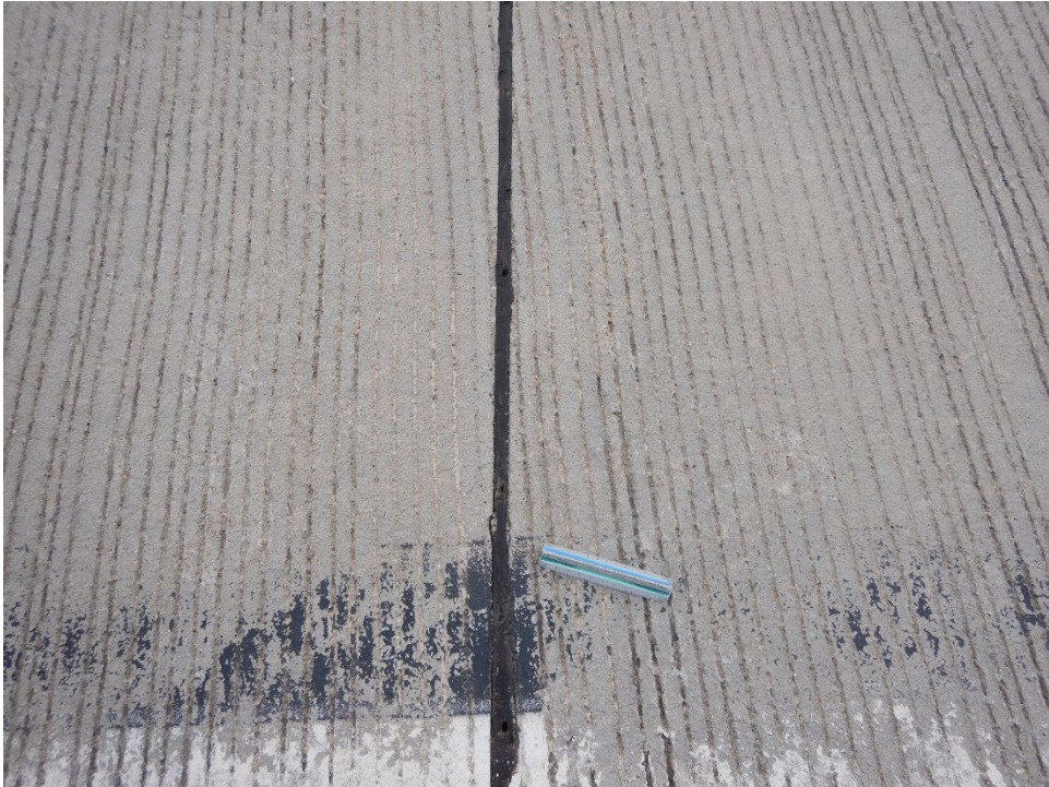
R10CH-02. Joint Seal Damage (Sample Unit No. 03).
