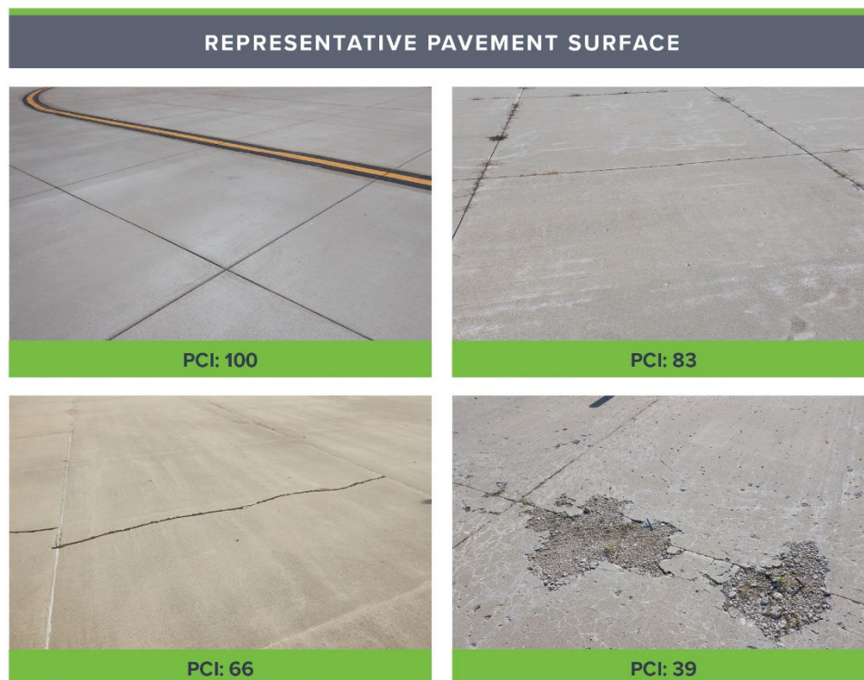
Figure 4. Visual representation of PCI scale on typical pavement surfaces.
