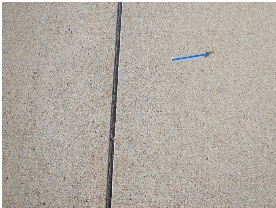
T04CH-01. Joint Seal Damage (Sample Unit No. 004).
