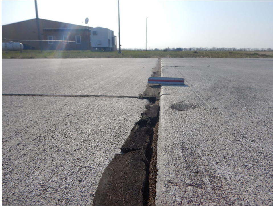
A02CH-02. Faulting (Sample Unit No. 01).
