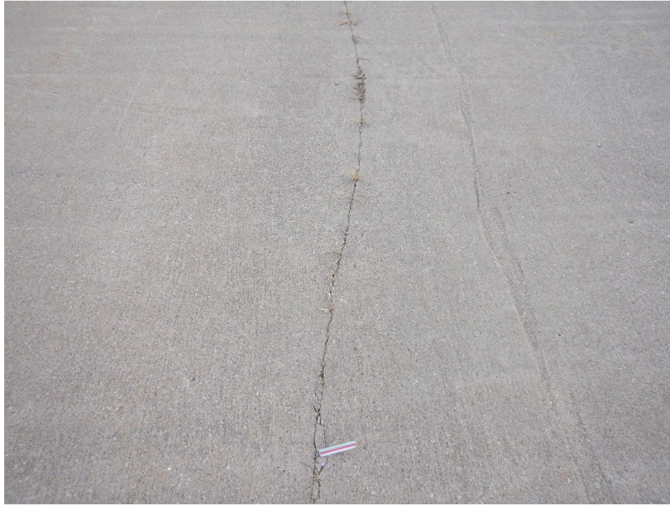
TH01CH-01. LTD Cracking (Sample Unit No. 01).
