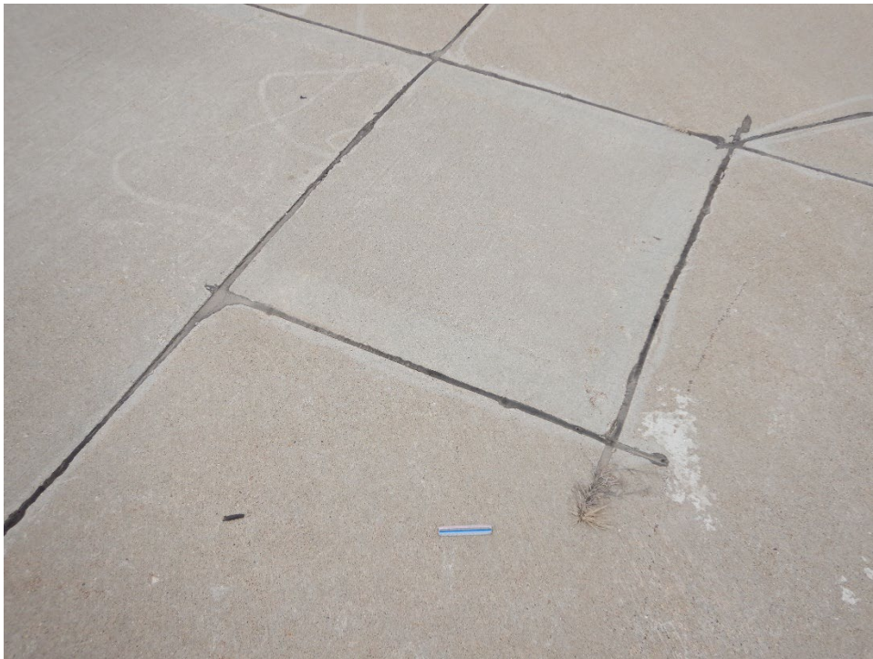
T01CH-01. Large Patching (Sample Unit No. 04).
