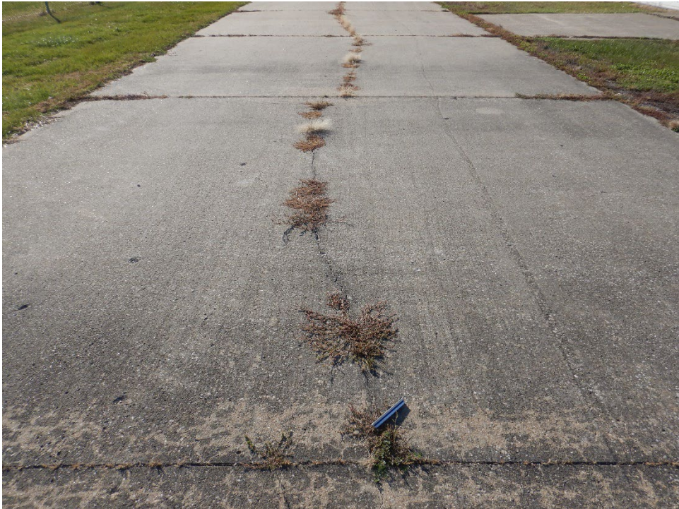
TH01CH-01. LTD Cracking (Sample Unit No. 01).
