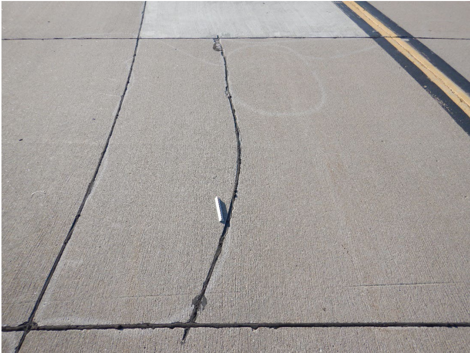
T02CH-01. LTD Cracking (Sample Unit No. 03).
