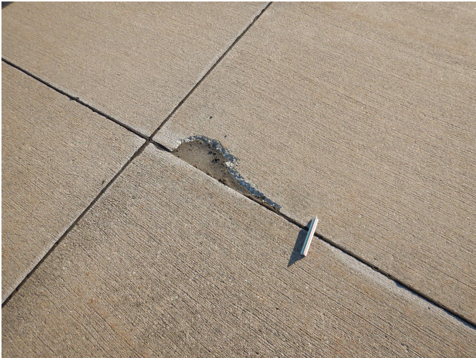
T03CH-01. Joint Spalling (Sample Unit No. 20).
