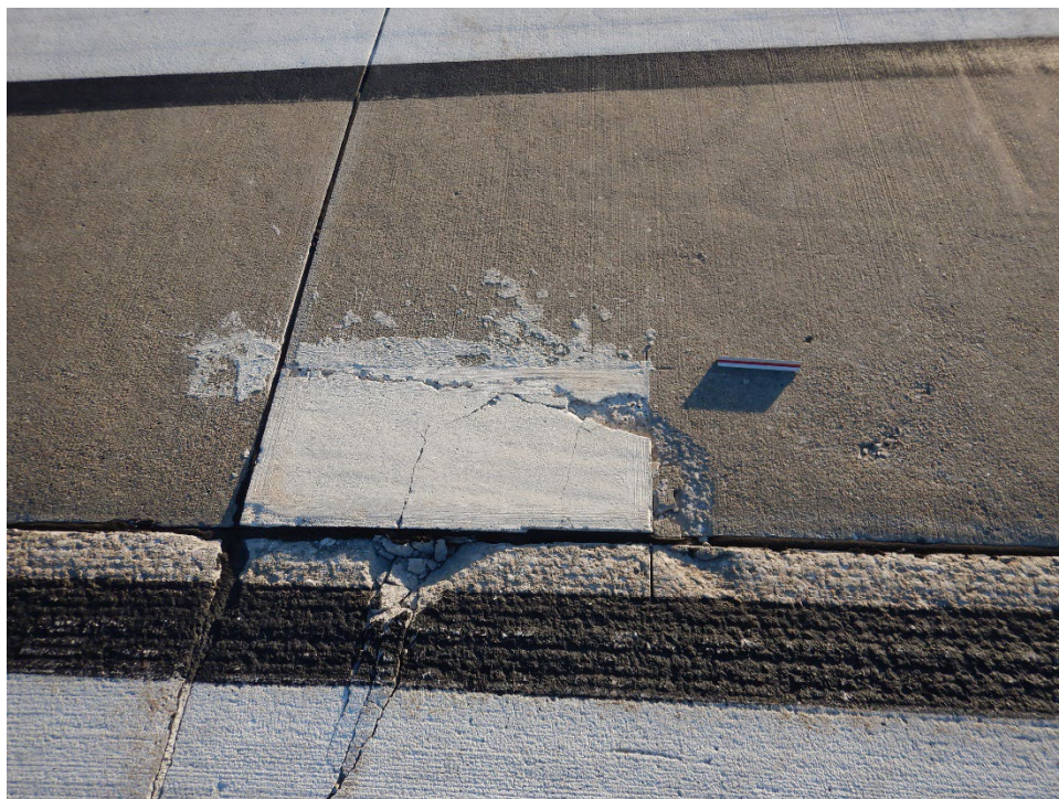
R17CH-01. Small Patching (Additional Sample Unit No. 04).
