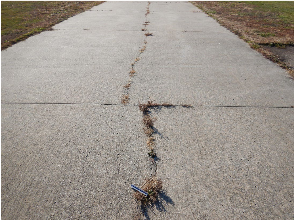
TH01CH-03. LTD Cracking (Sample Unit No. 01).
