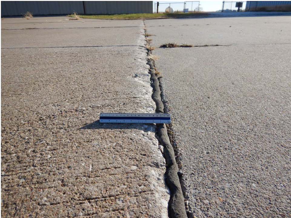
T02CH-01. Faulting (Additional Sample Unit No. 01).
