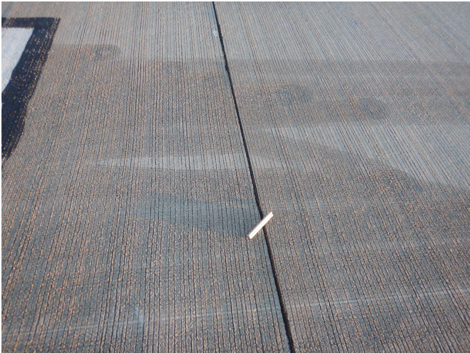
R10CH-02. Joint Seal Damage (Sample Unit No. 01).
