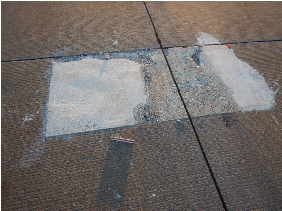
R10CH-01. Large Patching (Sample Unit No. 39).
