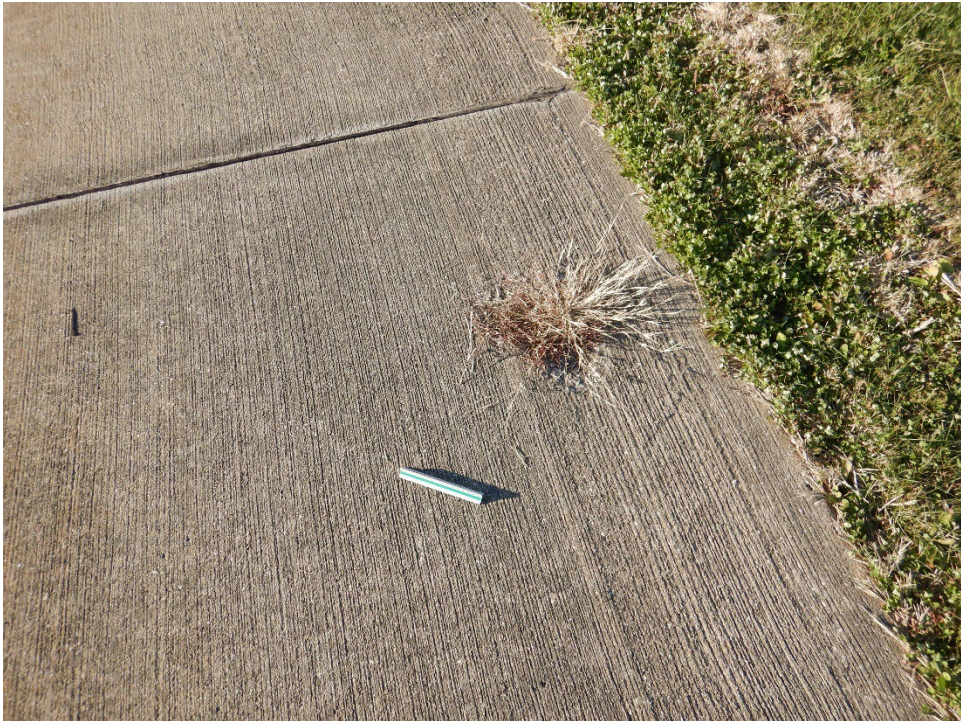
T03CH-01. Small Patching (Sample Unit No. 12).
