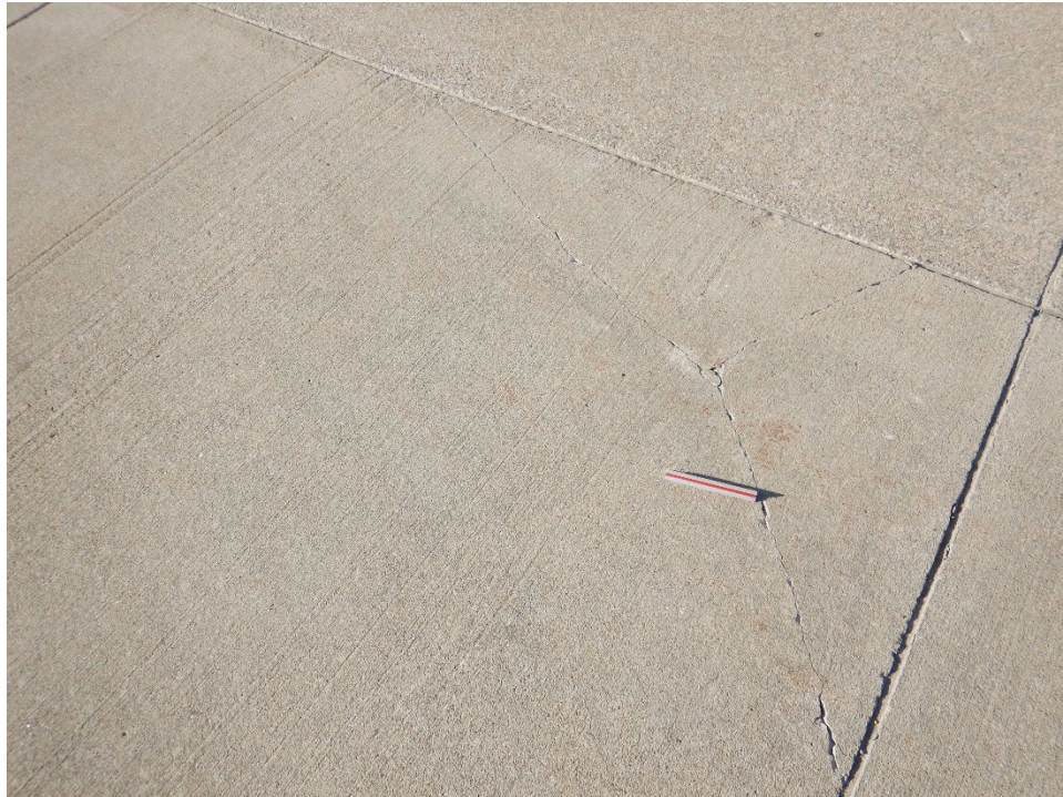
A01CH-01. LTD Cracking (Sample Unit No. 02).
