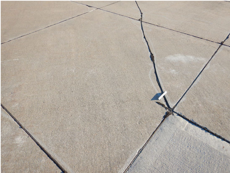
T01CH-01. LTD Cracking (Sample Unit No. 04).
