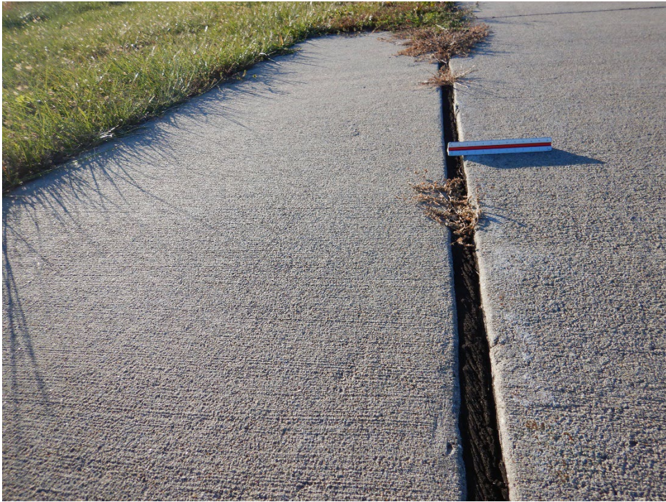
T04CH-01. Faulting (Sample Unit No. 15).
