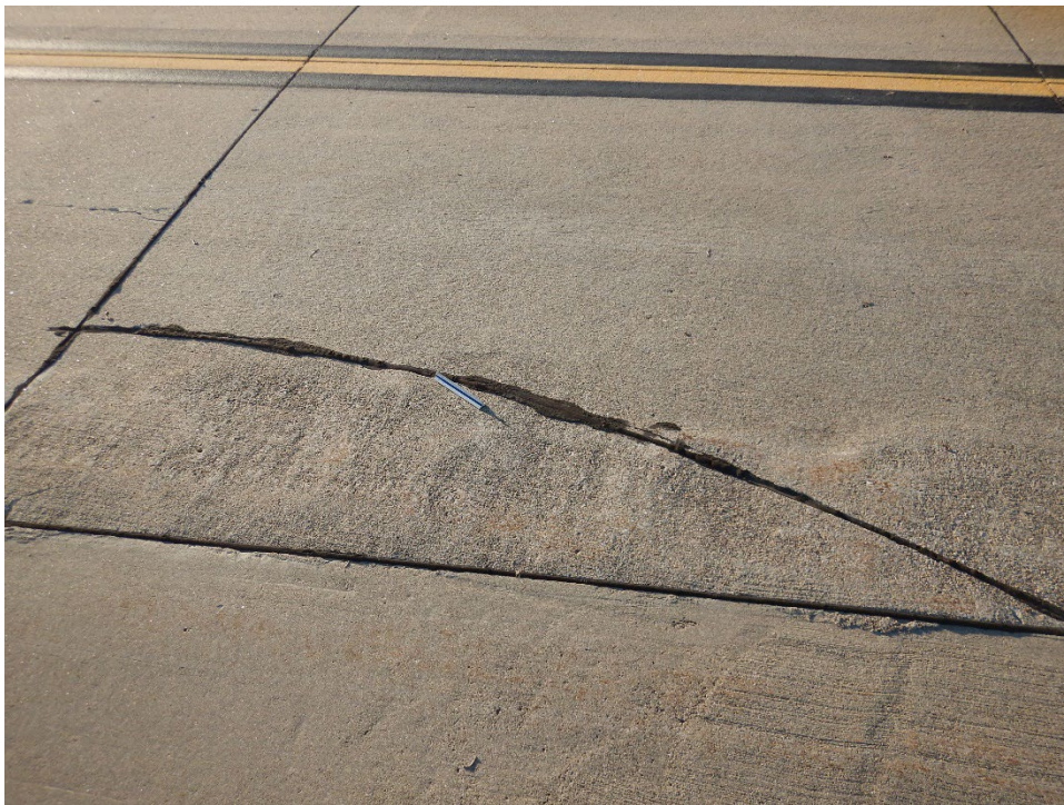
T01CH-02. LTD Cracking (Sample Unit No. 01).
