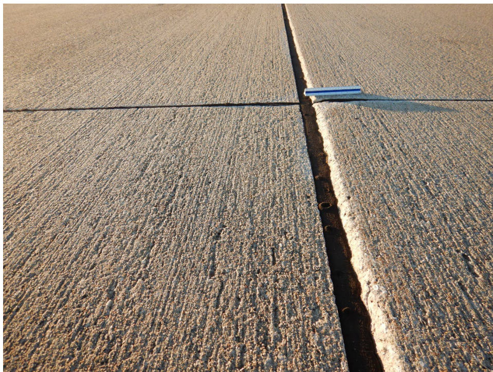
R17CH-01. Faulting (Sample Unit No. 45).
