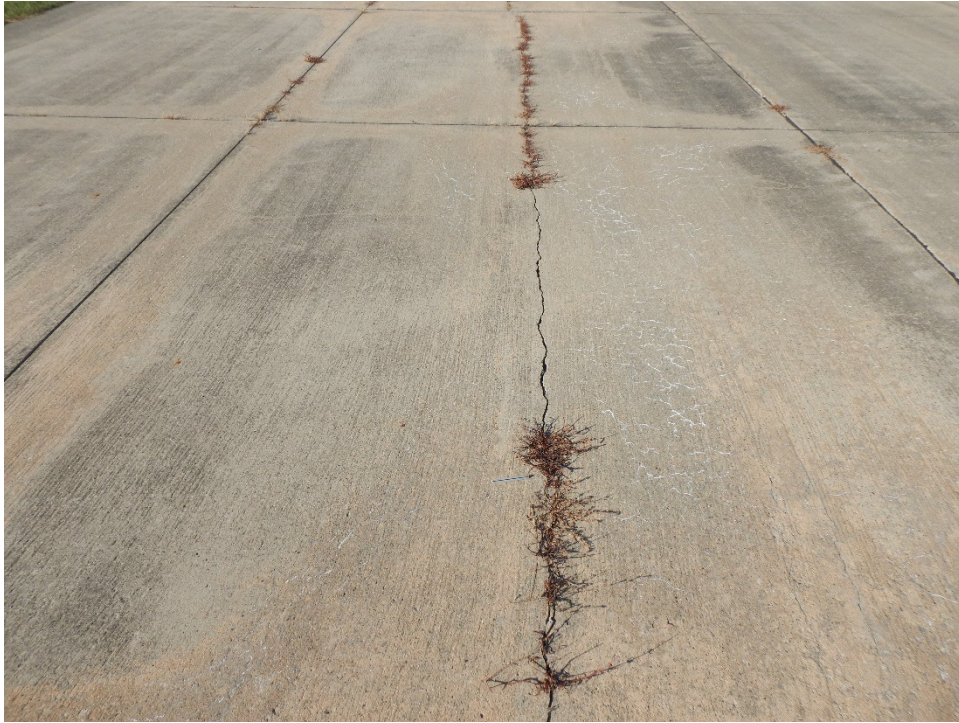
R16CE-03. LTD Cracking (Sample Unit No. 18).
