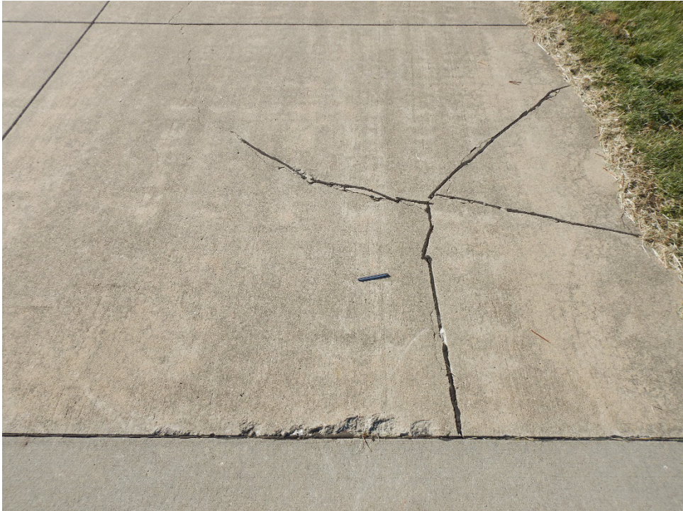
R16CE-01. Shattered Slab (Sample Unit No. 01).
