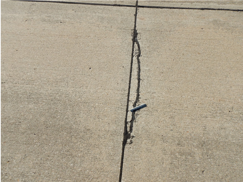
R16CE-02. Joint Spalling (Sample Unit No. 09).
