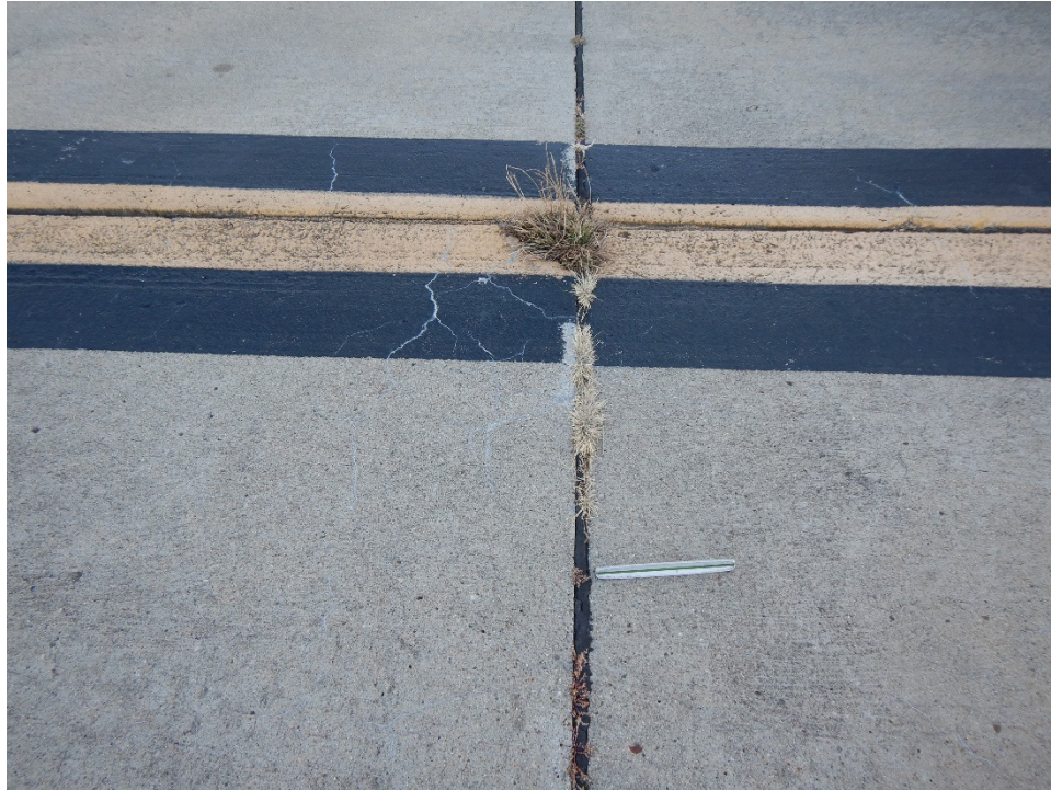
T01CE-01. Joint Seal Damage (Sample Unit No. 03).
