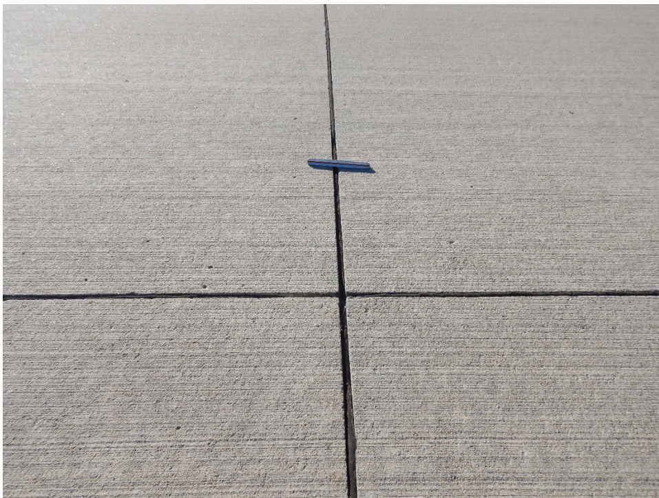
T03CE-01. Joint Seal Damage (Sample Unit No. 06).
