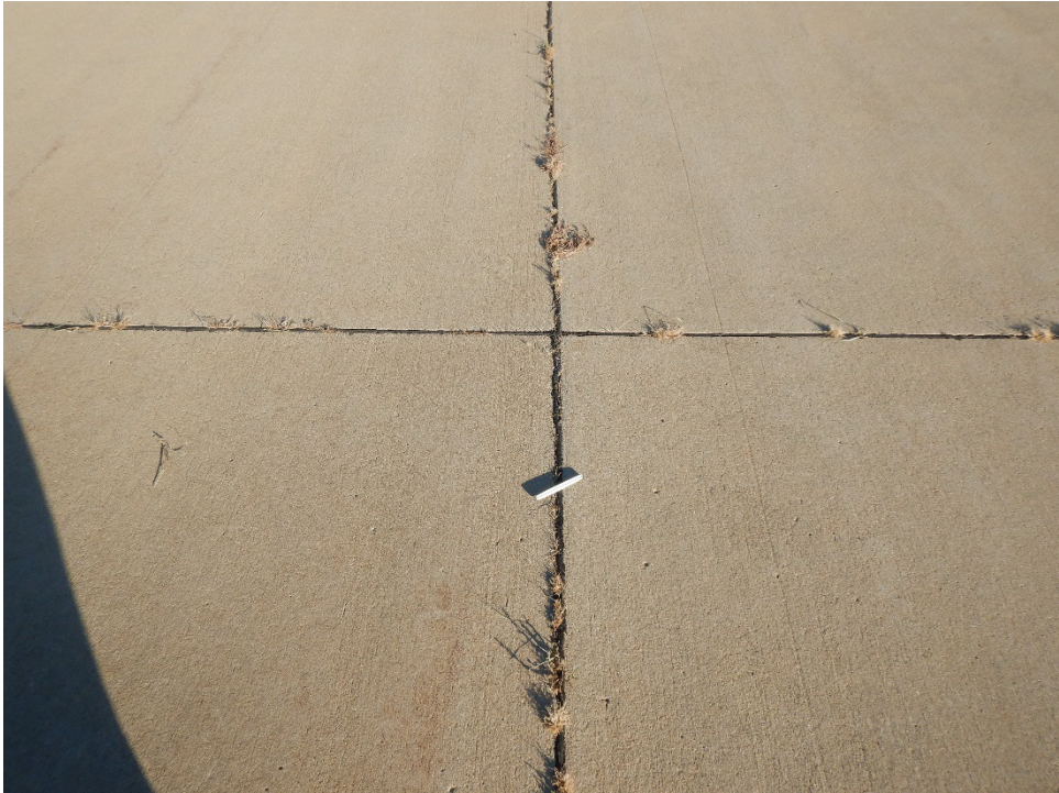
A01CE-01. Joint Seal Damage (Sample Unit No. 16).
