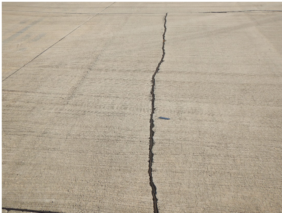
T01CE-02. LTD Cracking (Sample Unit No. 01).
