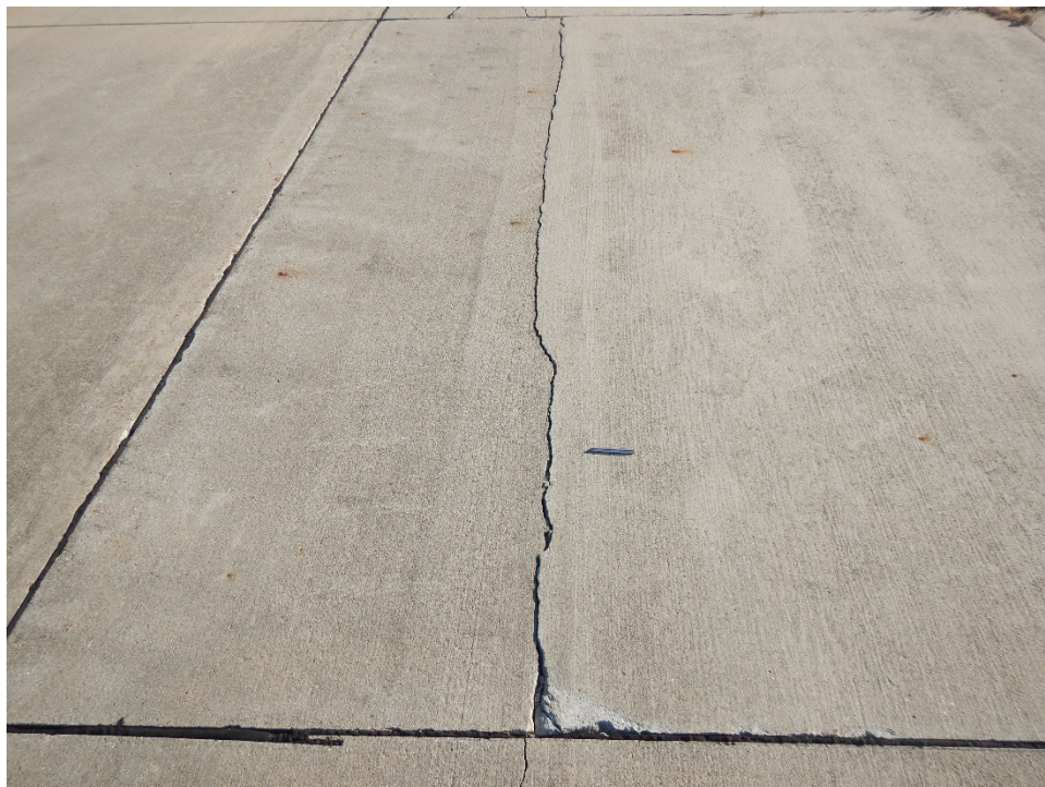
R16CE-04. LTD Cracking (Sample Unit No. 05).
