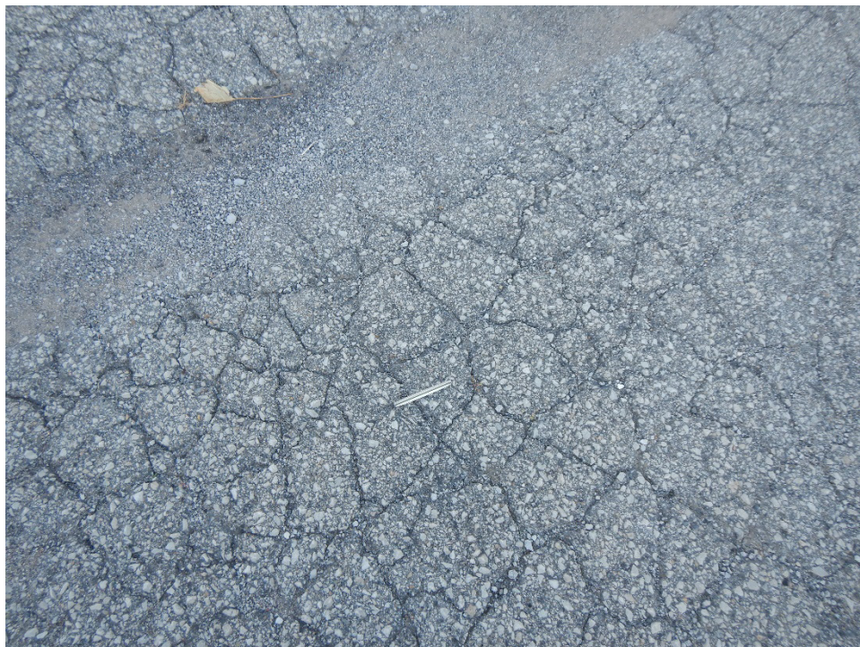
TH01CE-01. Alligator Cracking (Sample Unit No. 01).
