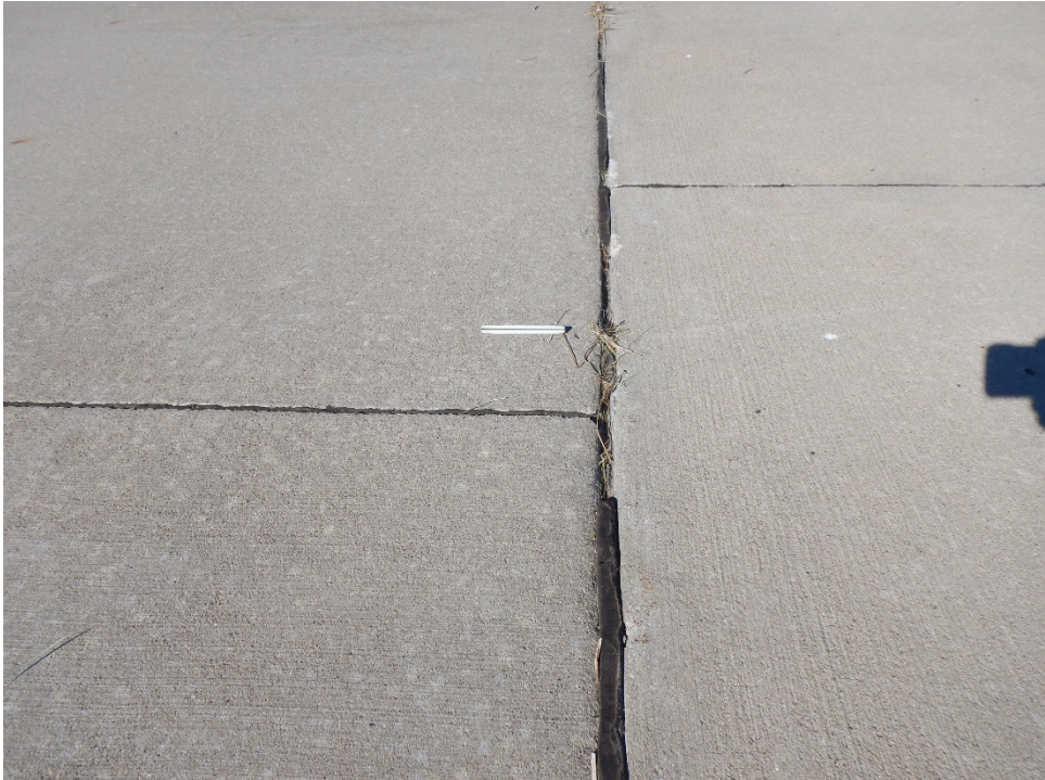
T02CE-01. Joint Seal Damage (Sample Unit No. 06).
