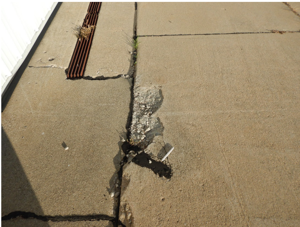
A01CE-02. Joint Spalling (Sample Unit No. 02).
