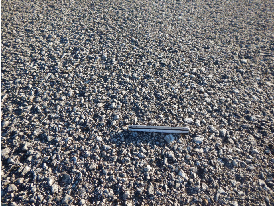
TH01CE-01. Weathering (Sample Unit No. 02).
