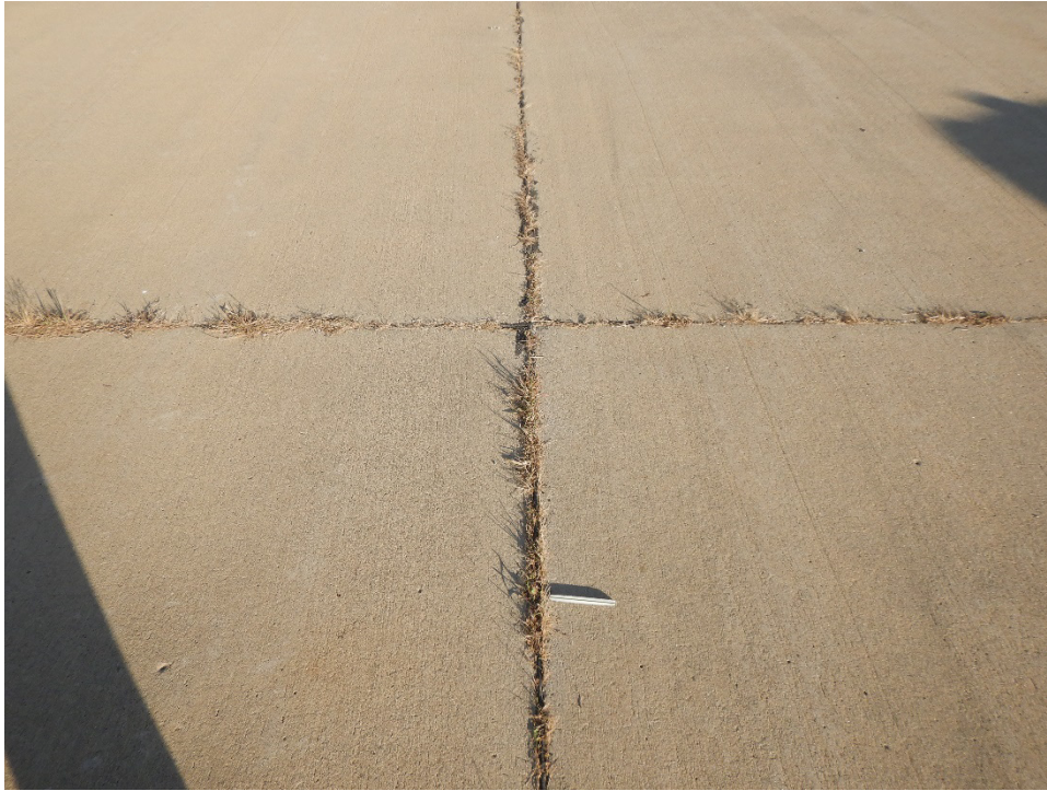
A01CE-02. Joint Seal Damage (Sample Unit No. 01).
