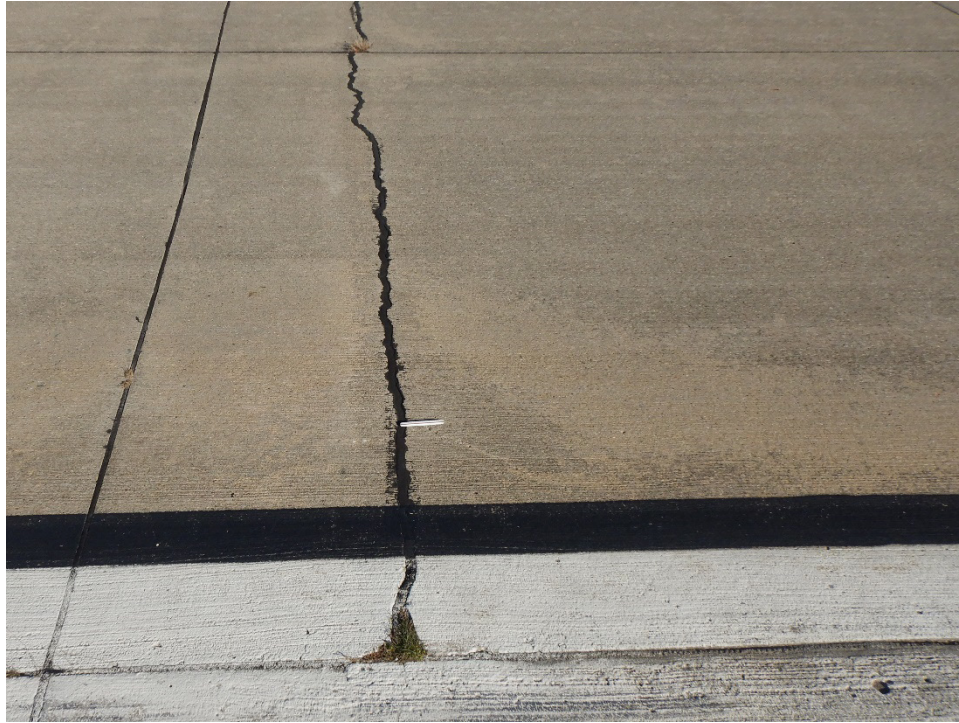
R16CE-02. LTD Cracking (Sample Unit No. 13).
