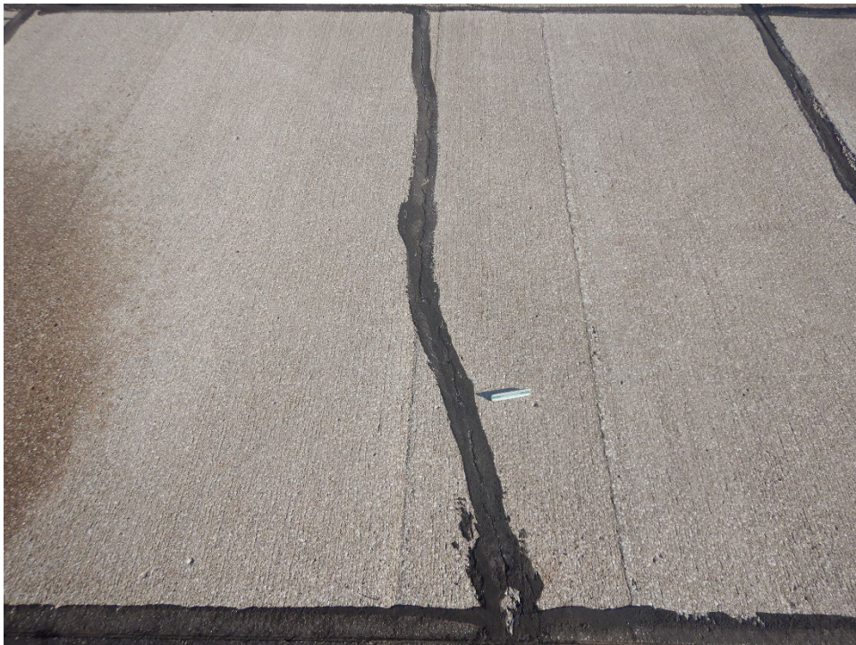
A01BR-02. LTD Cracking (Sample Unit No. 14).
