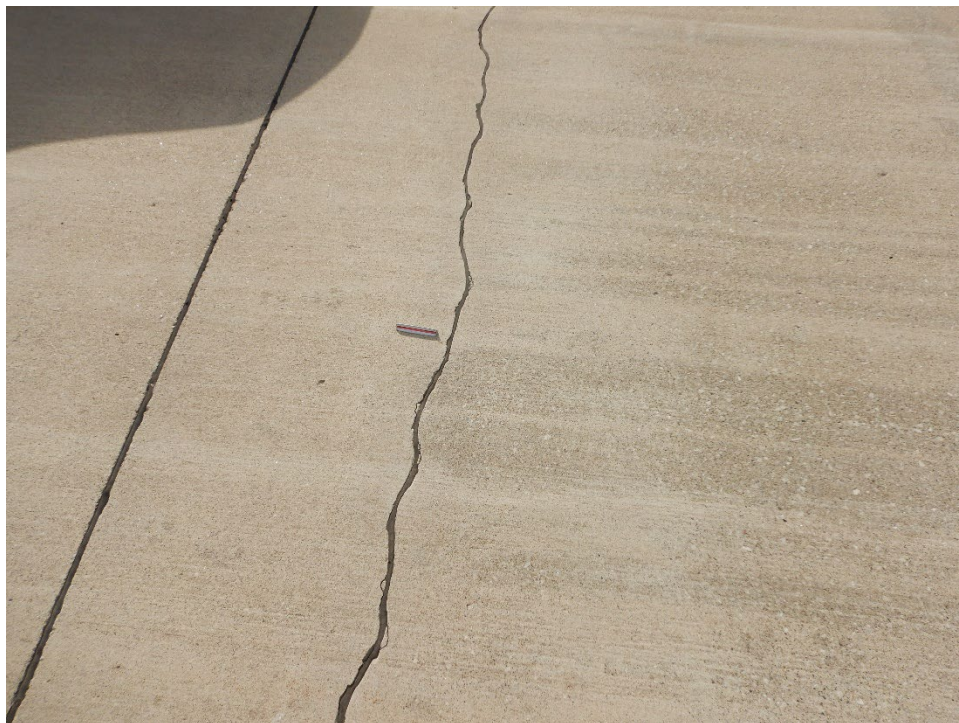
TABR-01. LTD Cracking (Sample Unit No. 05).
