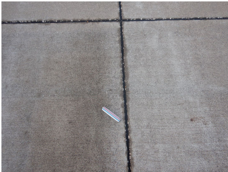
TH01BR-02. Joint Seal Damage (Sample Unit No. 08).
