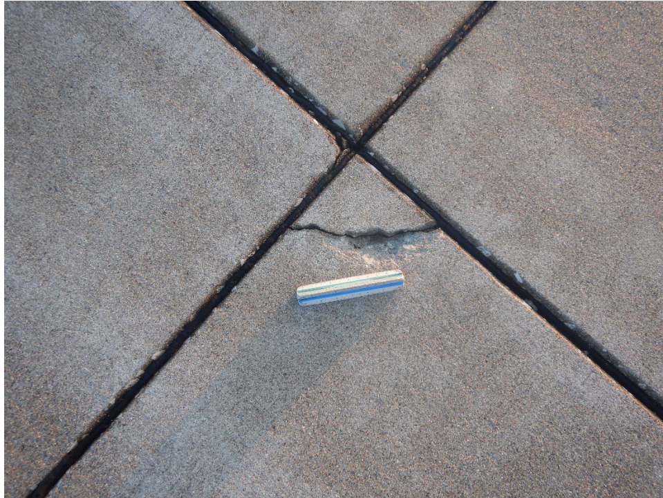
TH01BR-02. Corner Spalling (Sample Unit No. 04).
