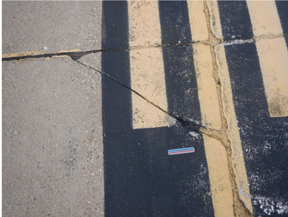
TABR-01. Corner Break (Sample Unit No. 03).
