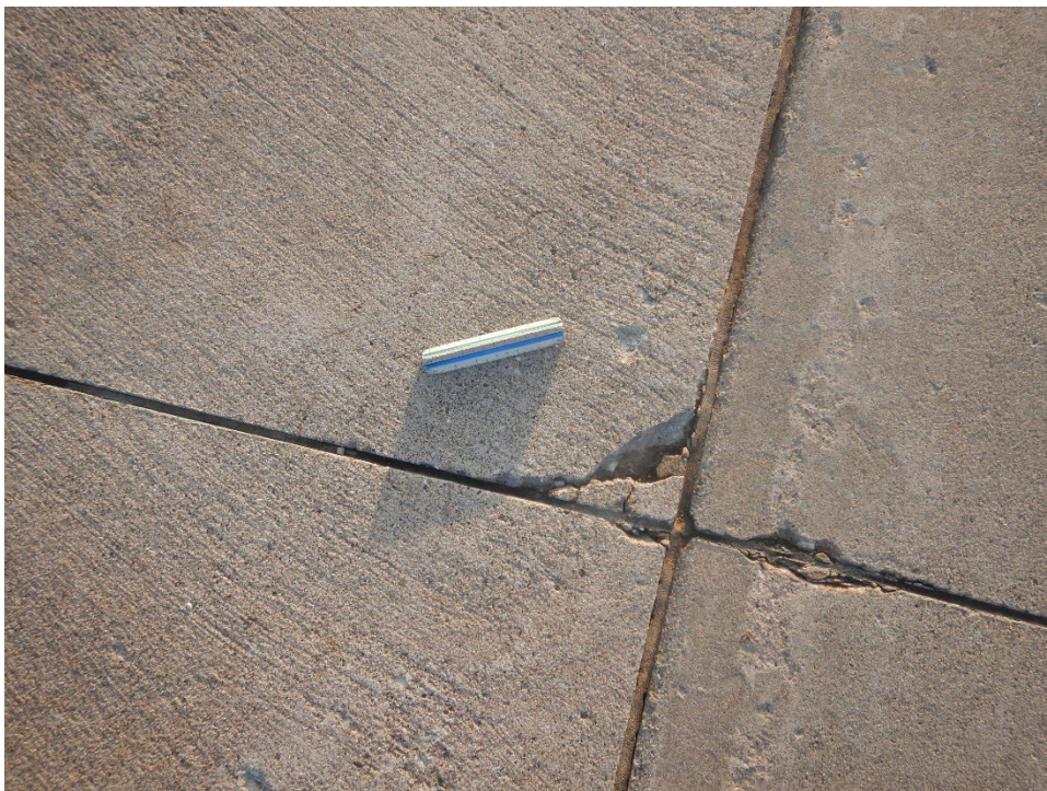
TA2BR-02. Corner Spalling (Sample Unit No. 05).
