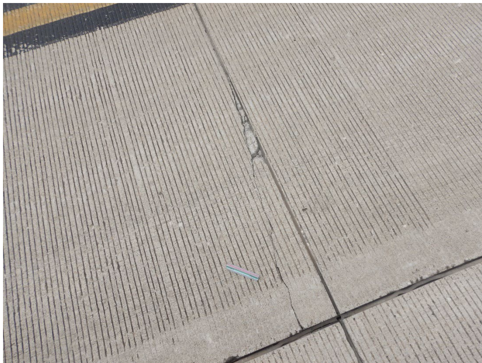
R12BR-02. Corner Spalling (Sample Unit No. 47).
