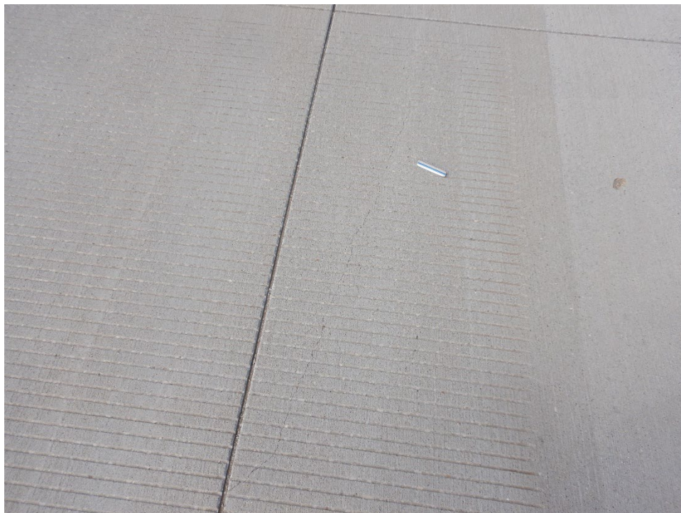
R12BR-03. LTD Cracking (Sample Unit No. 03).
