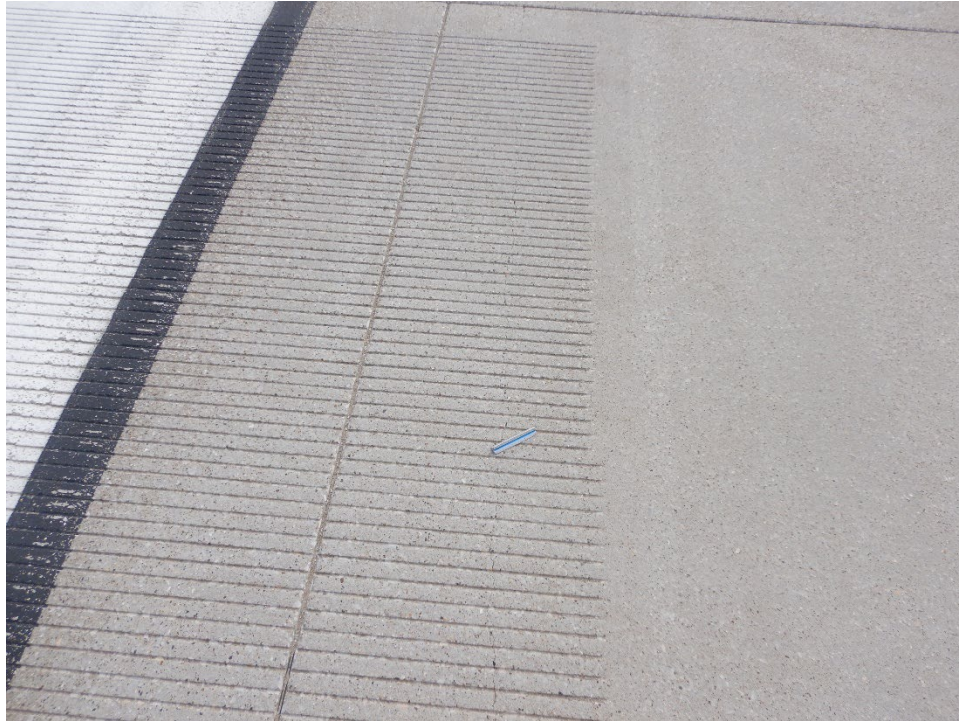
R18BR-01. LTD Cracking (Sample Unit No. 145).
