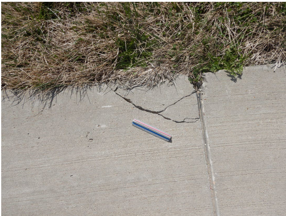
TBBR-03. Corner Spalling (Sample Unit No. 01).
