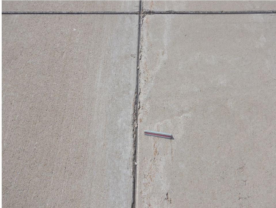
TA3BR-02. Joint Seal Damage (Sample Unit No. 02).
