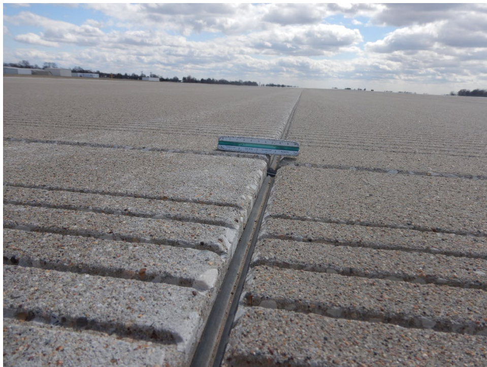
R18BR-01 Faulting. (Sample Unit No. 015).
