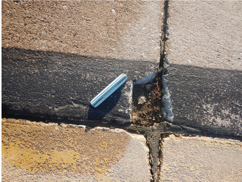
TDBR-03. Corner Spalling (Sample Unit No. 04).
