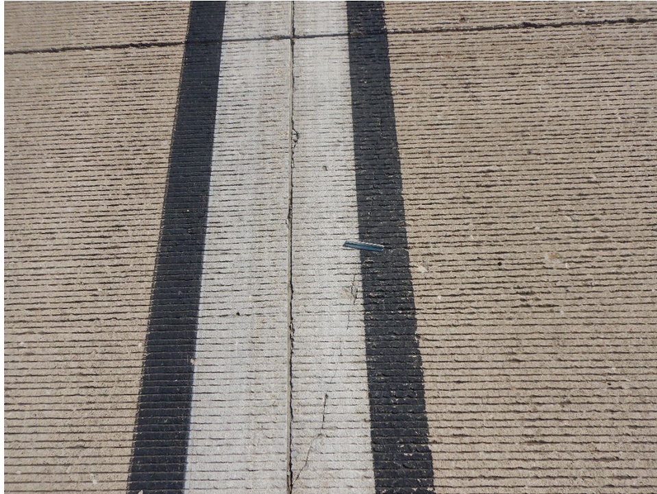
R12BR-01. Corner Spalling (Sample Unit No. 153).
