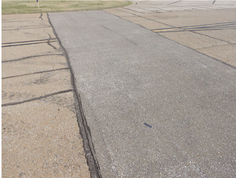
TDBR-04. Patching (Additional Sample Unit No. 07).
