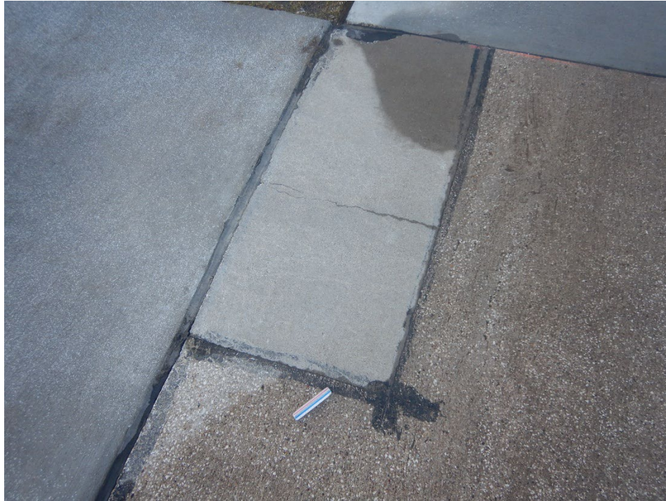
A01BR-02. Large Patching (Sample Unit No. 18).
