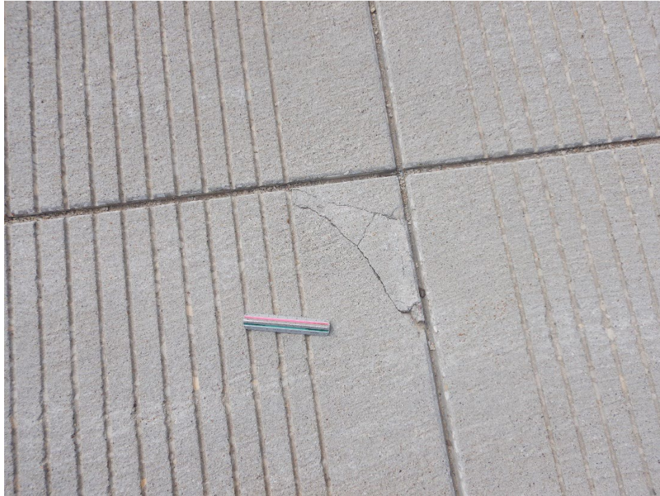
R12BR-03. Corner Spalling (Sample Unit No. 24).
