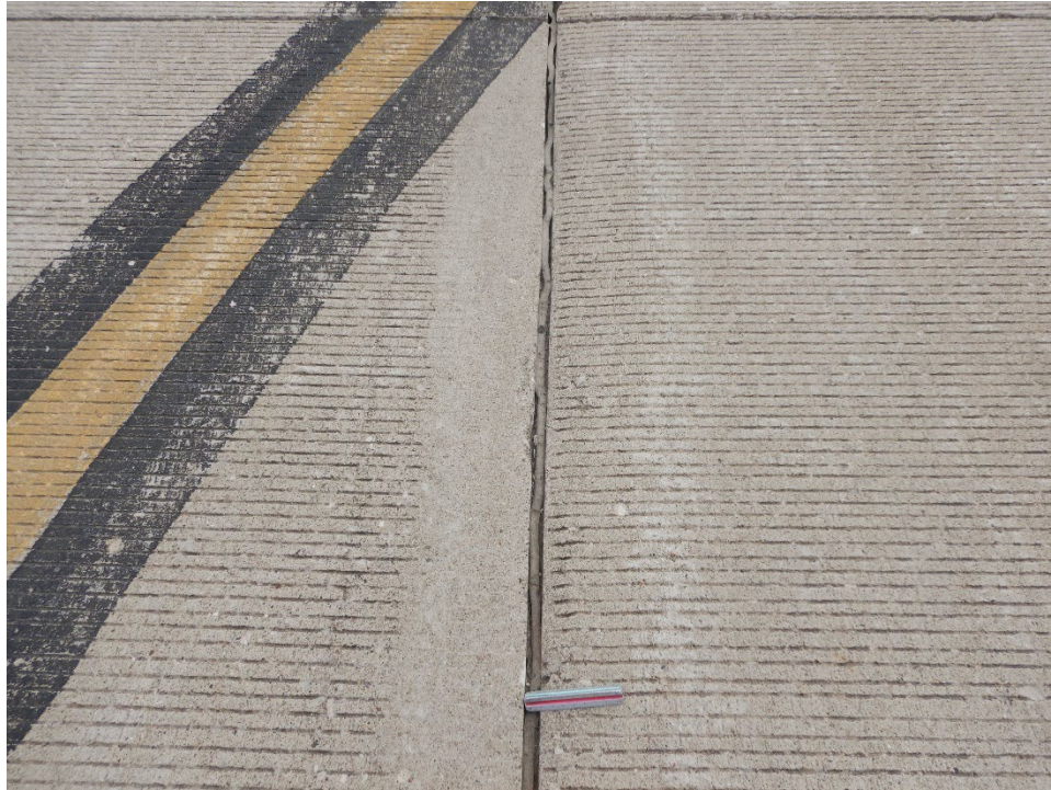
R12BR-02. Joint Seal Damage (Sample Unit No. 50).
