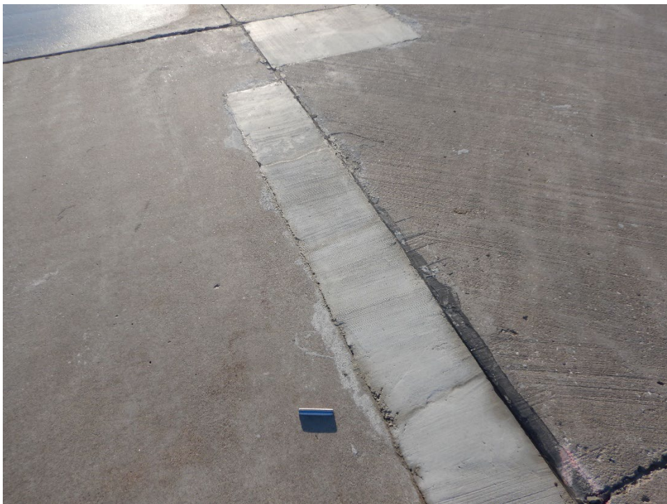
TCBR-01. Large Patching (Additional Sample Unit No. 11).
