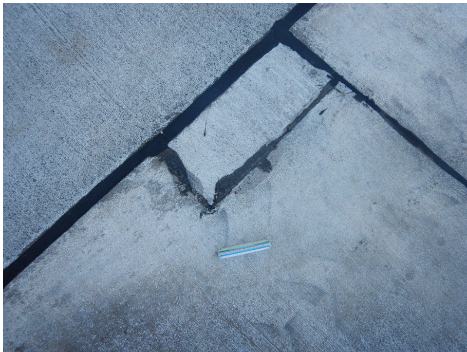
A01BR-03. Small Patching (Sample Unit No. 01).
