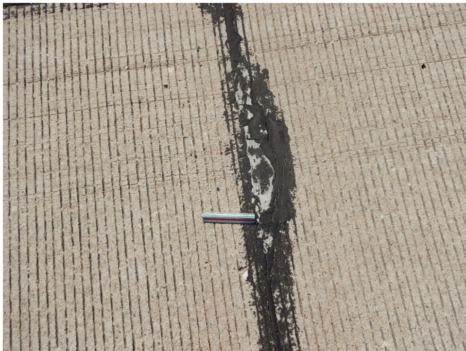
R12BR-01. Joint Spalling (Sample Unit No. 052).
