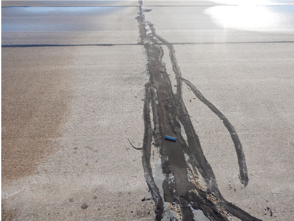
A01BR-02. Large Patching (Sample Unit No. 02).
