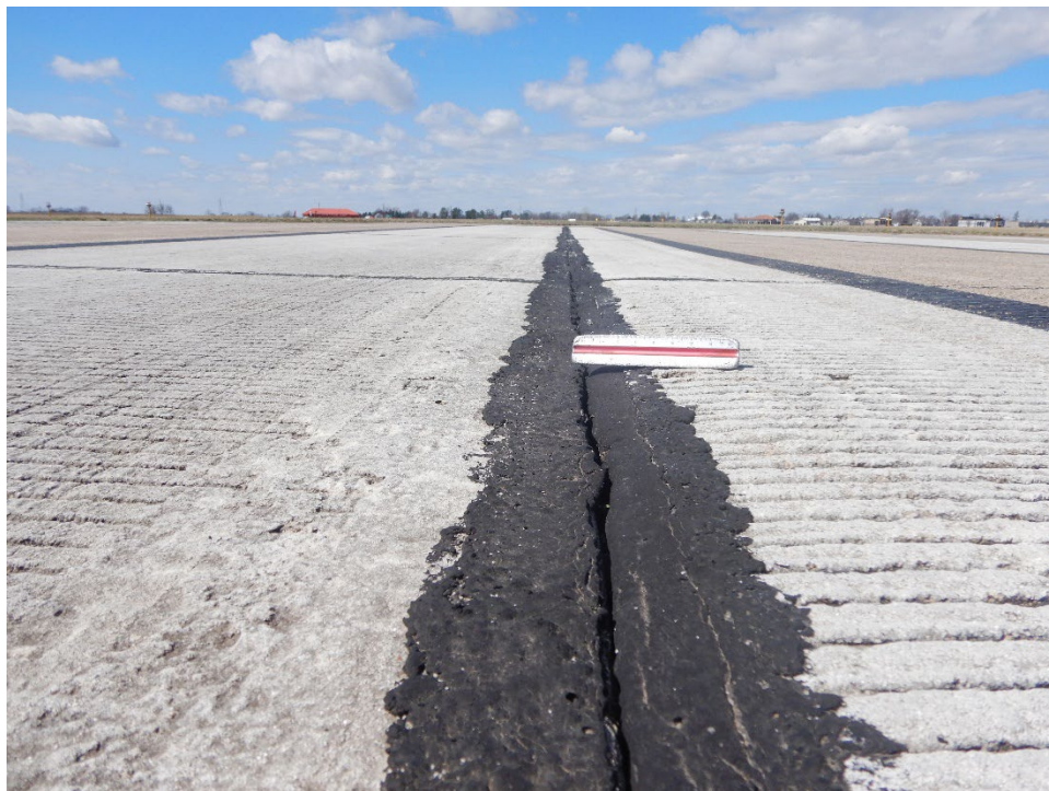
R12BR-01. Faulting (Sample Unit No. 004).
