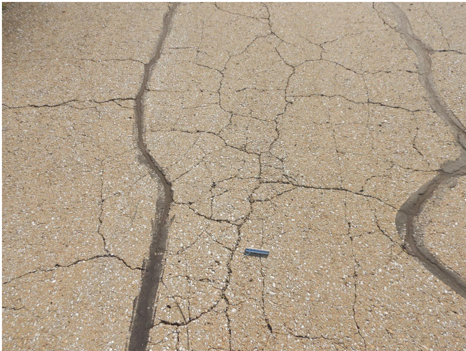
TDBR-04. Alligator Cracking (Sample Unit No. 02).
