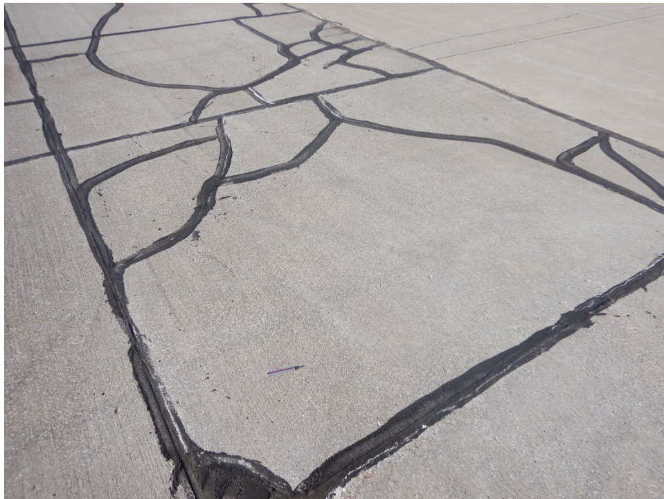
A01BR-02. Shattered Slab (Sample Unit No. 05).
