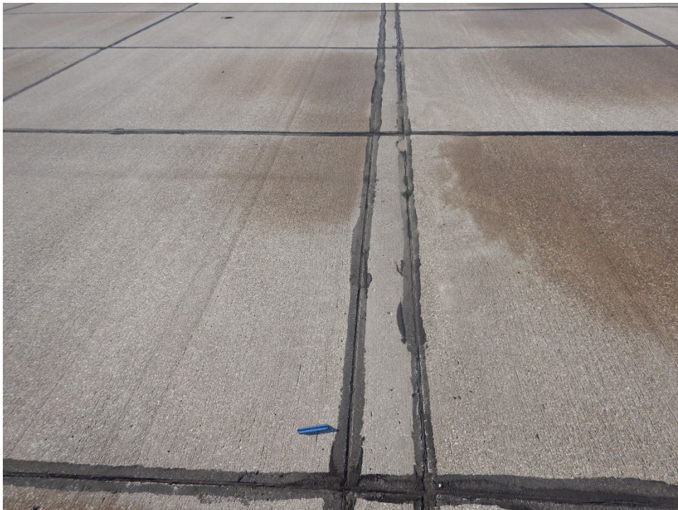
A01BR-02. Large Patching (Sample Unit No. 14).
