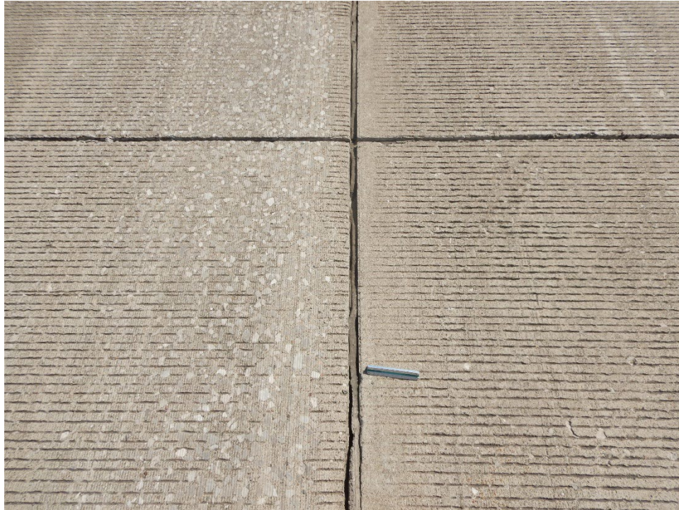
R12BR-01. Joint Seal Damage (Sample Unit No. 153).
