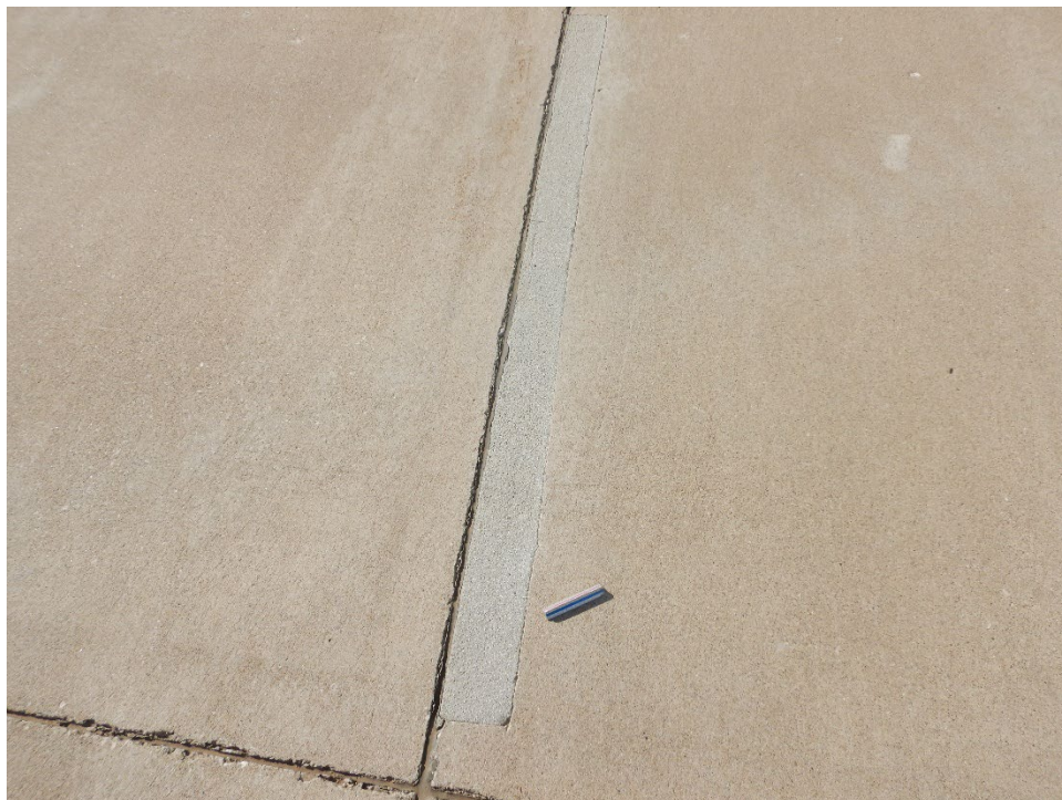
TBBR-02. Small Patching (Sample Unit No. 02).
