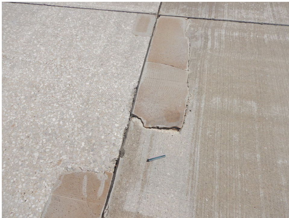
TABR-02. Large Patching (Sample Unit No. 94).
