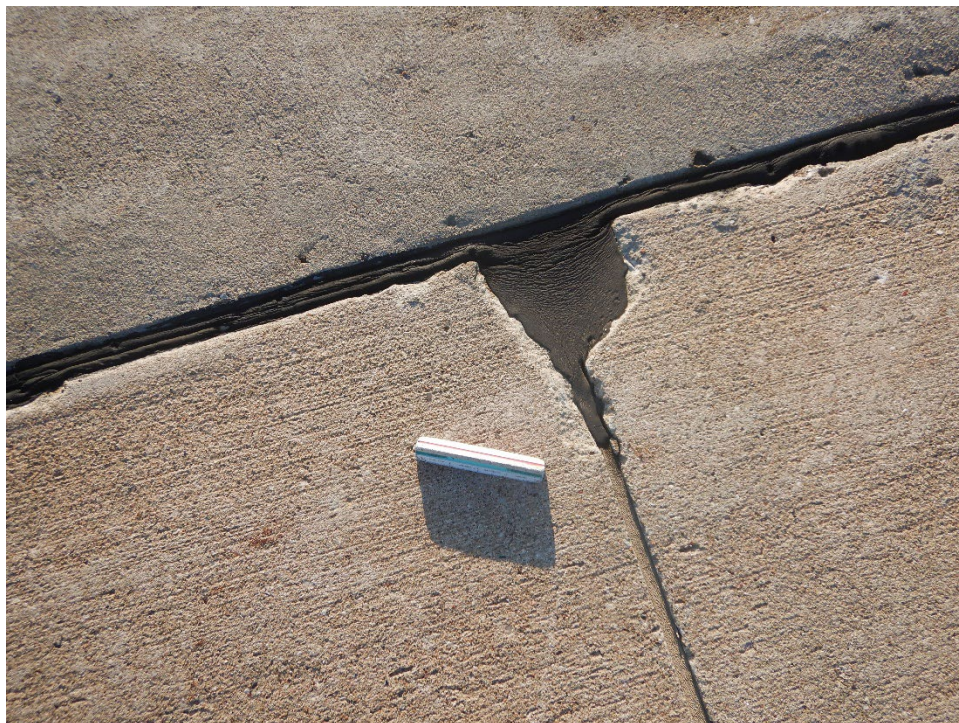
TDBR-03. Corner Spalling (Sample Unit No. 10).
