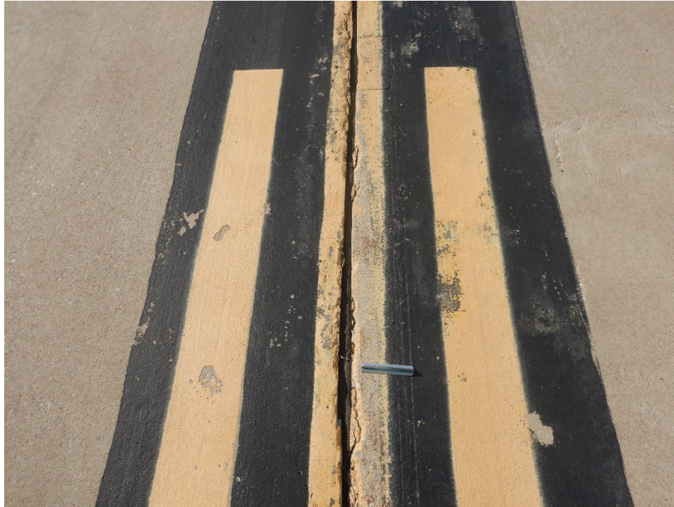
TBBR-02. Joint Seal Damage (Sample Unit No. 02).
