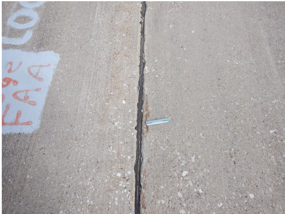
TA3BR-01. Joint Seal Damage (Sample Unit No. 03).
