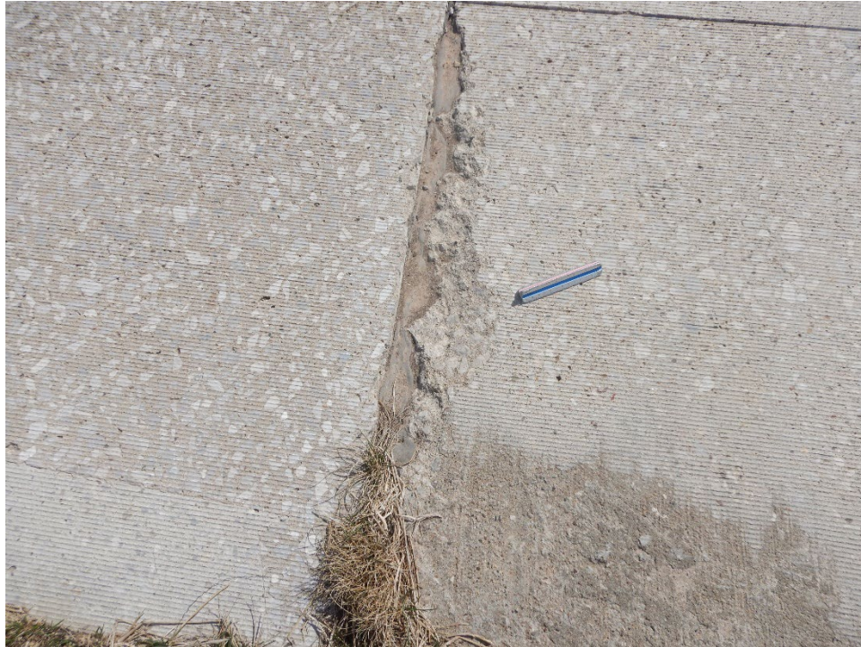
TABR-02. Joint Spalling (Sample Unit No. 94).
