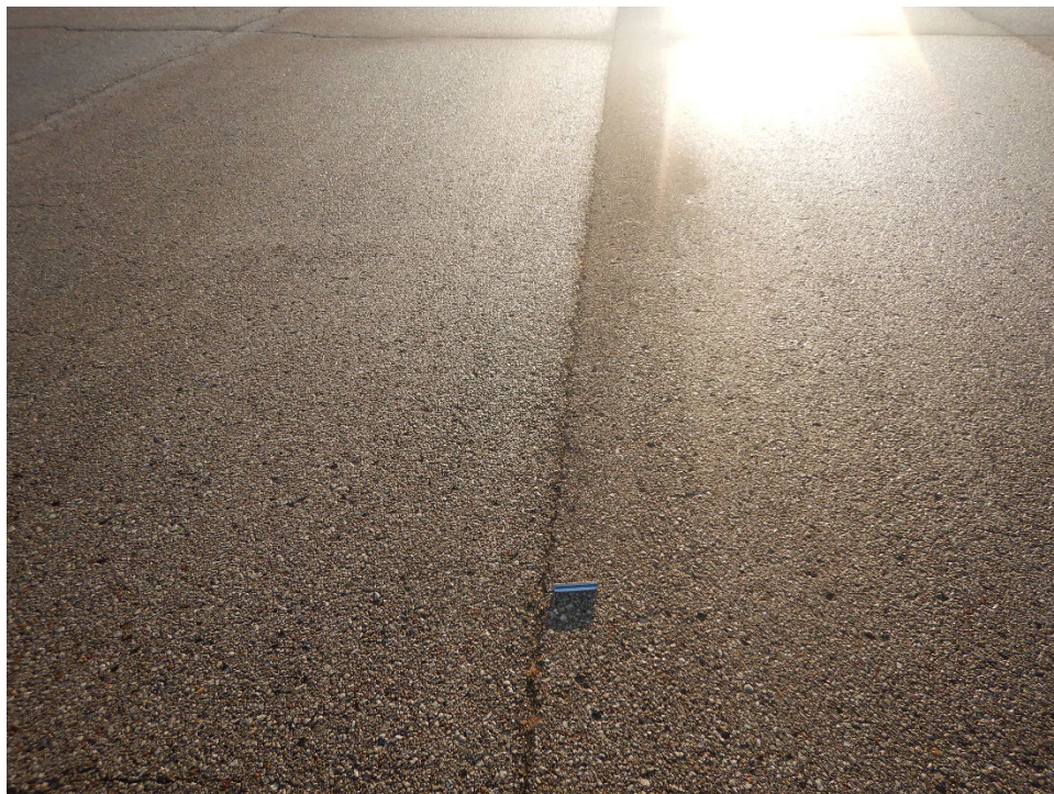
TH01BR-01. L&T Cracking (Sample Unit No. 02).
