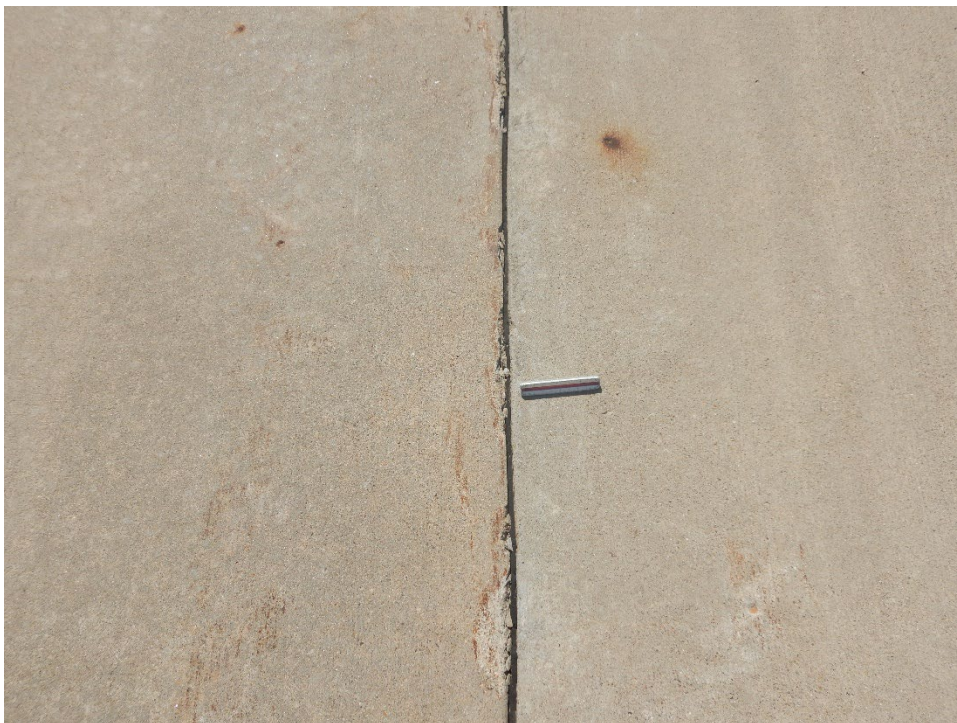
R18BL-02. Joint Seal Damage (Sample Unit No. 33).
