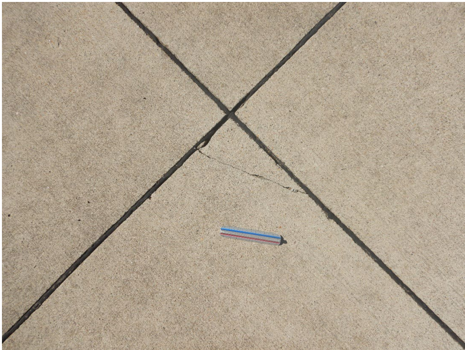
R18BL-01. Corner Spalling (Sample Unit No. 01).
