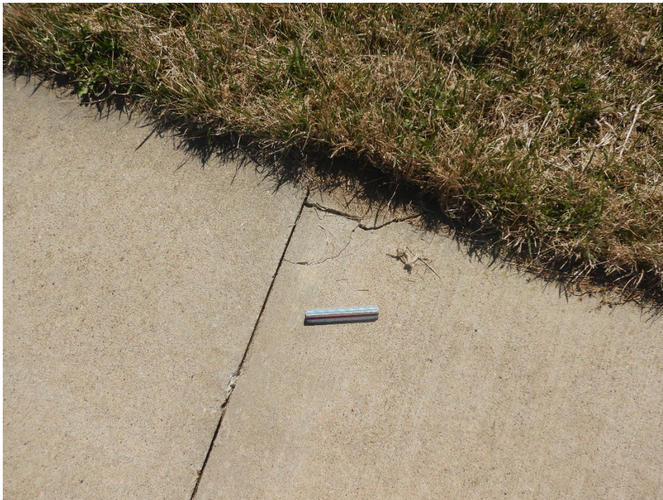
TH01BL-02. Corner Spalling (Sample Unit No. 01).
