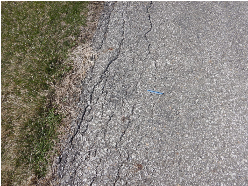
TH01BL-01. Alligator Cracking (Sample Unit No. 01).
