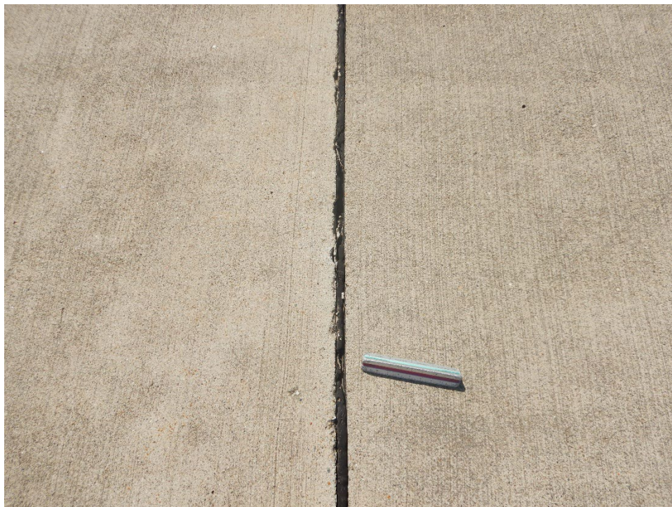
R18BL-01. Joint Seal Damage (Sample Unit No. 04).
