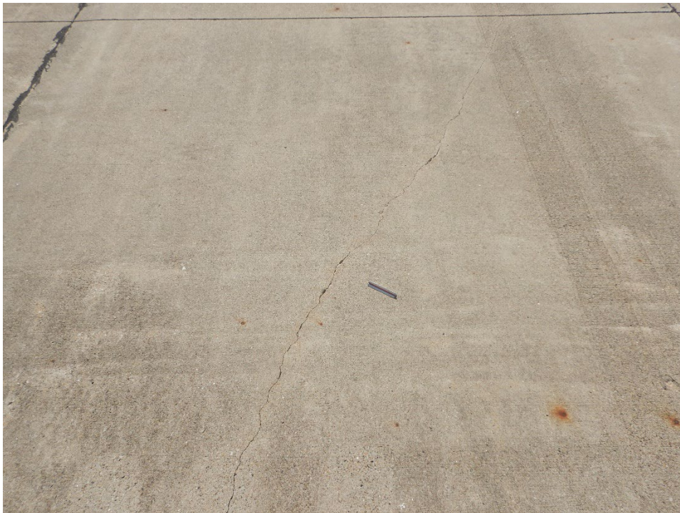
R18BL-03. LTD Cracking (Sample Unit No. 01).
