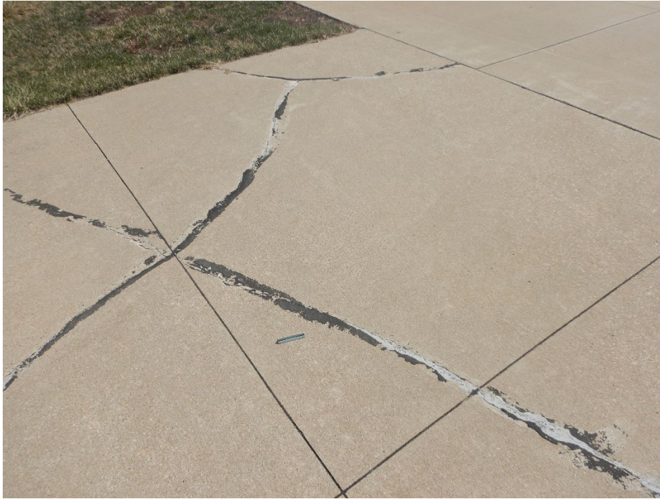
TH01BL-03. Shattered Slab (Sample Unit No. 01).
