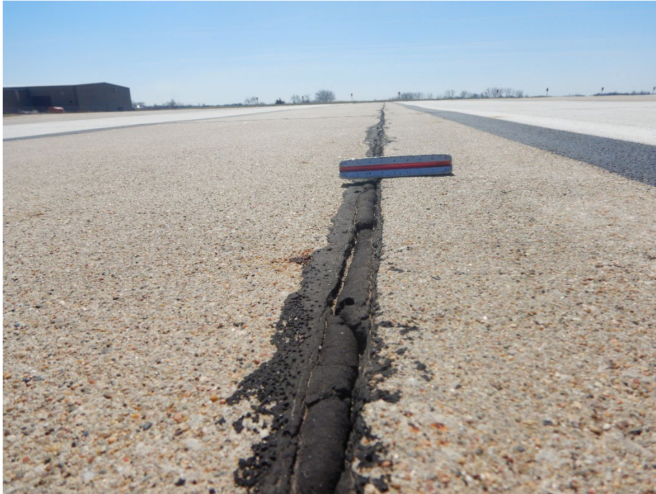
R18BL-03. Faulting (Sample Unit No. 03).
