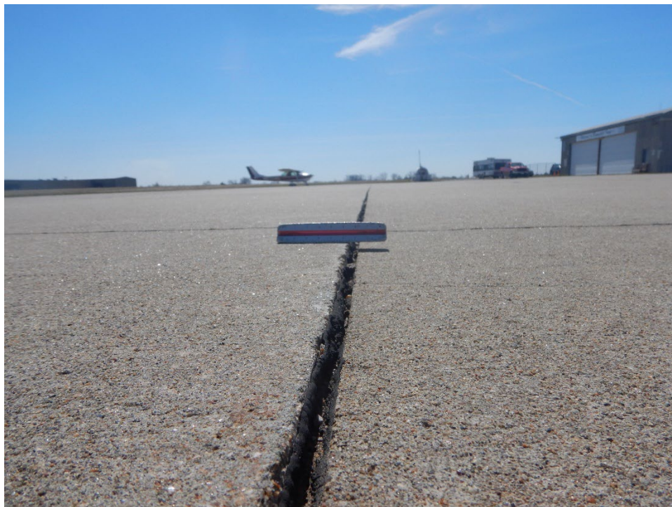
A01BL-01. Faulting (Sample Unit No. 05).
