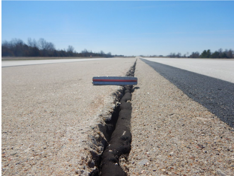
R18BL-01. Faulting (Sample Unit No. 09).
