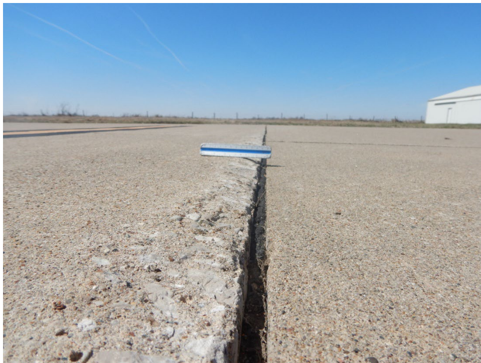
A01BL-02. Faulting (Sample Unit No. 02).
