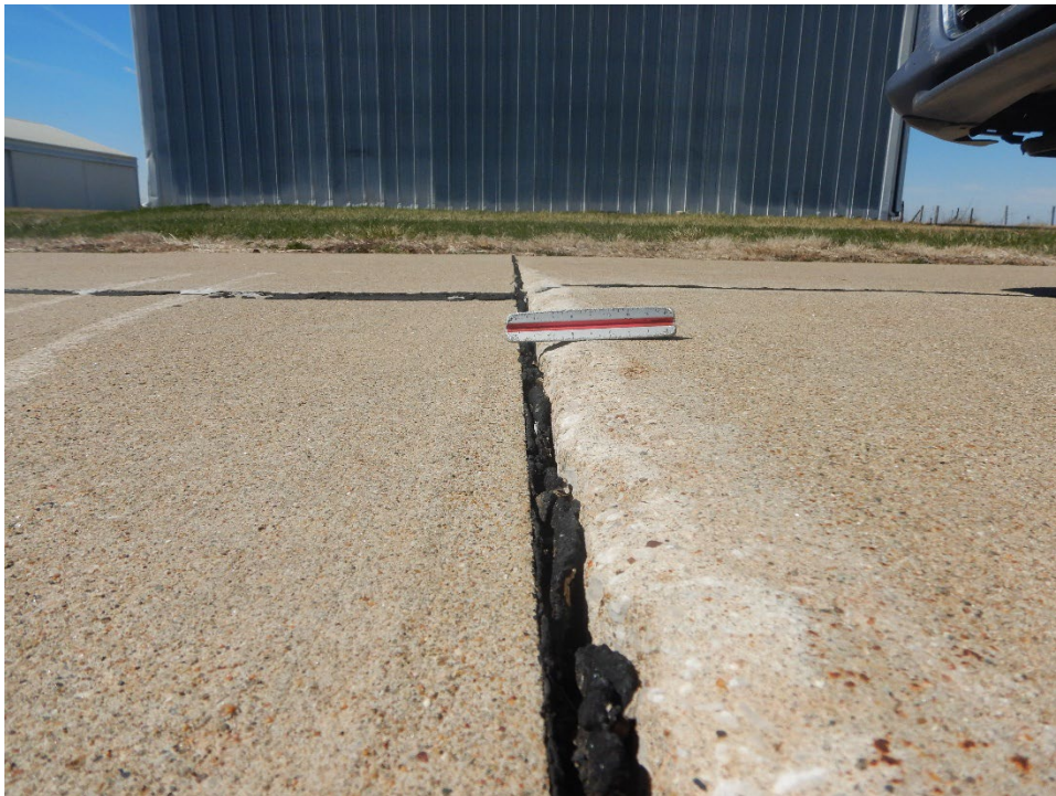
TH01BL-03. Faulting (Sample Unit No. 01).
