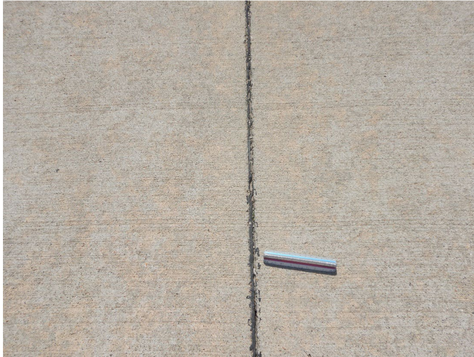
A01BL-01. Joint Seal Damage (Sample Unit No. 06).
