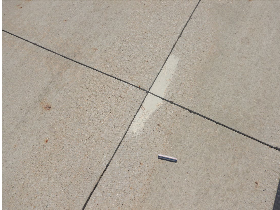
R18BL-02. Small Patching (Sample Unit No. 53).
