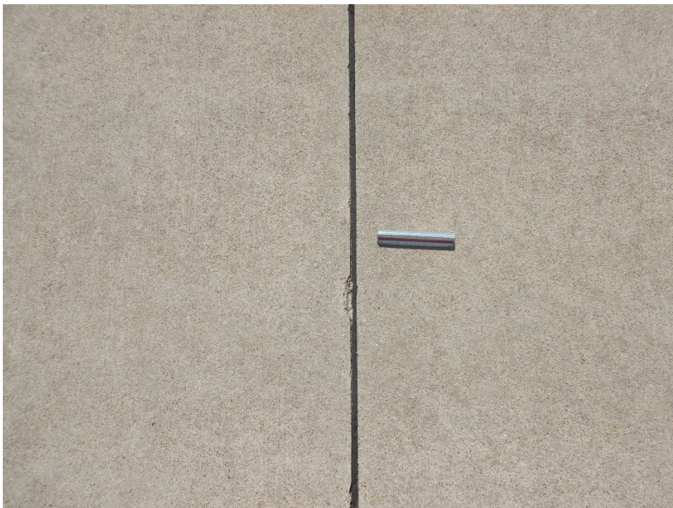
T01BL-01. Joint Seal Damage (Sample Unit No. 01).
