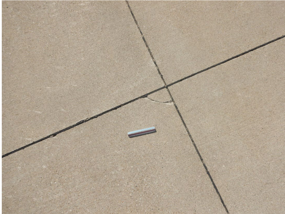
A01BL-02. Corner Spalling (Sample Unit No. 02).
