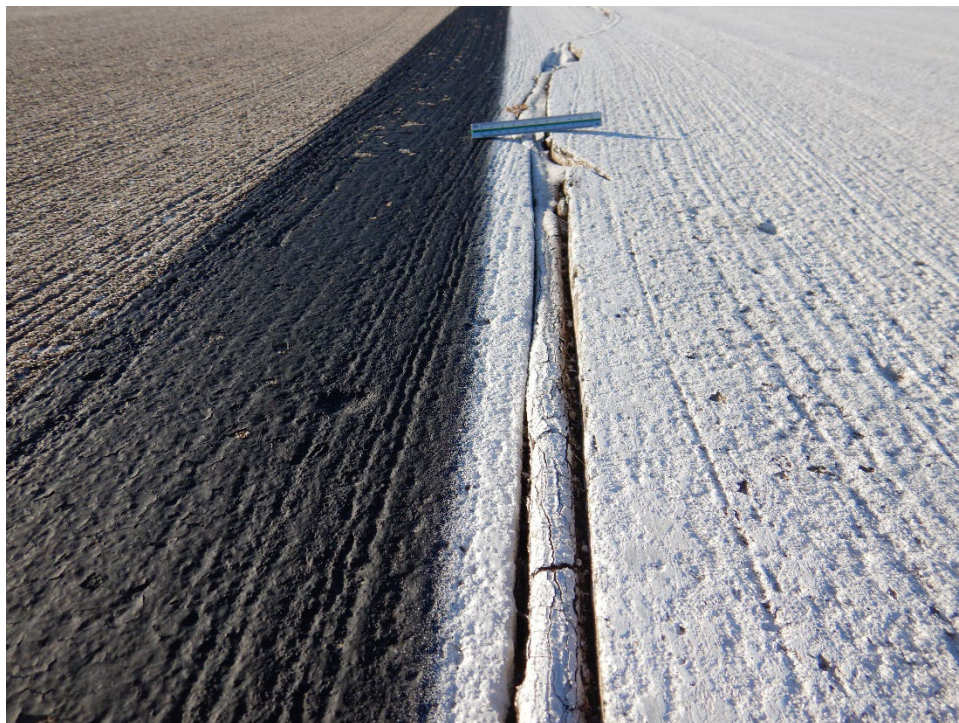
R18BP-01. Faulting (Sample Unit No. 75).
