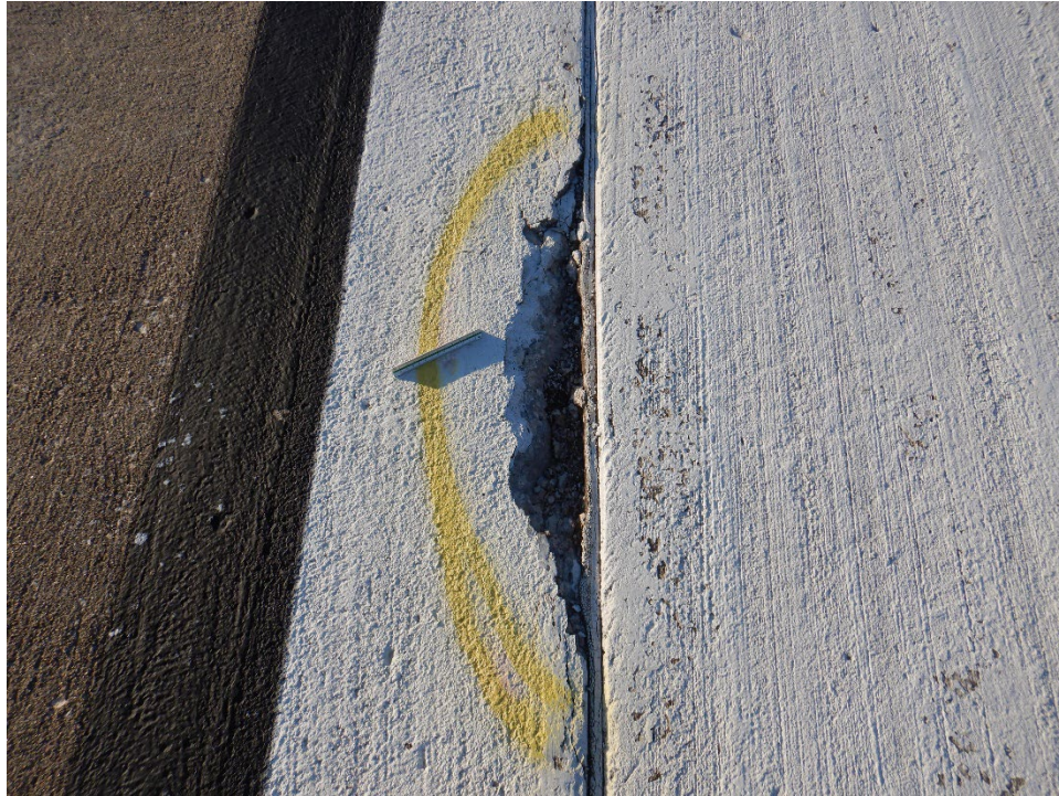
R18BP-01. Joint Spalling (Sample Unit No. 95).
