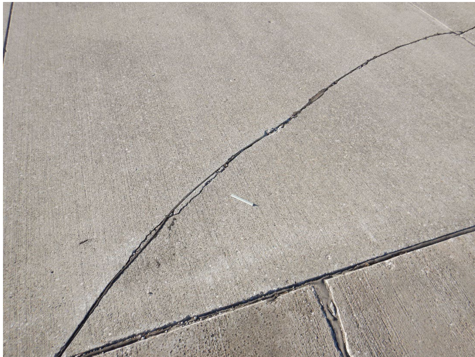
TH01BP-02. LTD Cracking (Sample Unit No. 01).
