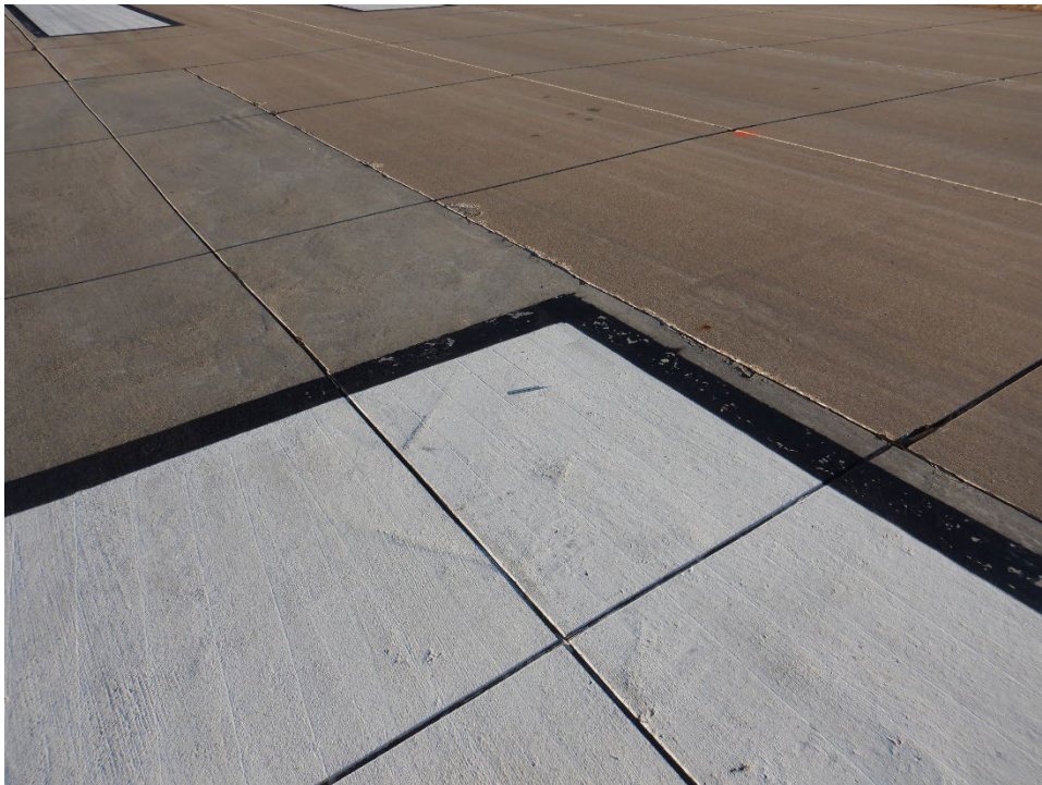
R18BP-01. Large Patching (Sample Unit No. 95).
