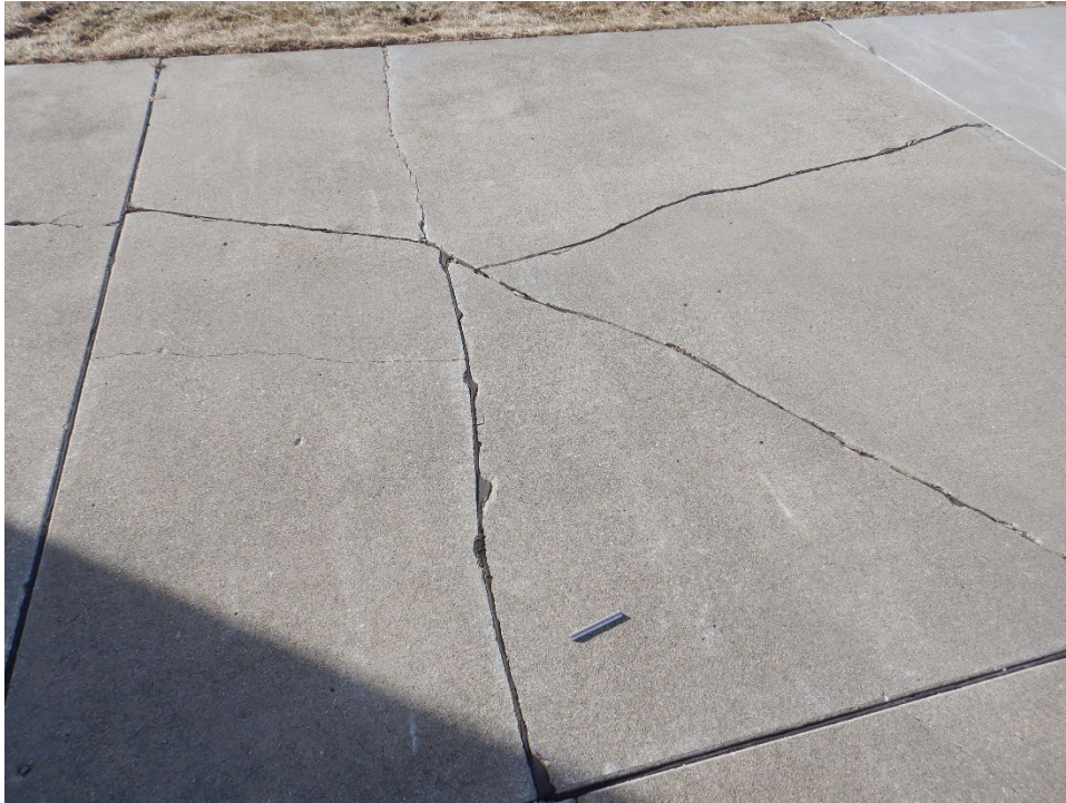
TH01BP-01. Shattered Slab (Sample Unit No. 01).
