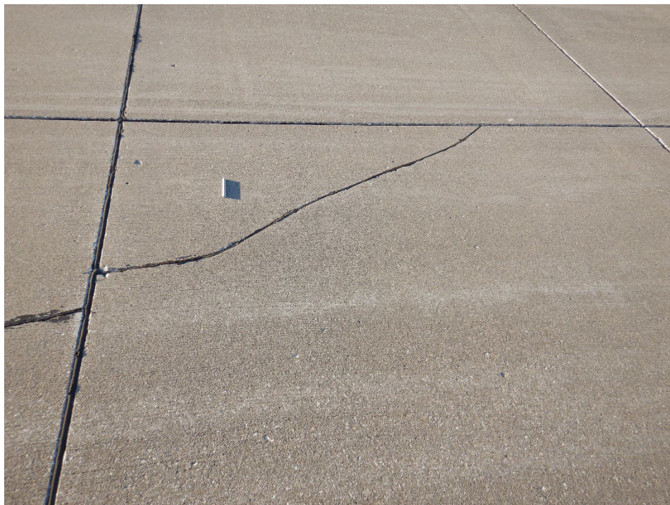
R18BP-01. LTD Cracking (Sample Unit No. 102).
