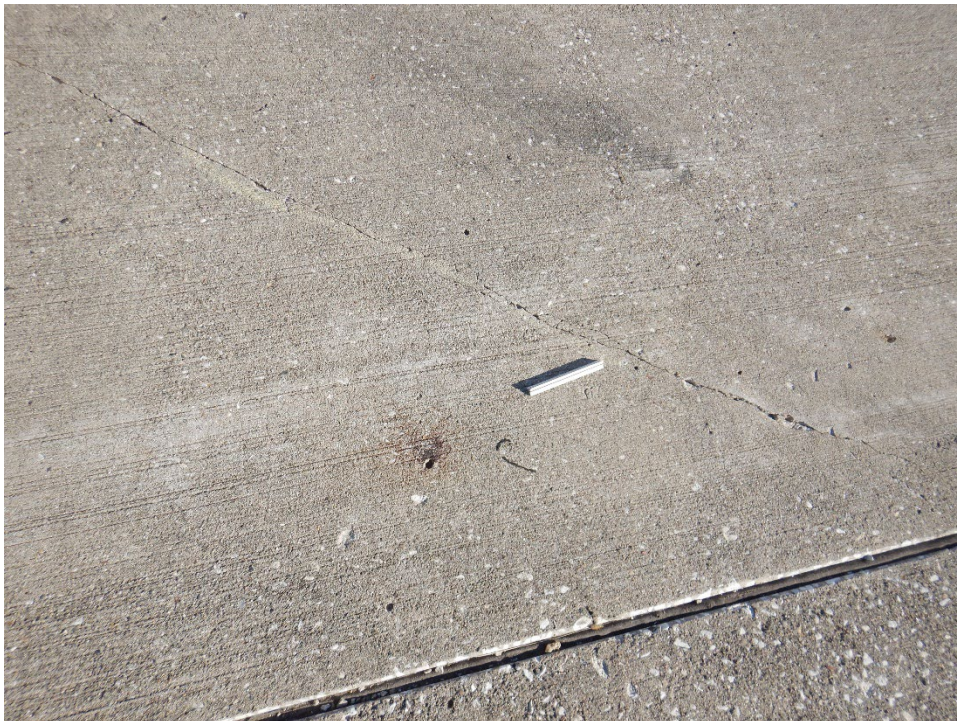
T01BP-01. LTD Cracking (Sample Unit No. 04).
