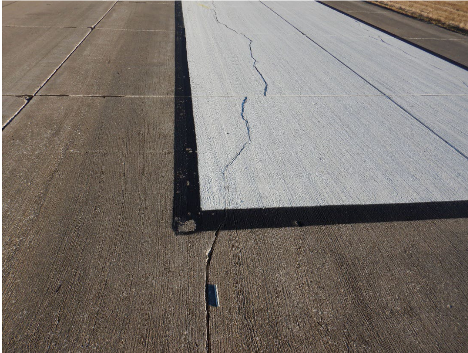
R18BP-01. LTD Cracking (Sample Unit No. 75).
