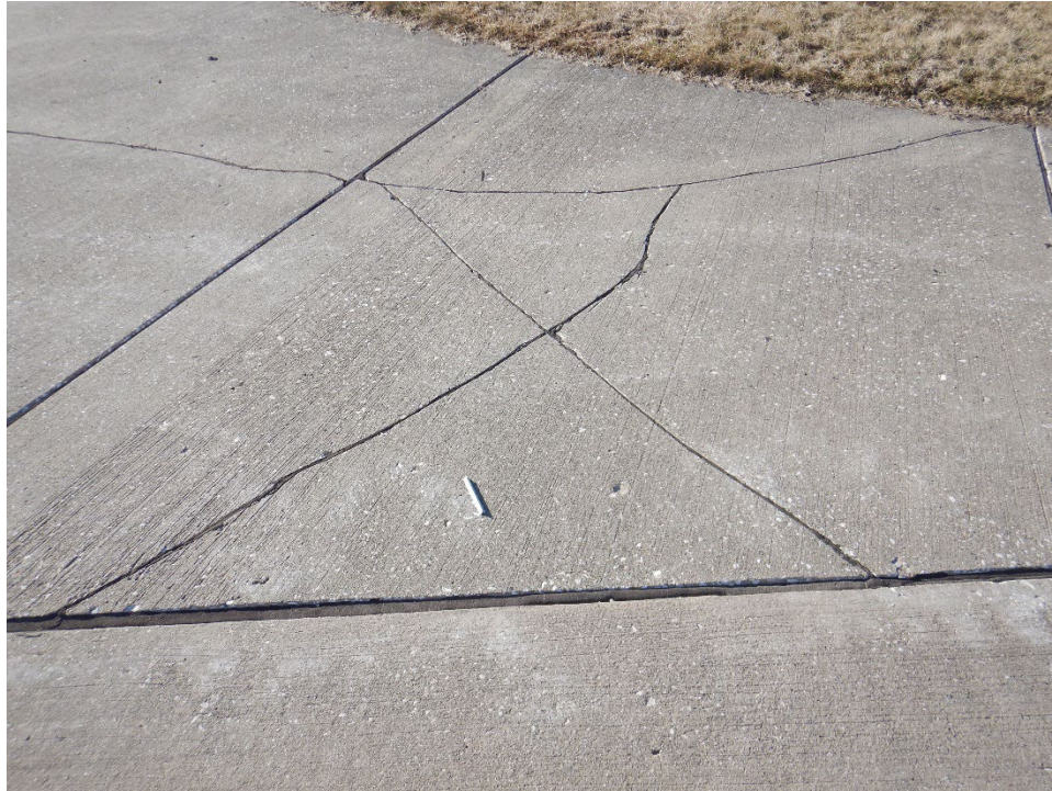
T01BP-01. Shattered Slab (Sample Unit No. 01).
