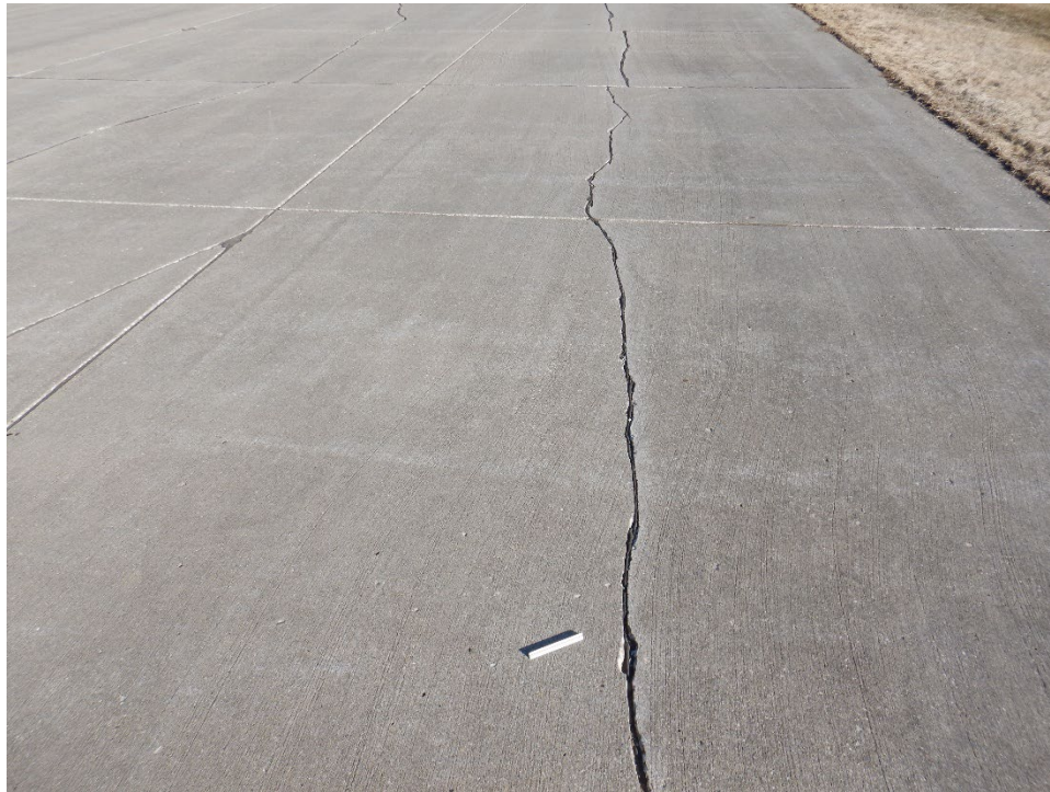
A01BP-01. LTD Cracking (Sample Unit No. 20).
