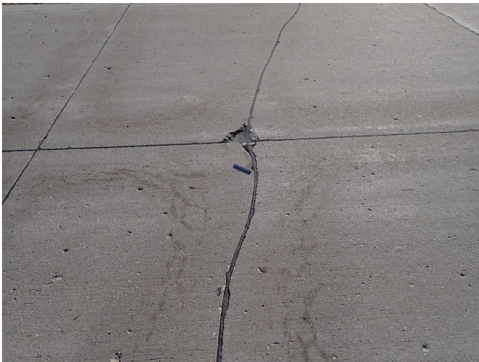
T02AN-01. LTD Cracking (Sample Unit No. 03).
