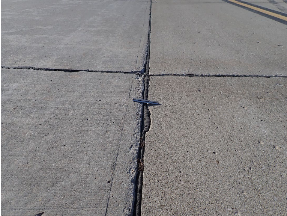
T02AN-01. Faulting (Sample Unit No. 12).
