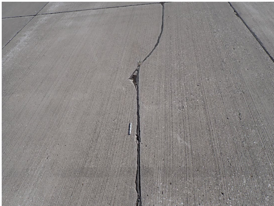
T08AN-01. LTD Cracking (Sample Unit No. 03).
