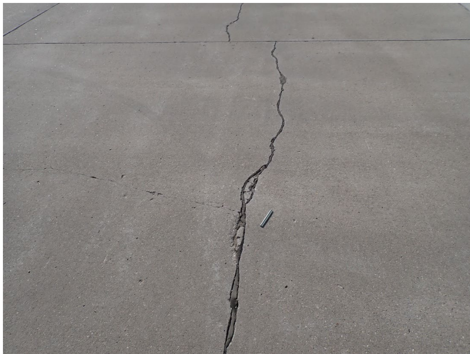
TH01AN-02. LTD Cracking (Sample Unit No. 18).
