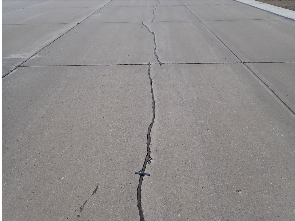
R18AN-02. LTD Cracking (Sample Unit No. 31).
