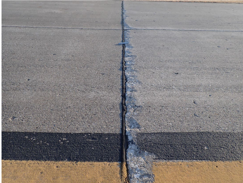
T09AN-01. Faulting (Sample Unit No. 07).
