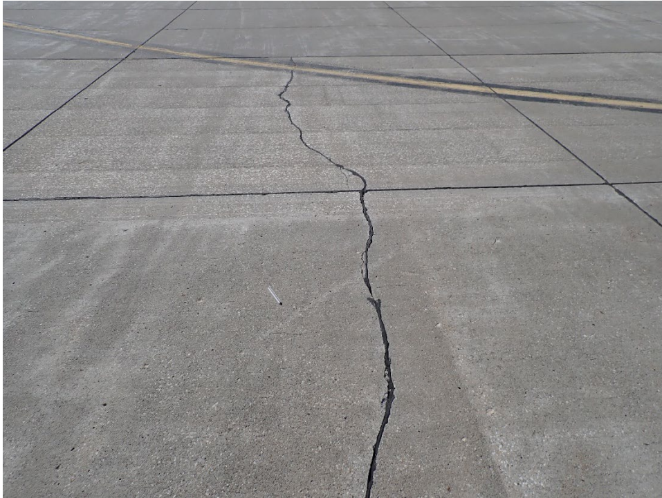
T05AN-01. LTD Cracking (Sample Unit No. 05).
