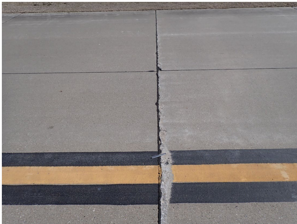
T12AN-01. Faulting (Sample Unit No. 09).
