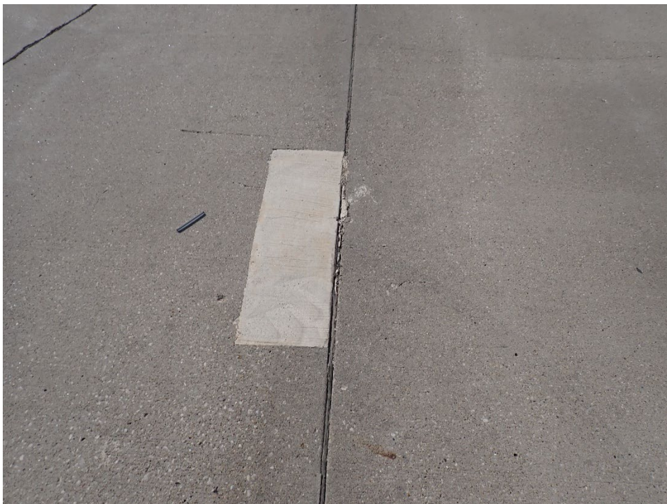
TH01AN-02. Small Patching (Sample Unit No. 18).
