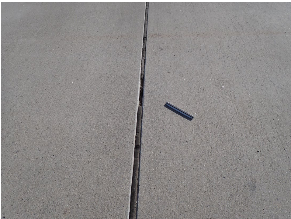
TH01AN-04. Joint Seal Damage (Sample Unit No. 07).
