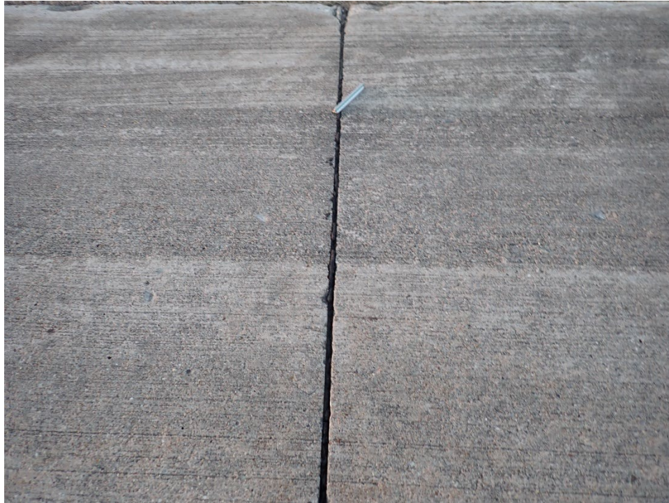
T01AN-01. Joint Seal Damage (Sample Unit No. 10).
