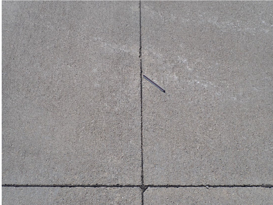
A01AN-03. Joint Seal Damage (Sample Unit No. 08).
