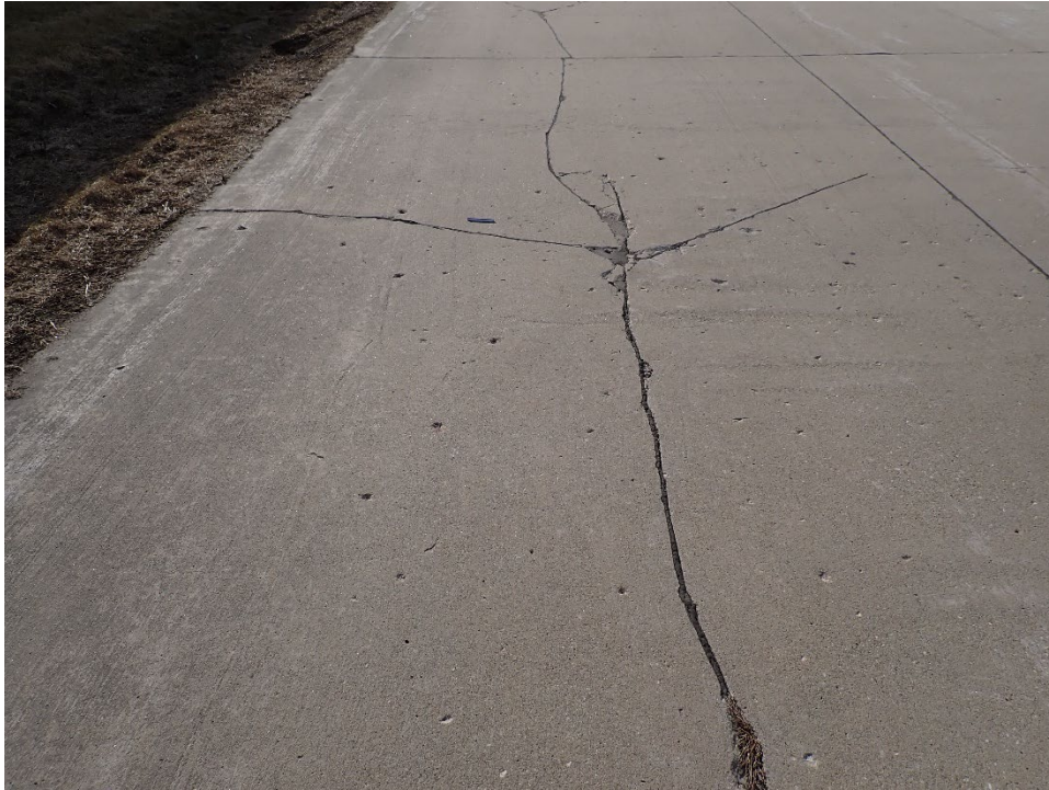
TH01AN-02. Shattered Slab (Sample Unit No. 02).
