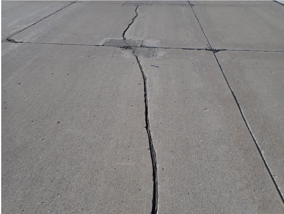
R18AN-01. LTD Cracking (Sample Unit No. 63).
