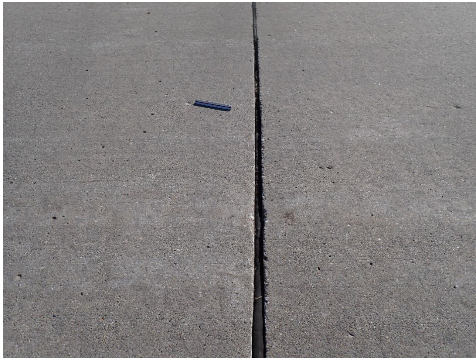
T04AN-01. Joint Seal Damage (Sample Unit No. 03).
