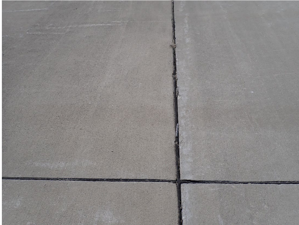
A02AN-01. Joint Seal Damage (Sample Unit No. 09).
