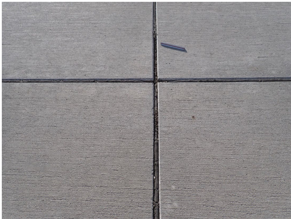
T01AN-01. Joint Seal Damage (Sample Unit No. 14).
