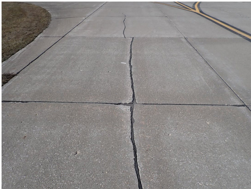
T03AN-01. LTD Cracking (Sample Unit No. 01).
