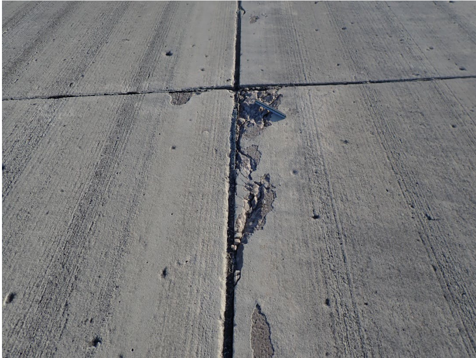
R04AN-01. Joint Spalling (Sample Unit No. 21).
