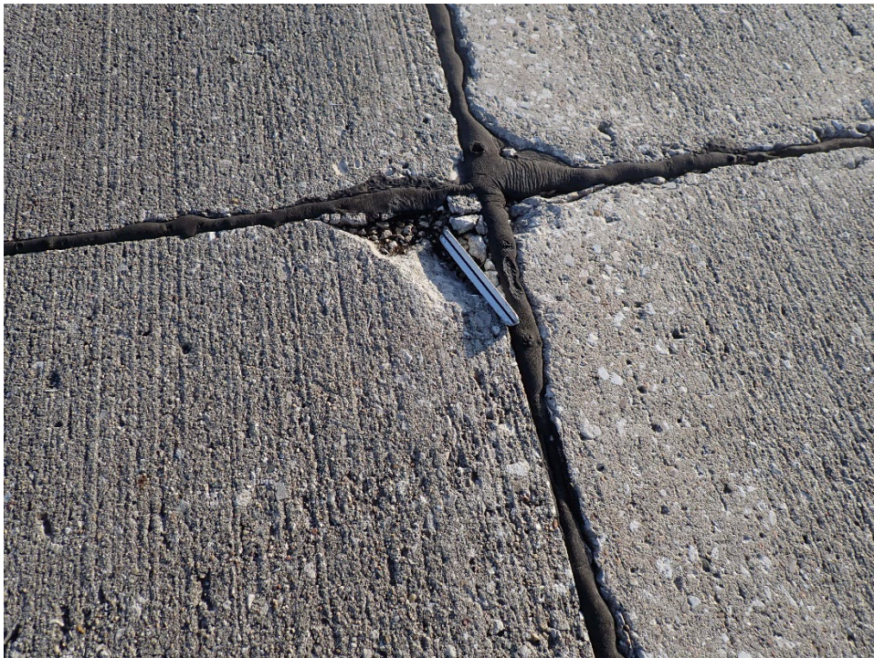
R04AN-01. Corner Spalling (Sample Unit No. 13).
