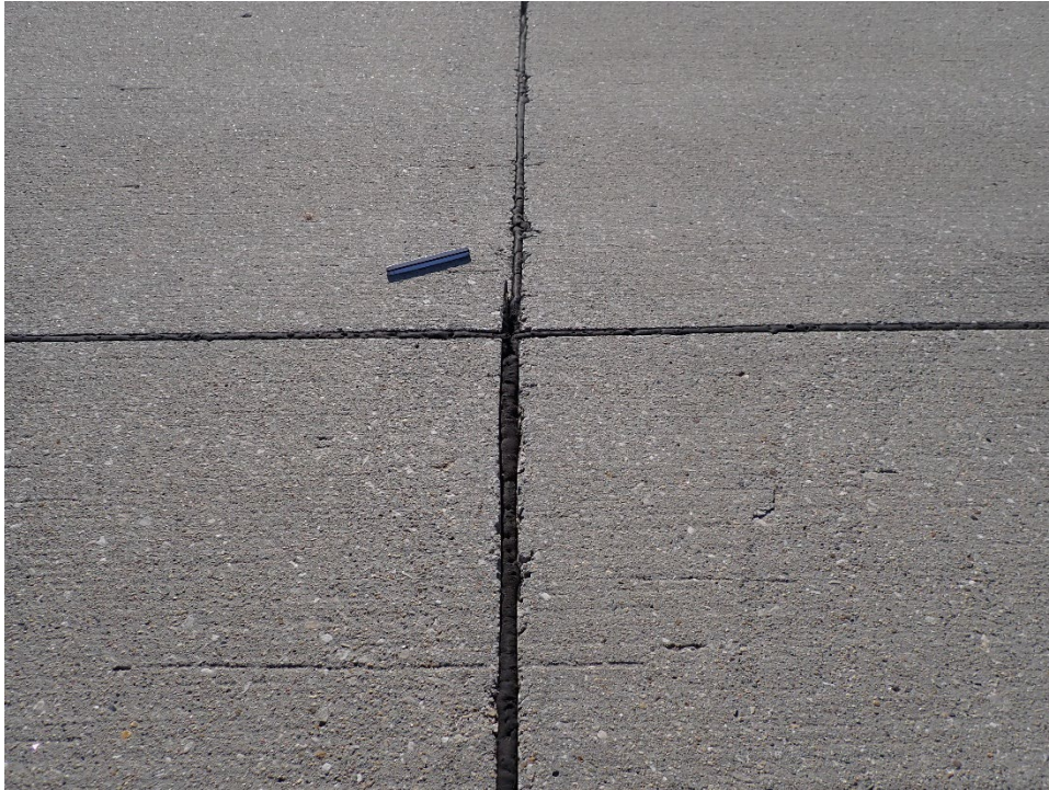
T12AN-01. Joint Seal Damage (Sample Unit No. 03).
