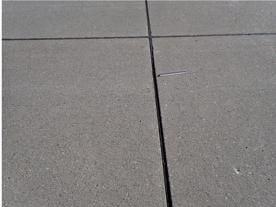
T06AN-01. Joint Seal Damage (Sample Unit No. 02).
