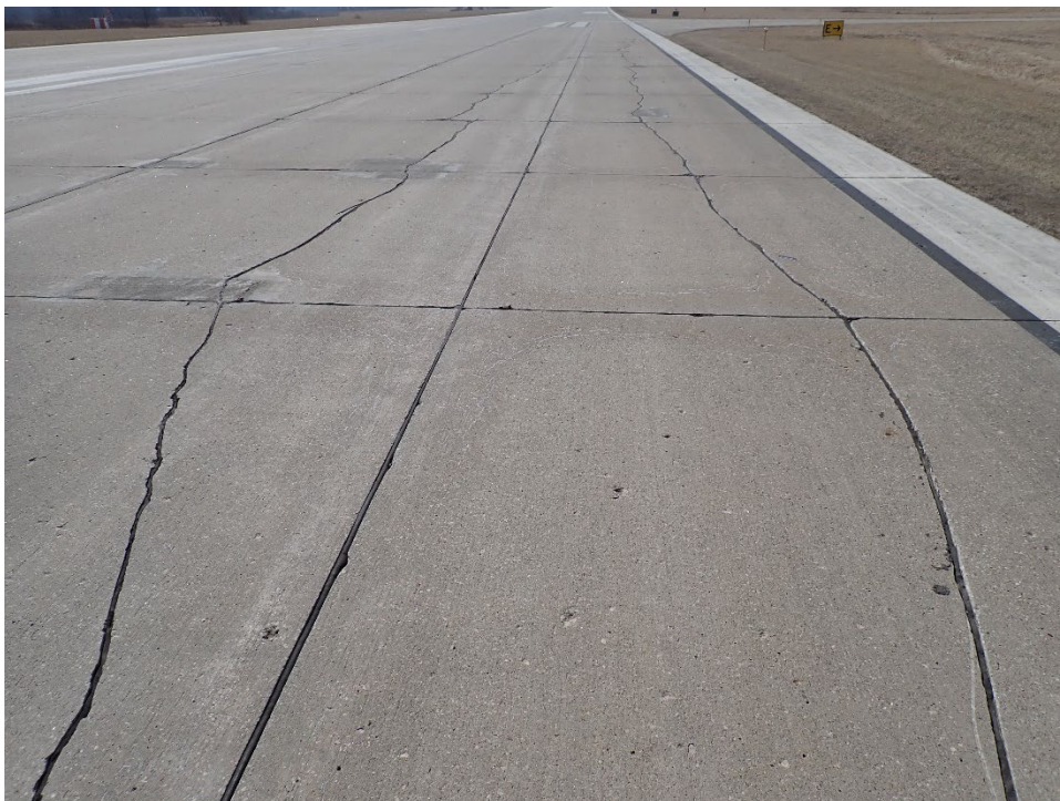
R18AN-01. LTD Cracking (Sample Unit No. 99).
