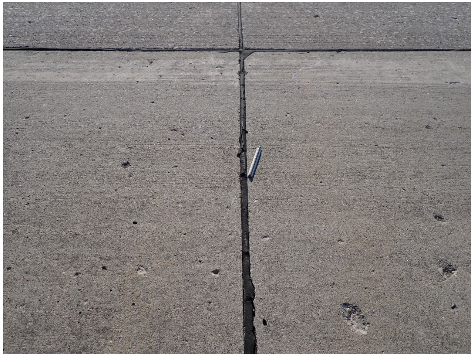
R04AN-02. Joint Seal Damage (Sample Unit No. 04).
