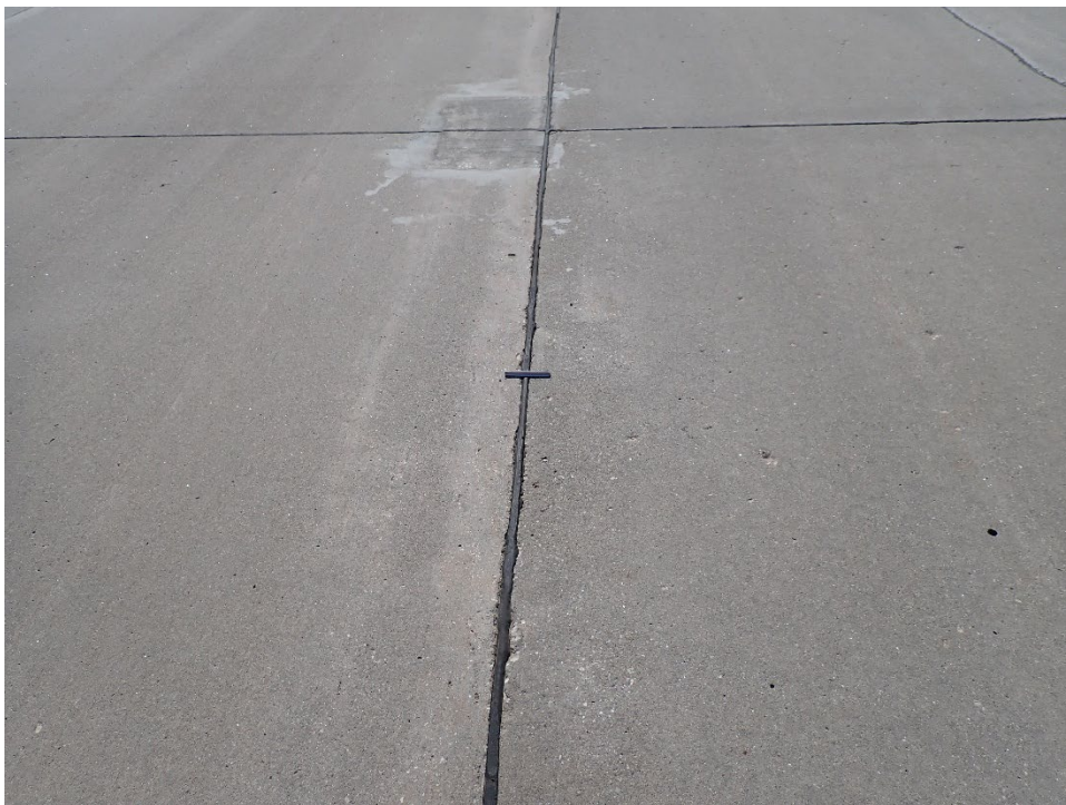
R18AN-02. Joint Seal Damage (Sample Unit No. 31).
