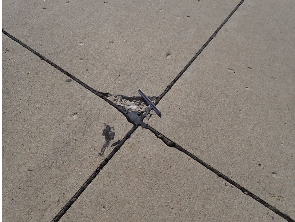
TH01AN-01. Corner Spalling (Sample Unit No. 09).
