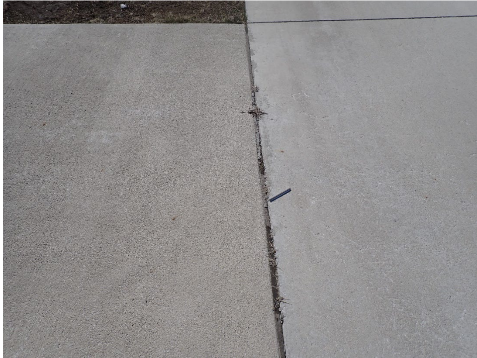
A02AN-02. Joint Seal Damage (Sample Unit No. 09).
