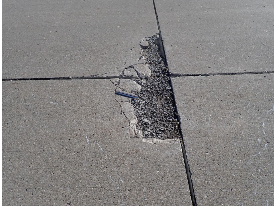
T04AN-01. Small Patching (Additional Sample Unit No. 18).
