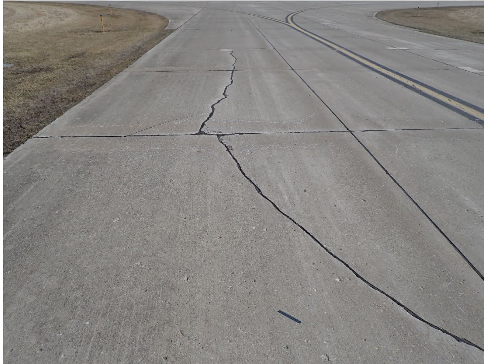
T03AN-01. LTD Cracking (Sample Unit No. 04).
