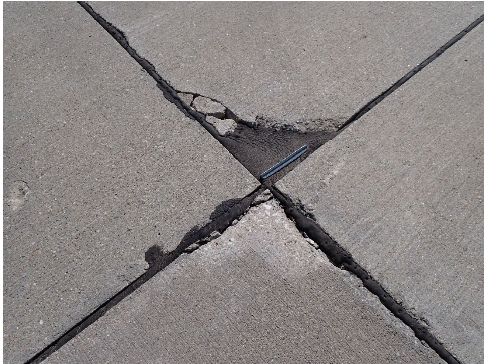
T12AN-01. Corner Spalling (Sample Unit No. 18).
