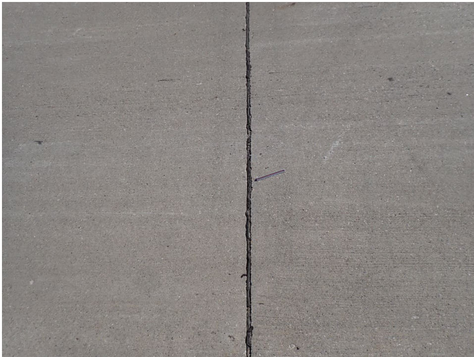
T12AN-01. Joint Seal Damage (Sample Unit No. 21).
