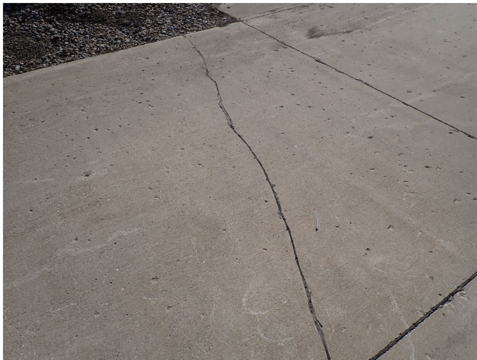
TH01AN-01. LTD Cracking (Sample Unit No. 09).
