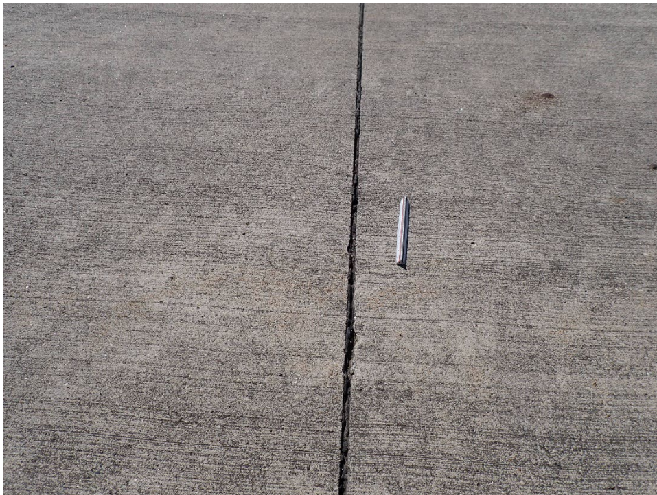
T13AN-01. Joint Seal Damage (Sample Unit No. 03).
