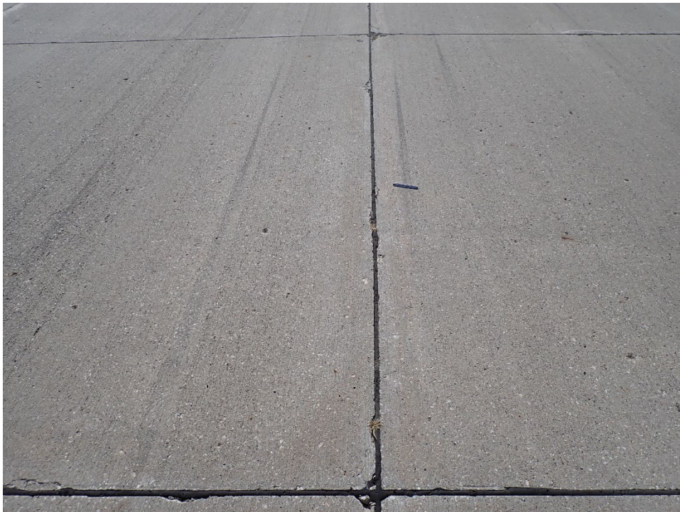
R04AN-04. Joint Seal Damage (Sample Unit No. 28).
