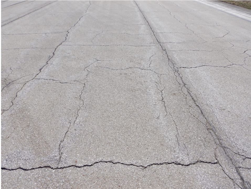
R01AM-01. Block Cracking (Sample Unit No. 91).
