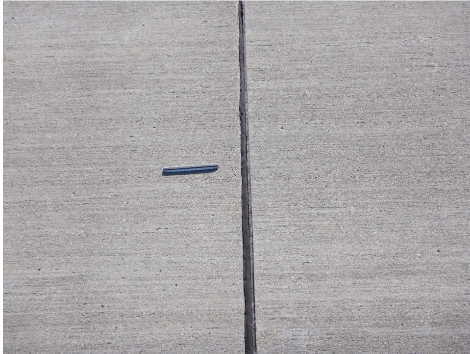
TAAM-07. Joint Seal Damage (Sample Unit No. 03).
