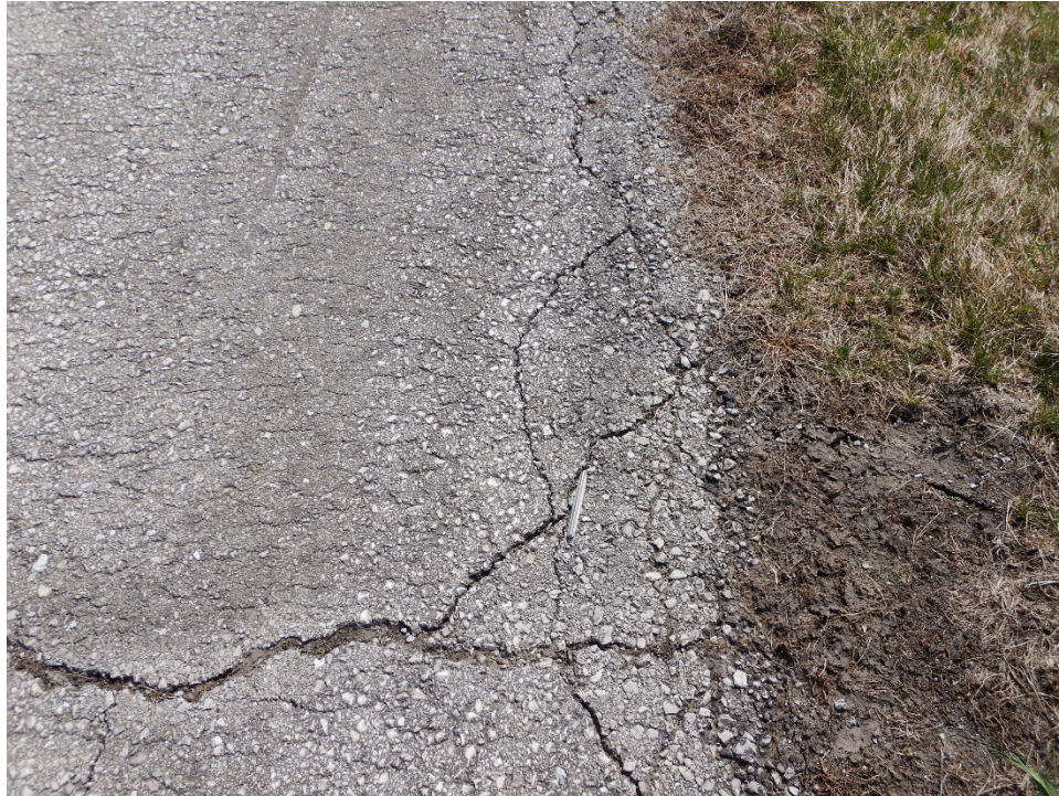
TBAM-04. Alligator Cracking (Sample Unit No. 02).
