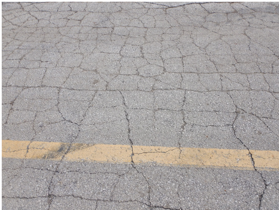
TH01AM-01. Alligator Cracking (Sample Unit No. 02).
