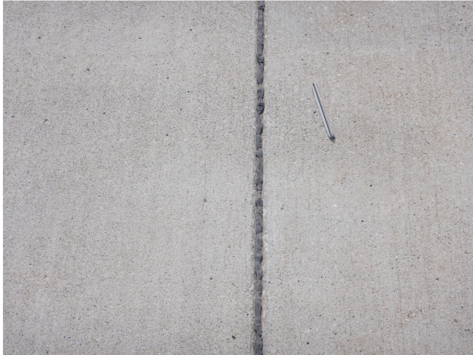
A01AM-02. Joint Seal Damage (Sample Unit No. 64).
