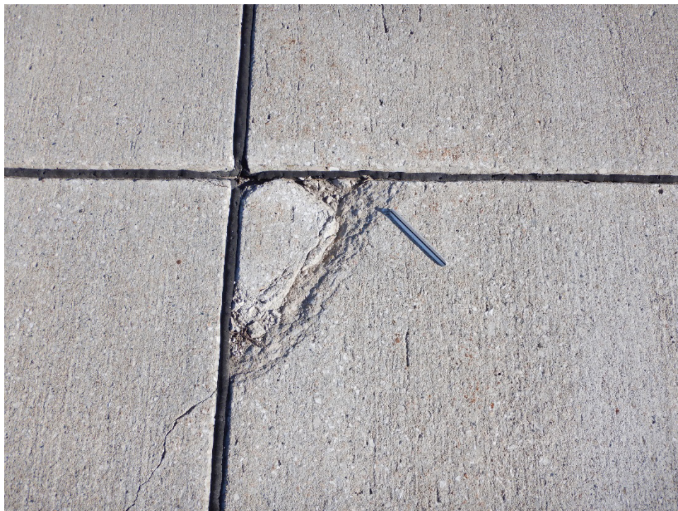
R13AM-04. Corner Spalling (Additional Sample Unit No. 05).
