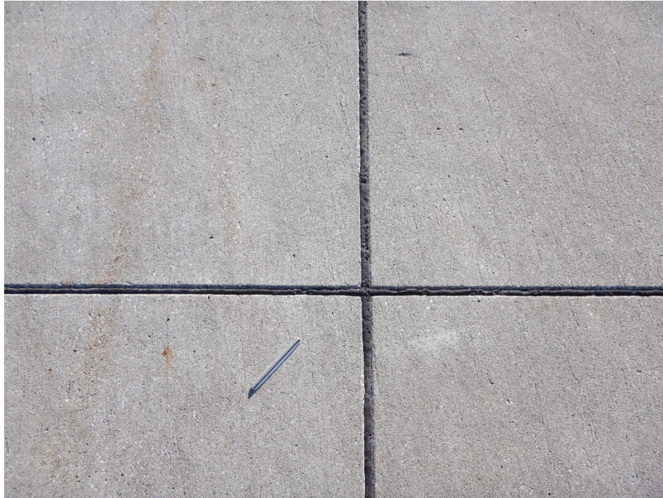
TB3AM-01. Joint Seal Damage (Sample Unit No. 02).
