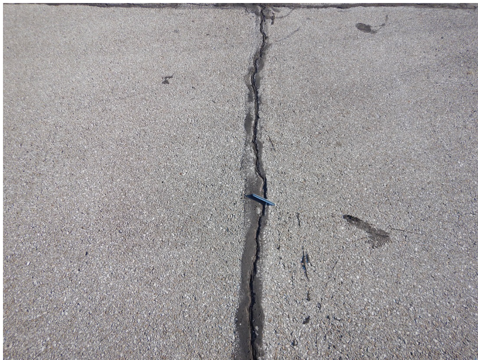
TA3AM-02. L&T Cracking (Sample Unit No. 01) (2).
