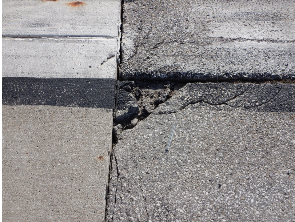
R13AM-03. L&T Cracking (Sample Unit No. 01) (2).
