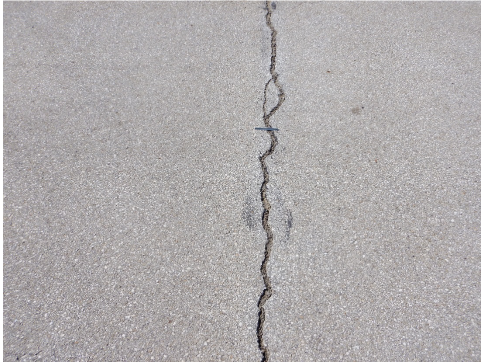
TA4AM-02. L&T Cracking (Sample Unit No. 01) (2).
