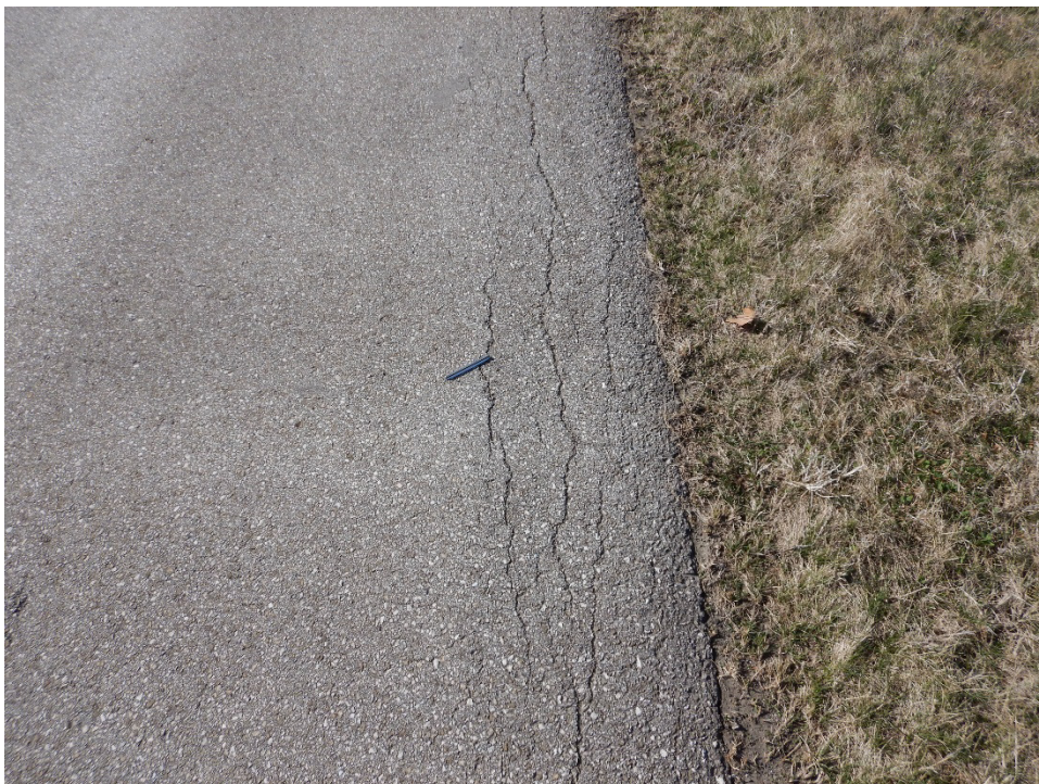
TAAM-04. Alligator Cracking (Sample Unit No. 05).
