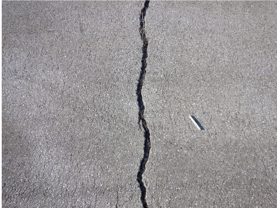
TA2AM-01. L&T Cracking (Sample Unit No. 01).
