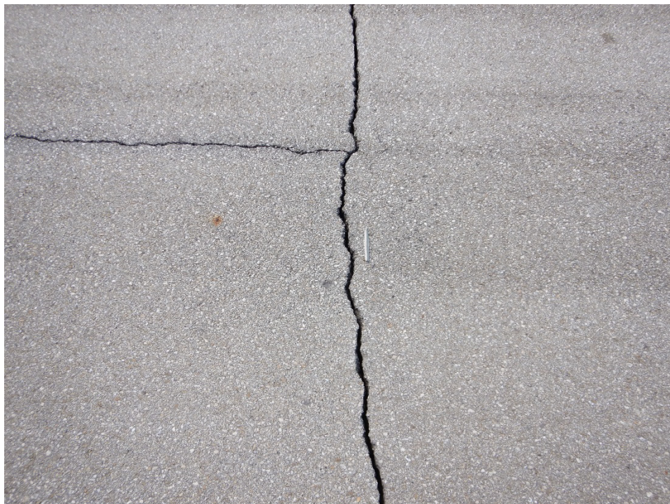
TBAM-03. L&T Cracking (Sample Unit No. 01).
