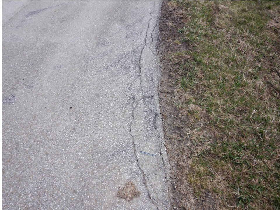
TBAM-03. Alligator Cracking (Sample Unit No. 01).
