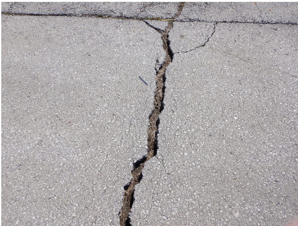
TB2AM-01. L&T Cracking (Sample Unit No. 01).
