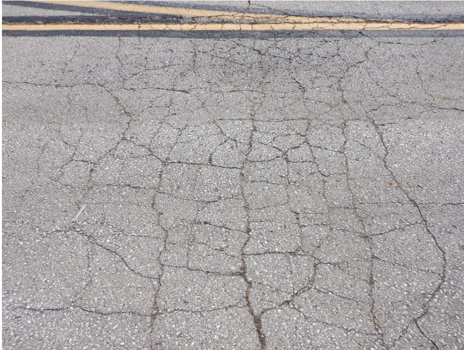
TB2AM-01. Alligator Cracking (Sample Unit No. 01).
