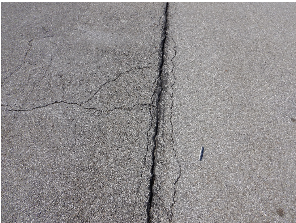
TAAM-03. L&T Cracking (Sample Unit No. 01).
