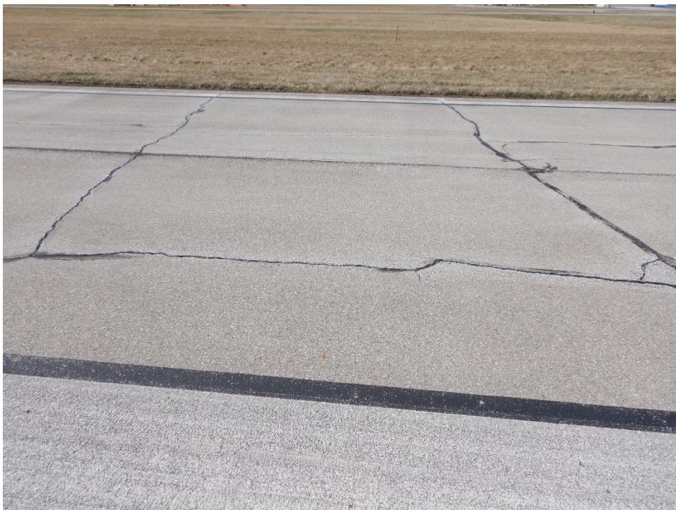
R01AM-01. Joint Reflection Cracking (Sample Unit No. 109).
