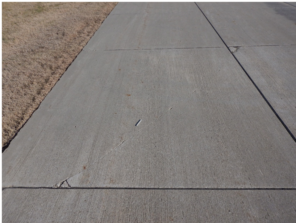
R13AM-04. LTD Cracking (Additional Sample Unit No. 05).
