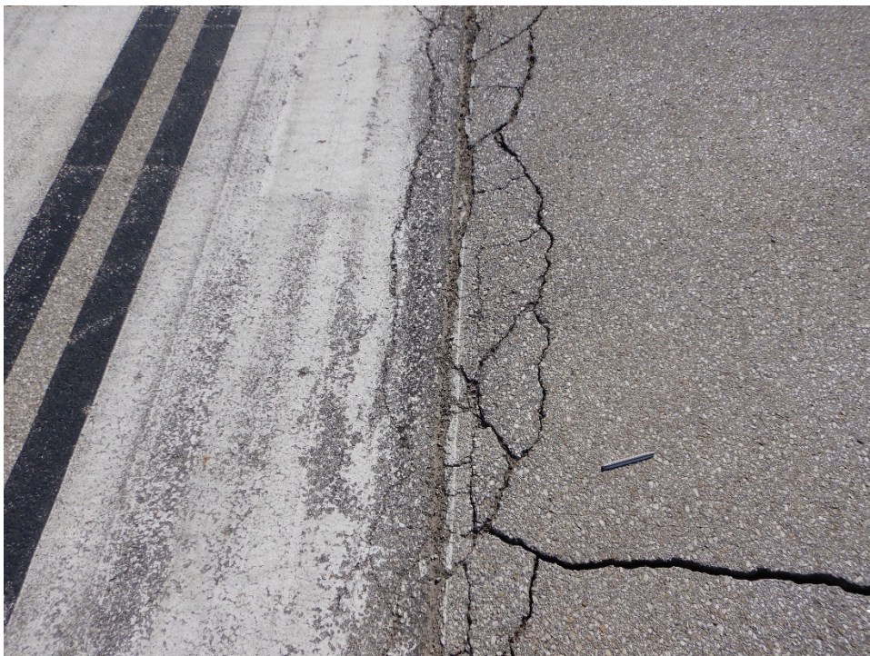
TA4AM-02. L&T Cracking (Sample Unit No. 01) (1).
