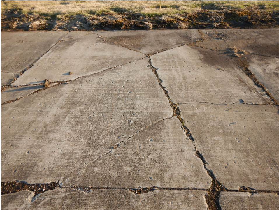
TAAM-10. Shattered Slab (Additional Sample Unit No. 07) (2).
