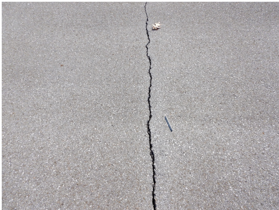
TAAM-04. L&T Cracking (Sample Unit No. 05).
