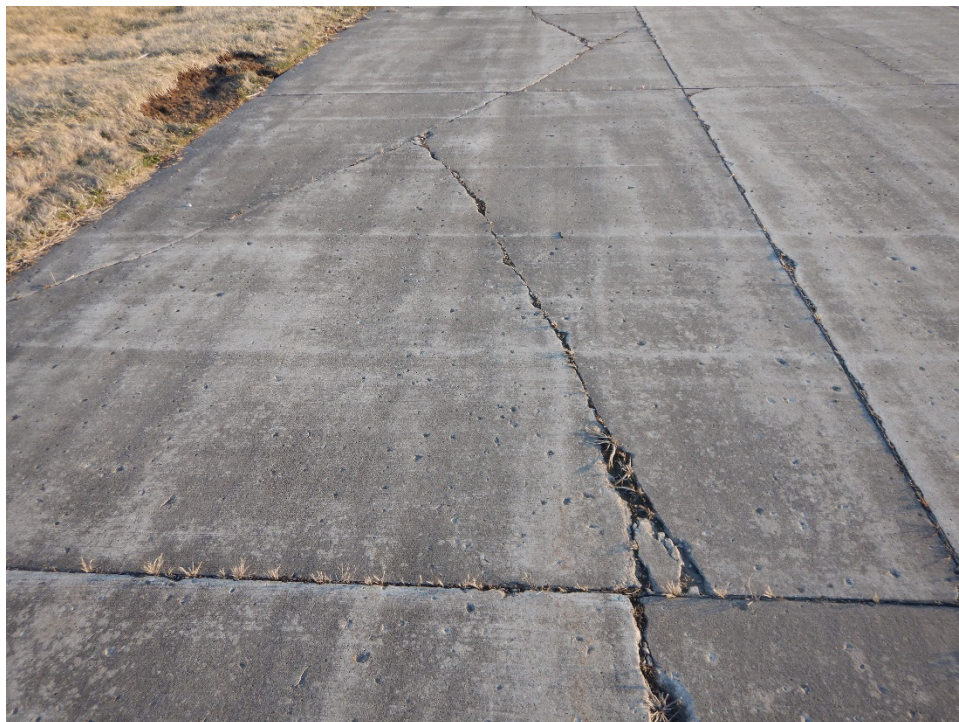
TAAM-10. LTD Cracking (Sample Unit No. 06).
