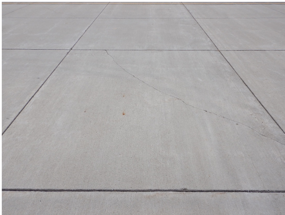
A01AM-02. LTD Cracking (Sample Unit No. 14).
