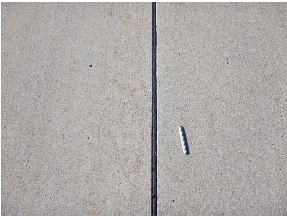
R13AM-01. Joint Seal Damage (Sample Unit No. 12).
