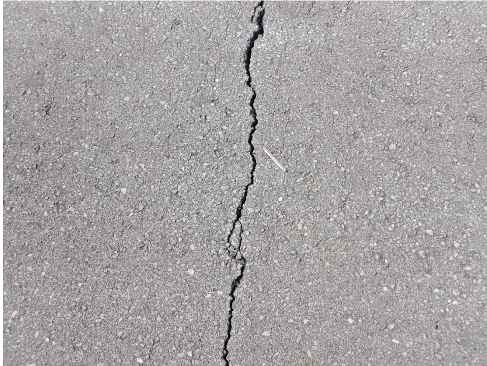
T13AM-02. L&T Cracking (Sample Unit No. 02) (2).
