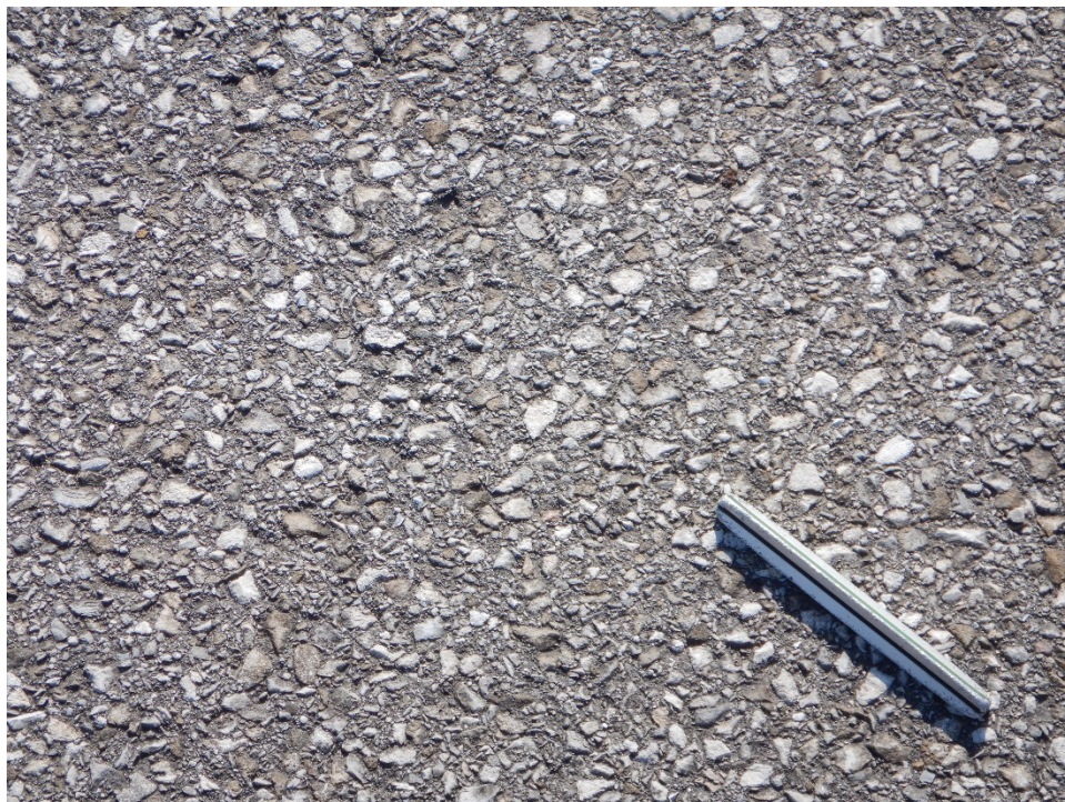
TAAM-03. Weathering (Sample Unit No. 01).
