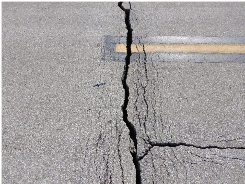
R13AM-02. L&T Cracking (Sample Unit No. 02).
