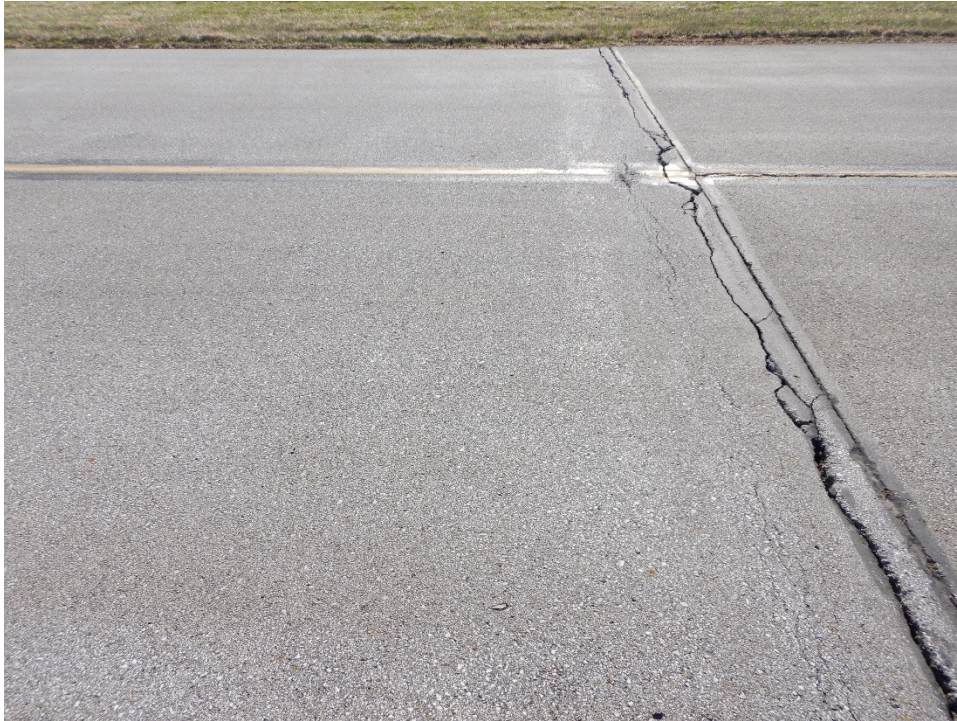
TAAM-02. Patching (Additional Sample Unit No. 17).
