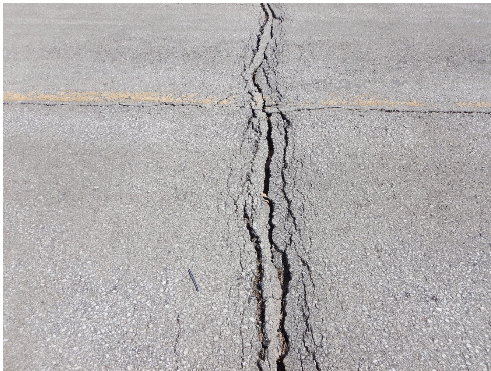
T13AM-02. L&T Cracking (Sample Unit No. 02) (1).
