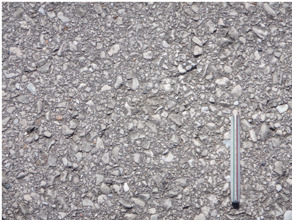
T13AM-02. Weathering (Sample Unit No. 02).
