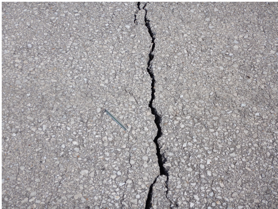
TBAM-04. L&T Cracking (Sample Unit No. 02).
