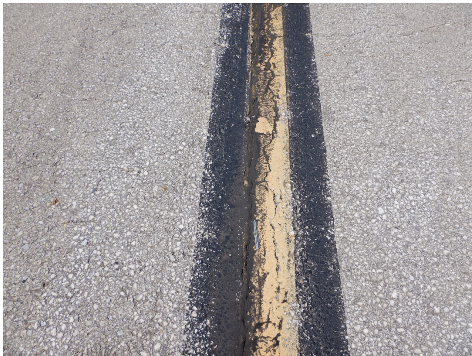
TBAM-01. L&T Cracking (Sample Unit No. 09) (2).
