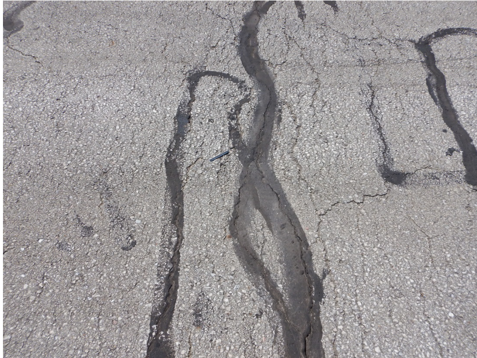
TBAM-01. L&T Cracking (Sample Unit No. 09) (1).
