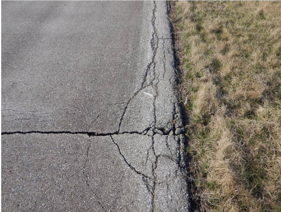
TAAM-02. Alligator Cracking (Sample Unit No. 13).
