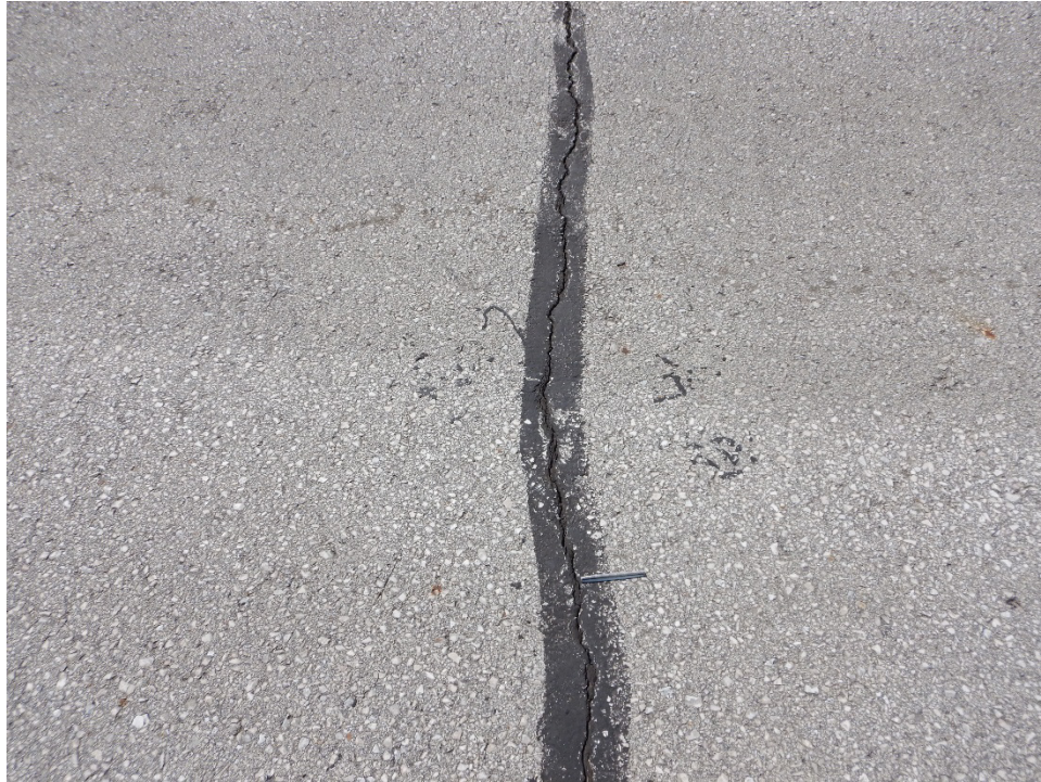
TBAM-01. L&T Cracking (Sample Unit No. 07) (1).
