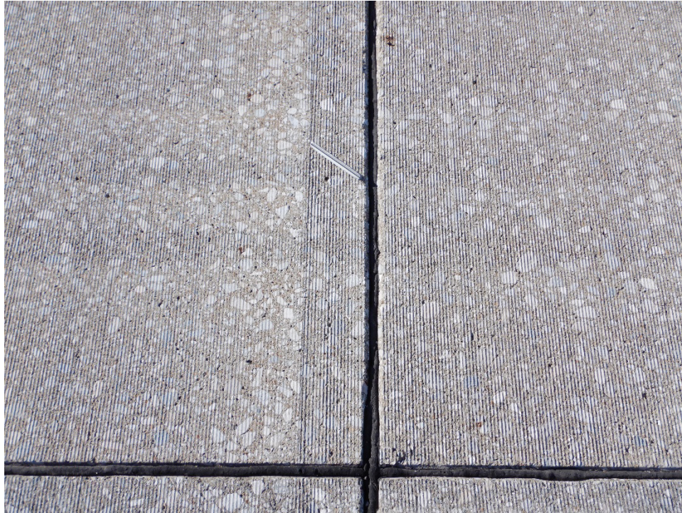
R13AM-04. Joint Seal Damage (Sample Unit No. 03).
