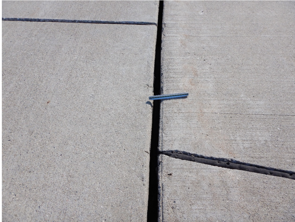
TA1AM-01. Faulting (Sample Unit No. 09).
