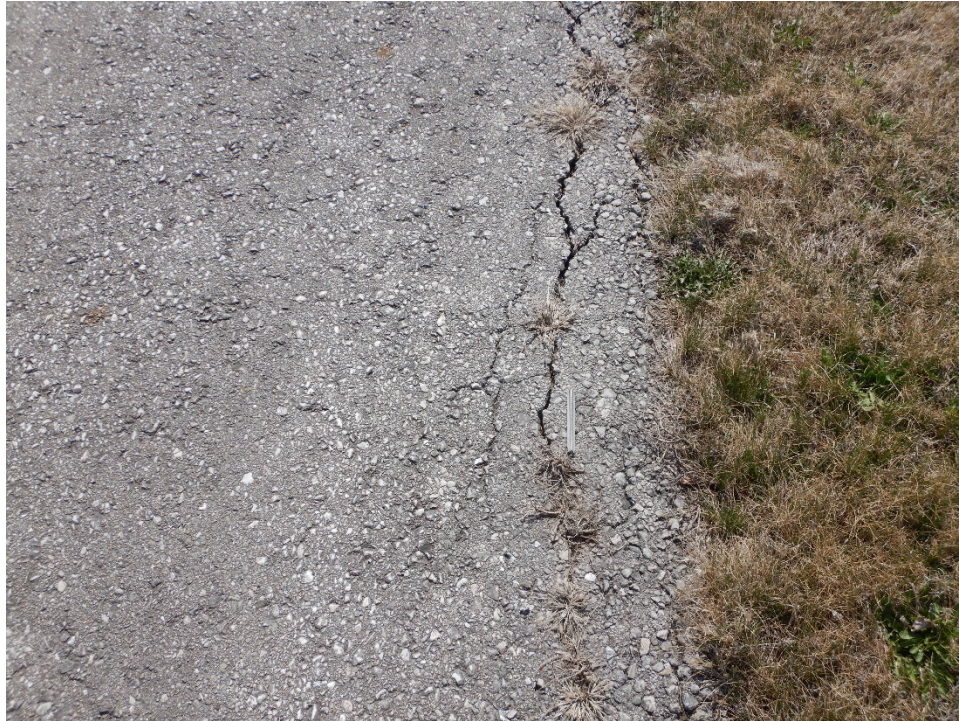
T13AM-02. Alligator Cracking (Sample Unit No. 02).
