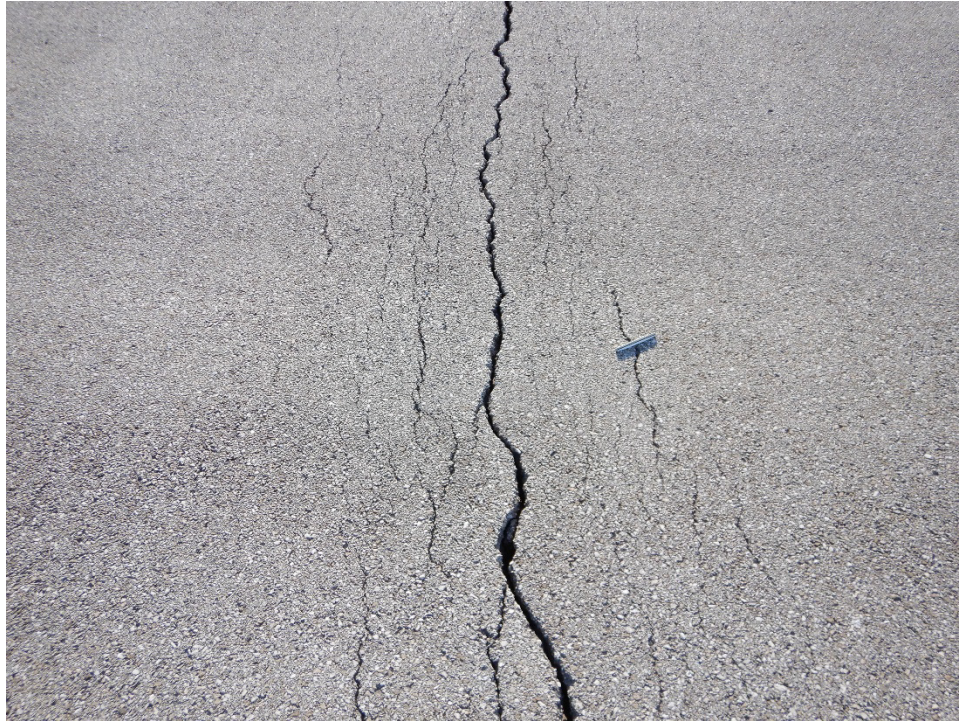
TAAM-02. L&T Cracking (Sample Unit No. 04) (2).
