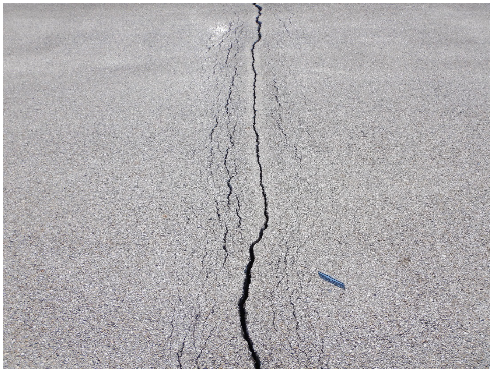
TAAM-02. L&T Cracking (Sample Unit No. 10).
