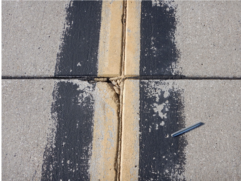
TAAM-05. Corner Spalling (Sample Unit No. 04).
