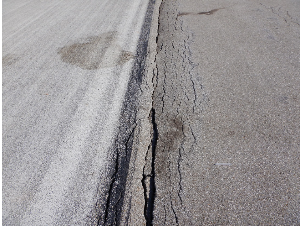
R13AM-02. L&T Cracking (Sample Unit No. 01).
