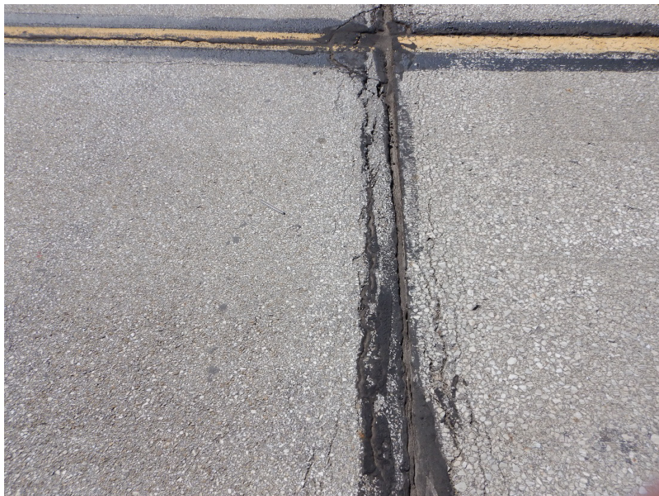
TBAM-02. L&T Cracking (Sample Unit No. 01) (2).
