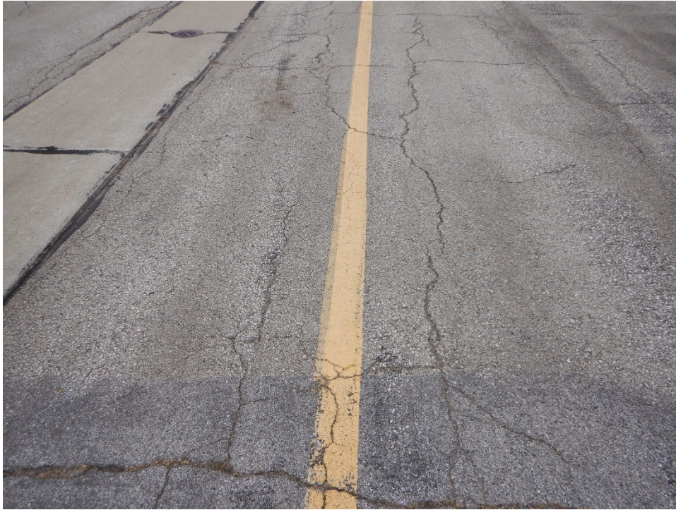
TH01AM-01. Block Cracking (Sample Unit No. 12).
