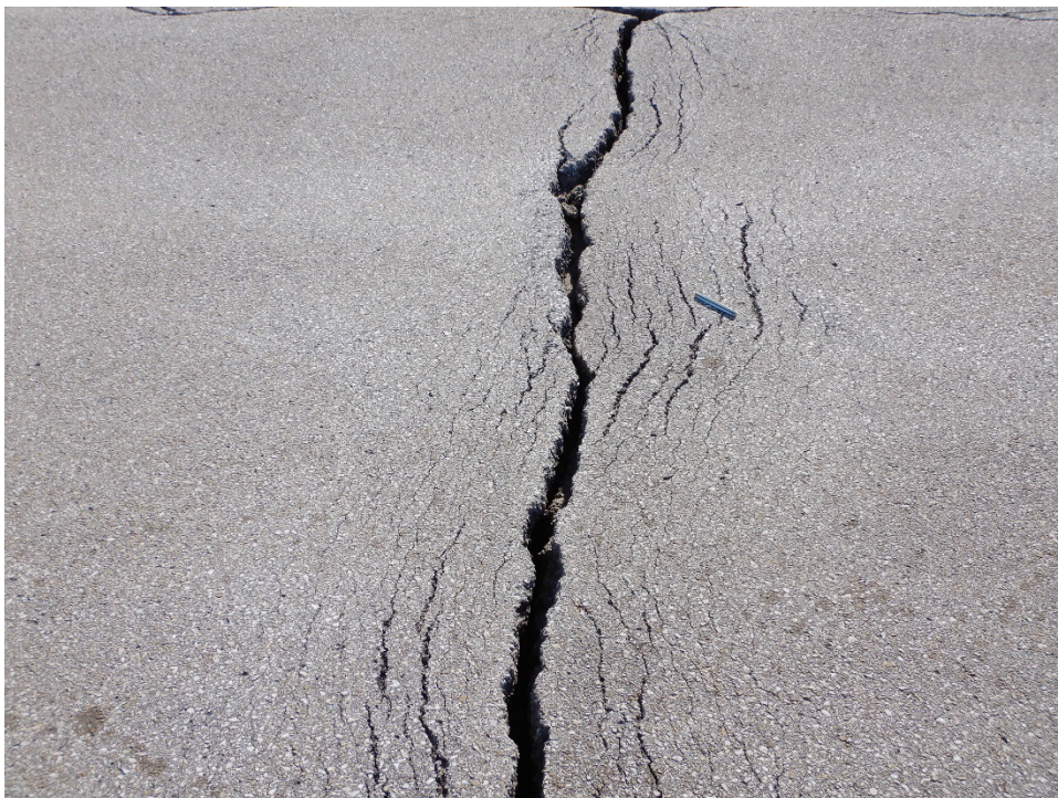
R13AM-03. L&T Cracking (Sample Unit No. 01) (1).
