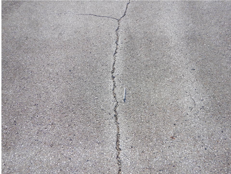
TA3AM-02. L&T Cracking (Sample Unit No. 01) (1).
