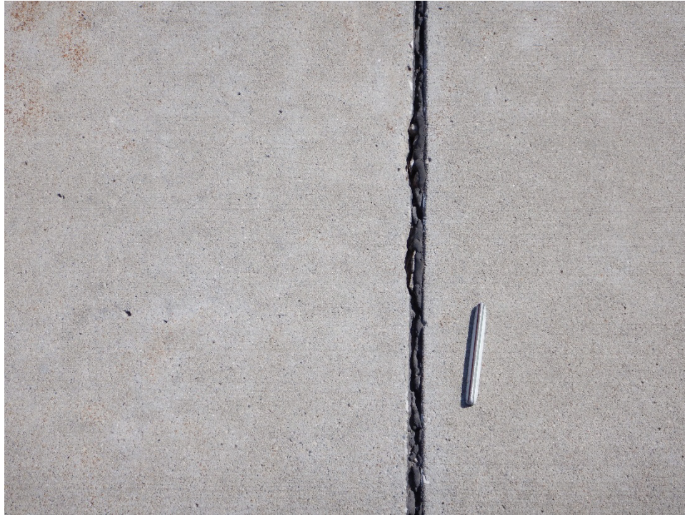
TB1AM-04. Joint Seal Damage (Sample Unit No. 02).
