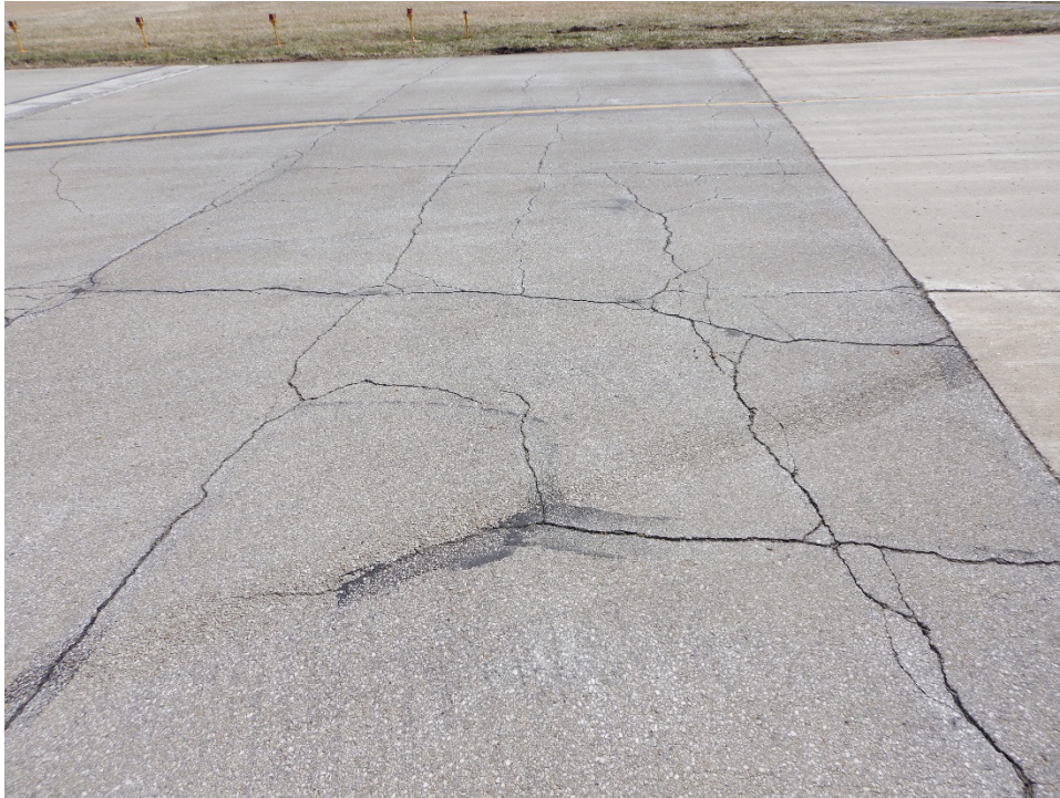
TA4AM-02. Block Cracking (Sample Unit No. 01).
