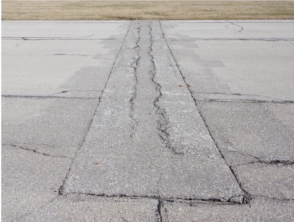
R01AM-01. Patching (Sample Unit No. 76).
