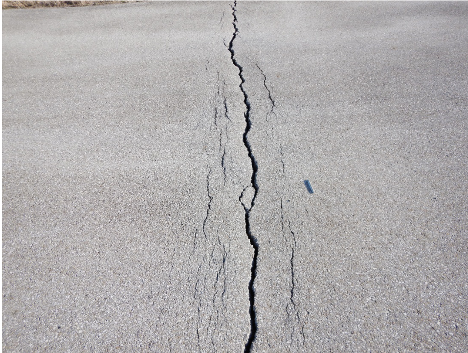
TA2AM-02. L&T Cracking (Sample Unit No. 01).
