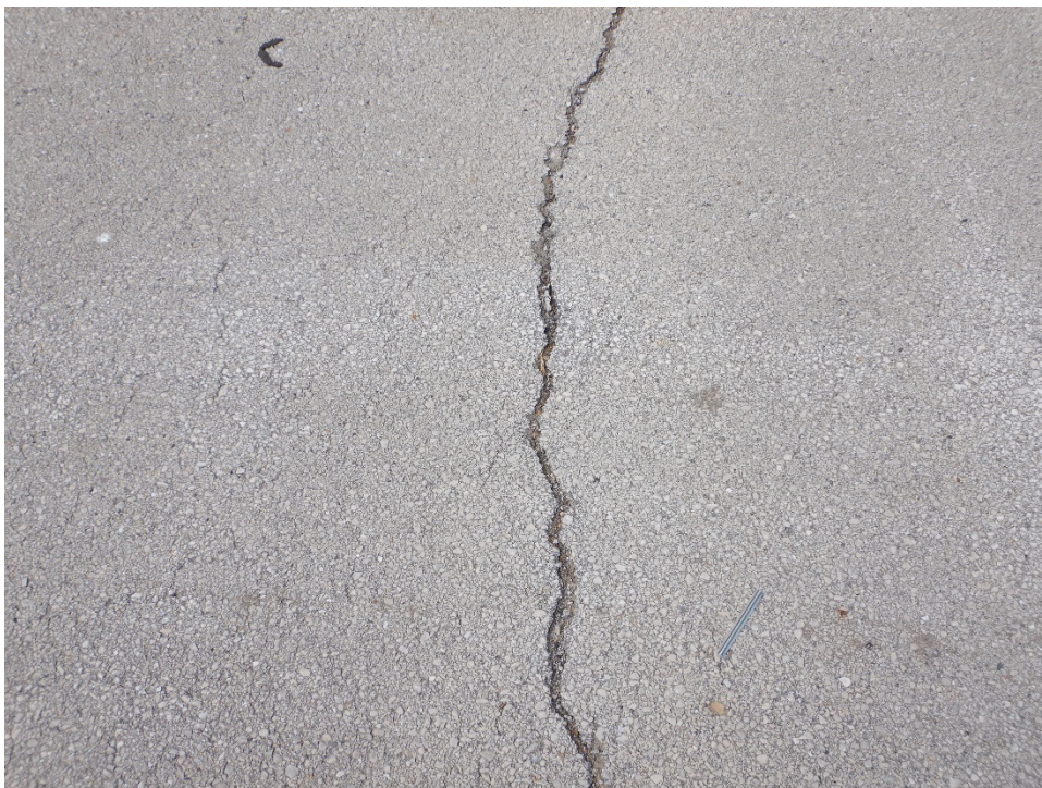
TH01AM-01. L&T Cracking (Sample Unit No. 02).
