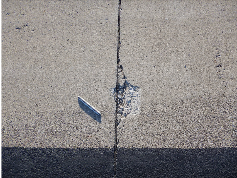
TAAM-08. Joint Spalling (Sample Unit No. 04).
