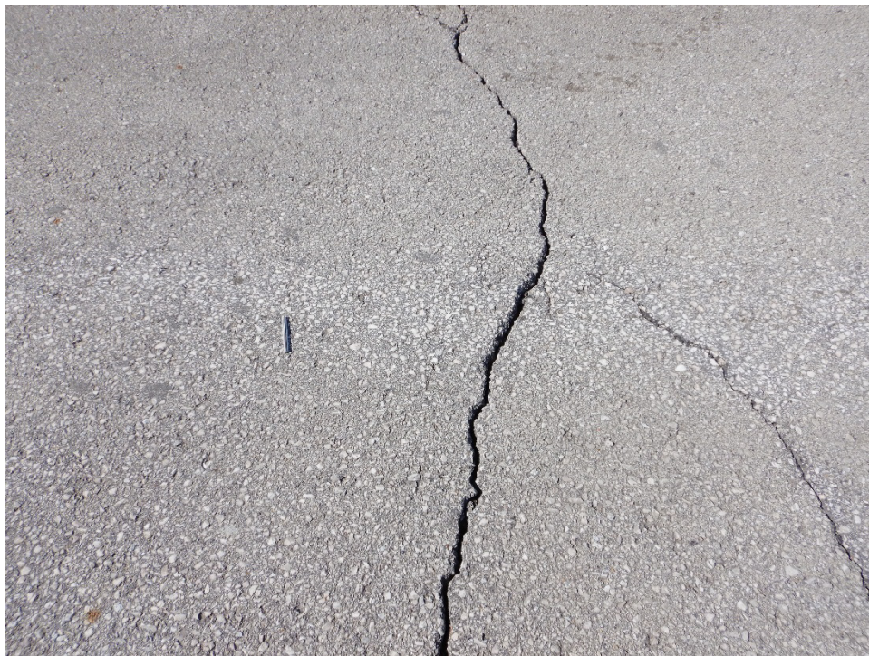
TA1AM-02. L&T Cracking (Sample Unit No. 03).
