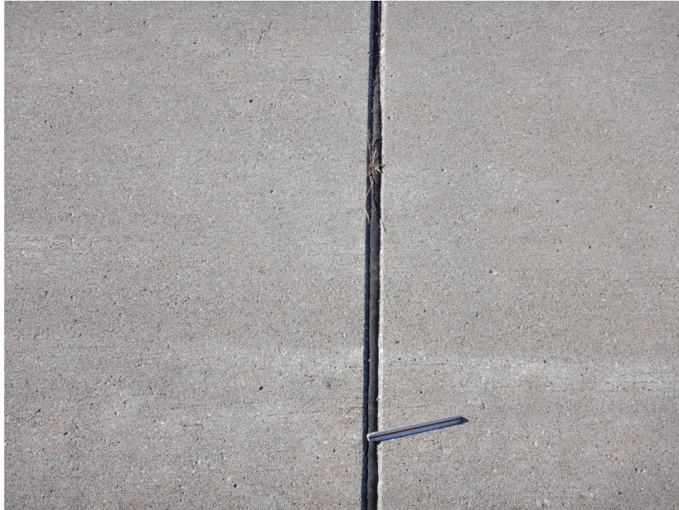
TB1AM-02. Joint Seal Damage (Sample Unit No. 03).
