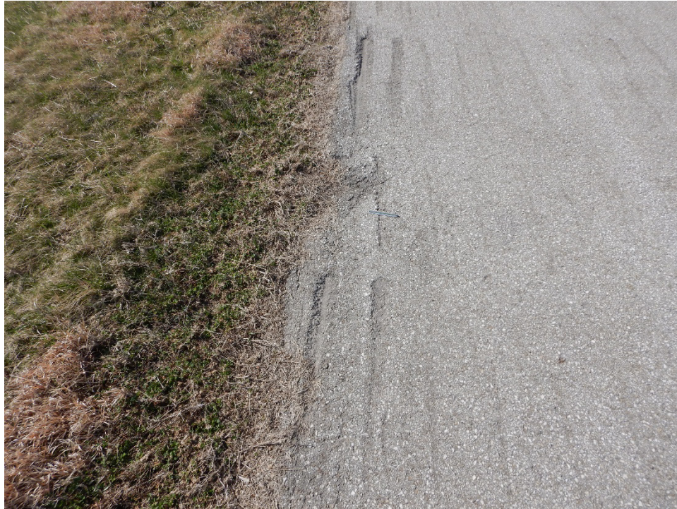
TAAM-04. Raveling (Sample Unit No. 05).
