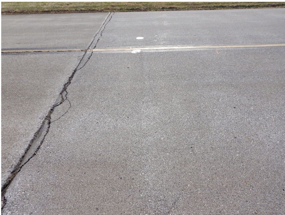
TAAM-02. Patching (Additional Sample Unit No. 18).
