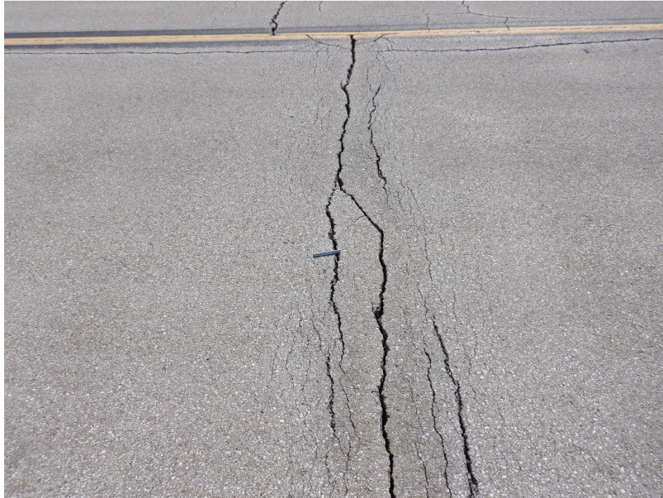
TAAM-04. L&T Cracking (Sample Unit No. 04).
