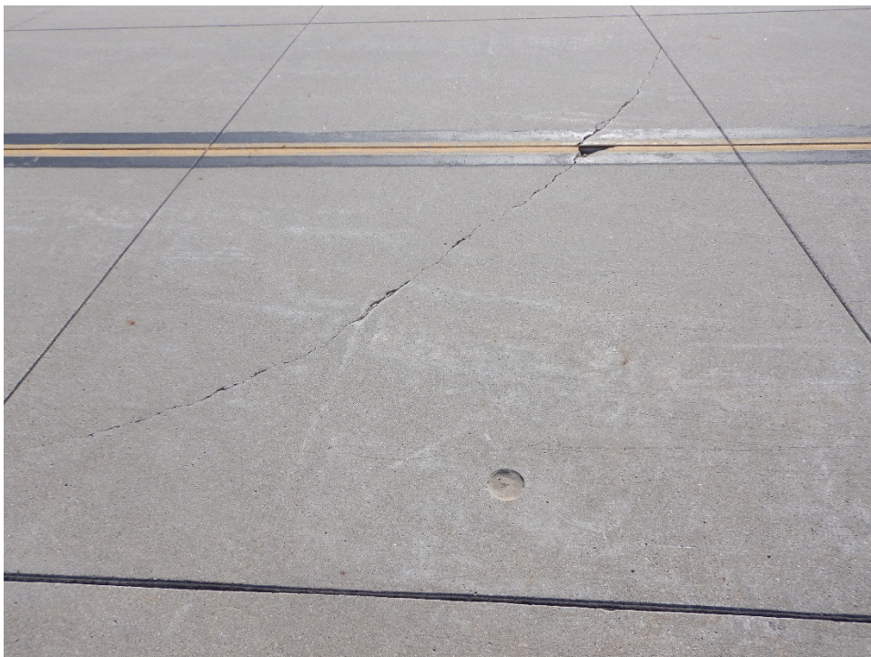
TAAM-06. LTD Cracking (Sample Unit No. 05).
