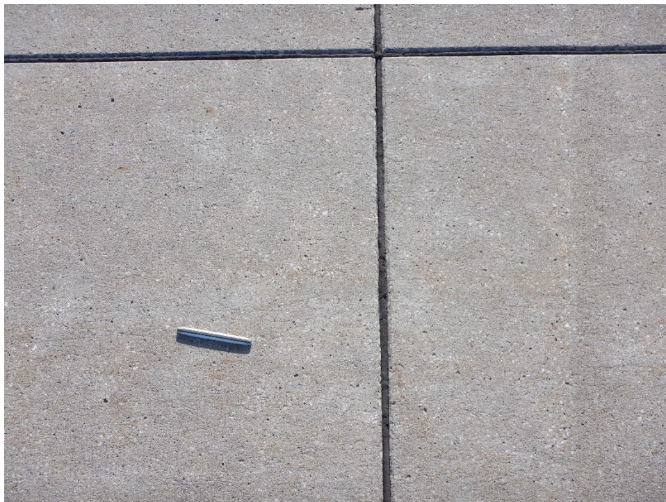
TAAM-05. Joint Seal Damage (Sample Unit No. 04).
