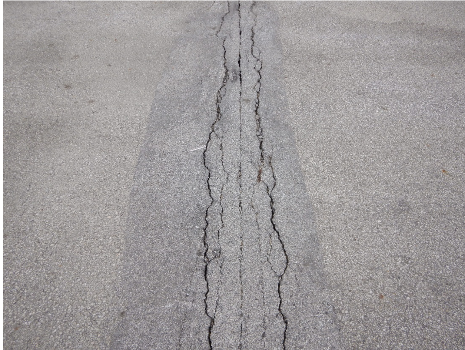
TH01AM-01. L&T Cracking (Sample Unit No. 18).
