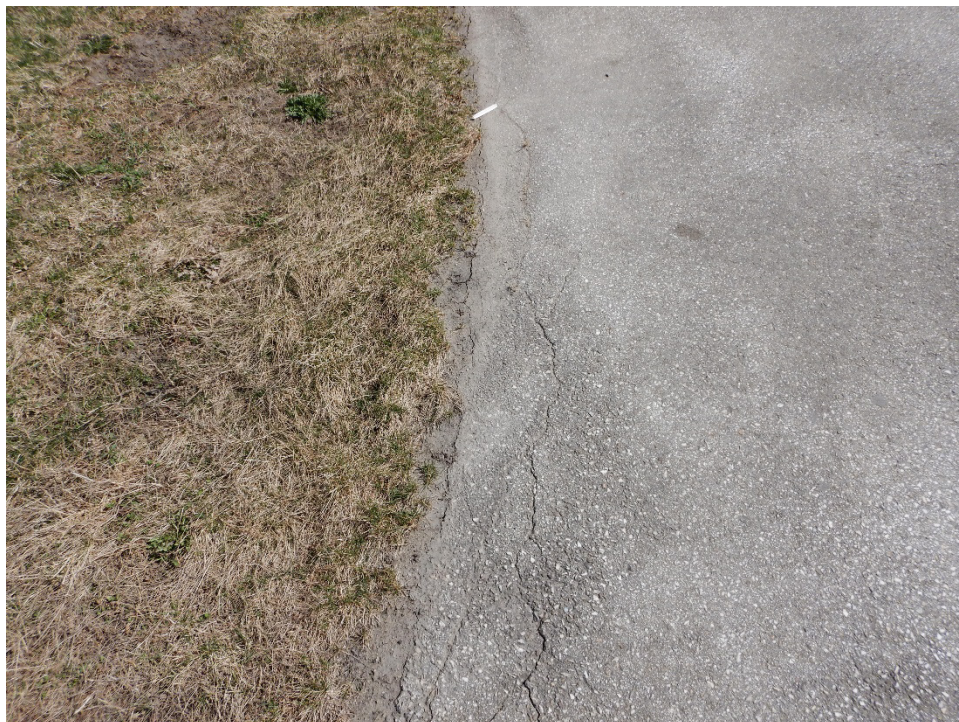
TBAM-02. Alligator Cracking (Sample Unit No. 01).
