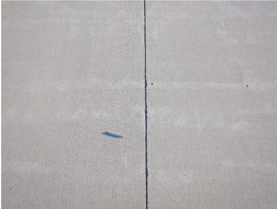
TA3AM-01. Joint Seal Damage (Sample Unit No. 06).
