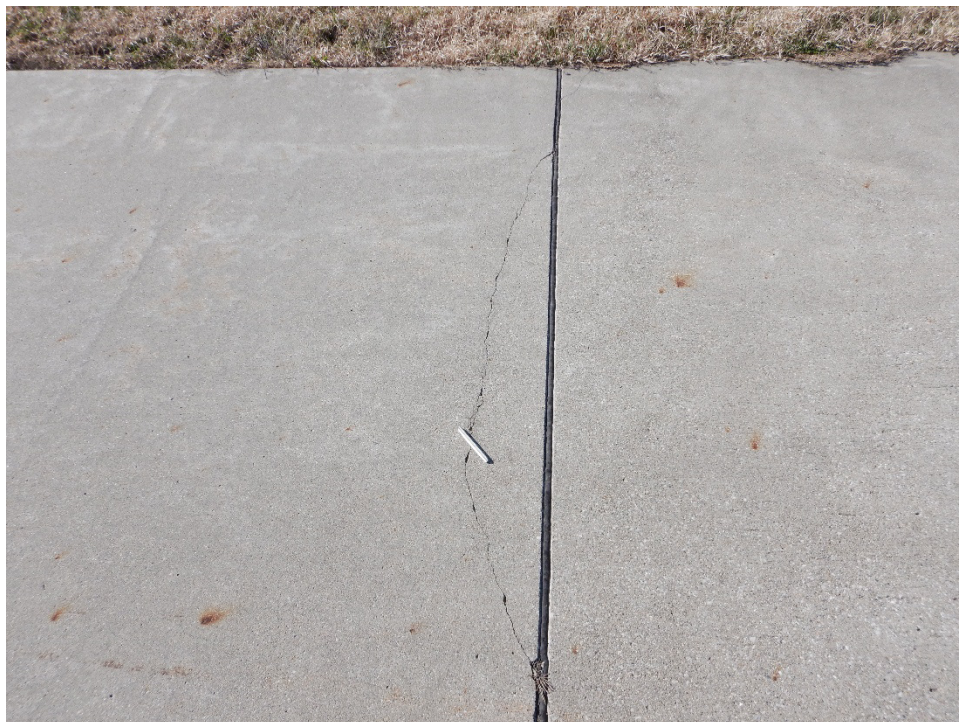
TB1AM-02. Joint Spalling (Sample Unit No. 04).
