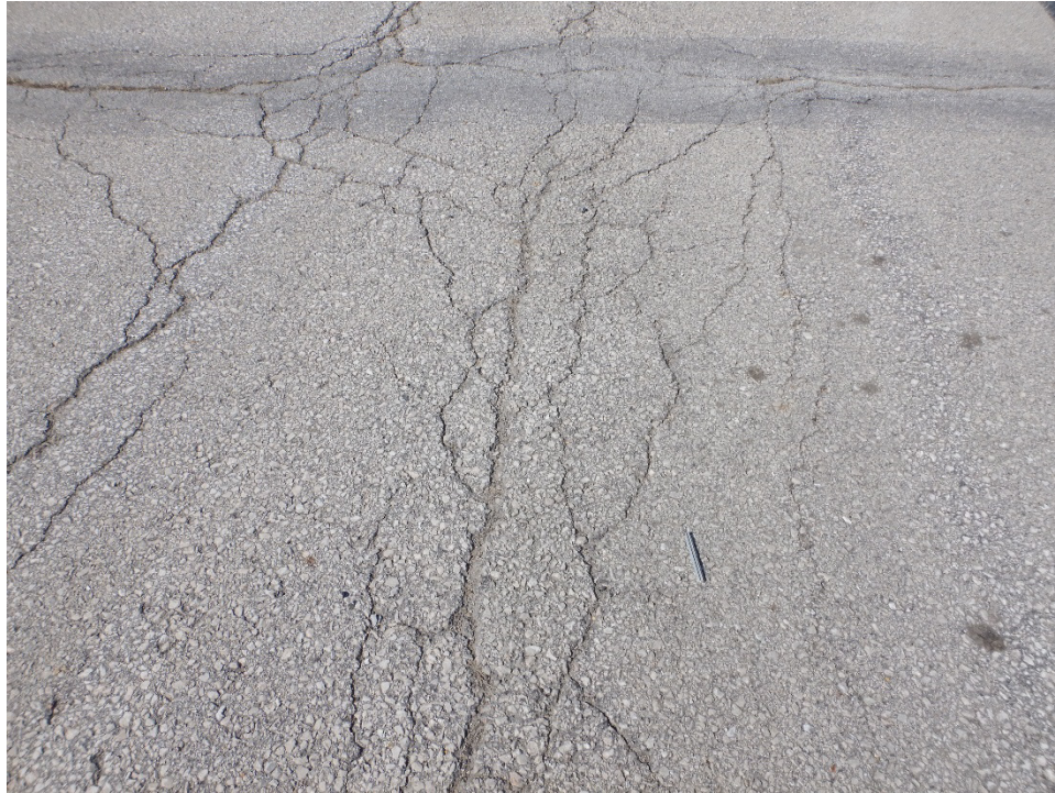
TA1AM-02. Alligator Cracking (Sample Unit No. 01).
