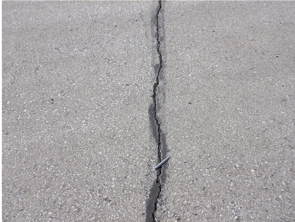
TB1AM-01. L&T Cracking (Sample Unit No. 02).
