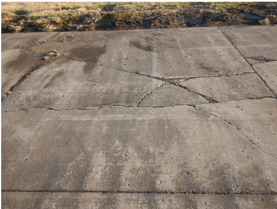
TAAM-10. Shattered Slab (Additional Sample Unit No. 07) (1).
