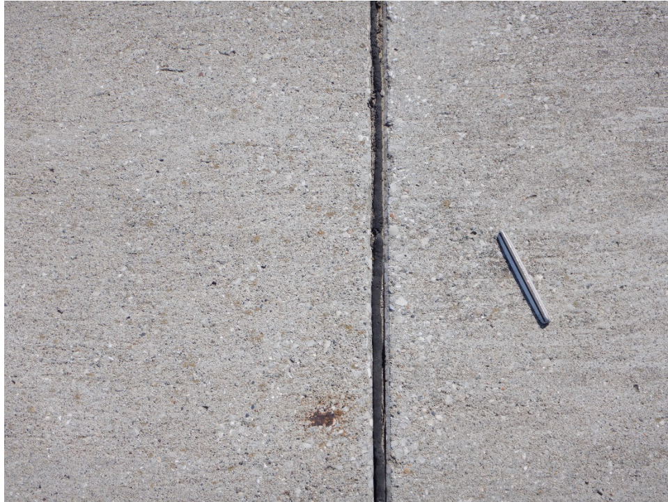
TB2AM-02. Joint Seal Damage (Sample Unit No. 02).
