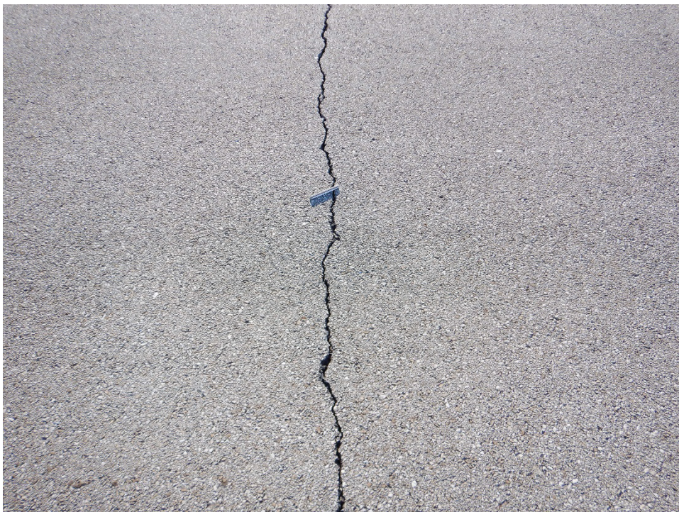
TAAM-02. L&T Cracking (Sample Unit No. 04) (1).
