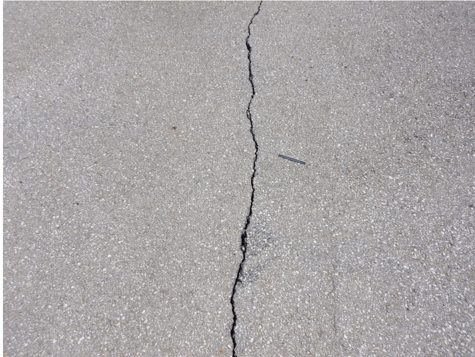
TBAM-02. L&T Cracking (Sample Unit No. 01) (1).
