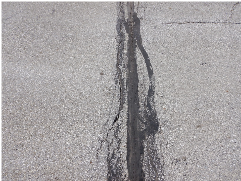
TBAM-01. L&T Cracking (Sample Unit No. 07) (2).
