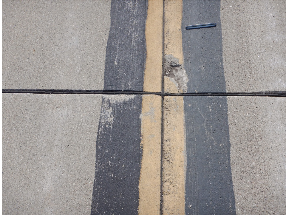
T13AM-01. Corner Spalling (Sample Unit No. 10).
