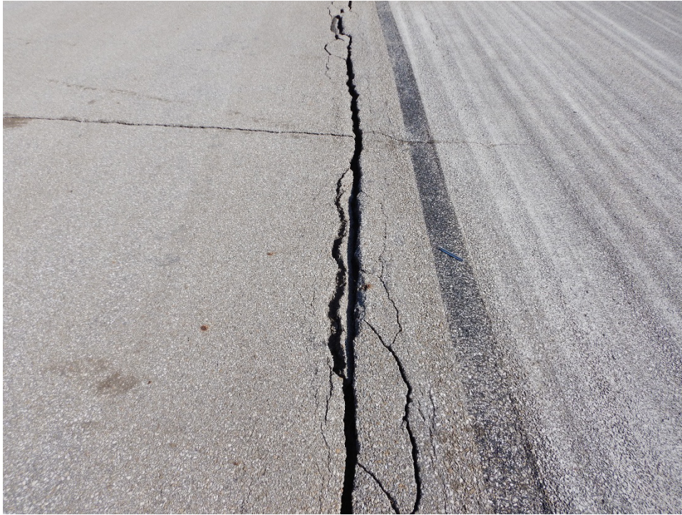
R13AM-02. L&T Cracking (Sample Unit No. 04).
