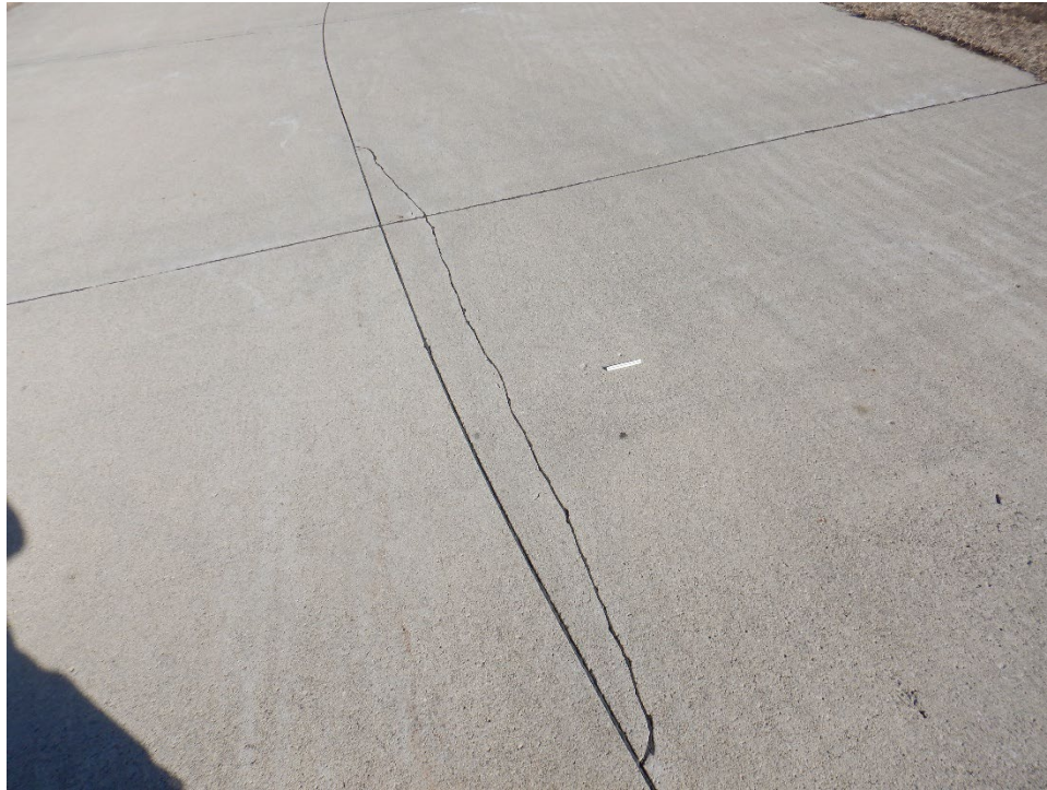
TH01AG-01. LTD Cracking (Sample Unit No. 01).
