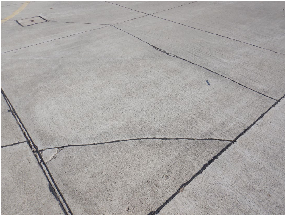
A01AG-02. Shattered Slab (Sample Unit No. 02).
