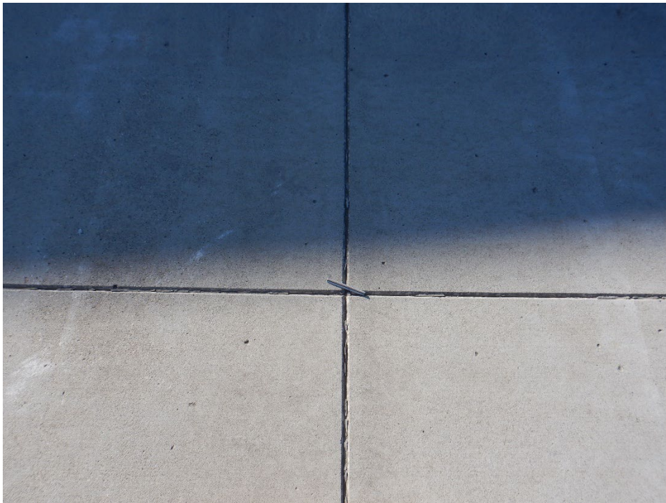
TH01AG-03. Joint Seal Damage (Sample Unit No. 01) (1).
