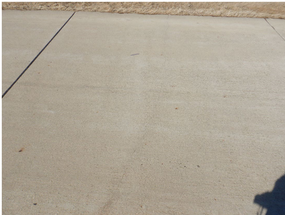
TH01AG-02. LTD Cracking (Sample Unit No. 03).
