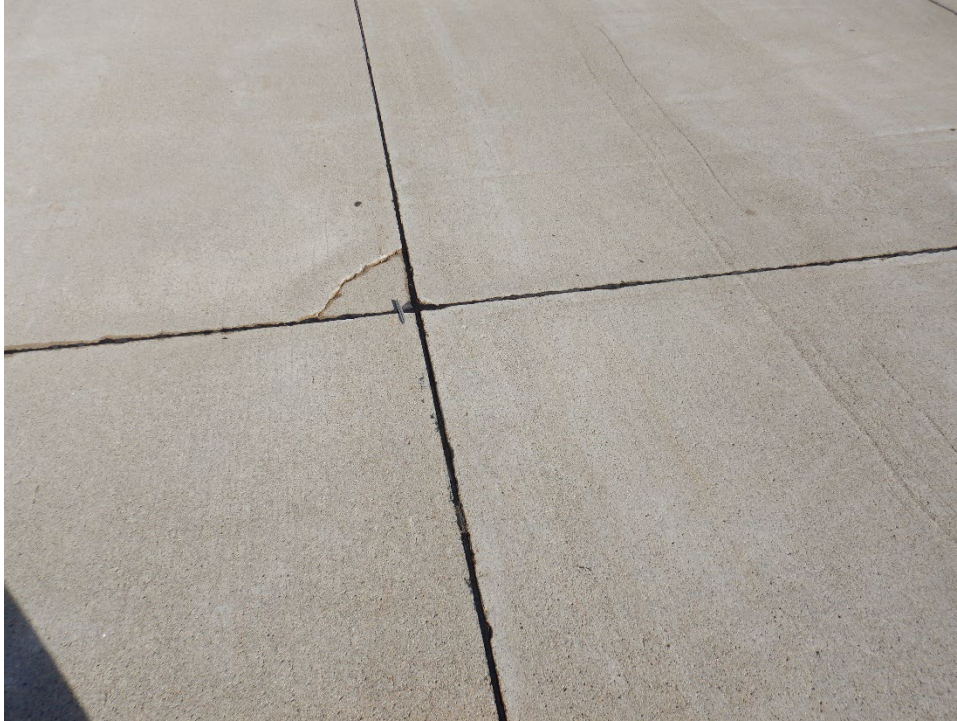
TH01AG-05. Joint Seal Damage (Sample Unit No. 01).
