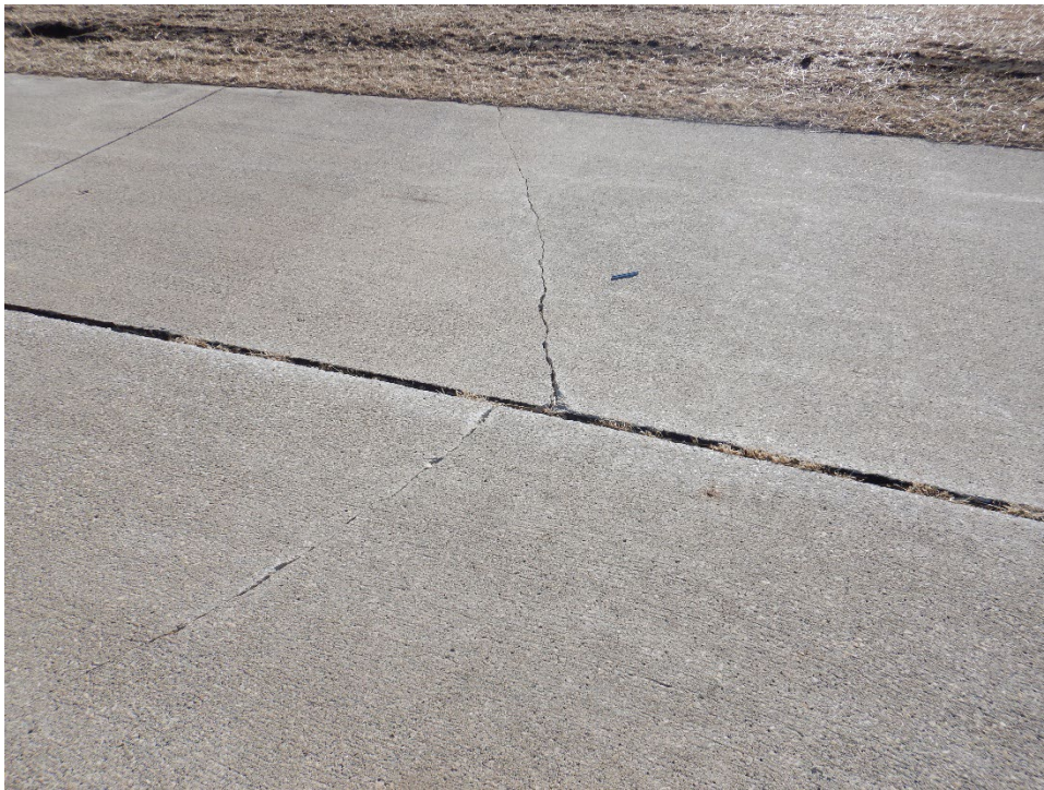
TA2AG-01. LTD Cracking (Sample Unit No. 05).
