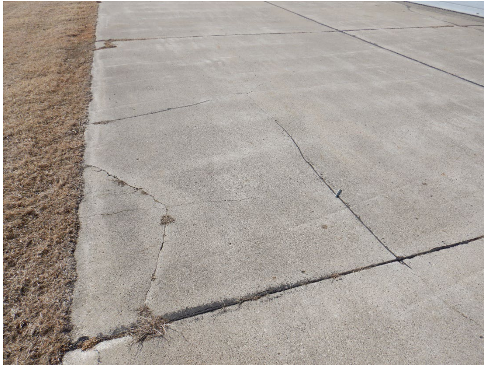
TH01AG-06. Shattered Slab (Sample Unit No. 01).
