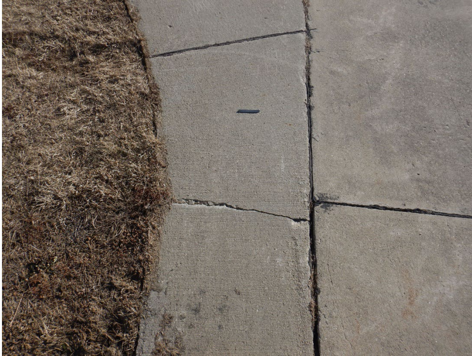
TH01AG-04. LTD Cracking (Sample Unit No. 02).
