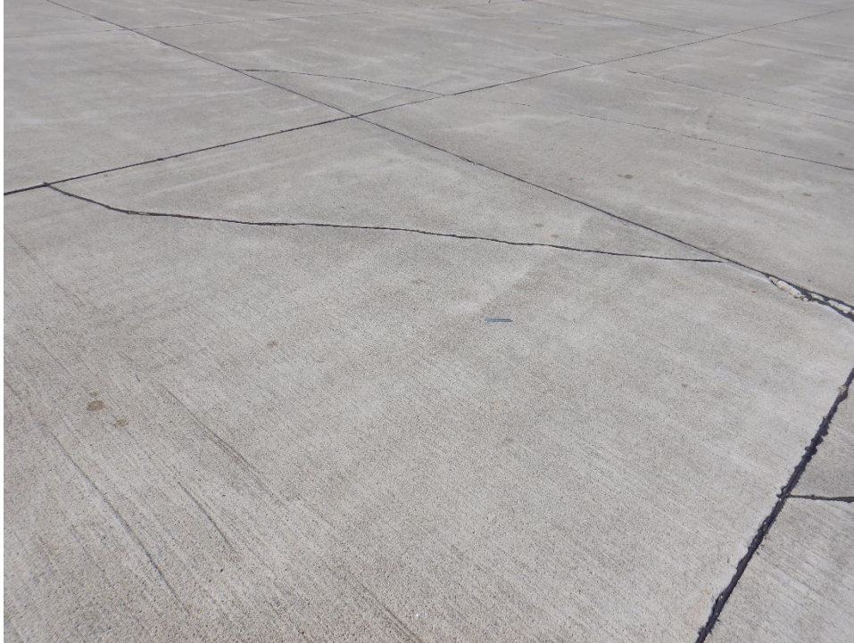
A01AG-02. LTD Cracking (Sample Unit No. 02).
