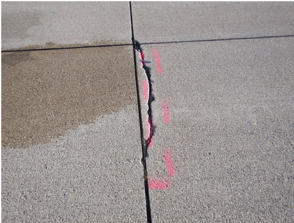
R13AG-01. Joint Spalling (Sample Unit No. 44).
