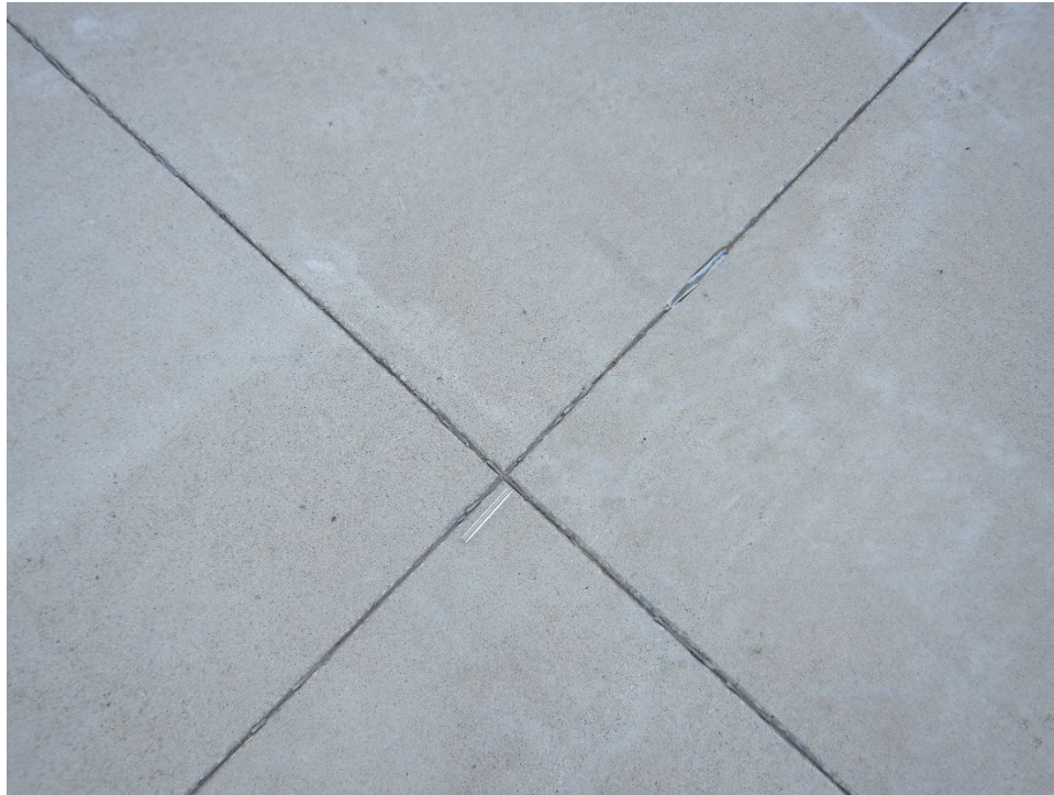
TH01AG-03. Joint Seal Damage (Sample Unit No. 01) (2).
