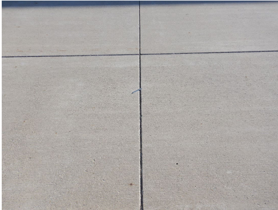
TH01AG-02. Joint Seal Damage (Sample Unit No. 02).
