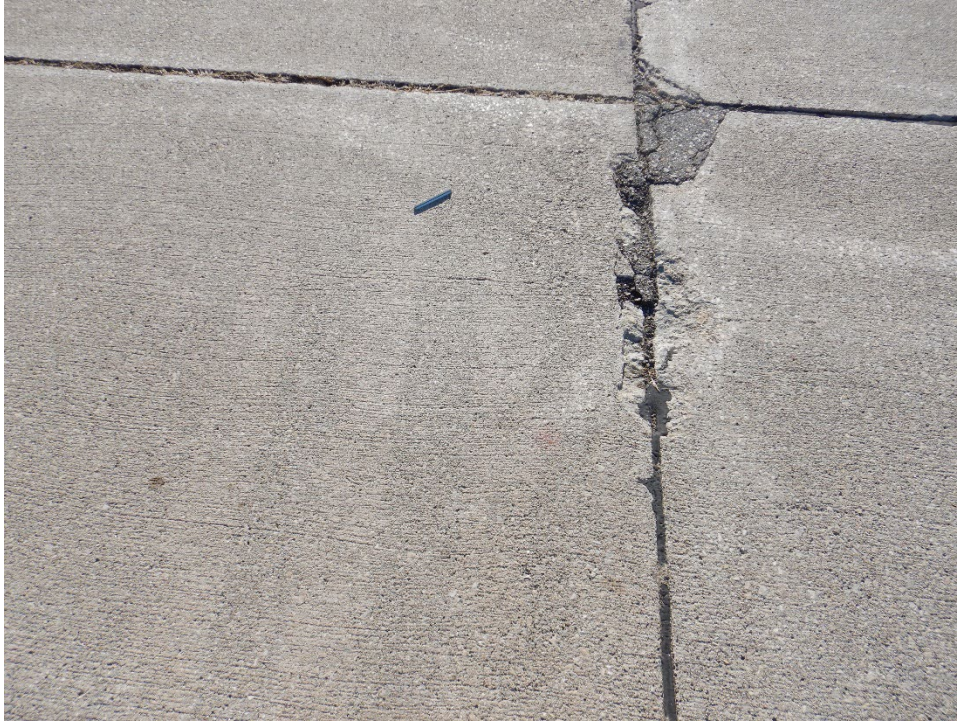
TA2AG-01. Joint Seal Damage (Sample Unit No. 05).
