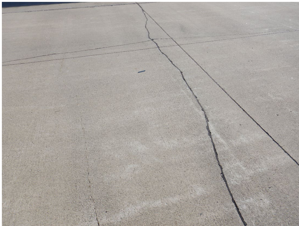
TH01AG-01. LTD Cracking (Sample Unit No. 02).
