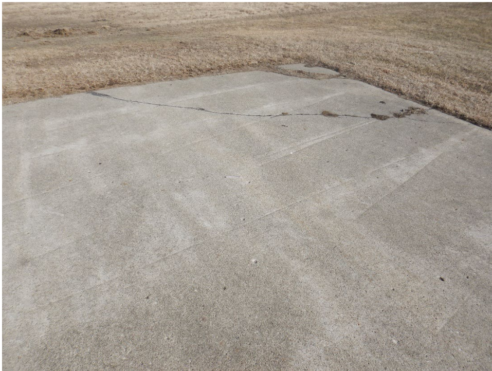
TH01AG-06. LTD Cracking (Sample Unit No. 01).
