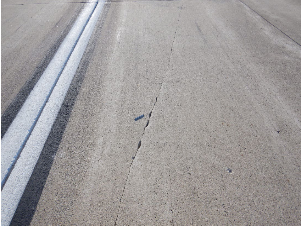
R13AG-01. LTD Cracking (Sample Unit No. 39).
