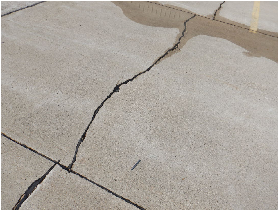
TH01AG-05. LTD Cracking (Sample Unit No. 01).
