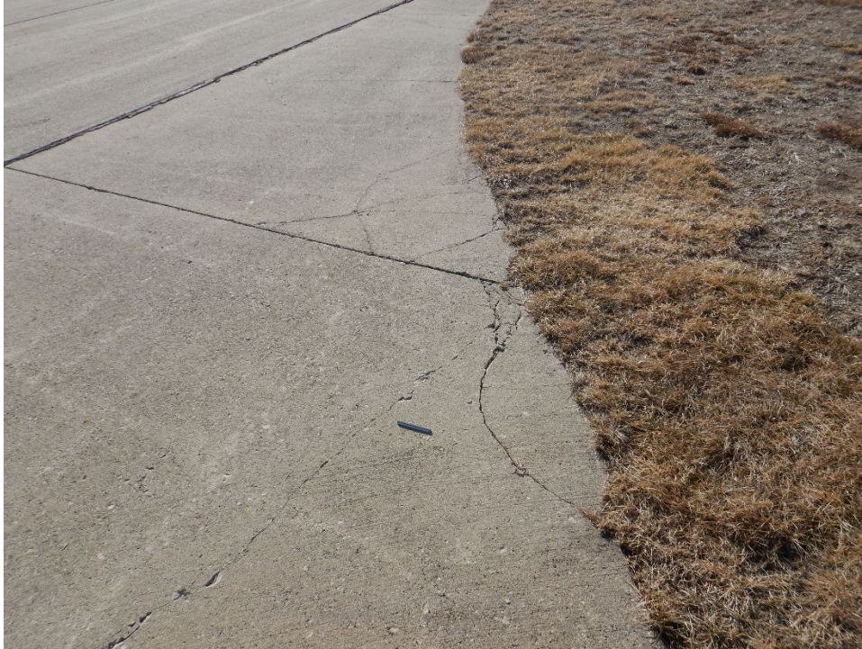
TH01AG-01. Shattered Slab (Sample Unit No. 01).
