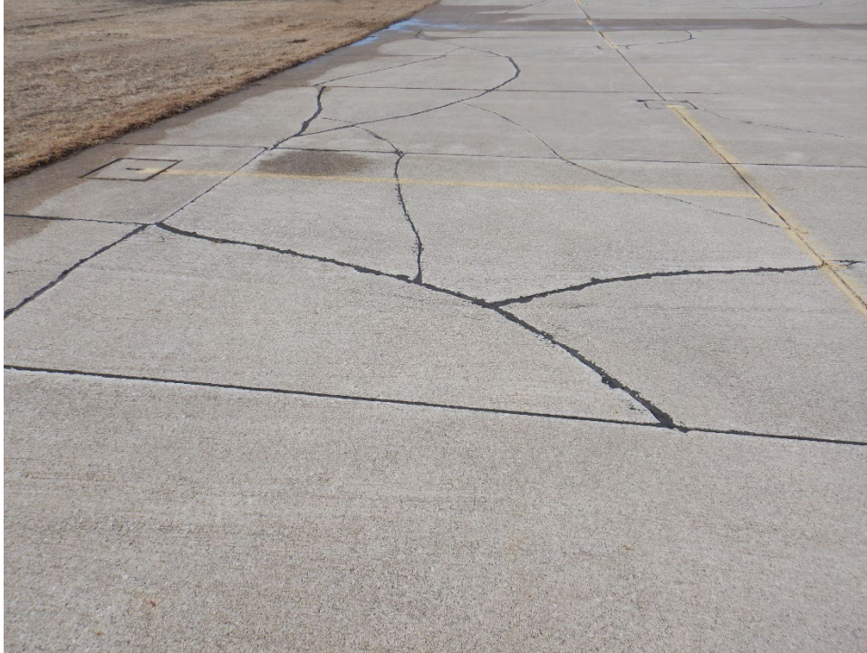
A01AG-01. Shattered Slab (Sample Unit No. 06).
