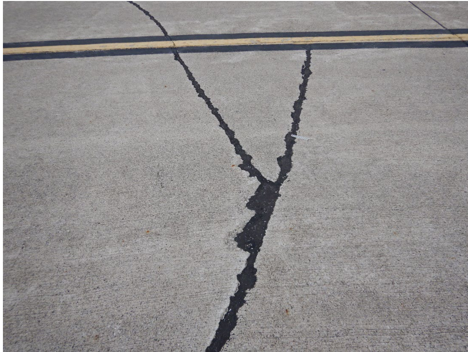
T01AG-01. LTD Cracking (Sample Unit No. 04).
