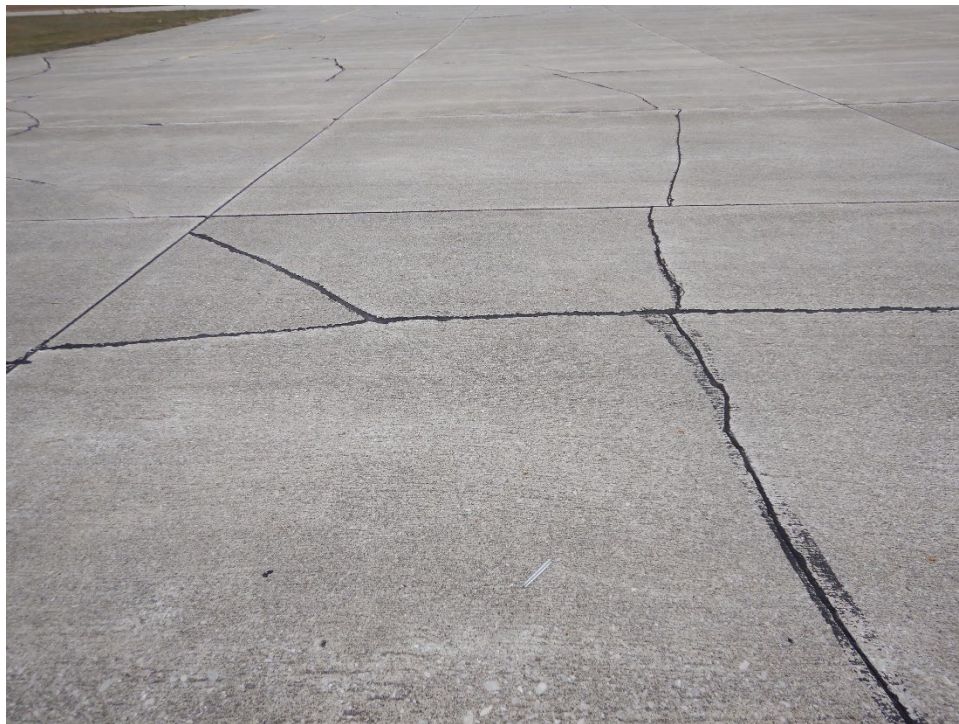
A01AG-01. Shattered Slab (Sample Unit No. 06).
