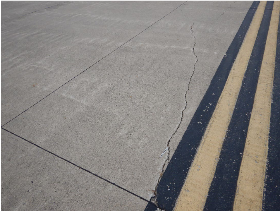
R12AG-02. LTD Cracking (Sample Unit No. 01).
