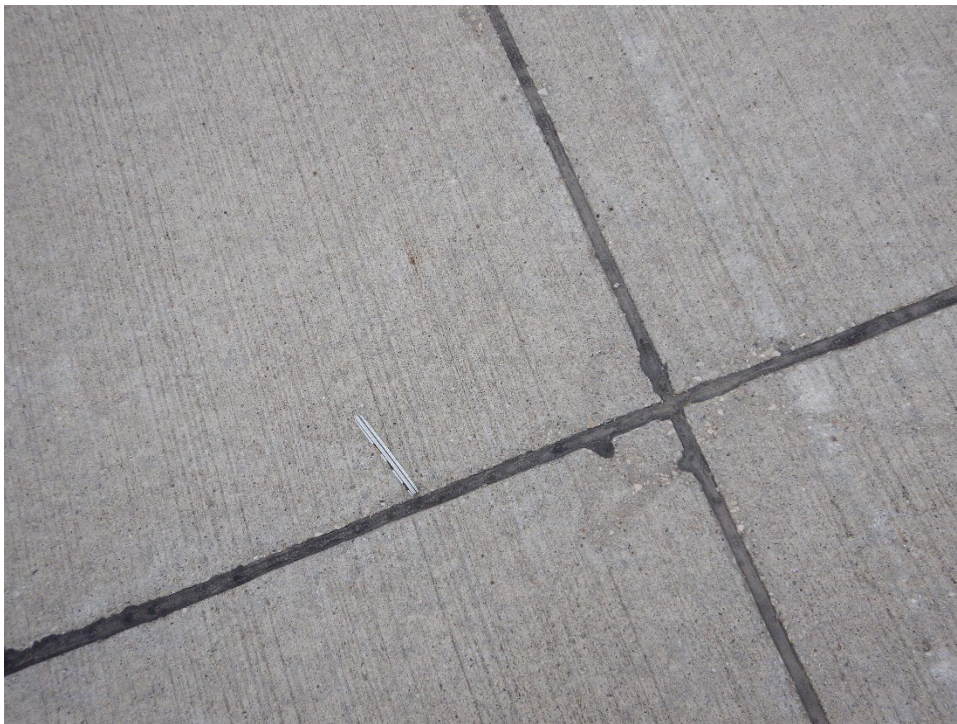
TH01AG-04. Joint Seal Damage (Sample Unit No. 02).
