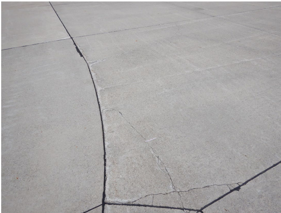
TH01AG-06. Shattered Slab (Sample Unit No. 05).
