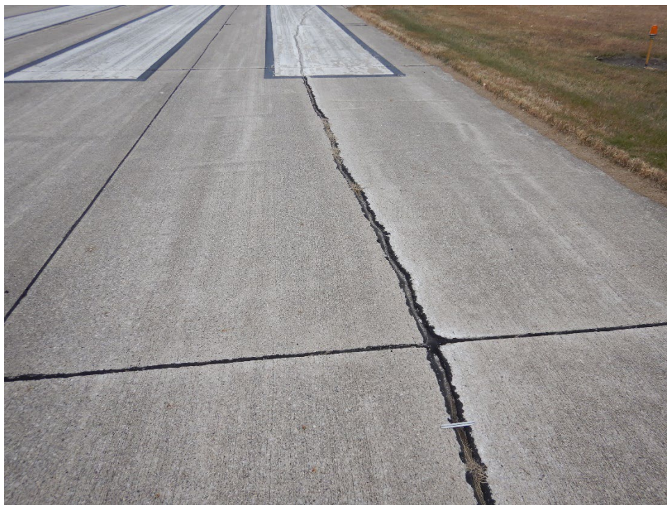
R12AG-01. LTD Cracking (Sample Unit No. 05).
