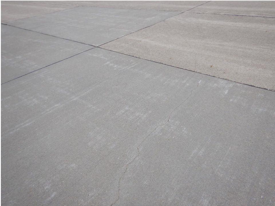
R12AG-01. LTD Cracking (Sample Unit No. 32).
