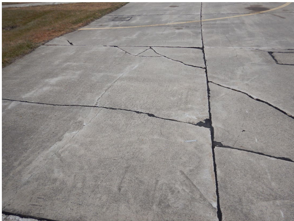
A01AG-02. Shattered Slab (Sample Unit No. 01).
