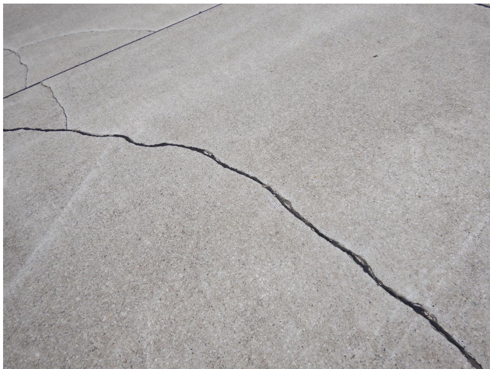
TH01AG-05. LTD Cracking (Sample Unit No. 01).
