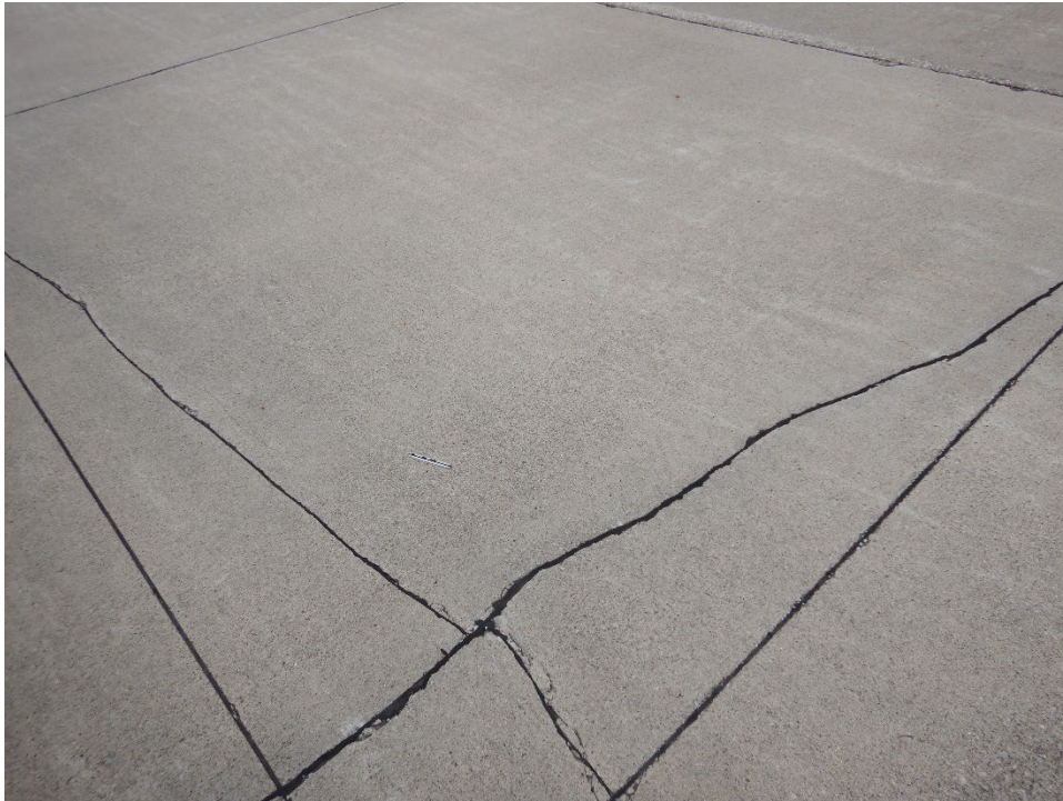
TH01AG-01. Shattered Slab (Sample Unit No. 03).
