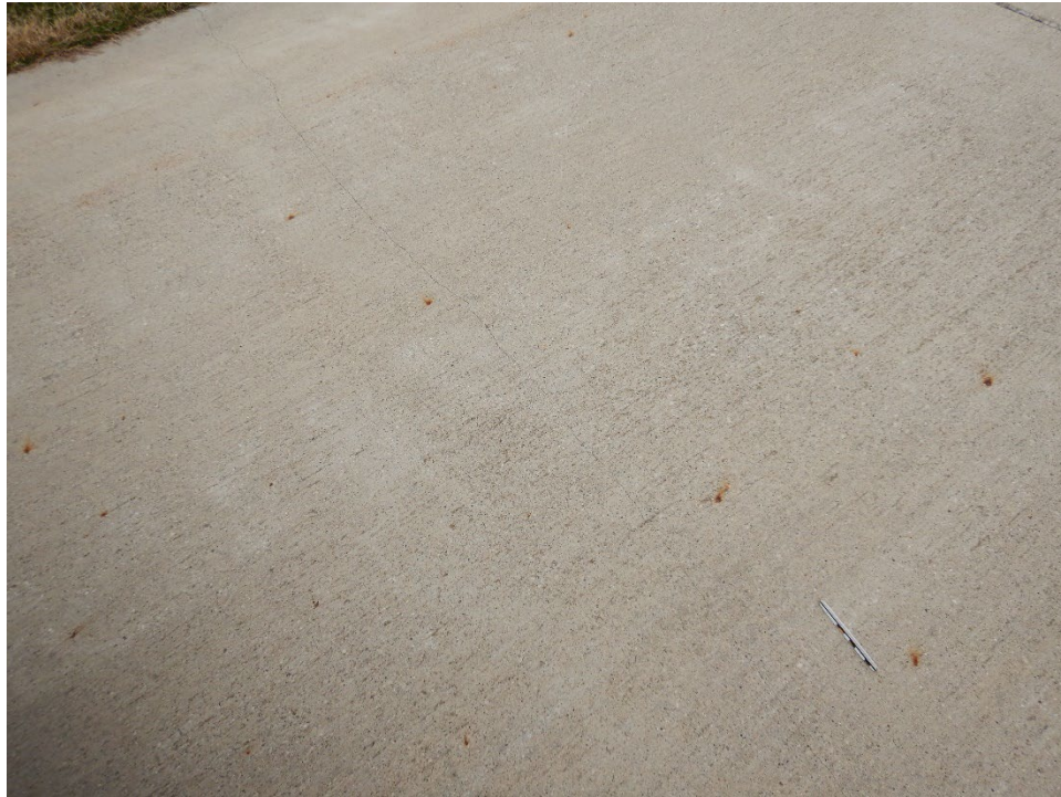
TH01AG-02. LTD Cracking (Sample Unit No. 03).
