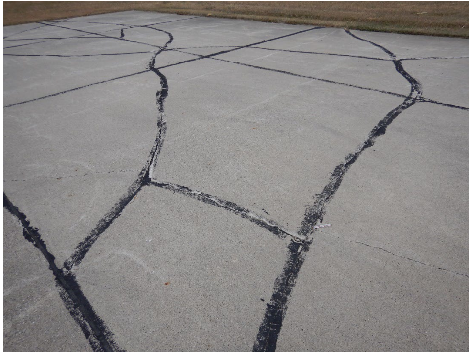
R12AG-03. Shattered Slab (Sample Unit No. 01).
