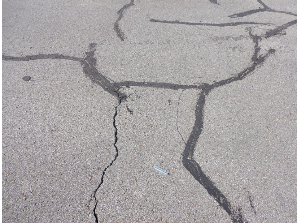
R13AL-02. L&T Cracking (Sample Unit No. 01).
