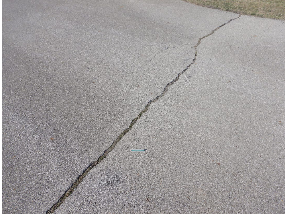
TH01AL-02. L&T Cracking (Sample Unit No. 01).
