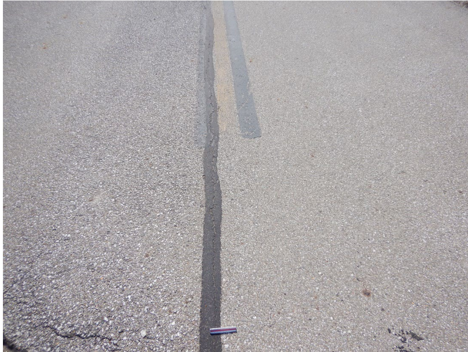
T02AL-01. L&T Cracking (Sample Unit No. 01) (2).
