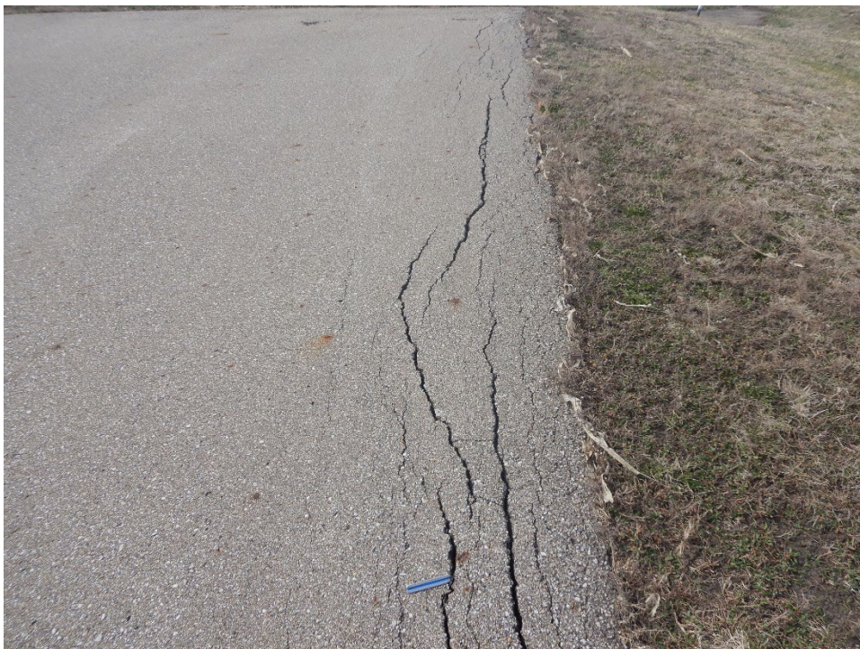
T03AL-01. Alligator Cracking (Sample Unit No. 01).
