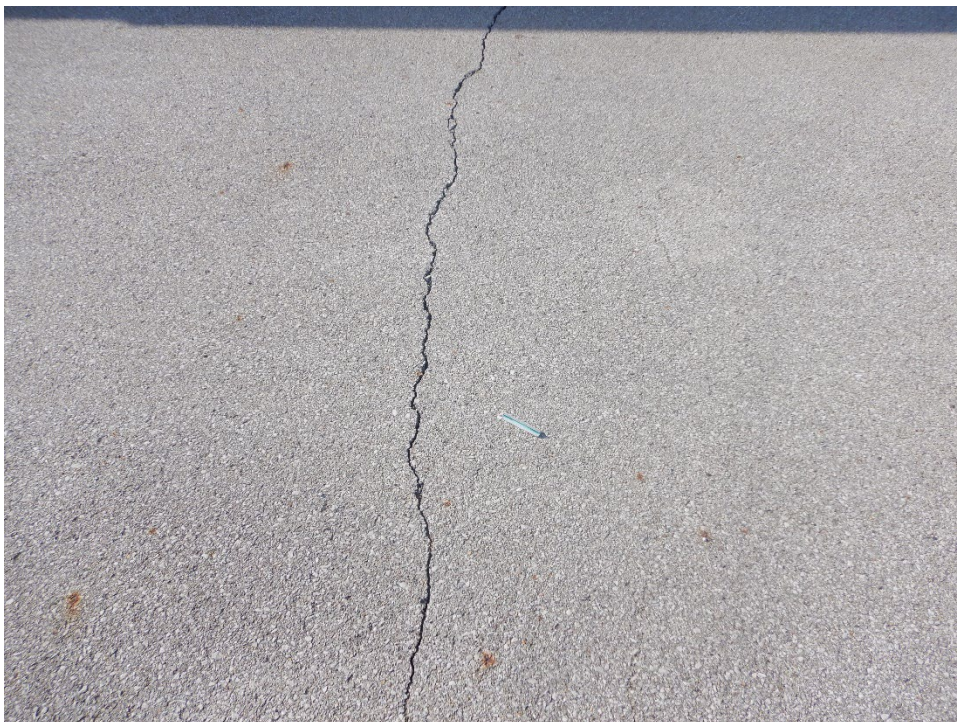
A01AL-03. L&T Cracking (Sample Unit No. 01).
