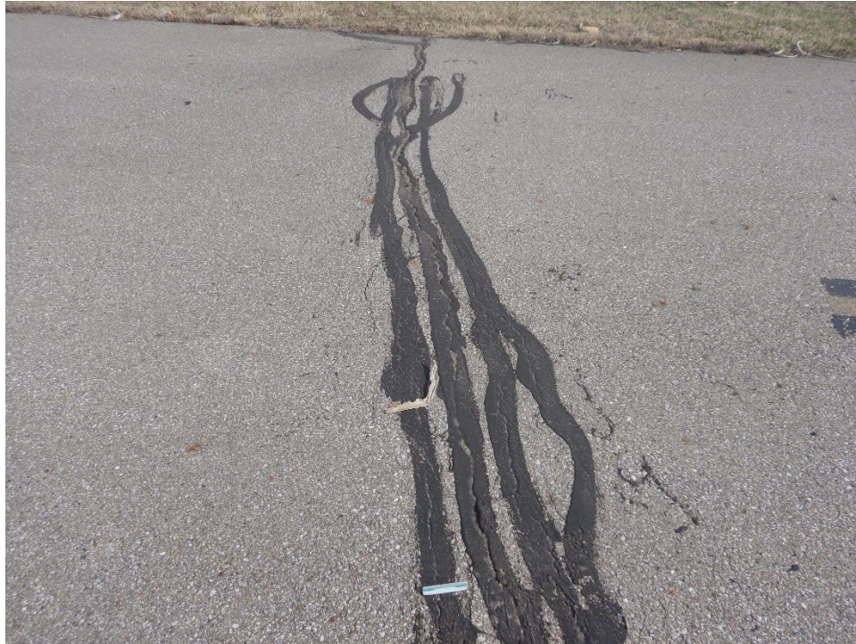
T03AL-01. L&T Cracking (Sample Unit No. 01).
