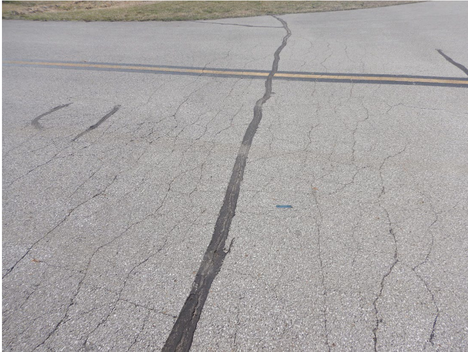
T01AL-01. Alligator Cracking (Sample Unit No. 01).
