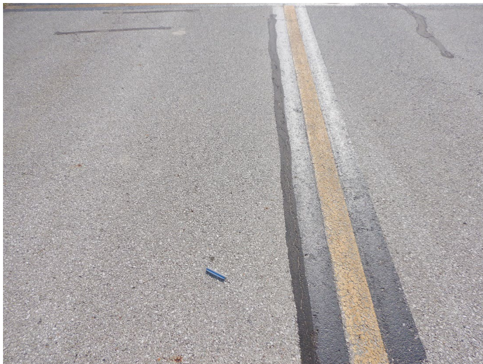
T01AL-01. L&T Cracking (Sample Unit No. 01) (2).
