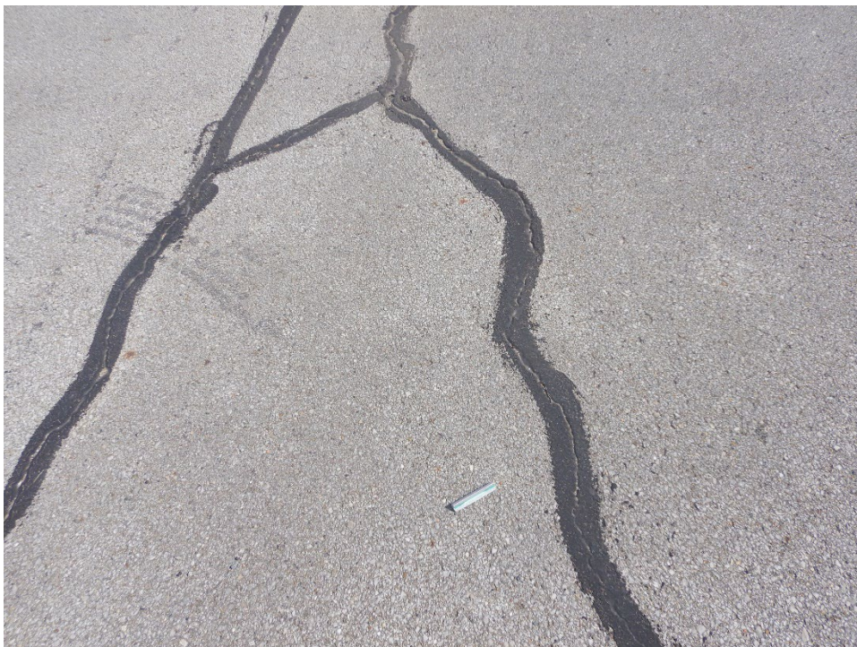
R13AL-05 L&T. Cracking (Sample Unit No. 01).
