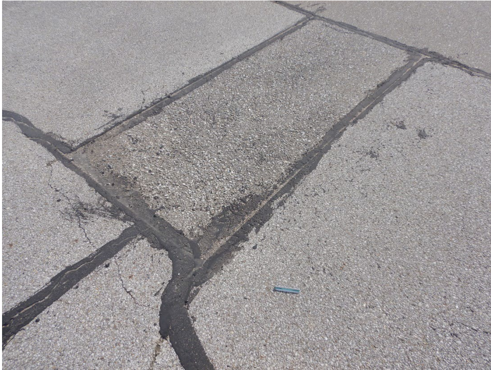
R13AL-05. Patching (Sample Unit No. 01).
