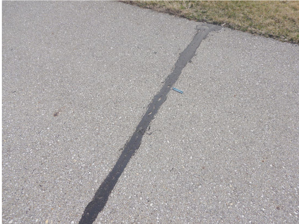
R13AL-04. L&T Cracking (Sample Unit No. 04).
