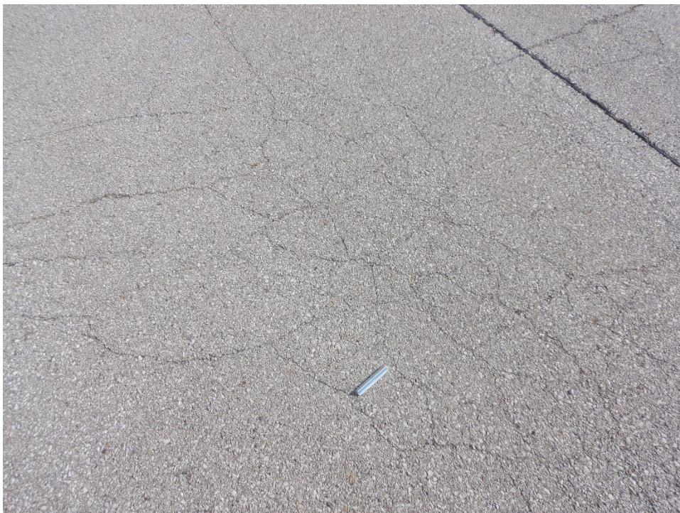
A01AL-01. Alligator Cracking (Sample Unit No. 05).
