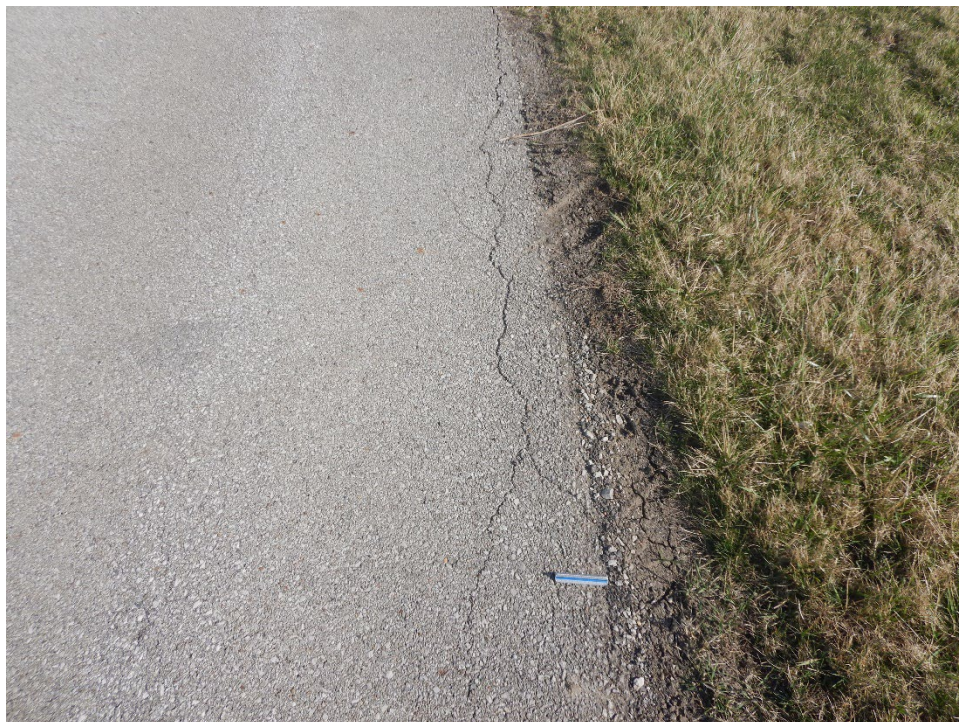
TH01AL-02. Alligator Cracking (Sample Unit No. 01).
