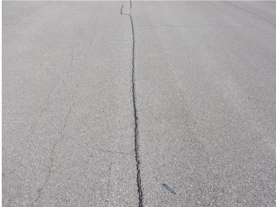
A01AL-01. L&T Cracking (Sample Unit No. 05).
