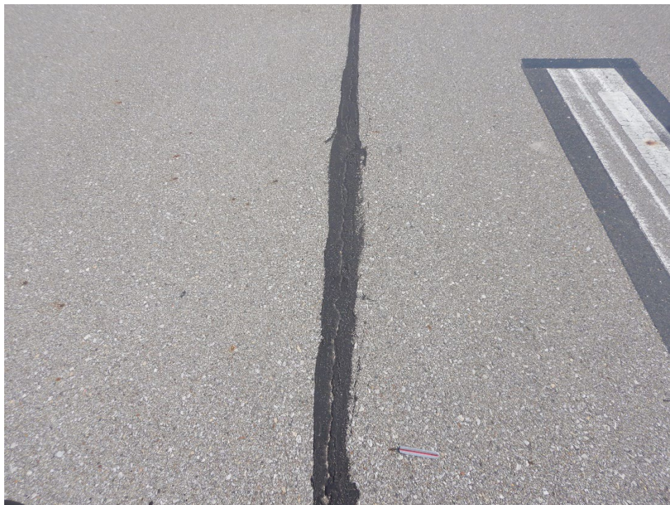
R13AL-01. L&T Cracking (Sample Unit No. 025).
