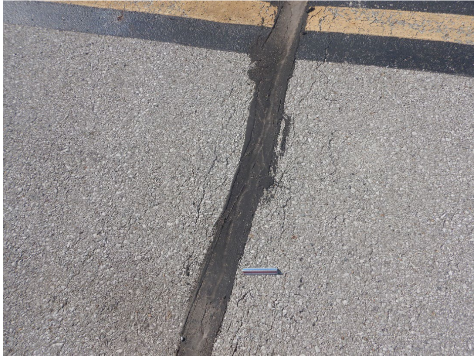
T01AL-01. L&T Cracking (Sample Unit No. 01) (1).
