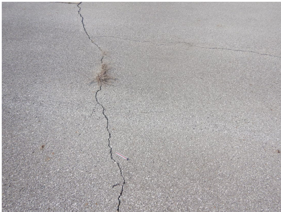
A01AL-02. L&T Cracking (Sample Unit No. 03).
