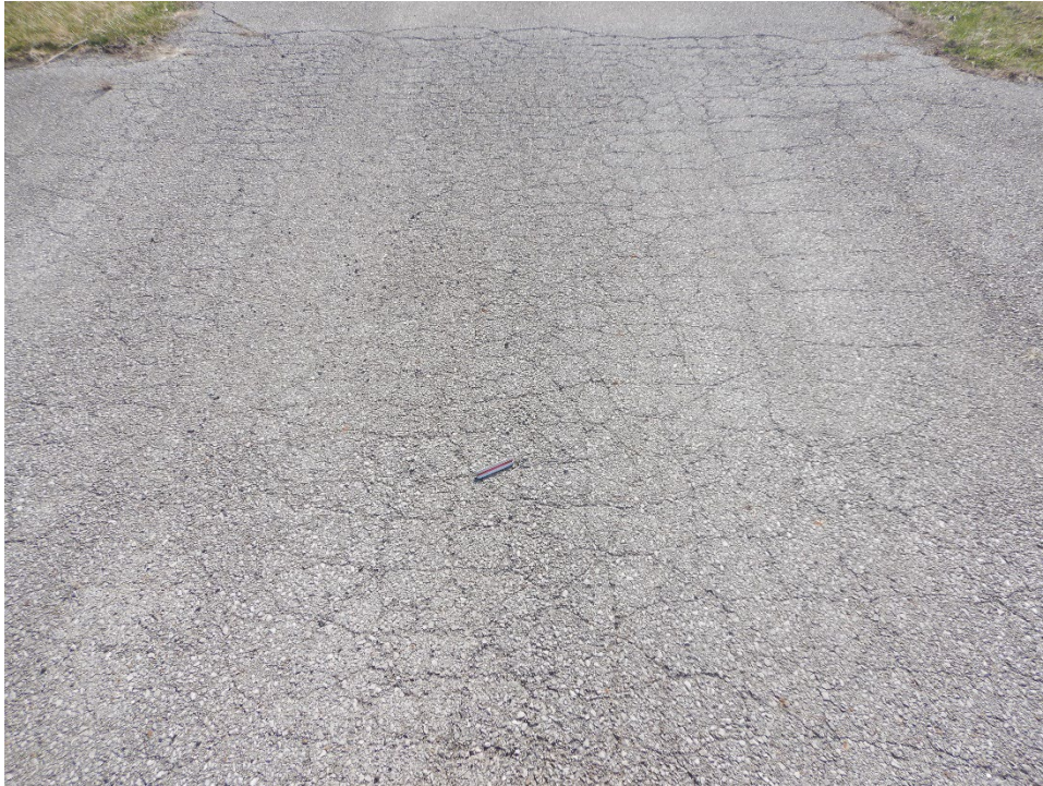
TH01AL-01. Alligator Cracking (Sample Unit No. 01).
